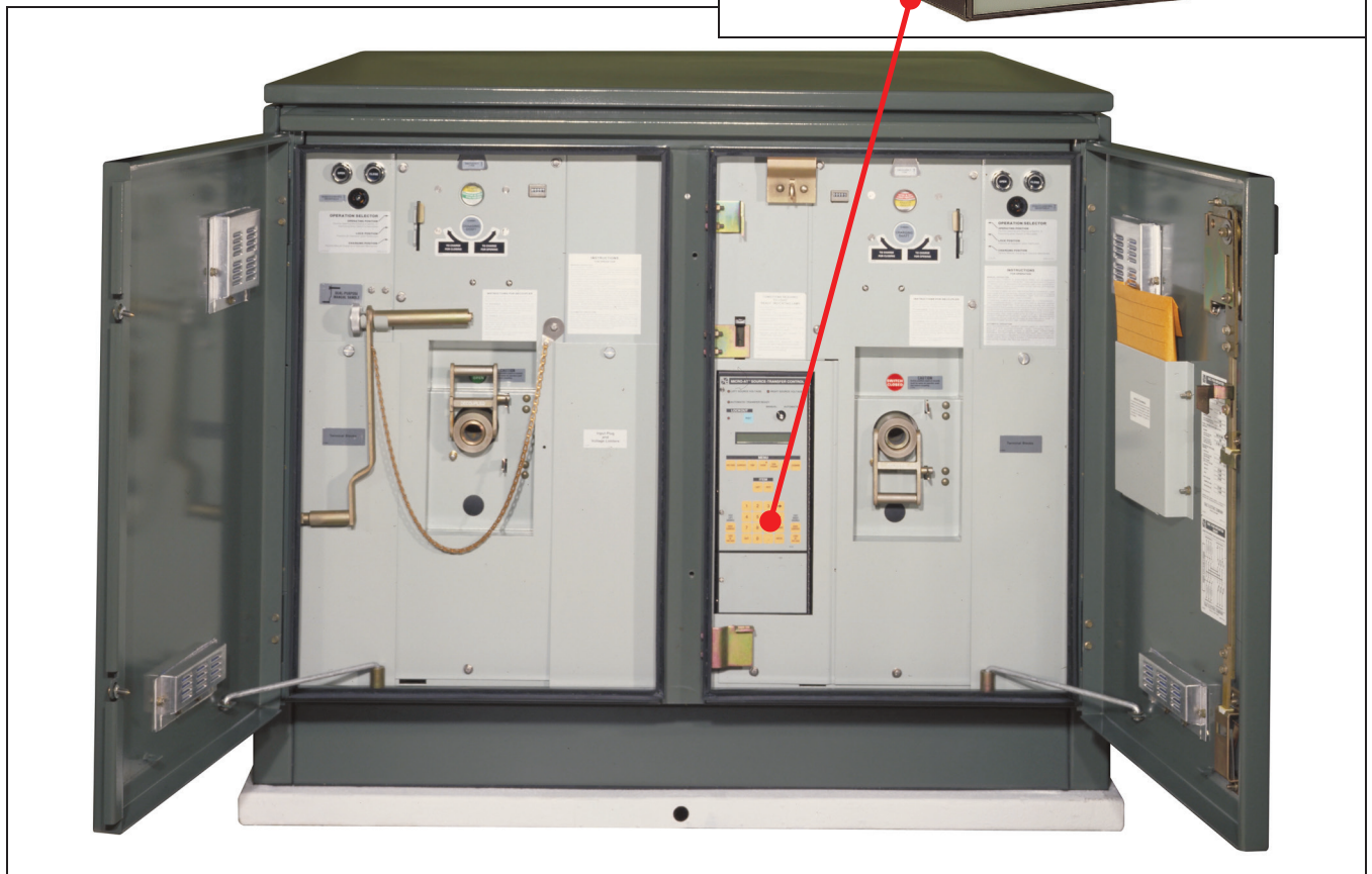
Figure 1. Micro-AT control installed in the S&C Source-Transfer Pad-Mounted Gear.
