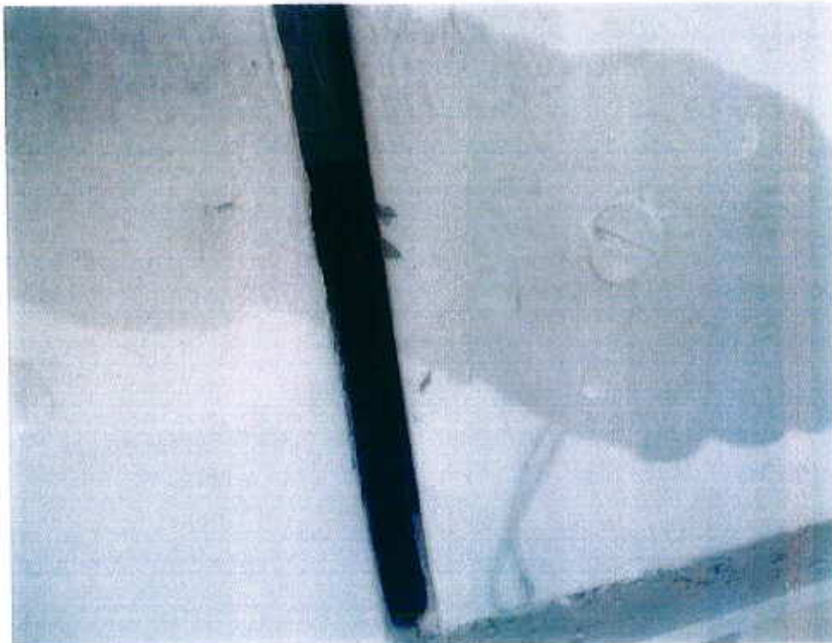
Description: Open Joint in metal
