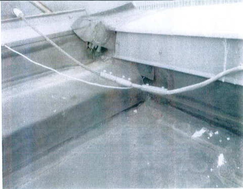
Description: Inadequate flashing detail
