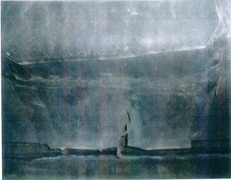
Description: Split in flashing
