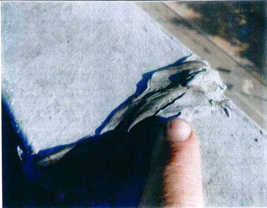
Description: Split sealant
