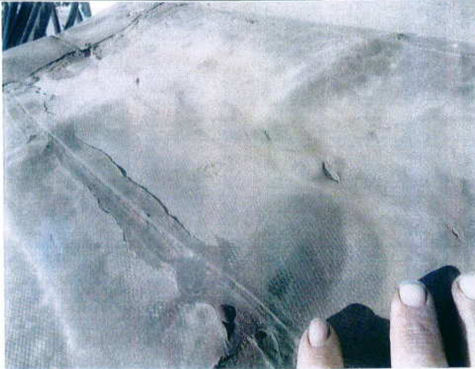
Description: Failed Coverstrip
