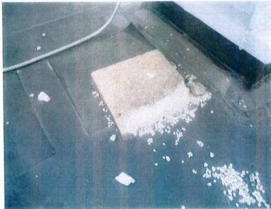
Description: Deteriorated Pavers
