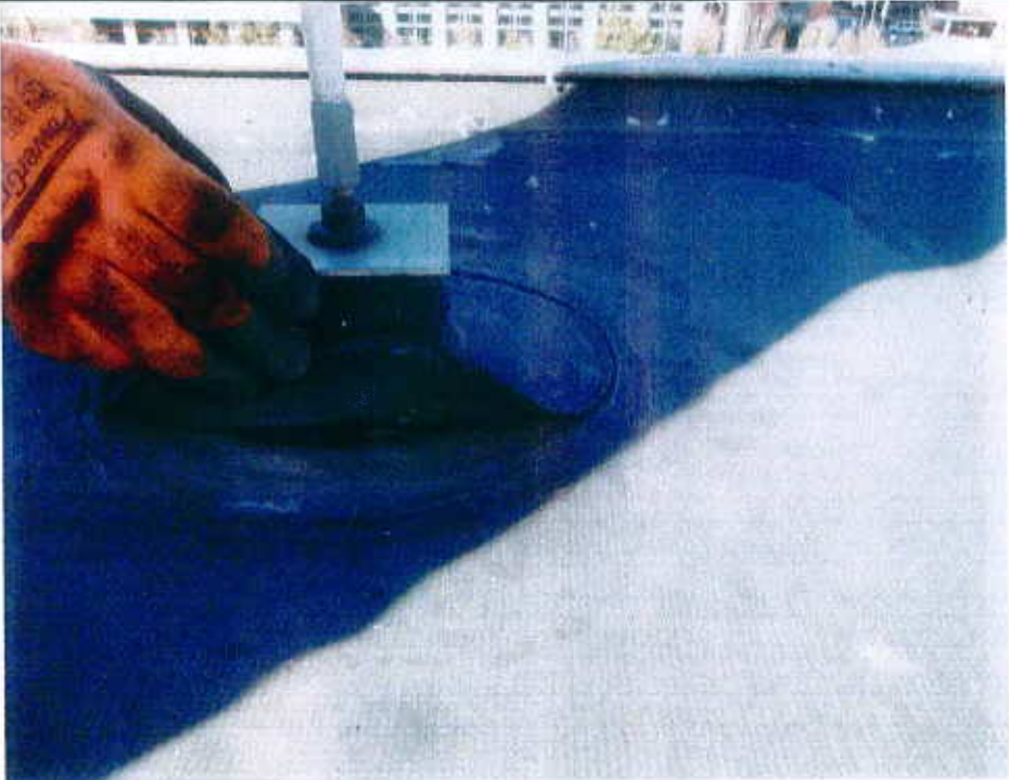
Description: Curling and brittle edges
