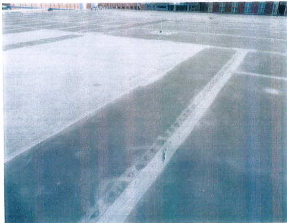
Description: Previous Repairs
