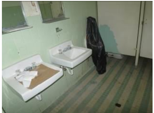
Non-Working Sink & Urinal
