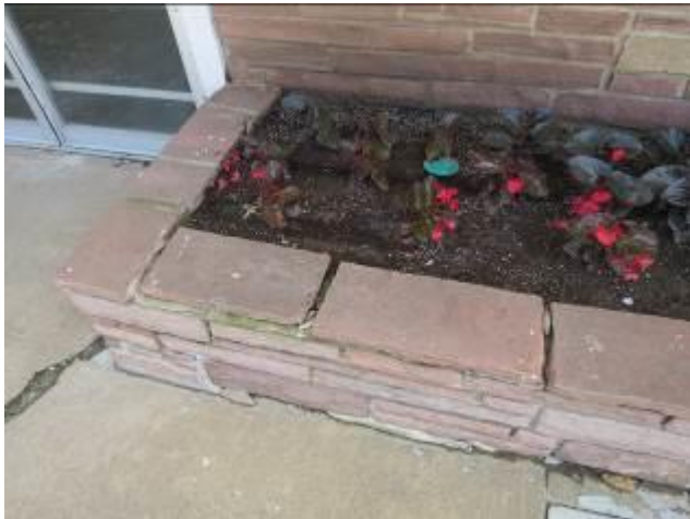
Deteriorated Sidewalk Landscaping Planter
