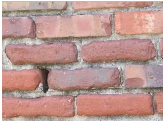
Wall Cracks – Vacant Building
