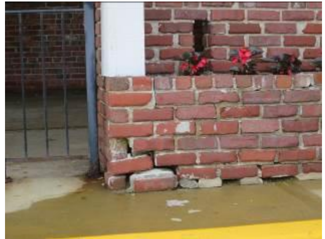
Deteriorated Sidewalk Landscaping Planter
