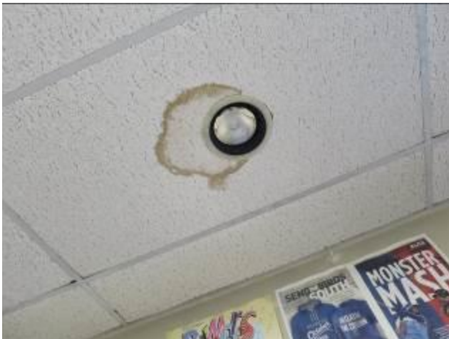
Ceiling Damage In Small Shops
