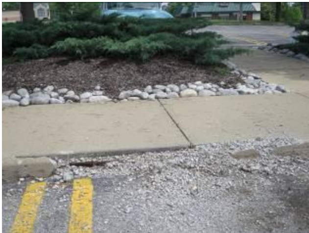
Deteriorated Curbing North Side Parking Lot
