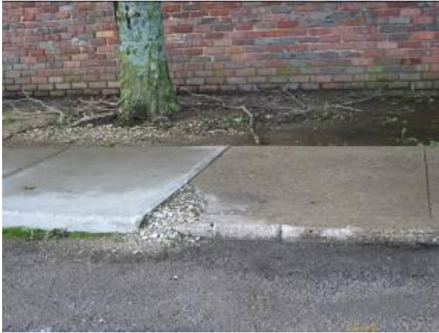
Deteriorated Sidewalk Grocery Store (N)
