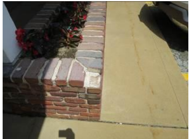
Damaged Sidewalk Landscaping Planter
