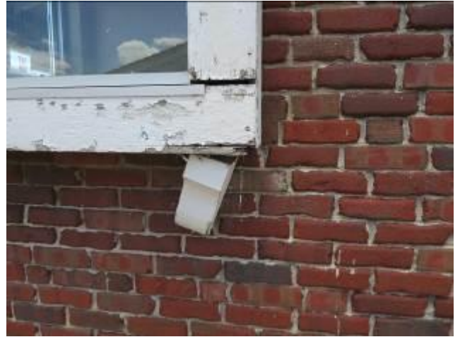
Broken Window Frame Support – Retail Strip
