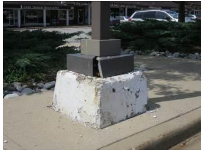
Deteriorated Parking Lot Lighting (N)
