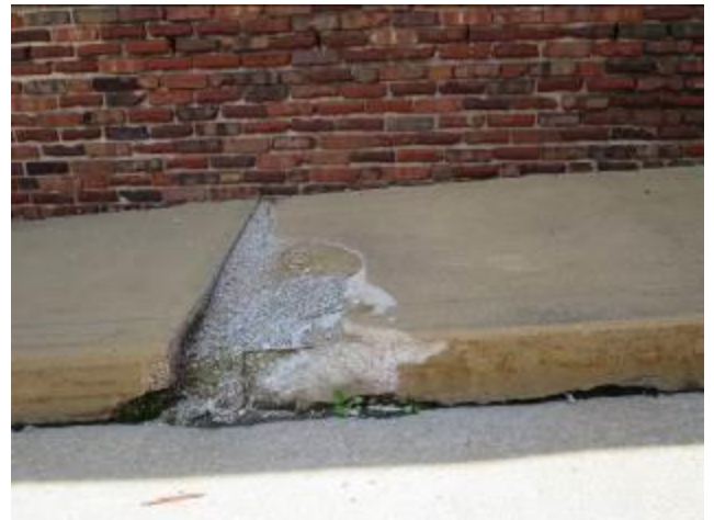
Deteriorated Sidewalk To Courtyard Dock
