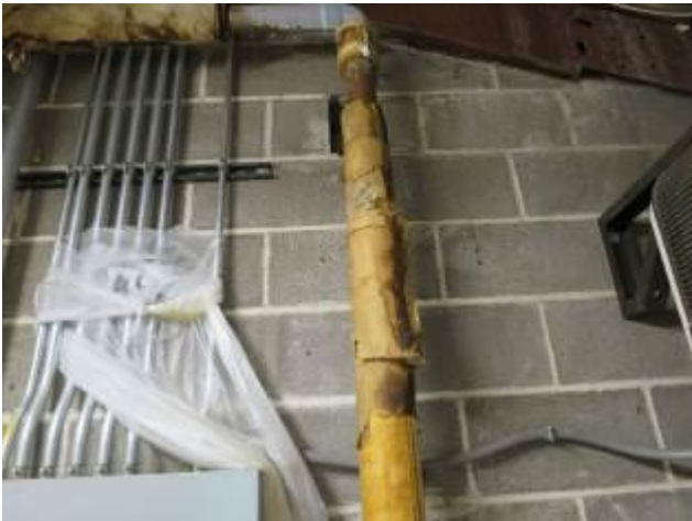
Compromised ACMs In Pipe Wrapping
