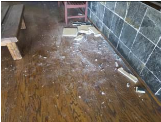
Ceiling Collapse In Vacant Restaurant
