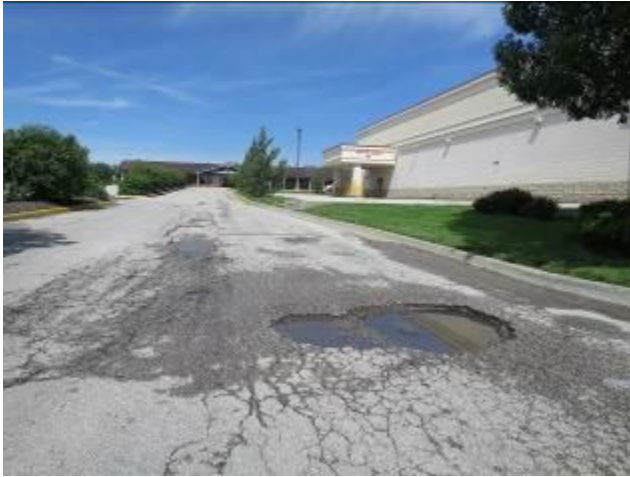
Damage At Holmes Road Central Entrance
