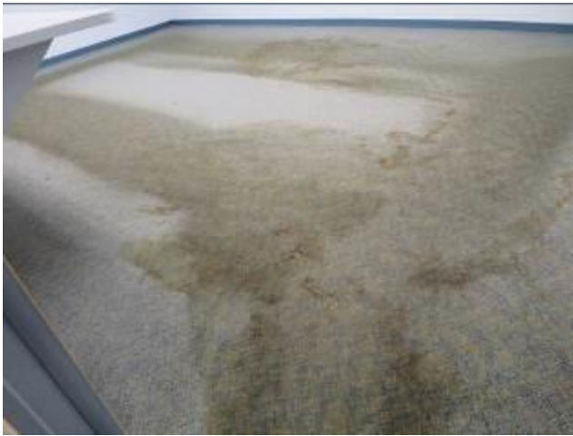
Mold In Walls & On Floors
