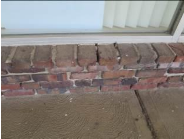
Wall Deterioration – Retail Strip
