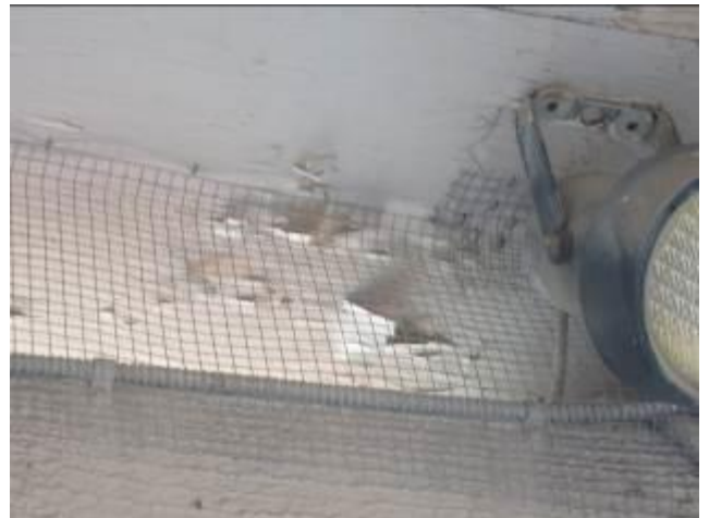
Deteriorating Grocer Entry Canopy
