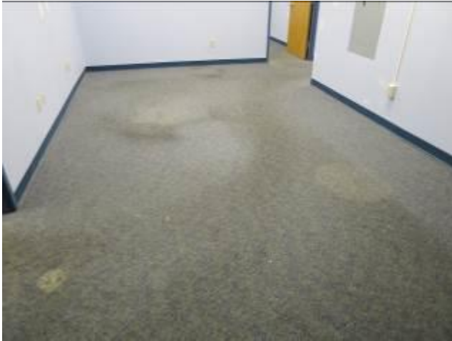
Damage & Mold In Carpets In Vacant Building
