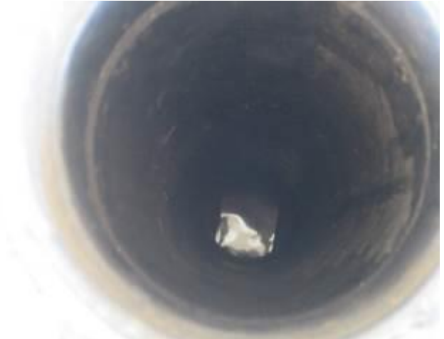
Unsecured Opening (6½" Diameter) In Sidewalk
