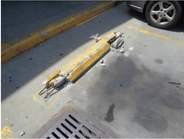
Exposed Rebar On Parking Block Grocery Store
