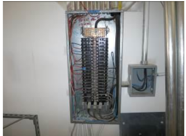
Obsolete Wiring In Small Shops
