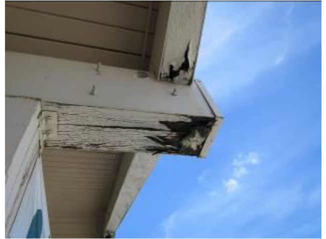
Rotted Canopy Beam – Vacant Building
