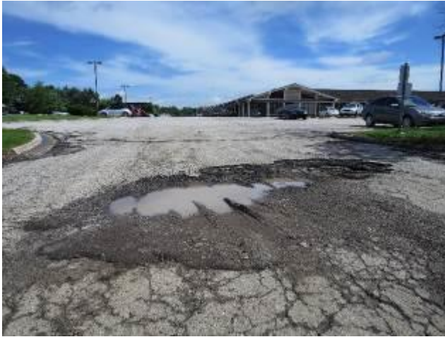
Parking Lot Damage
