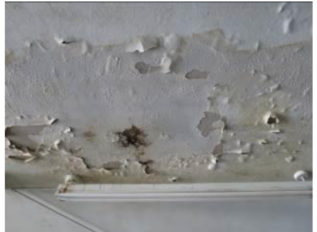
Ceiling Damage In Small Shops
