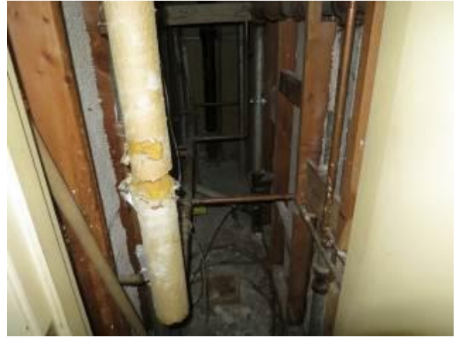
Compromised ACMs In Pipe Wrapping
