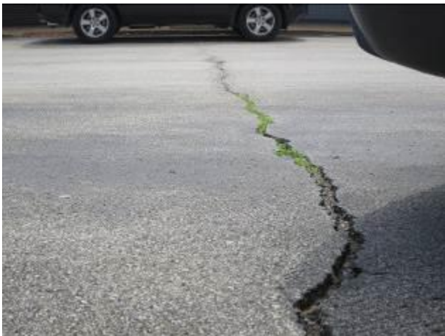
Deteriorated Parking Lot Between Vacant & Strip
