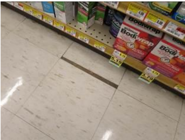
Damage Tile In Grocery
