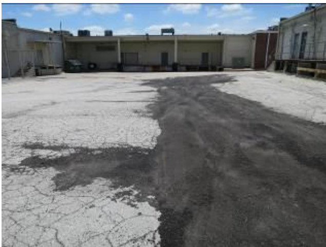
Deteriorating Asphalt Paving
