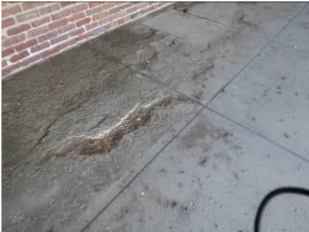
Deteriorated Sidewalk Grocery Store
