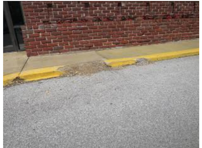
Deteriorated Curbing Retail Strip Building (E)
