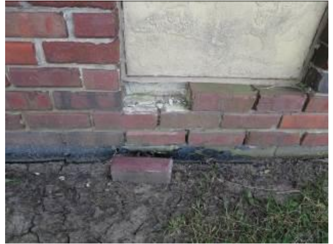
Wall Damage – Grocery Store
