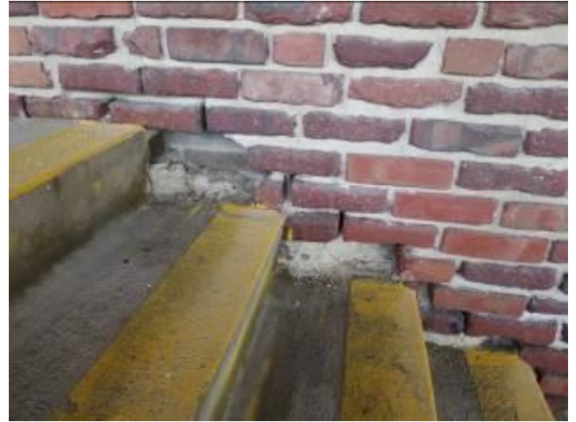
Wall Damage – Retail Strip Building
