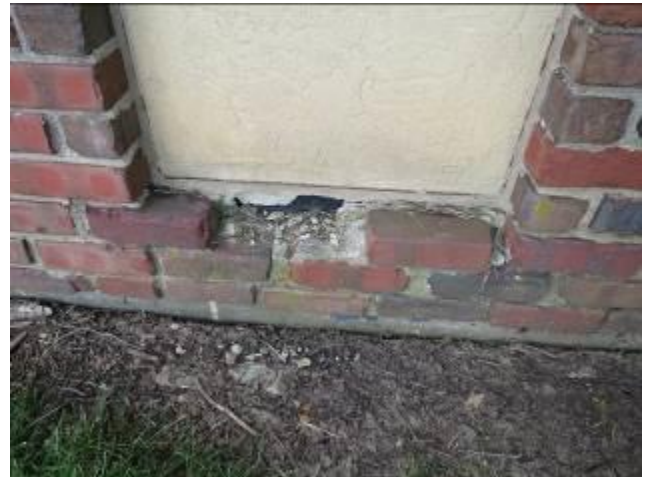
Wall Damage – Grocery Store
