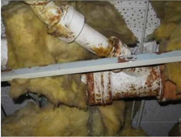
Aging Rusted Piping – Small Shops
