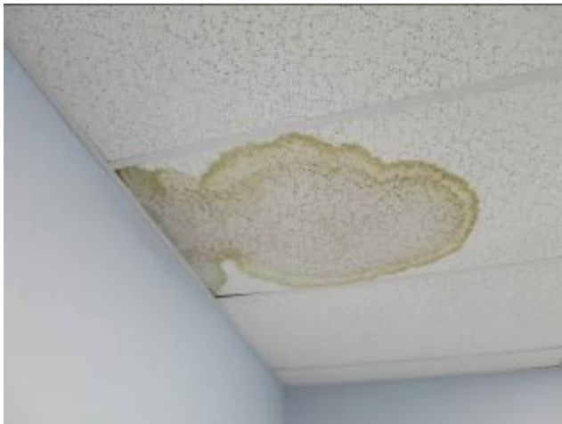
Ceiling Damage In Vacant Building
