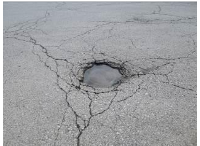
Deteriorated Central Parking Lot
