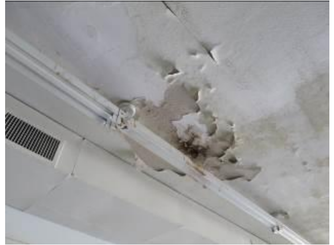
Ceiling Damage In Small Shops
