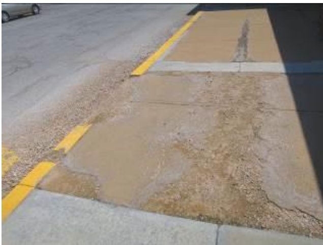
Deteriorated Sidewalk Retail Strip Building (E)
