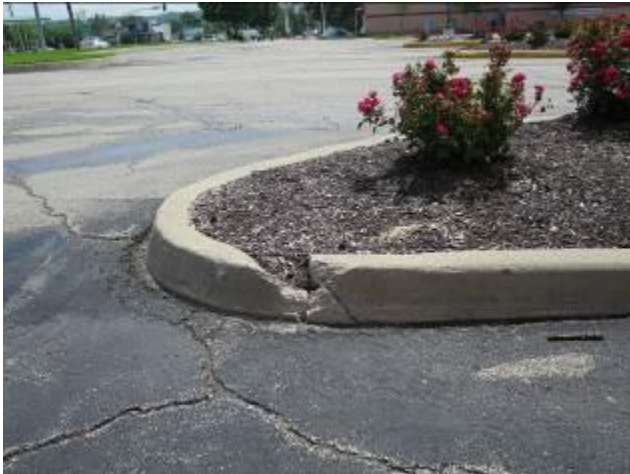
Deteriorated Landscape Planter Central Parking Lot
