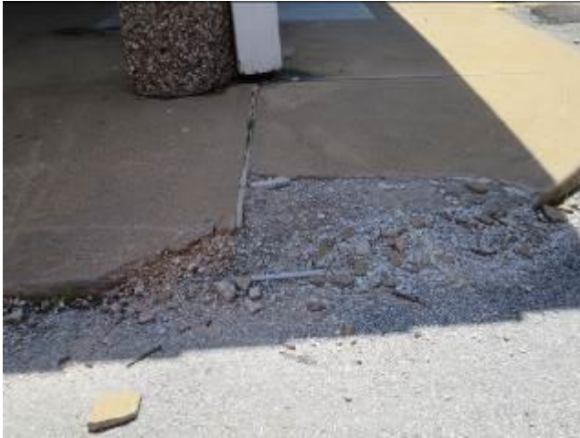
Deteriorated Sidewalk Retail Strip Building (SE)
