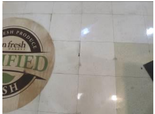
Damage Tile In Grocery
