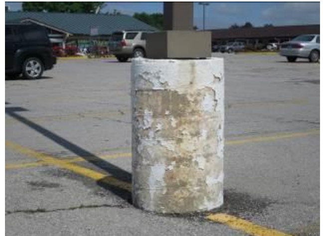
Deteriorated Parking Lot Lighting (SEC)
