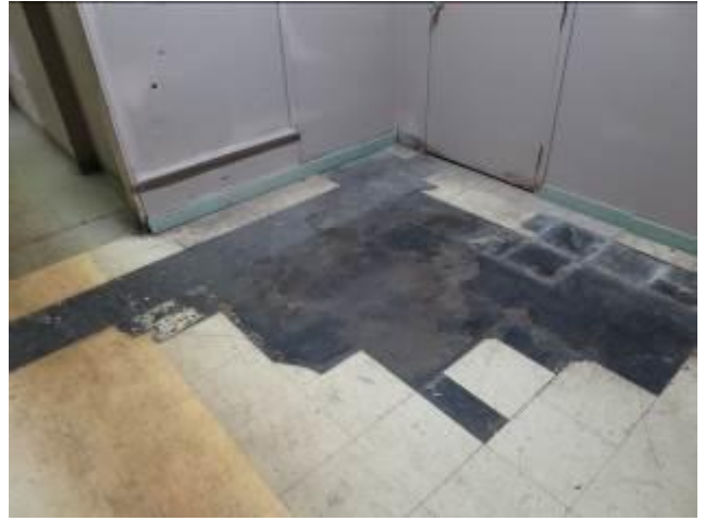
Damaged Floors In Small Shops
