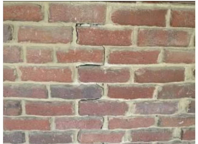
Wall Cracks – Retail Strip Building
