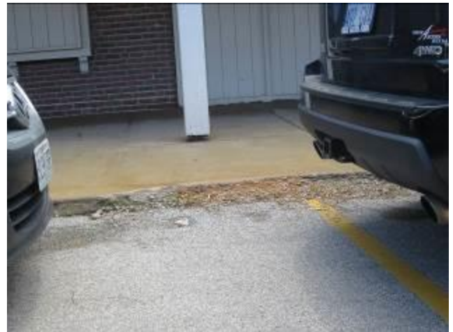
Deteriorated Curbing Retail Strip Building (W)
