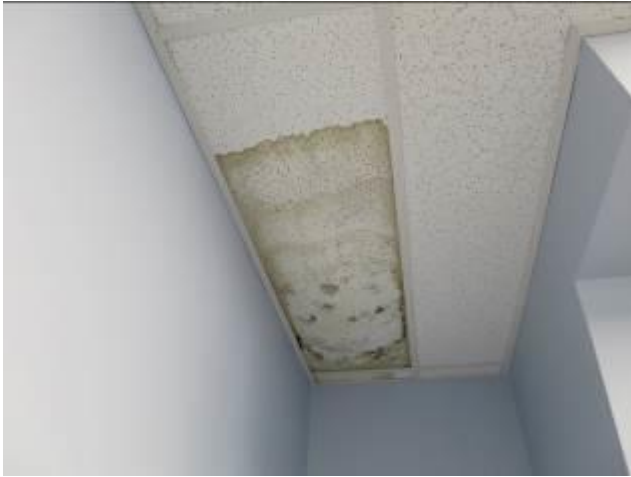
Ceiling Damage In Vacant Building
