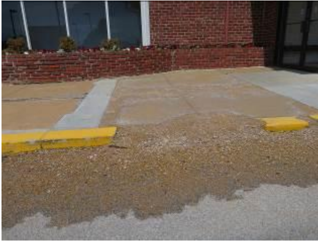
Deteriorated Sidewalk Retail Strip Building (E)
