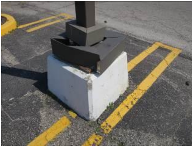
Deteriorated Parking Lot Lighting (SWC)
