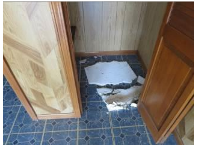
Ceiling Collapse In Vacant Small Shop
