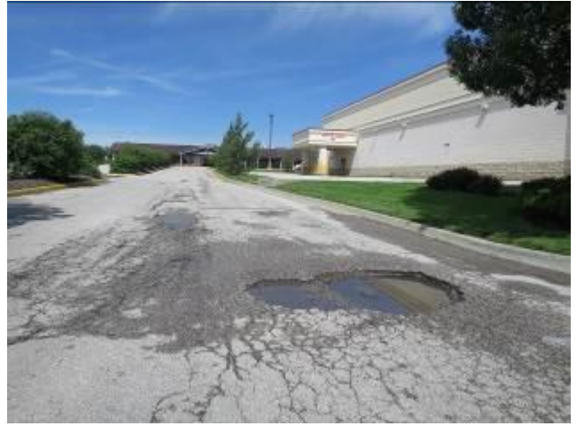
Entrance Damage & Pothole
