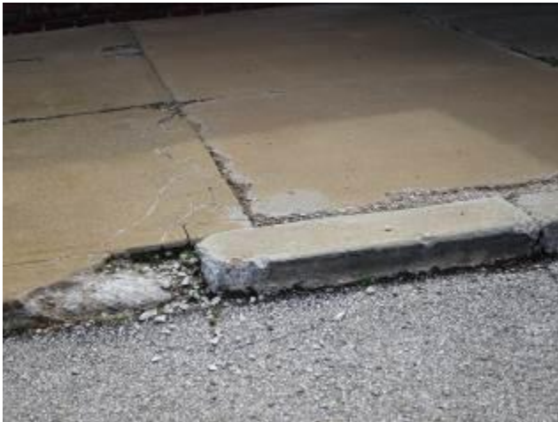
Deteriorated Curbing Retail Strip Building
