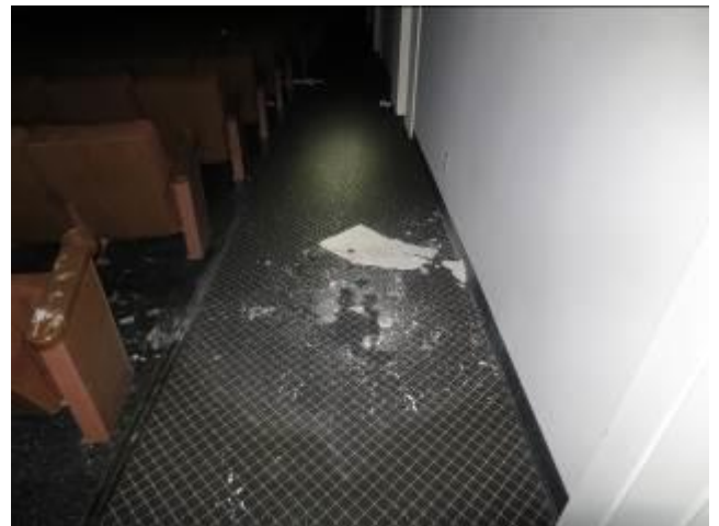
Ceiling Collapse In Former Theater
