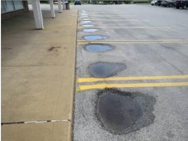
Deteriorated Parking Along Strip Building
