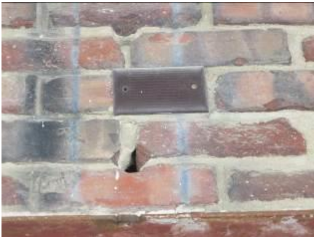
Wall Damage – Retail Strip Building
