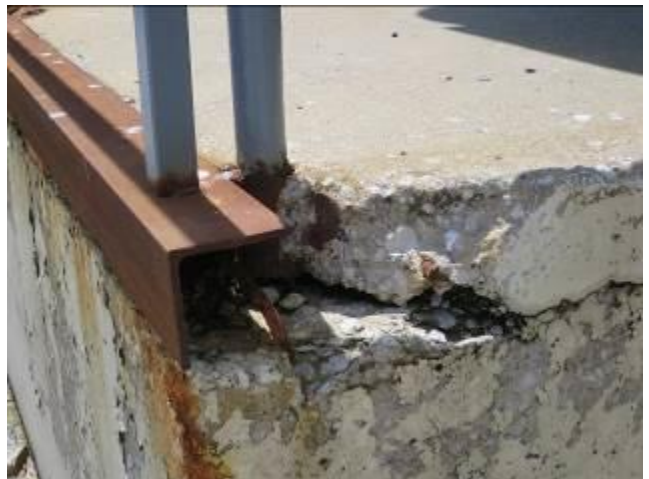
Deteriorating Dock & Railing
