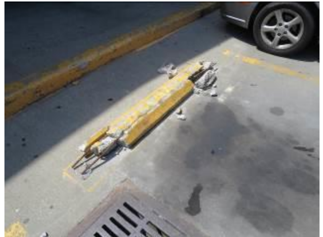
Deteriorated Parking Block At Grocer
