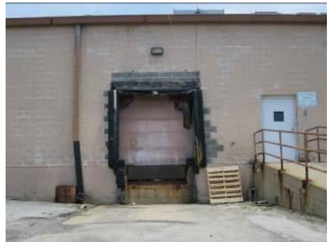
Deteriorating & Unsightly Dock At Grocery Store
