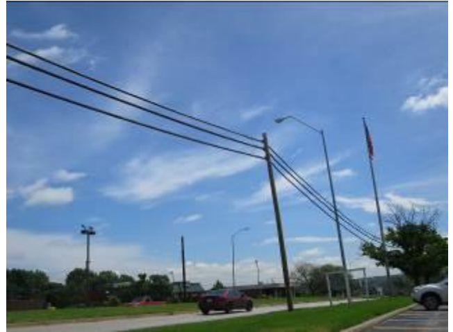
Unsightly Overhead Power Lines On Red Bridge Rd.
