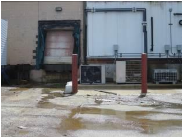
Deteriorating & Unsightly Dock Area – Grocer
