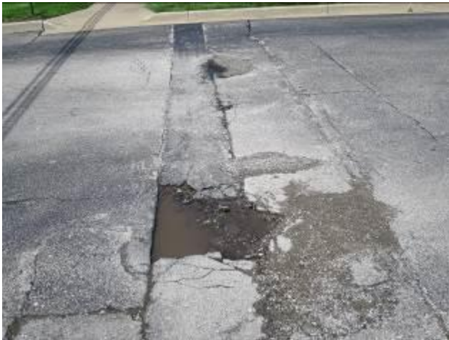
Deteriorated NWC Parking Lot
