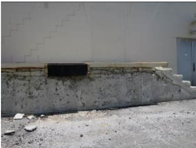
Deteriorating Dock & Wall Cracks
