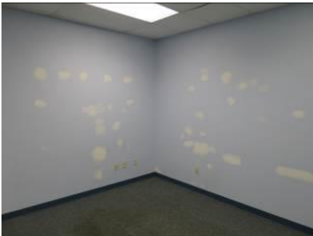
Unsightly Walls In Vacant Building
