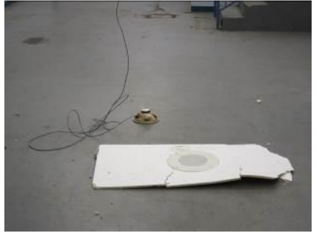
Ceiling Damage In Vacant Building
