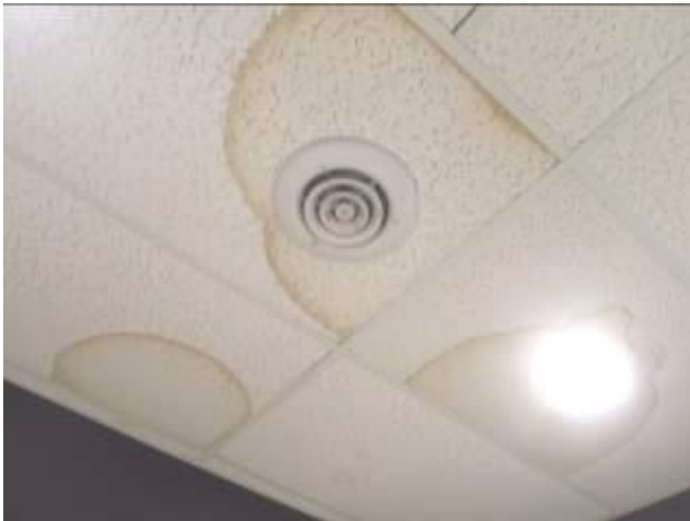
Ceiling Damage In Small Shops
