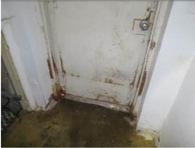
Rusting Interior Door – Retail Strip
