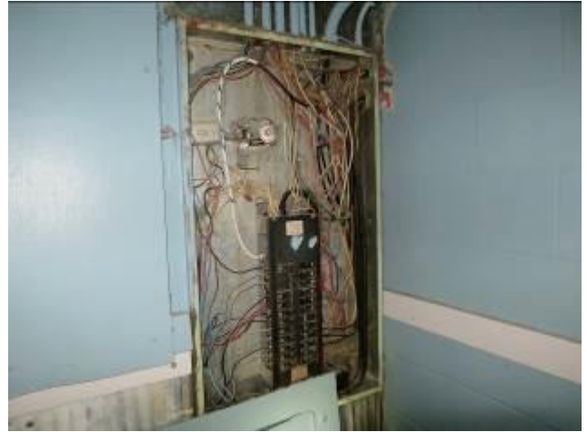
Obsolete Wiring – Small Shops
