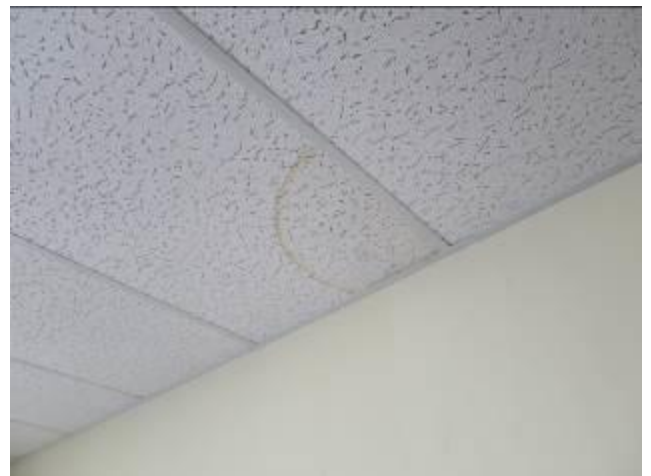
Ceiling Damage In Small Shops
