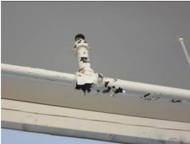
Deteriorating Fire Sprinklers – Vacant Building
