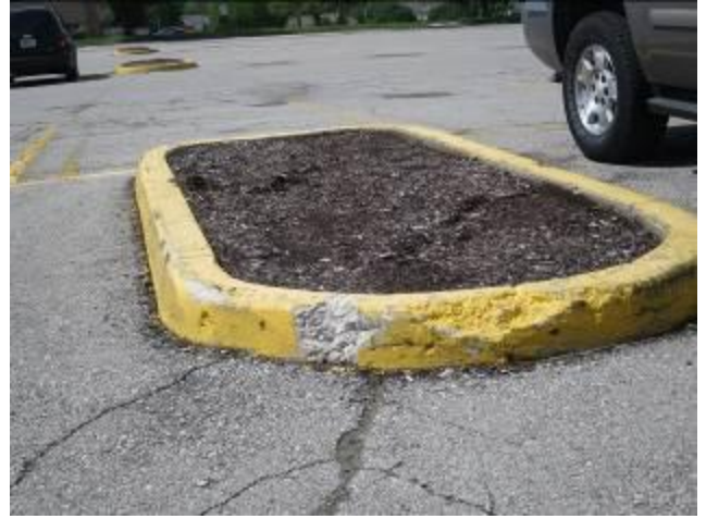
Deteriorated Landscape Planter SEC Parking Lot
