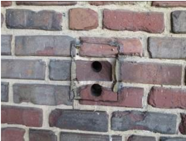
Wall Damage – Retail Strip Building
