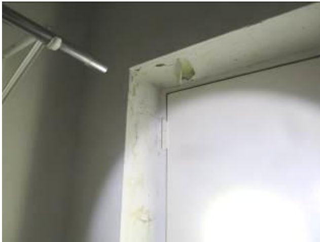
Wall Damage In Small Shops
