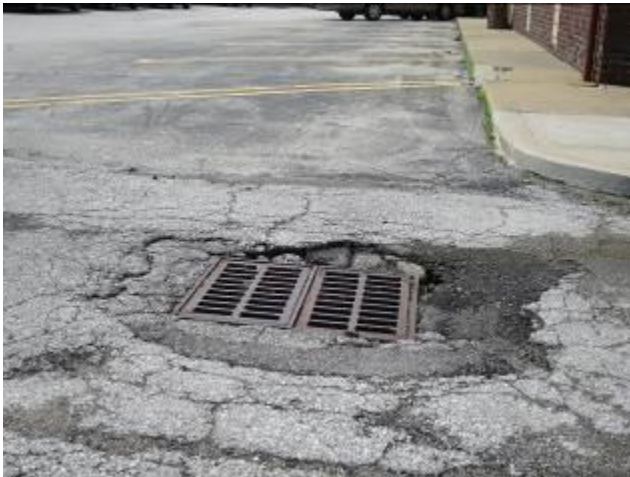
Deteriorated Central Parking Lot
