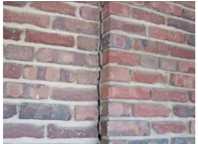
Wall Cracks – Retail Strip Building
