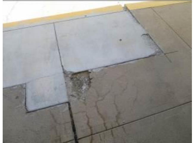
Deteriorated Sidewalk Retail Strip Building (S)
