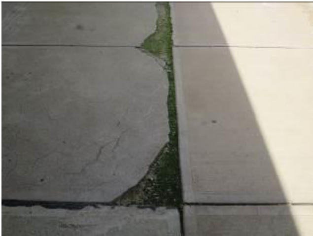
Deteriorated Sidewalk Retail Strip Building (N)
