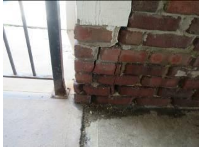
Deteriorated Sidewalk Landscaping Planter/Support
