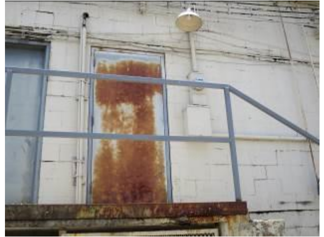
Rusting Exterior Door – Retail Strip
