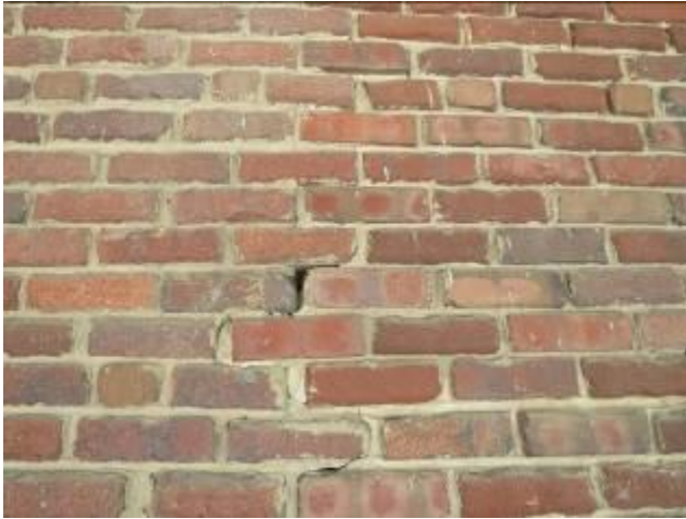
Wall Damage – Retail Strip Building
