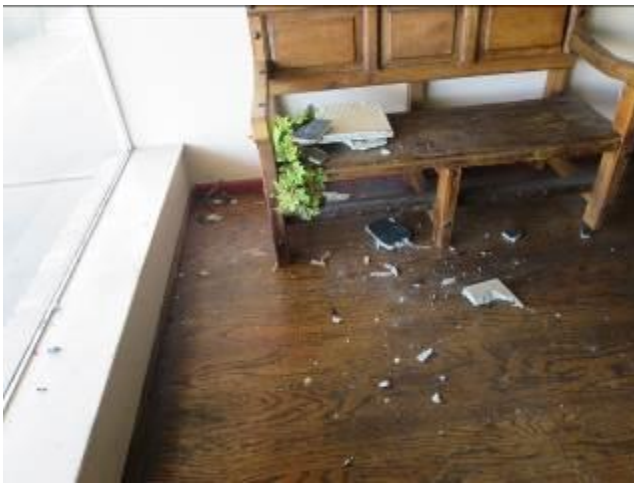
Ceiling Collapse In Vacant Restaurant
