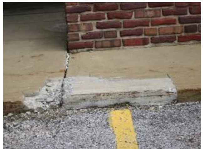
Deteriorated Sidewalk Retail Strip Building (W)
