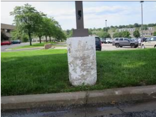
Deteriorated Parking Lot Lighting (SWC)
