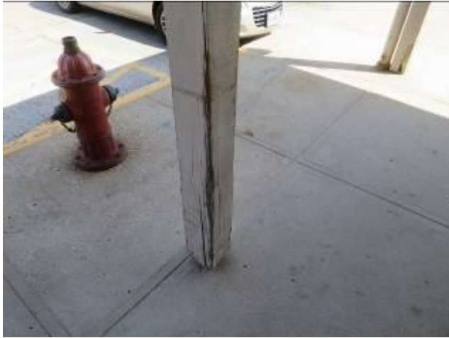
Deteriorating Canopy Support – Grocery Store
