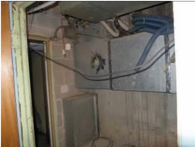
Wiring Hanging Below Door Opening (Small Shops)
