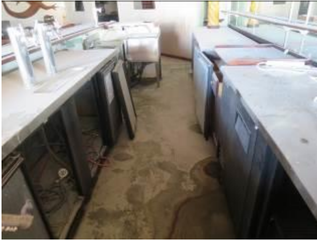
Deteriorated Floors In Small Shops
