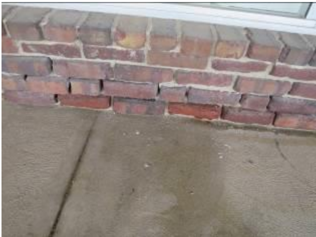
Wall Damage – Retail Strip Building
