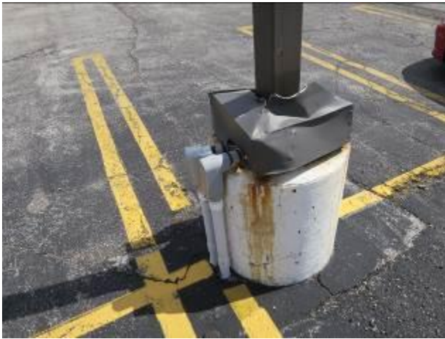
Deteriorated Parking Lot Lighting (SEC)
