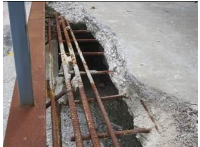
Rebar And Opening In Dock Tenant Had Partially Covered With Carpet
