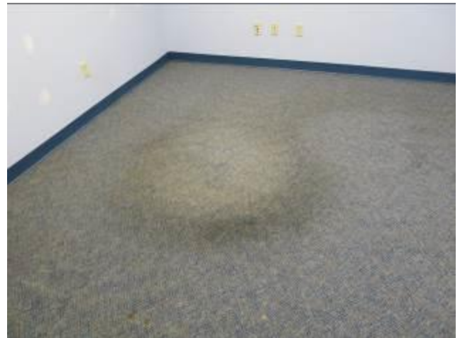
Damage & Mold In Carpets In Vacant Building
