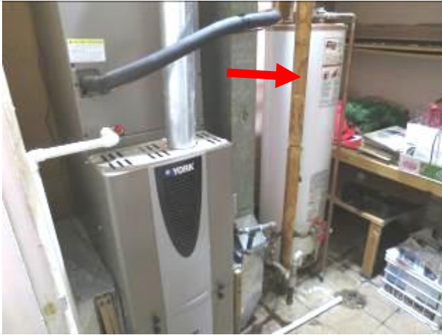
Compromised ACMs In Pipe Wrapping
