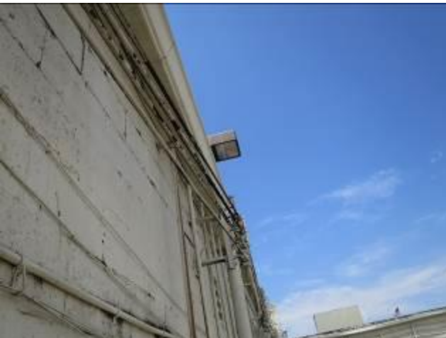
Hot/Exposed Wiring Surrounding Courtyard Dock
