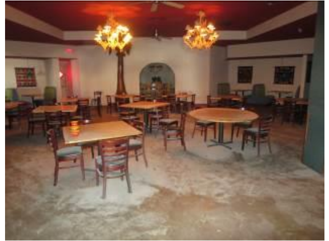
Deteriorated Floors In Small Shops
