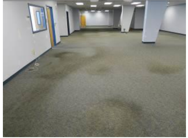
Damage & Mold In Carpets In Vacant Building
