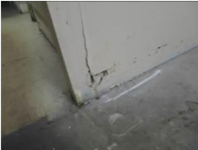
Wall Damage In Small Shops
