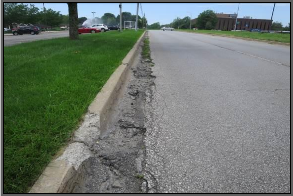
Deteriorating Curbing & Pavement Drop (To Gutter) Along Eastbound Lane of Red Bridge Road
