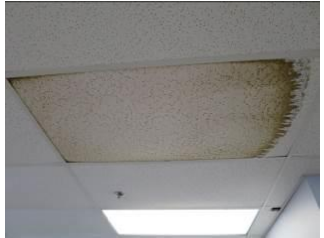
Ceiling Damage In Vacant Building
