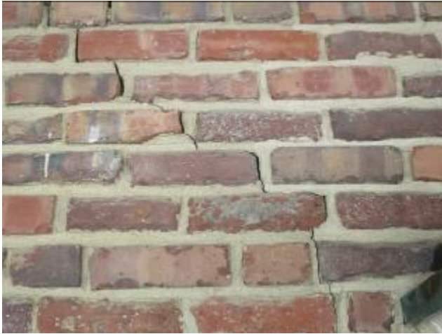
Wall Cracks – Retail Strip Building
