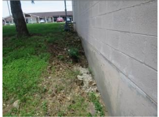
Erosion Around Foundation Of Grocery Store
