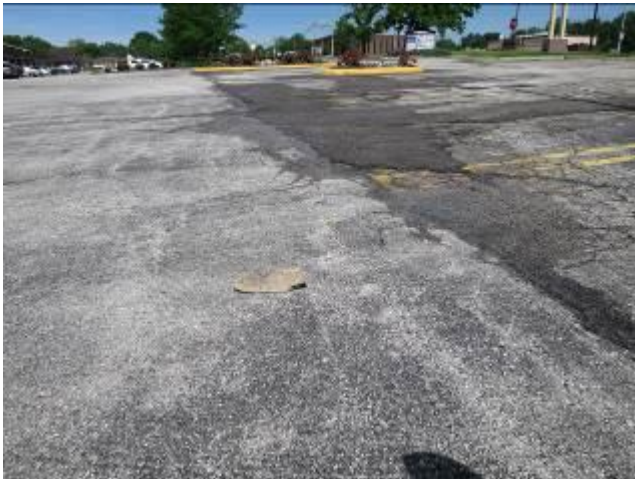
Deteriorated East-Central Parking Lot
