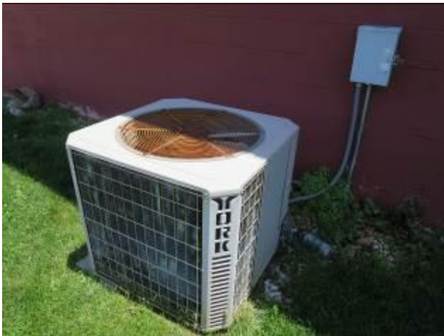
Aging HVAC – Vacant Building
