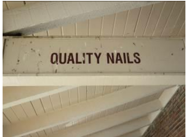
Poor Space Signage – Retail Strip
