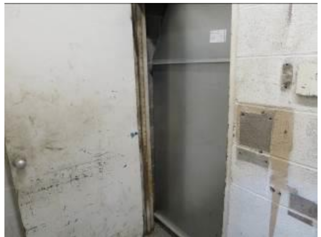
Poor Access To Air Handling Units (Vacant Bldg.)
