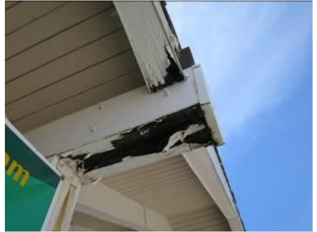
Rotted & Deteriorating Canopy – Vacant Building
