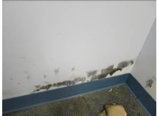
Wall Damage/Mold In Vacant Building
