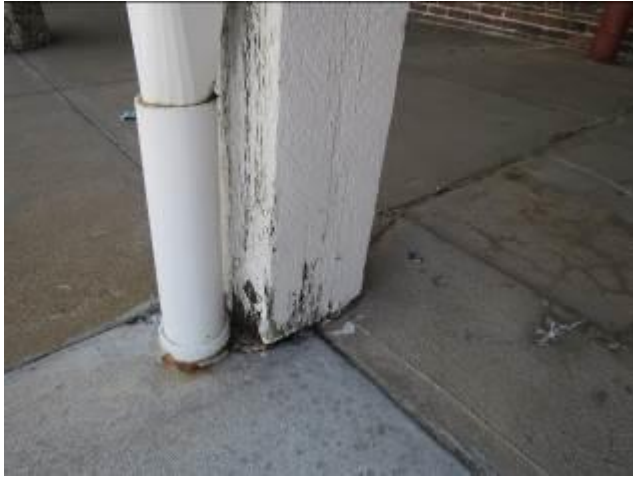
Deteriorating Canopy Support – Retail Strip
