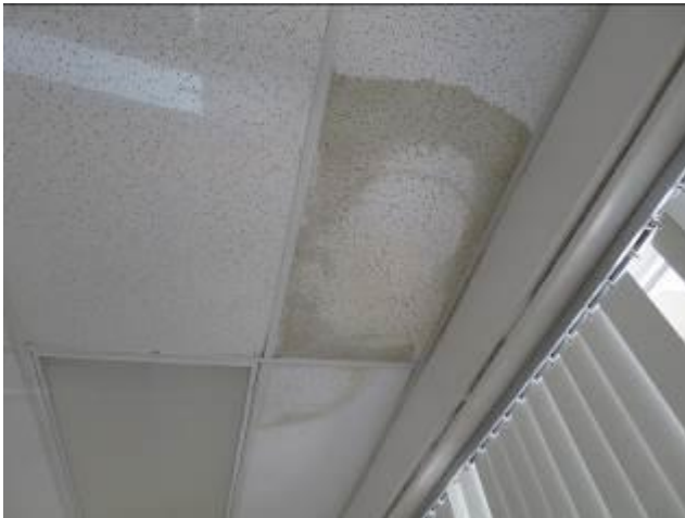
Ceiling Damage In Small Shops
