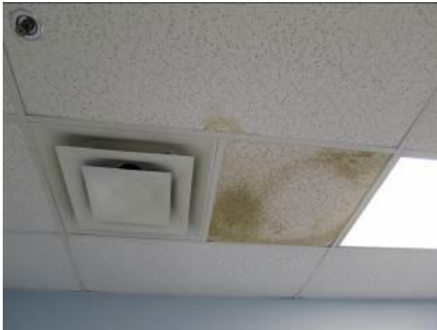
Ceiling Damage In Vacant Building
