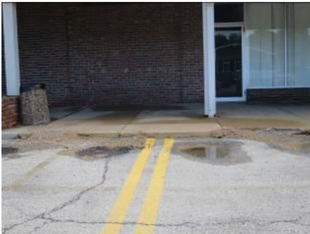
Deteriorated Curbing Vacant Building
