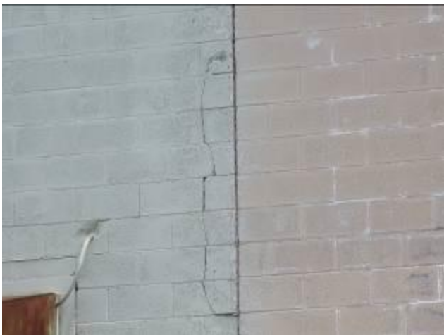
Wall Crack – Grocery Store
