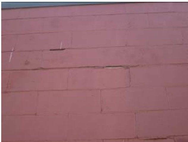
Wall Cracks – Vacant Building
