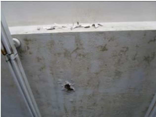
Ceiling Damage In Small Shops
