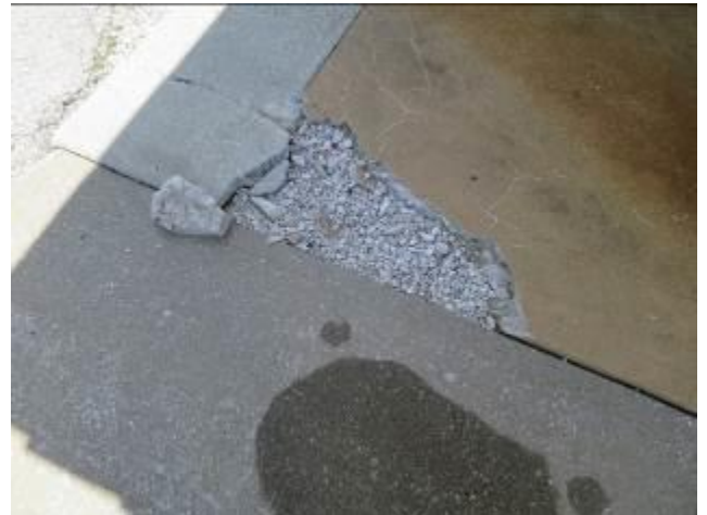
Deteriorated Sidewalk Retail Strip Building (N)
