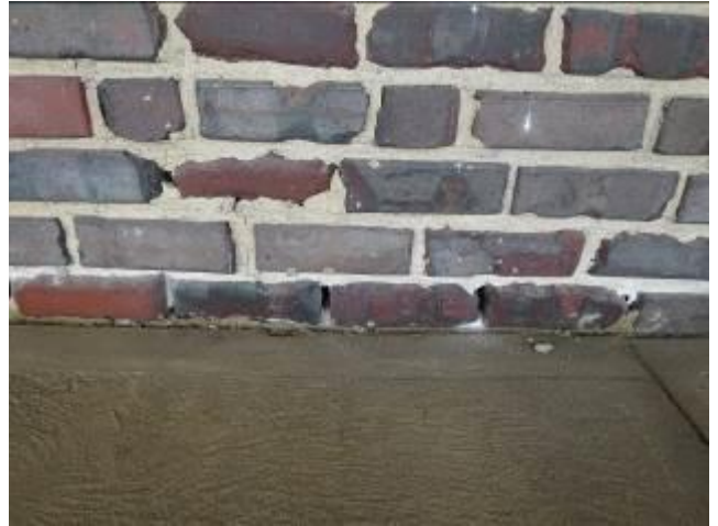
Wall Damage – Retail Strip Building
