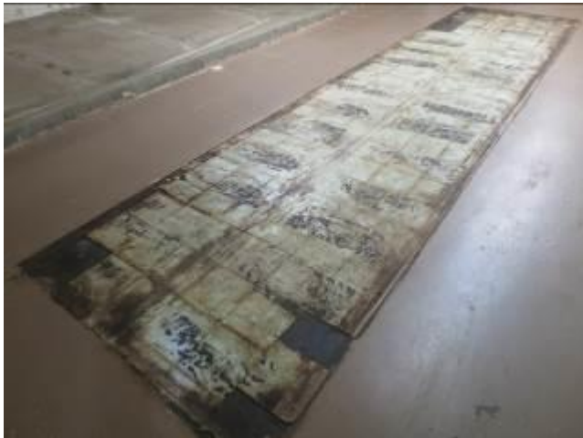
Damaged Floors In Small Shops
