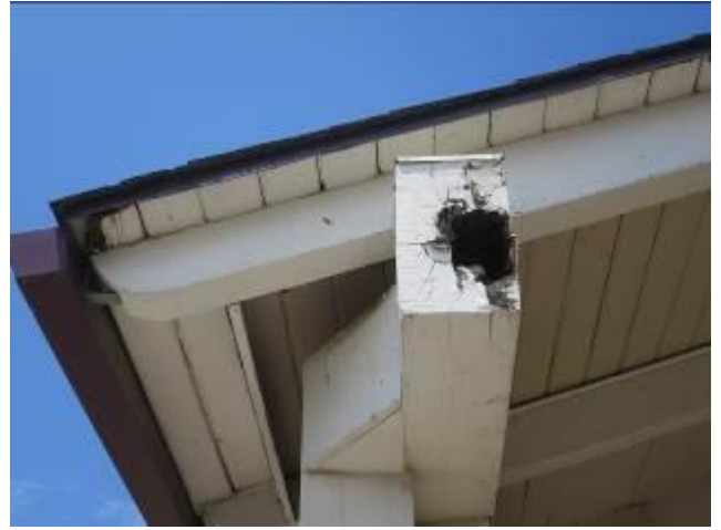
Deteriorating & Rotted Canopy Beam – Retail Strip
