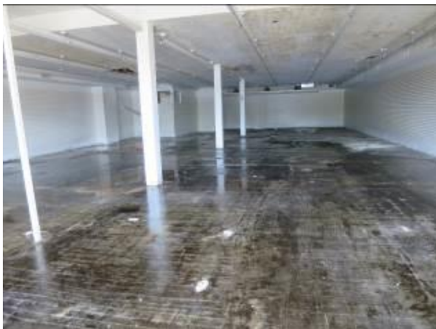
Water Infiltration In Vacant Small Shop
