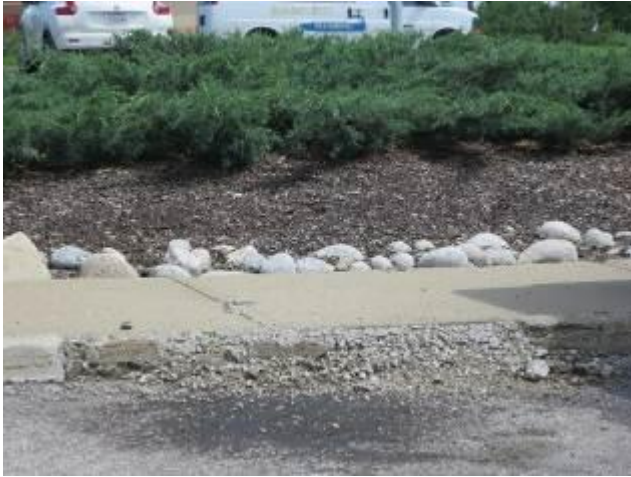
Deteriorated Curbing North-Central Parking Lot
