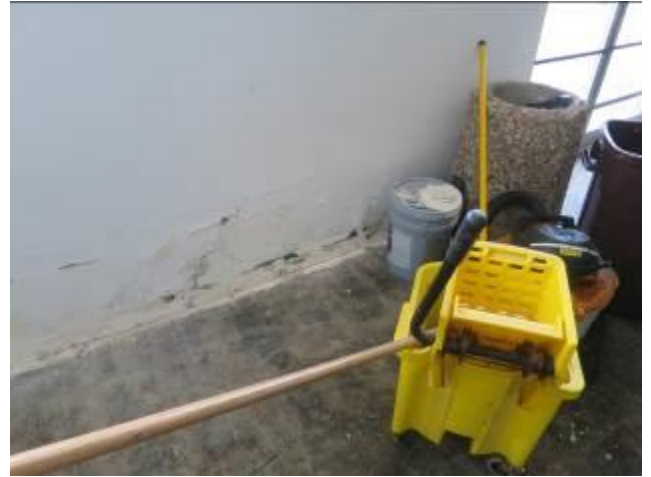
Wall Damage/Mold In Small Shops
