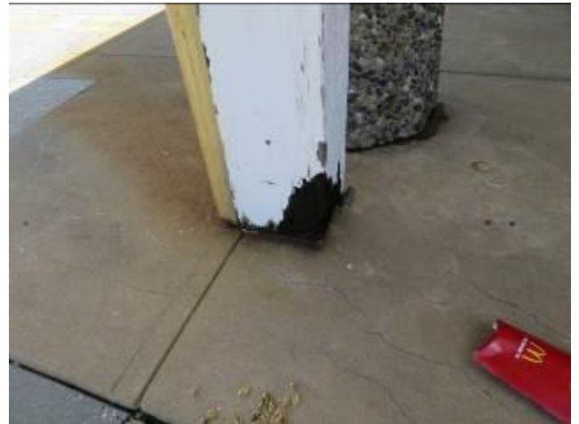
Rotted Canopy Support – Vacant Building
