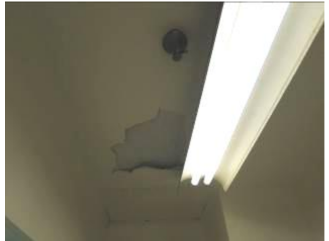
Ceiling Damage In Small Shops
