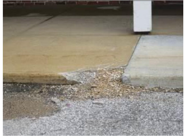
Deteriorated Curbing Retail Strip Building (S)
