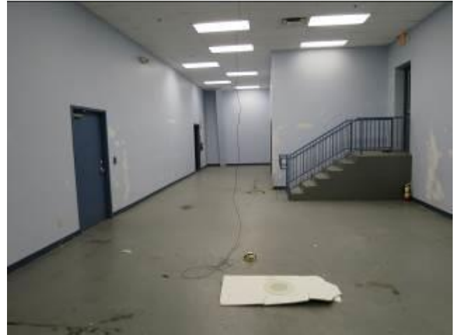
Ceiling Collapse In Vacant Building
