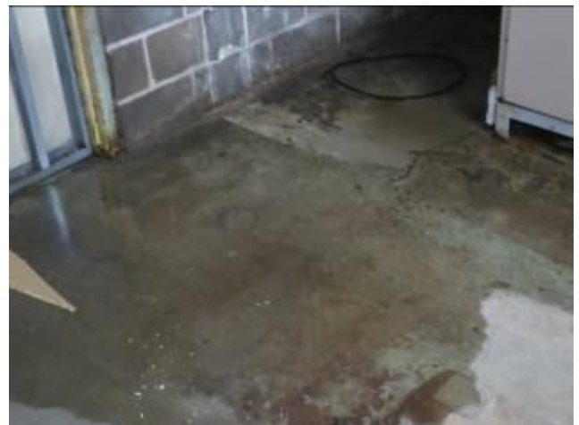
Water Infiltration In Vacant Building
