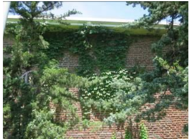
Vegetation On Wall – Vacant Building
