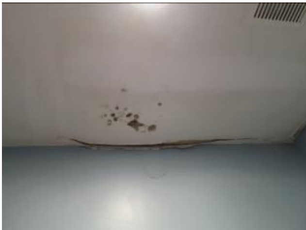
Mold In Water Damaged Ceiling
