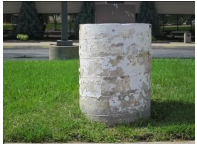
Deteriorated Parking Lot Lighting (S)
