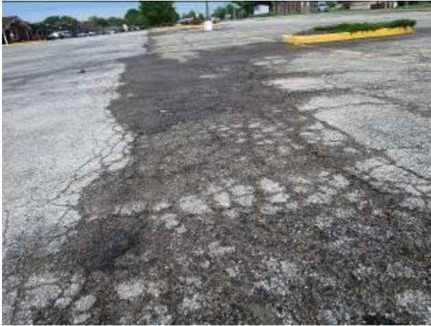
Deteriorated North-Central Parking Lot
