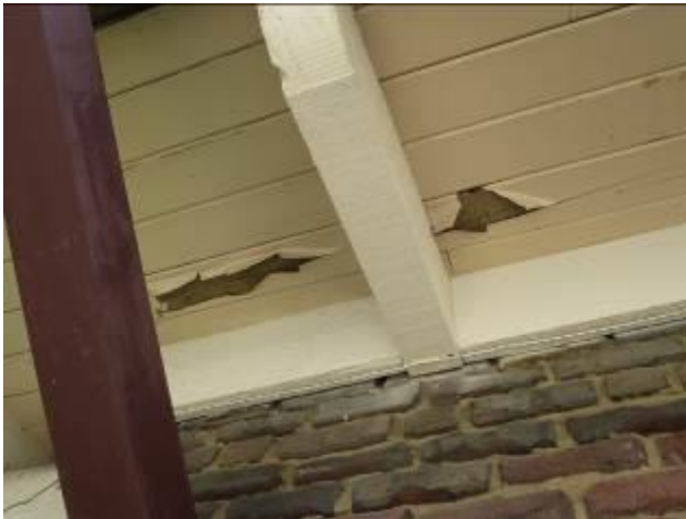
Deteriorating Canopy – Retail Strip
