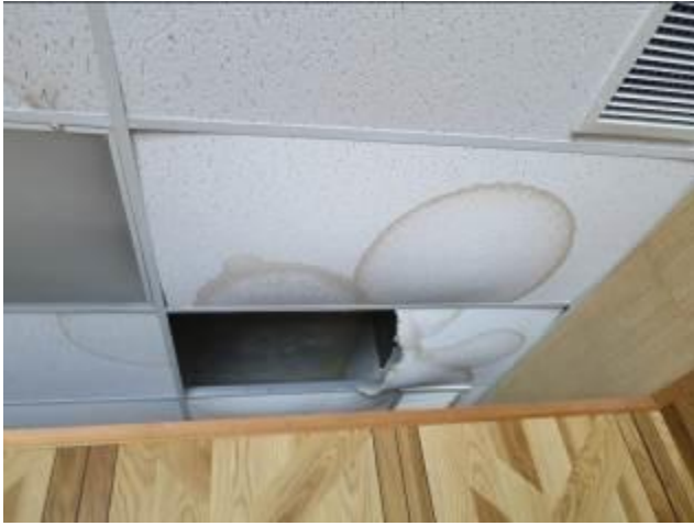
Ceiling Damage In Small Shops
