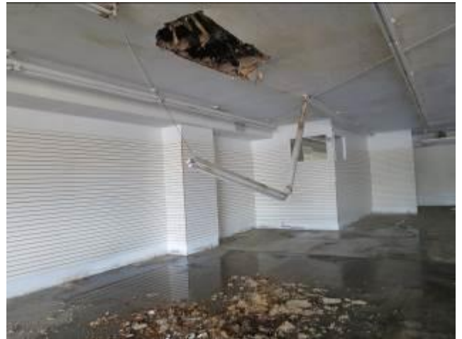
Ceiling Damage In Small Shops
