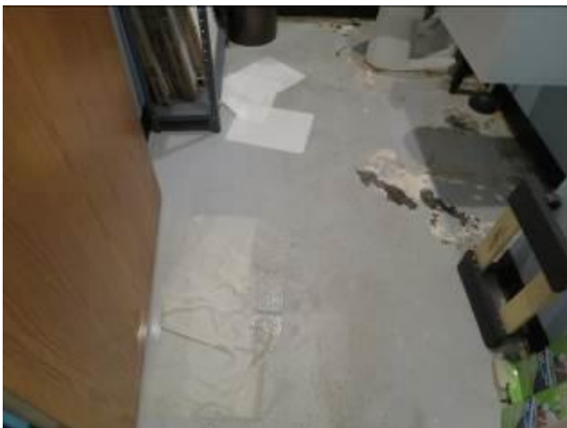
Wet Floors From Leaking Ceiling In Small Shops
