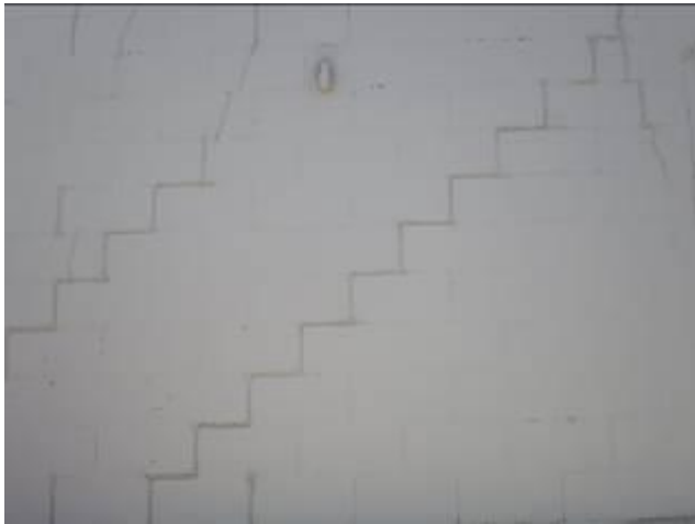
Wall Cracks – Courtyard Dock Area
