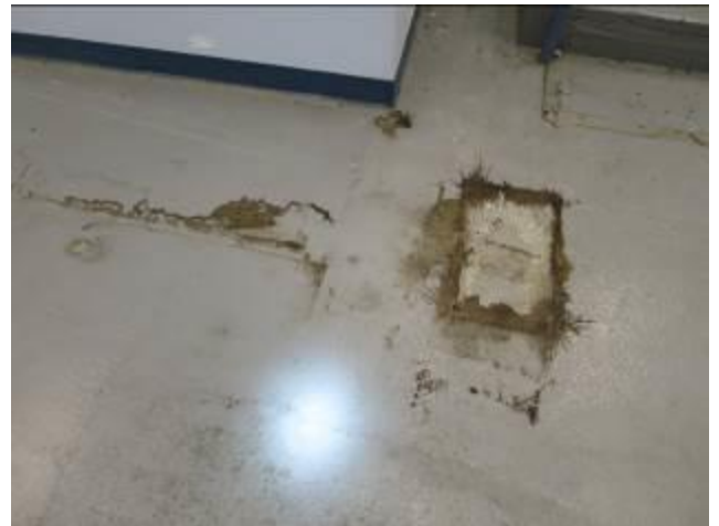
Deteriorated Floors In Small Shops
