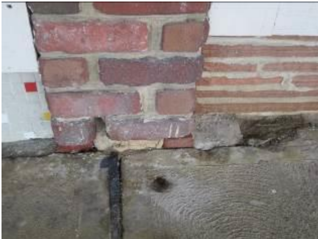
Wall Damage – Retail Strip Building
