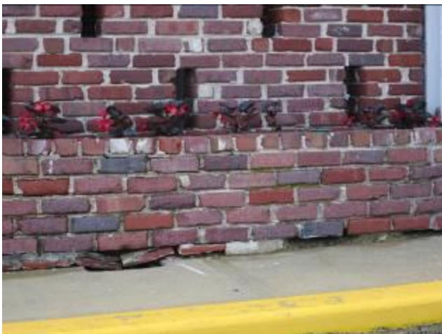
Deteriorated Sidewalk Landscaping Planter
