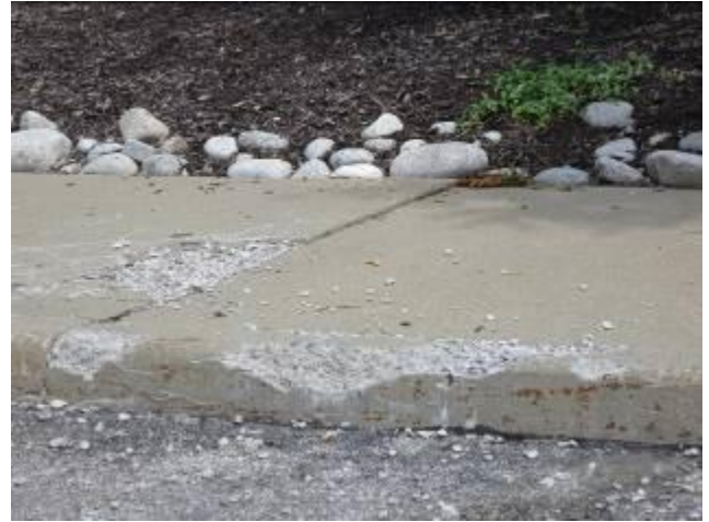
Deteriorated Sidewalk North-Central Parking Lot
