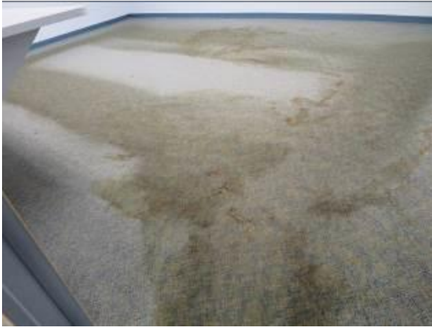
Damage & Mold In Carpets In Vacant Building
