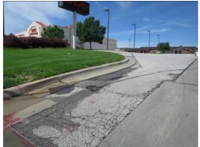
Damage At Holmes Road North Entrance
