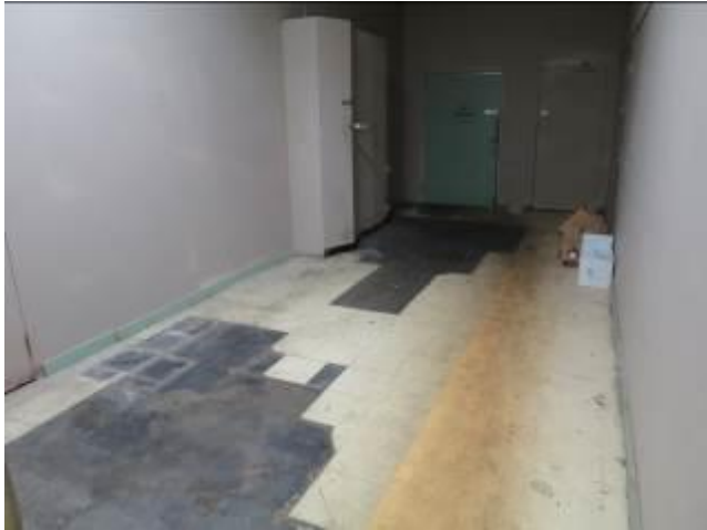
Damaged Floors In Small Shops
