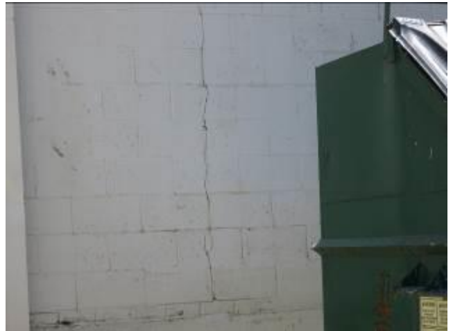
Wall Shearing – Courtyard Dock Area
