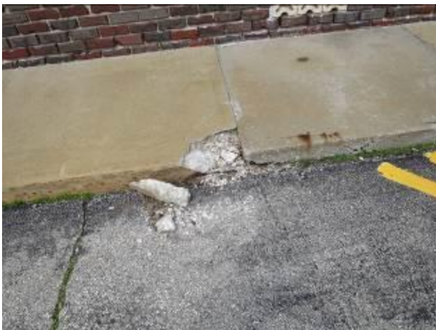
Deteriorated Sidewalk Vacant Building (E)
