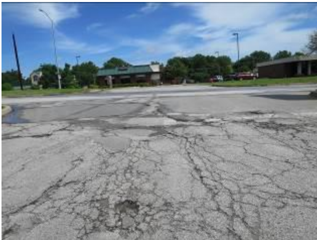
Damage At Red Bridge Road West Entrance
