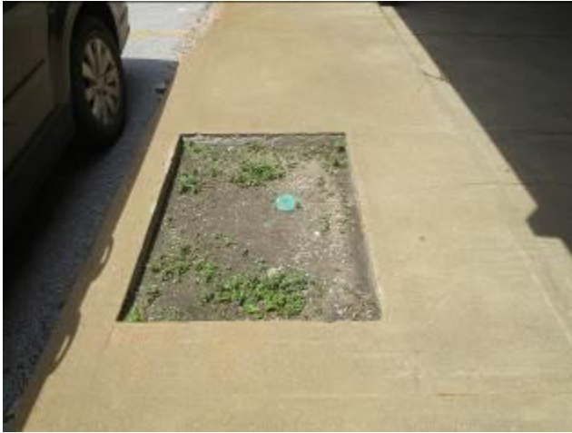
Sidewalk Planter – No Landscaping / Fall Hazard
