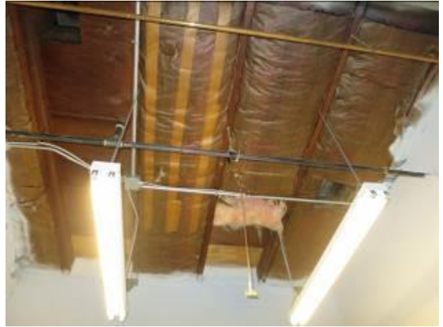
Lack Of Interior Ceiling Finish
