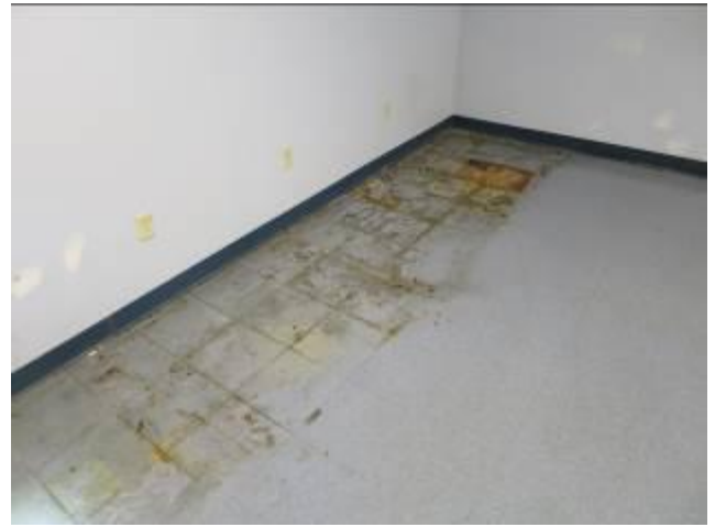
Damage & Mold In Tile In Vacant Building
