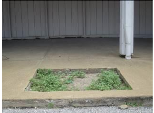
Sidewalk Planter – No Landscaping / Fall Hazard
