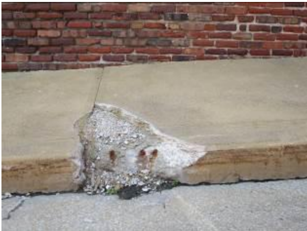
Deteriorated Sidewalk To Courtyard Dock
