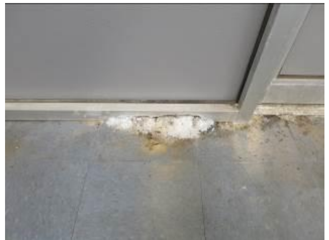
Rusting Exterior Door – Vacant Building
