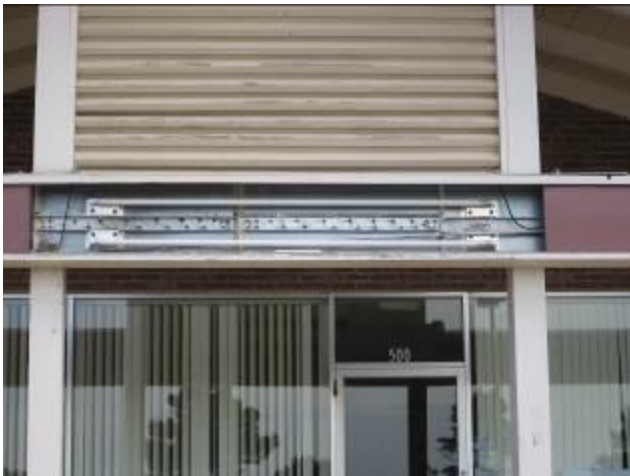
Damaged Signage Area – Retail Strip
