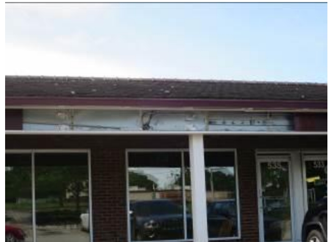
Damaged Signage Area – Retail Strip
