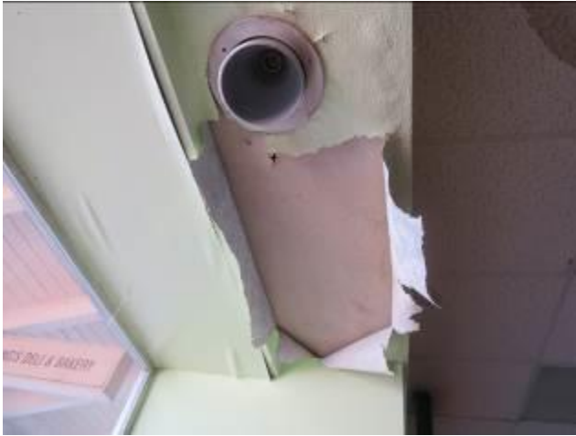
Ceiling Damage In Small Shops
