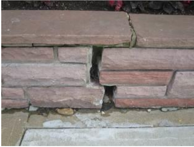
Deteriorated Sidewalk Landscaping Planter
