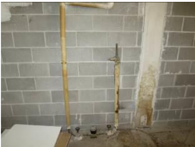
Compromised ACMs In Pipe Wrapping
