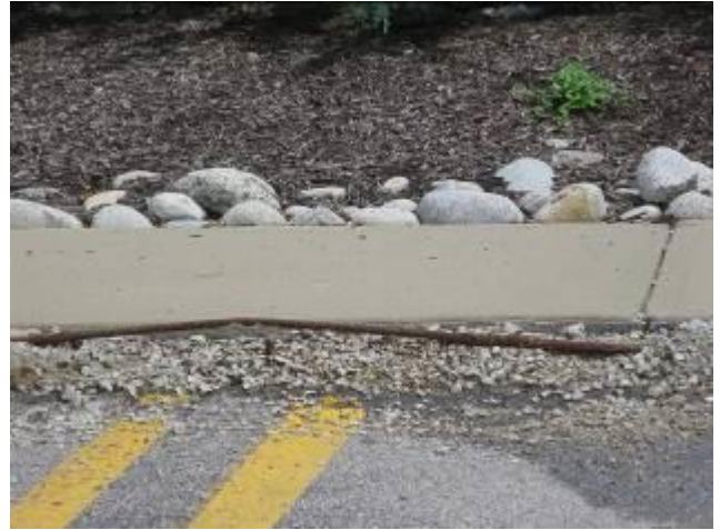
Exposed Rebar On Sidewalk Curbing
