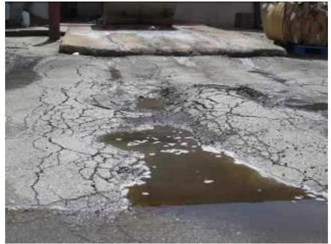
Discolored Standing Water
