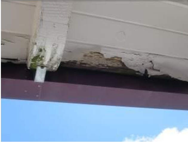
Rotted & Deteriorating Canopy – Retail Strip
