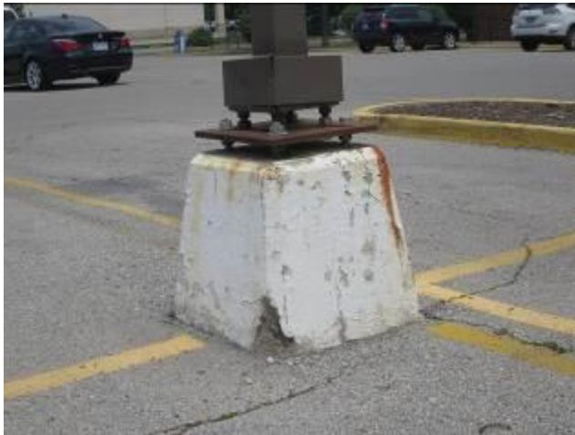
Deteriorated Parking Lot Lighting (East-Central)
