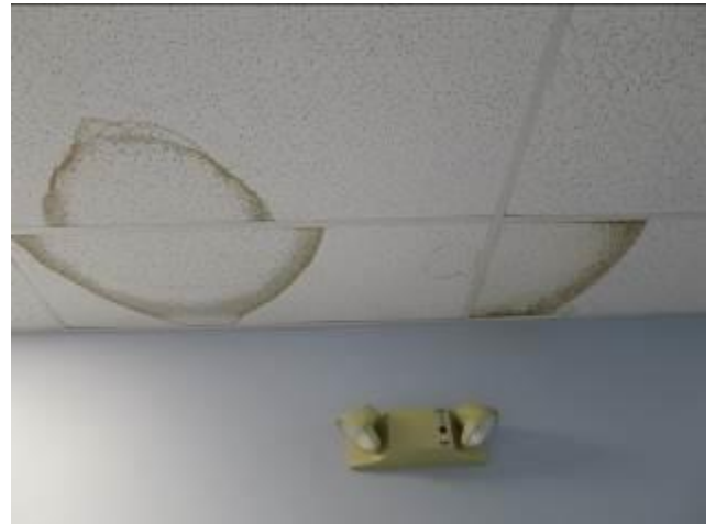
Ceiling Damage In Vacant Building
