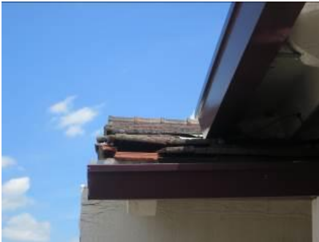
Deteriorating Roof Underlay
