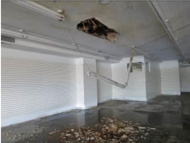
Ceiling Collapse In Vacant Small Shop (Roofer No Longer Allows Workers On This Roof)
