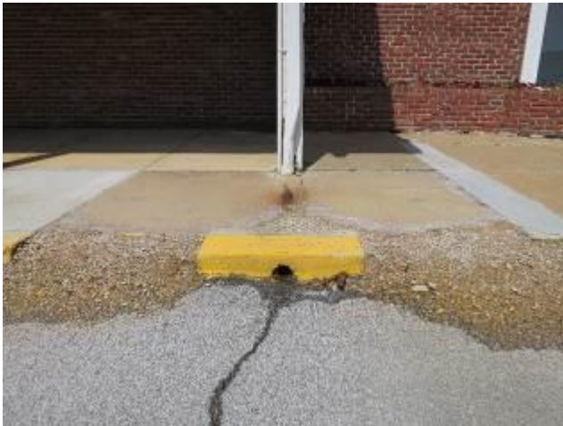
Deteriorated Curbing Retail Strip Building (E)
