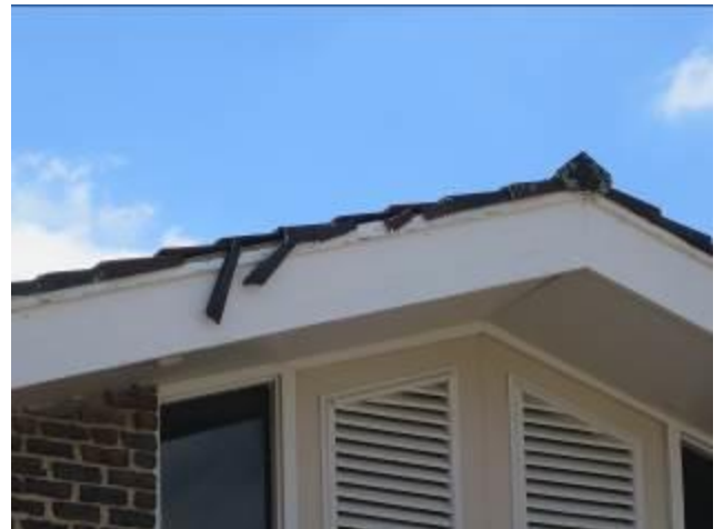
Damaged Roofing Retail Strip Building
