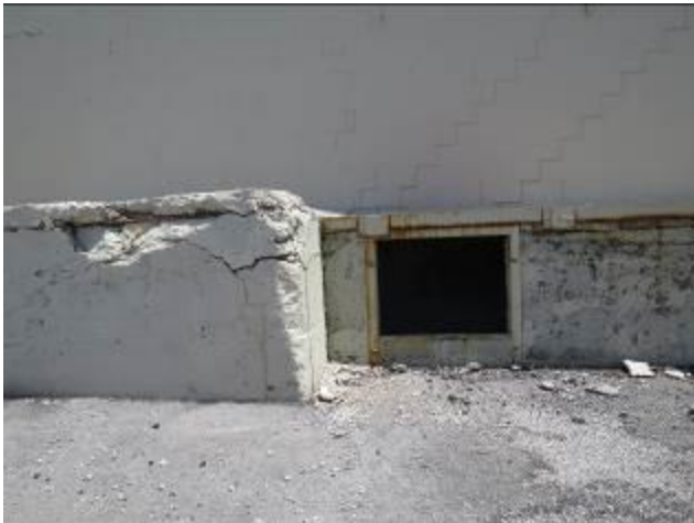
Rusted & Crumbling Dock Area
