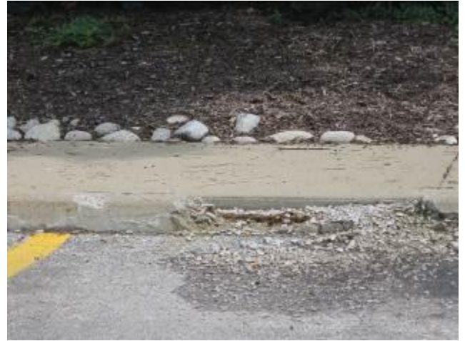
Deteriorated Curbing North-Central Parking Lot
