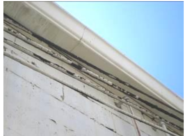
Hot/Exposed Wires (Google Workers Shocked)
