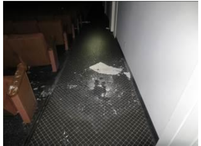
Ceiling Damage In Former Theater
