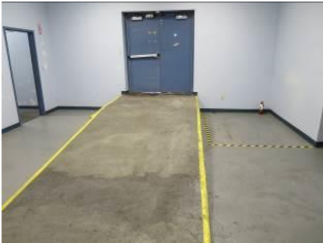
Ramp With No Railings – Vacant Building
