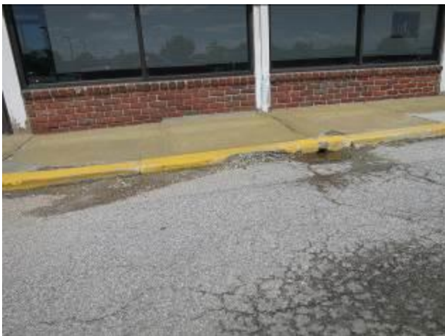
Deteriorated Curbing Retail Strip Building (E)
