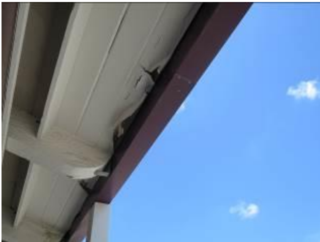
Rotted & Deteriorating Canopy – Retail Strip
