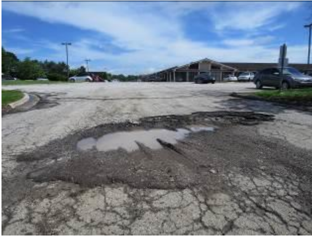
Deteriorated SWC Parking Lot
