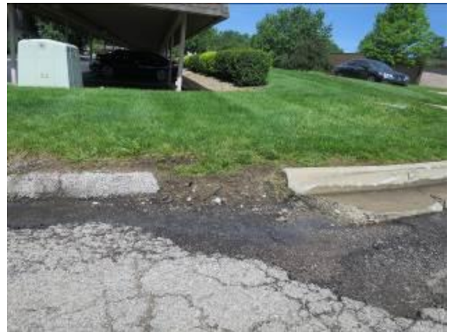
Damage Along E 112 th Street
