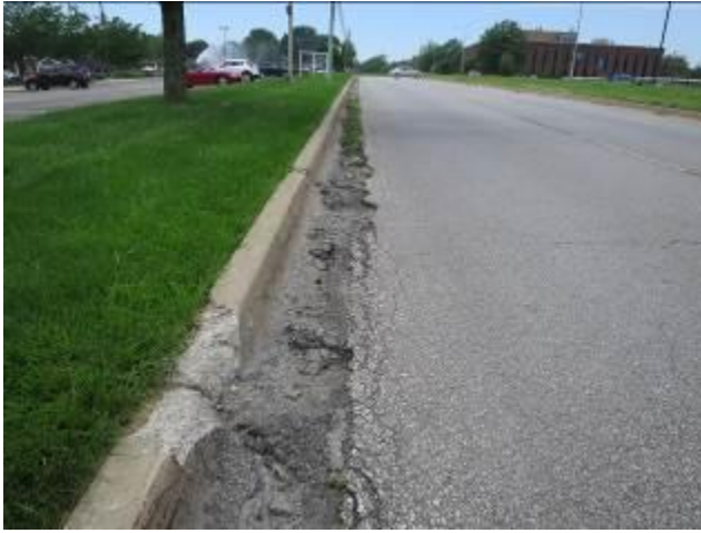
Deep Asphalt Lip On South Side Of Red Bridge Rd.
