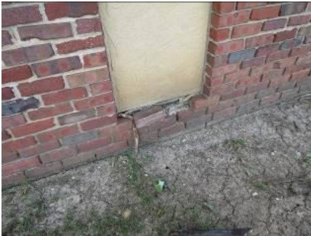
Wall Damage – Grocery Store
