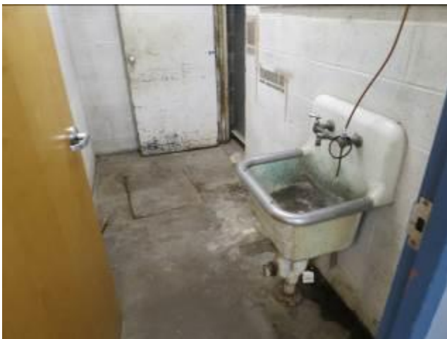
Unsightly Finish – Vacant Building
