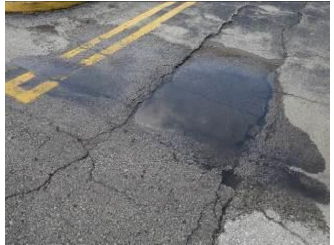
Deteriorated Central Parking Lot
