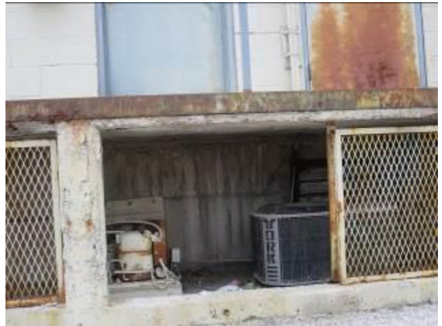
Obsolete A/C Compressors
