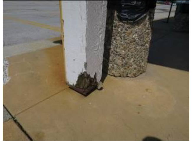
Rotted Canopy Support – Vacant Building
