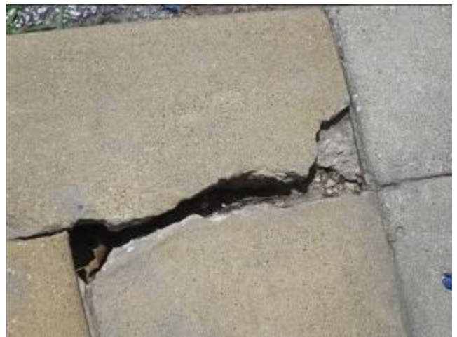
Deteriorated Sidewalk Retail Strip Building (N)
