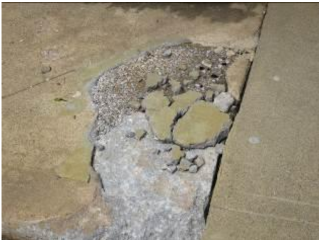
Deteriorated Sidewalk Retail Strip Building (W)
