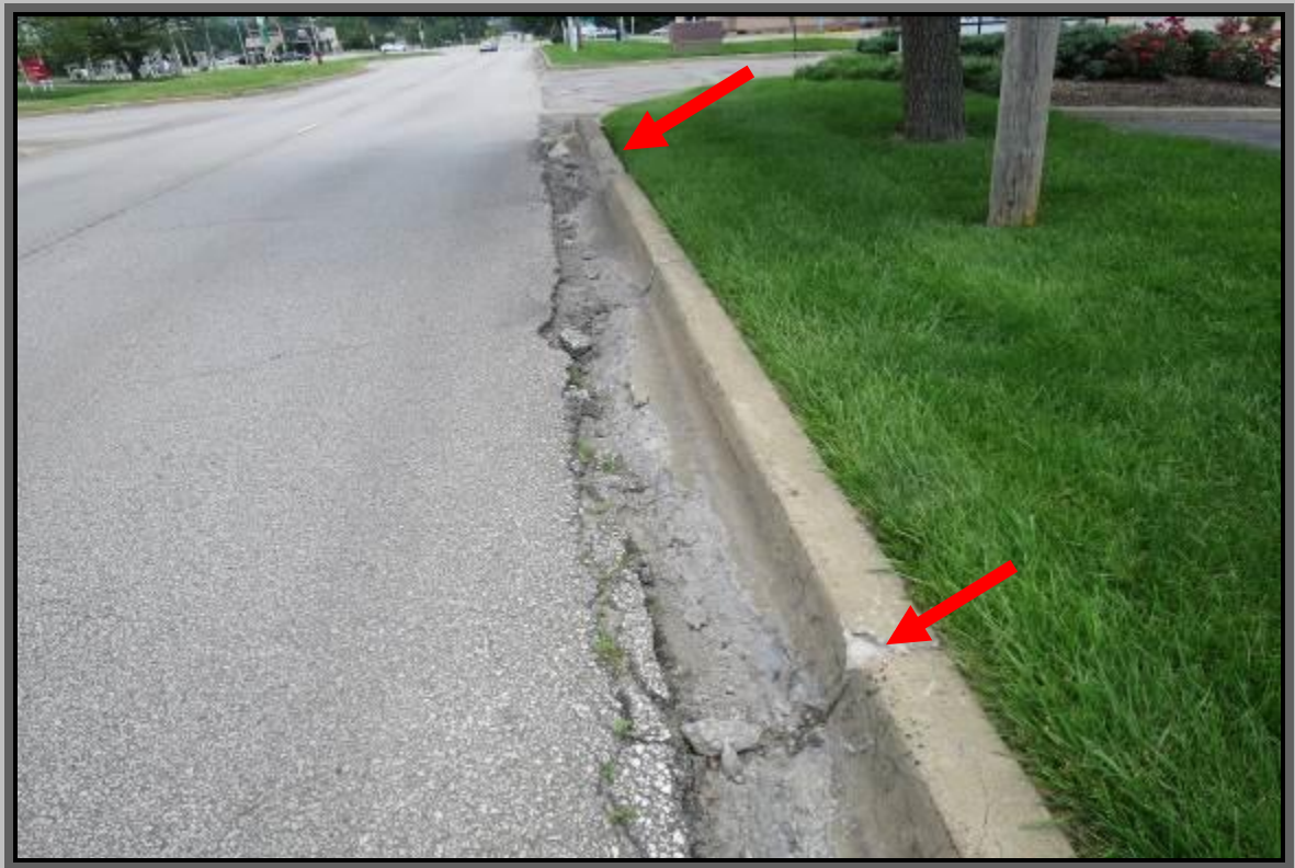
Deteriorating Curbing & Pavement Drop (To Gutter) Along Eastbound Lane of Red Bridge Road
