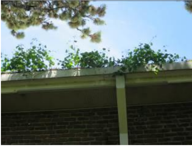
Vegetation Growth In Vacant Building Gutter
