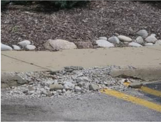
Deteriorated Sidewalk North-Central Parking Lot
