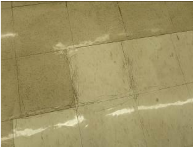
Deteriorating Tile In Grocery
