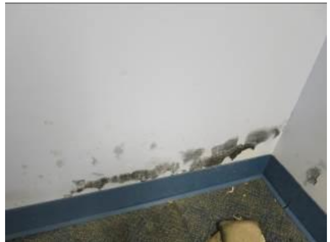
Mold In Wall & Carpet
