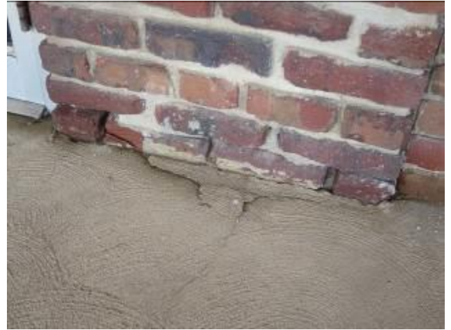
Wall Damage – Retail Strip Building
