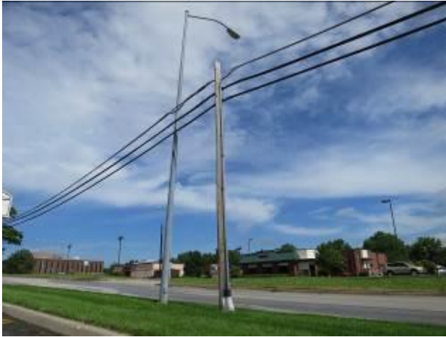
Unsightly Overhead Power Lines
