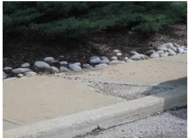
Deteriorated Sidewalk North-Central Parking Lot
