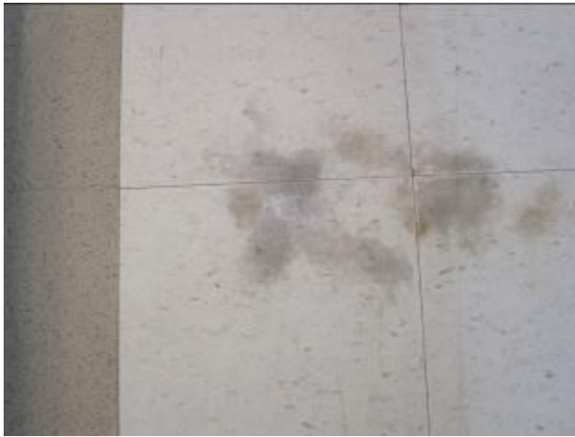
Deteriorating Tile In Grocery
