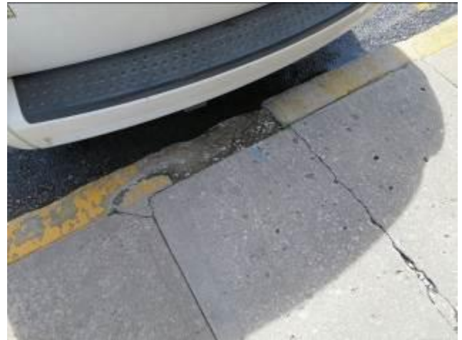
Deteriorated Curbing Retail Strip Building (S)
