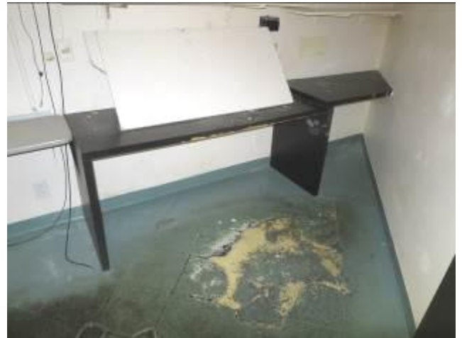
Deteriorated Floors In Small Shops
