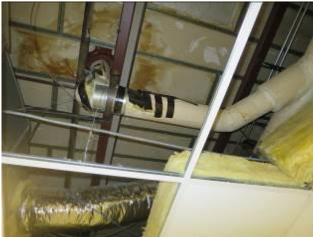
ACMs In Pipe Wrapping
