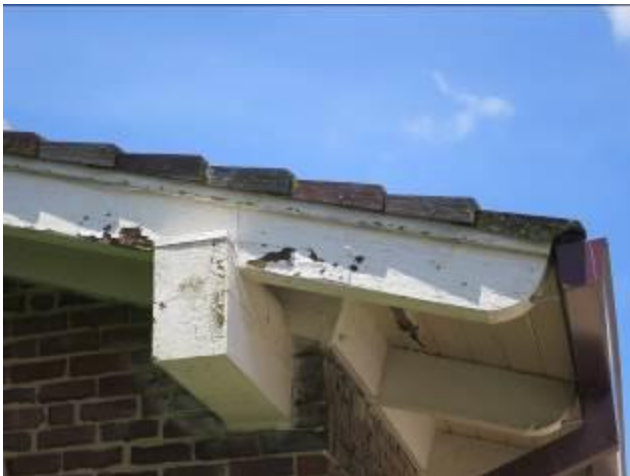
Deteriorating Roof Supports & Soffit – Retail Strip
