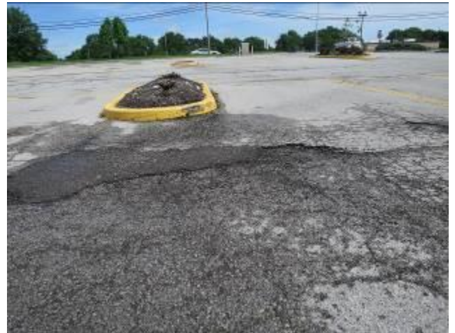
Deteriorated North-Central Parking Lot
