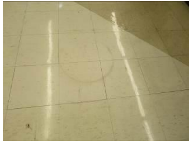
Deteriorating Tile In Grocery
