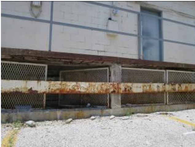
Deteriorating Dock Area
