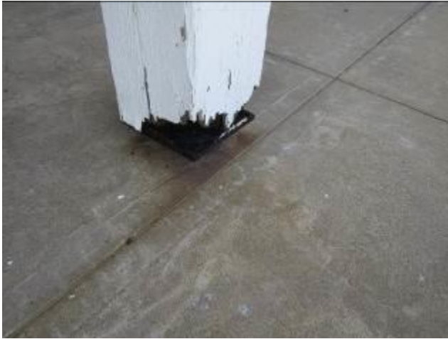
Rotted Canopy Support – Retail Strip
