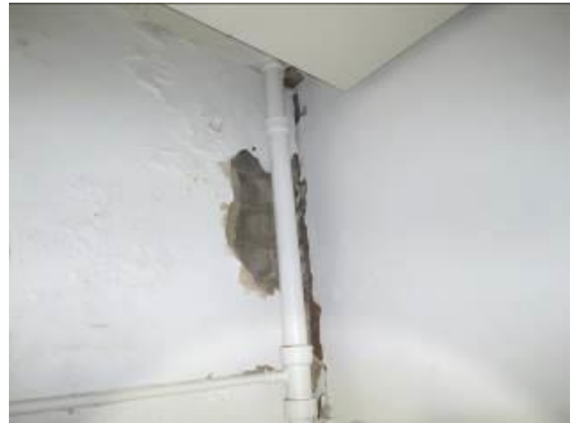
Wall Damage In Small Shops
