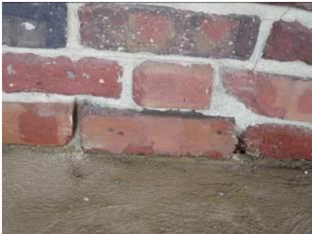
Deteriorated Sidewalk Landscaping Planter
