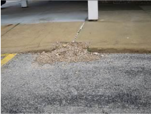
Deteriorated Curbing Retail Strip Building (E)
