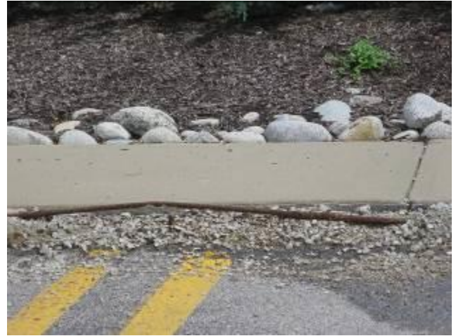
Deteriorated Curbing North-Central Parking Lot
