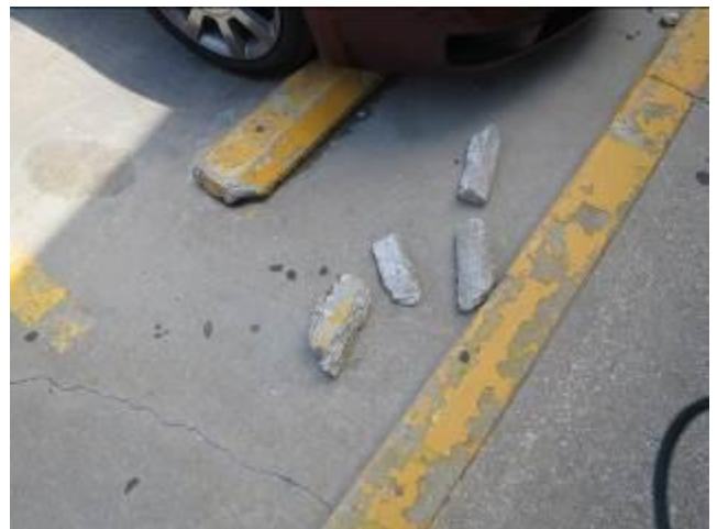
Deteriorated Parking Block At Grocer
