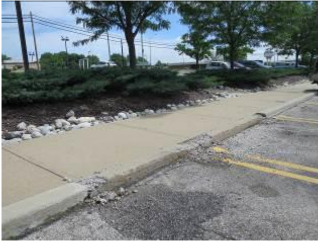
Deteriorated Curbing North-Central Parking Lot
