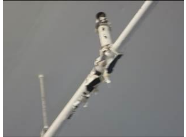
Deteriorating Fire Sprinklers – Vacant Building
