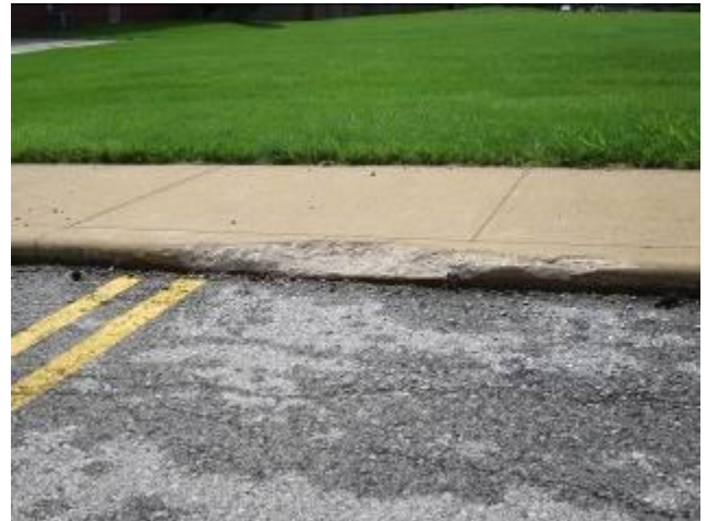
Deteriorated Curbing Northwest Parking Lot
