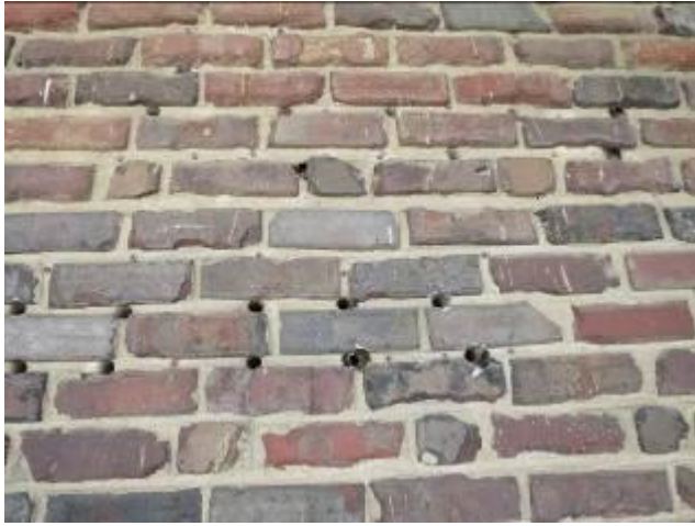
Wall Damage – Vacant Building
