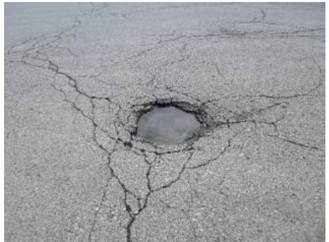
Parking Lot Pothole
