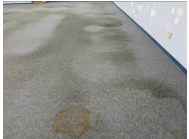
Damage & Mold In Carpets In Vacant Building
