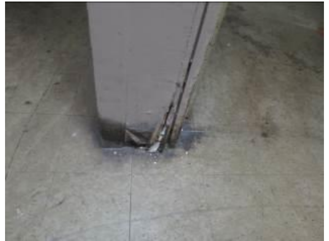
Wall Damage In Small Shops
