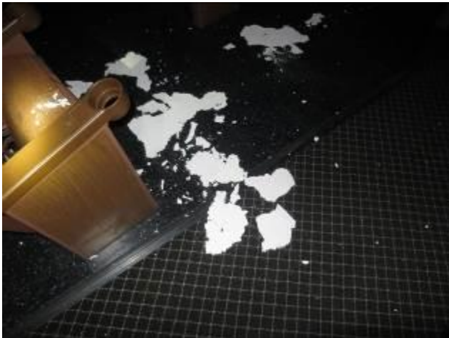
Ceiling Damage In Former Theater
