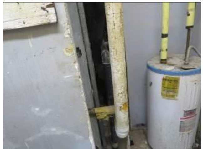
Compromised ACMs In Pipe Wrapping
