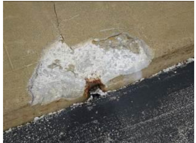
Deteriorated Vacant Building (E)
