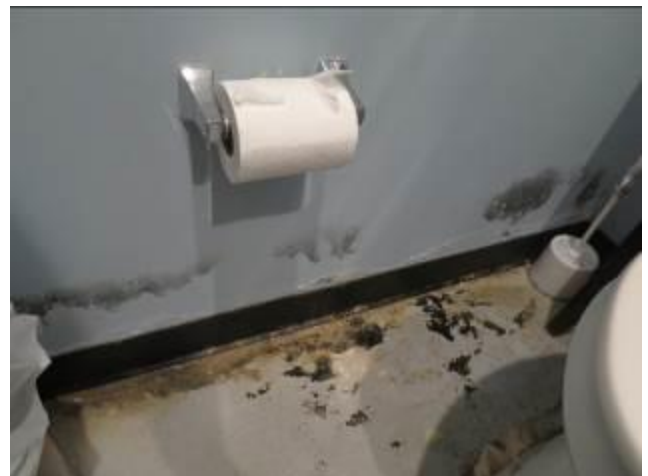
Mold In Wall & Tile
