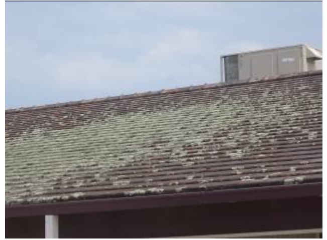
Lichen Growth On Clay Tile Mansard – Retail Strip
