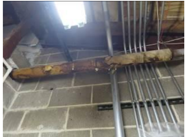
Compromised ACMs In Pipe Wrapping
