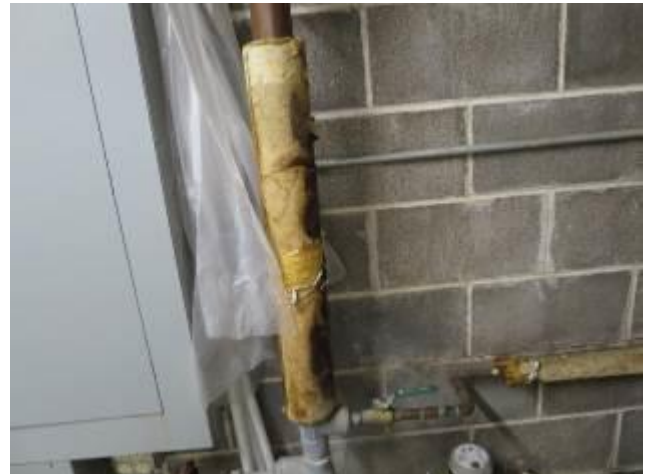
Compromised ACMs In Pipe Wrapping
