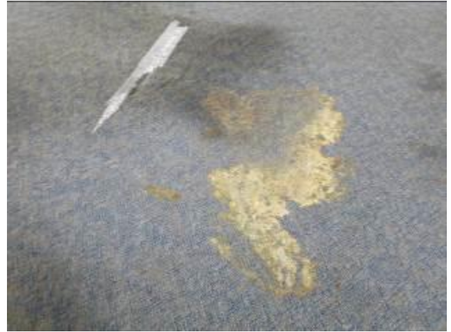
Damage & Mold In Carpets In Vacant Building
