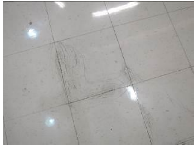
Deteriorating Tile In Grocery
