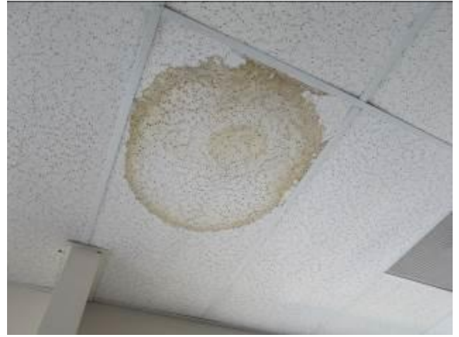
Ceiling Damage In Small Shops
