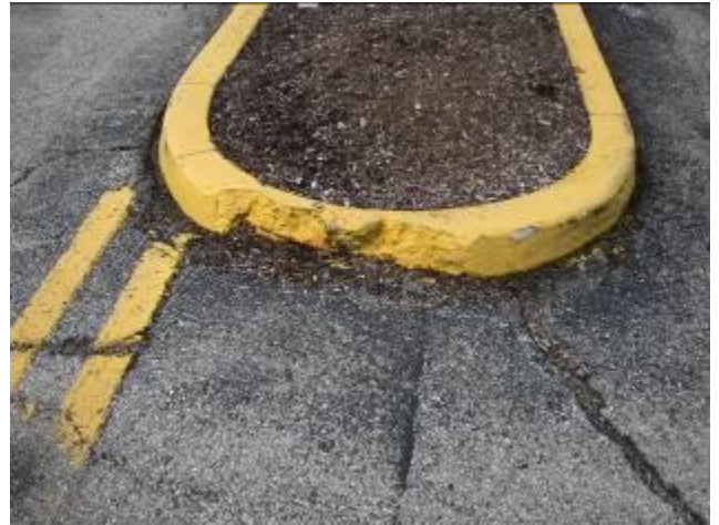
Deteriorated Landscape Planter SWC Parking Lot
