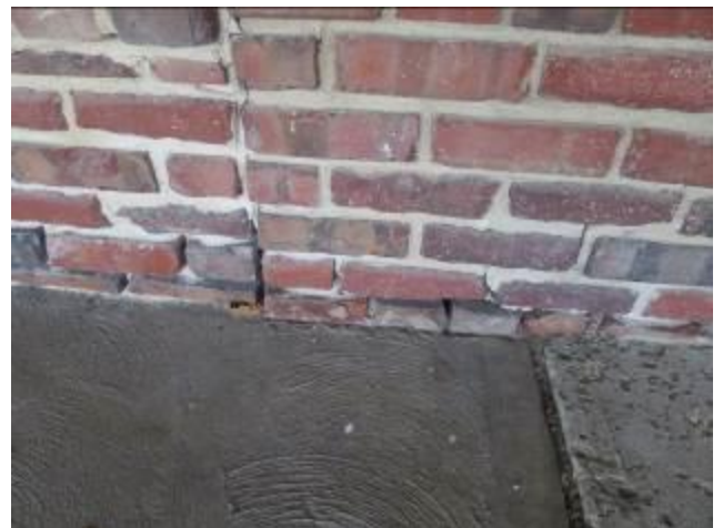
Wall Deterioration – Retail Building
