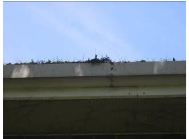
Filled Gutters In Vacant Building
