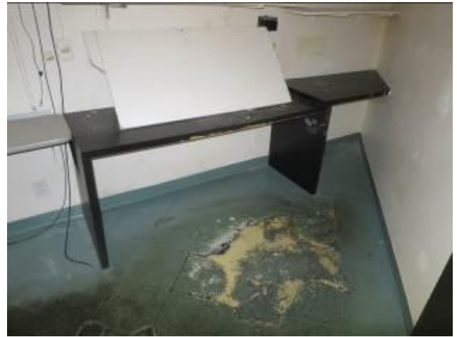
Compromised ACT Flooring (ACMs)
