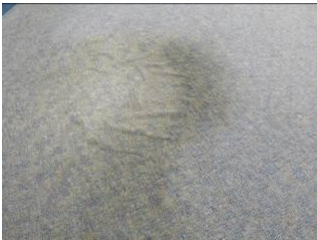
Damage & Mold In Carpets In Vacant Building
