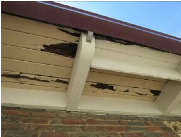
Rotted & Deteriorating Canopy Retail Strip
