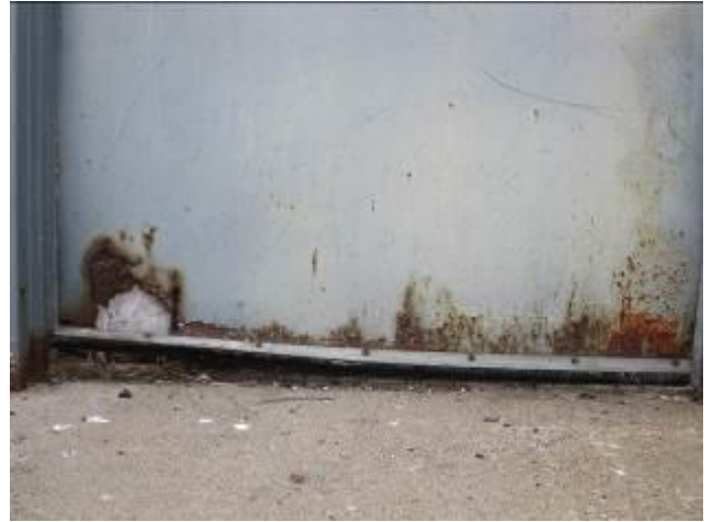
Rusted Door – Retail Strip
