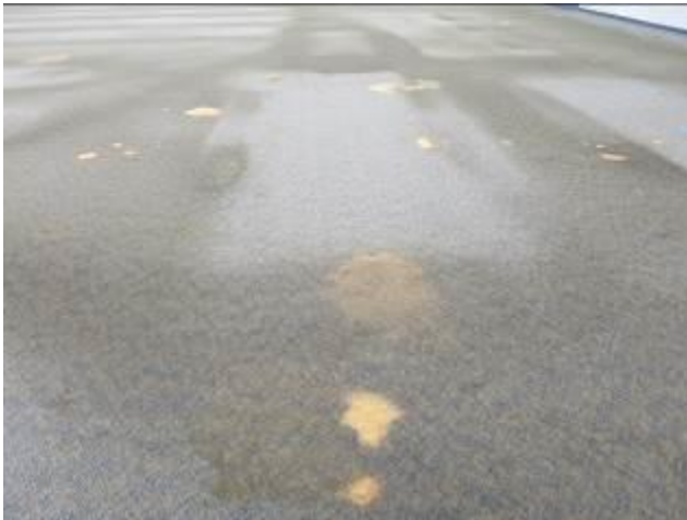
Damage & Mold In Carpets In Vacant Building
