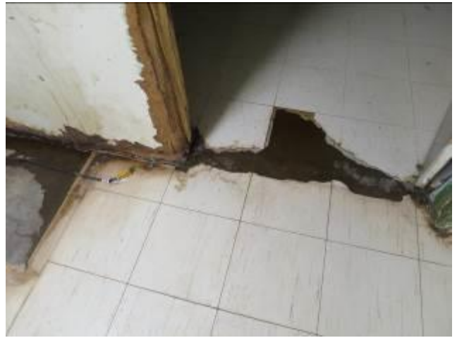
Damaged Floors In Small Shops
