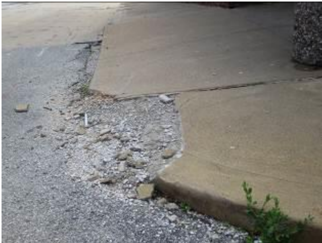
Deteriorated Sidewalk Retail Strip Building (NW)
