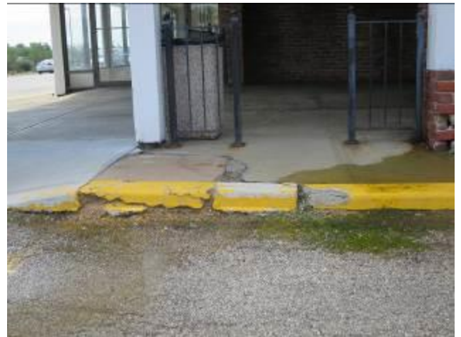
Deteriorated Curbing Retail Strip Building (NEC)
