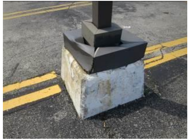
Deteriorated Parking Lot Lighting (W)
