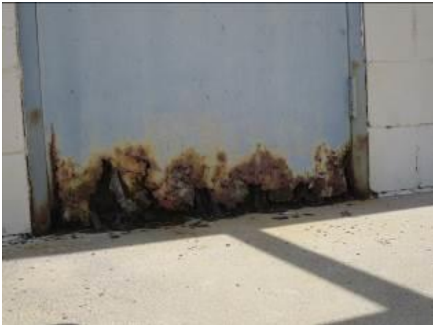
Rusting Exterior Door – Retail Strip
