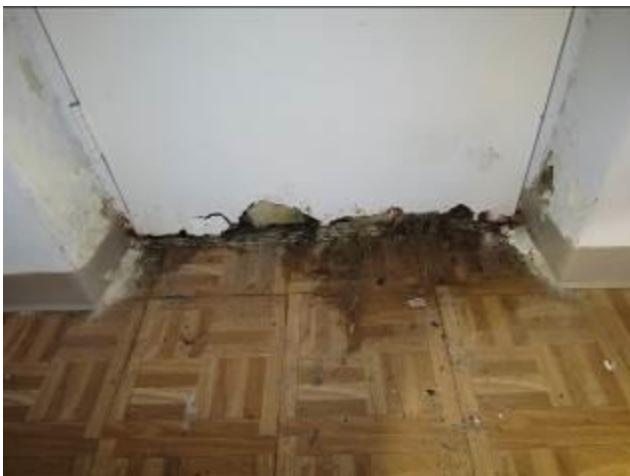
Rusting Interior Door – Retail Strip
