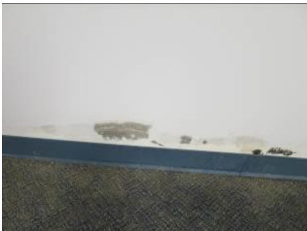
Mold In Wall & Carpet
