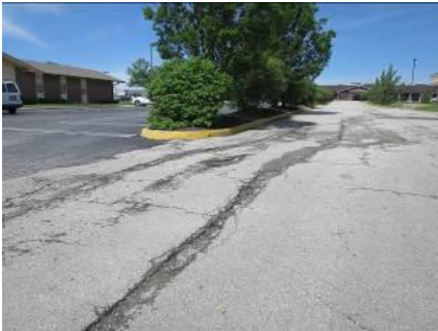
Damage At Holmes Road Central Driveway
