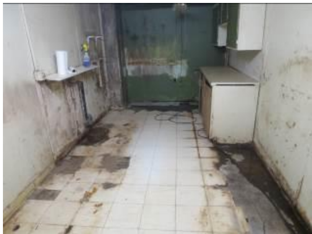
Damage & Mold In Floors Small Shops
