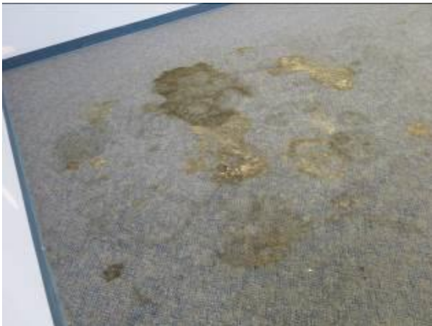
Damage & Mold In Carpets In Vacant Building
