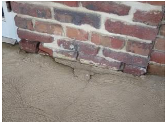
Deteriorated Sidewalk Landscaping Planter
