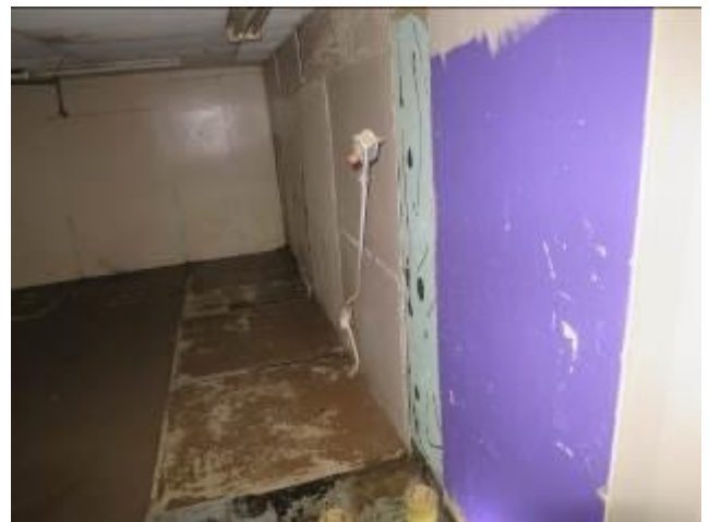
Damaged/Deteriorating Wall & Floors Small Shop
