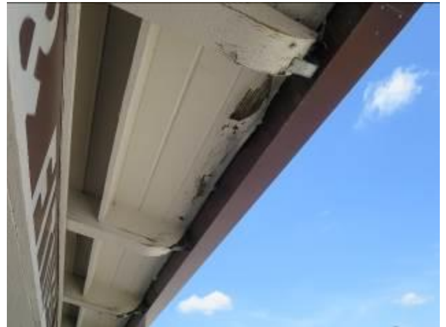
Rotted & Deteriorating Canopy – Retail Strip
