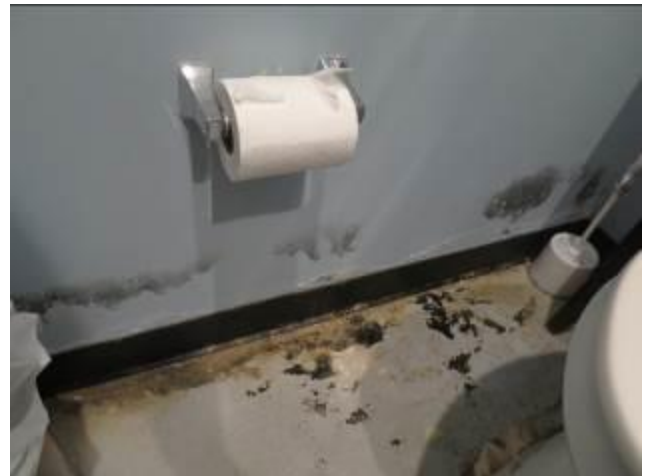
Wall Damage/Mold In Small Shops
