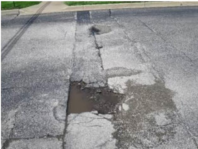
Parking Lot Pothole
