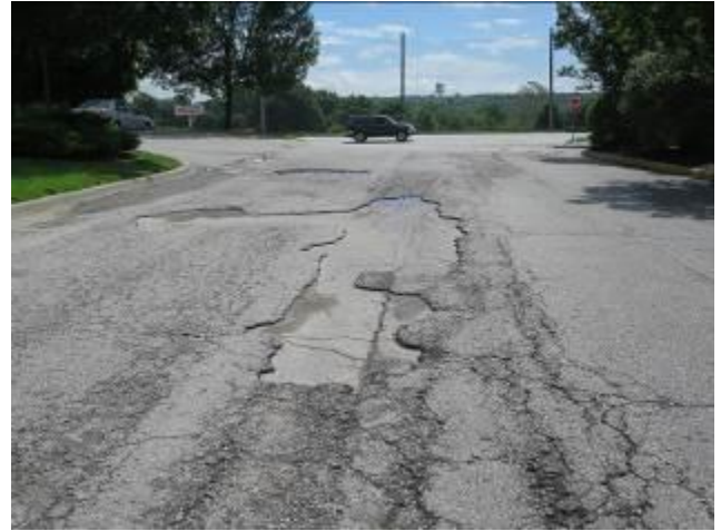
Damage At Holmes Road Central Entrance
