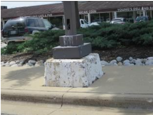
Deteriorated Parking Lot Lighting (N)
