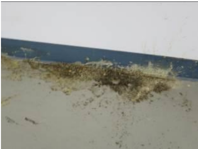
Deteriorated Floors In Small Shops
