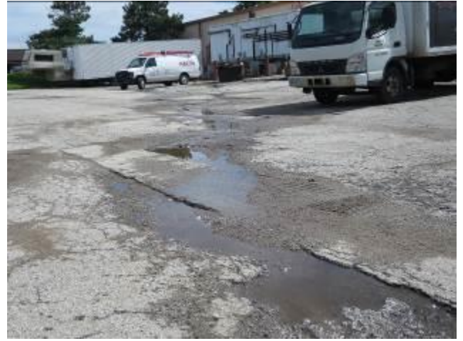
Deteriorated Parking Lot Behind Grocer
