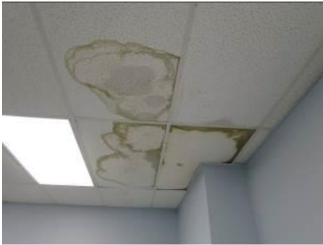
Ceiling Damage In Vacant Building
