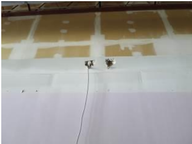
Wall Damage In Small Shops
