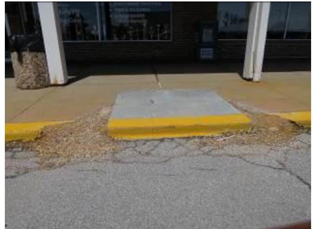
Deteriorated Sidewalk Retail Strip Building (E)
