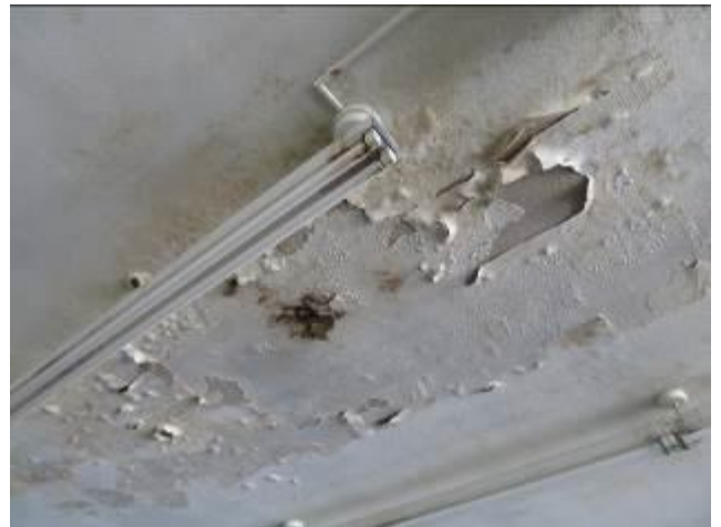
Ceiling Damage In Small Shops
