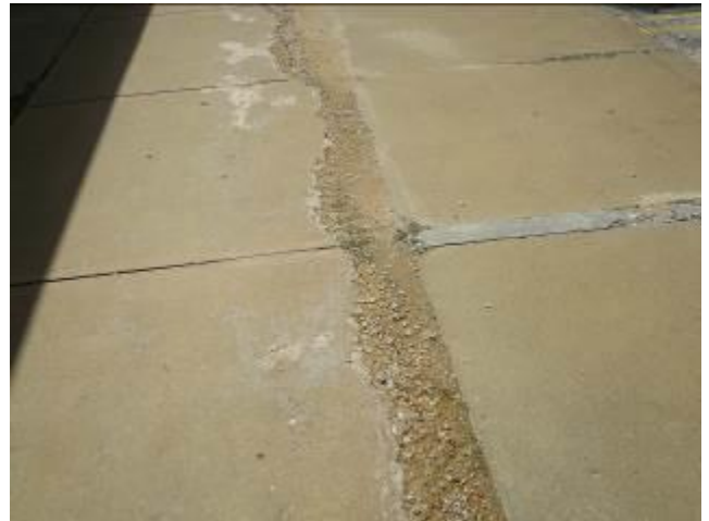
Deteriorated Sidewalk Vacant Building (N)
