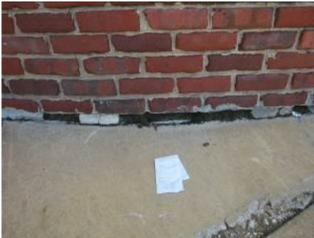
Deteriorated Sidewalk Landscaping Planter
