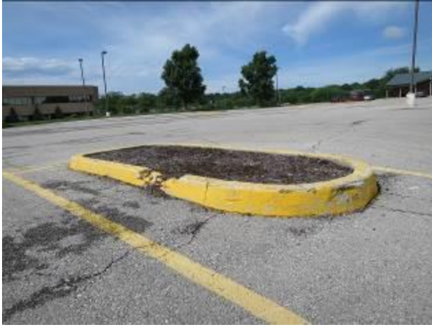
Deteriorated Landscape Planter NEC Parking Lot
