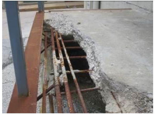
Deteriorating Dock Area
