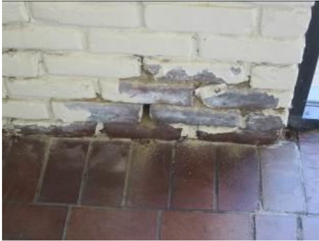
Wall Damage In Theater
