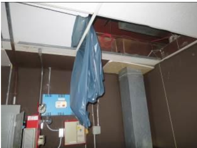
Ceiling Damage In Former Theater
