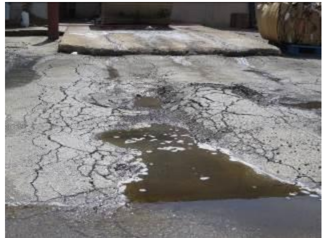
Deteriorated Grocery Dock Area
