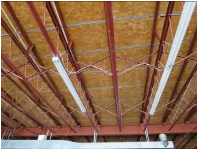
Lack Of Interior Ceiling Finish
