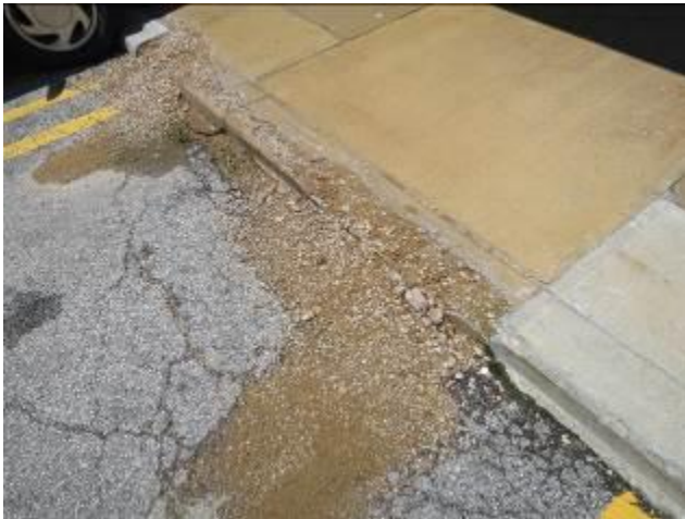
Deteriorated Curbing Retail Strip Building (E)
