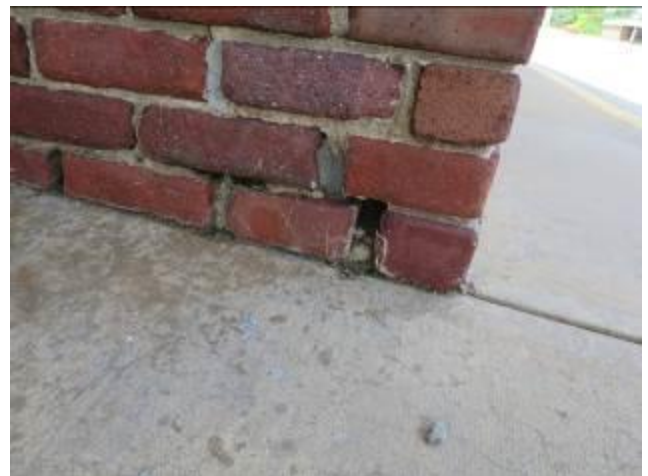
Deteriorated Sidewalk Landscaping Planter
