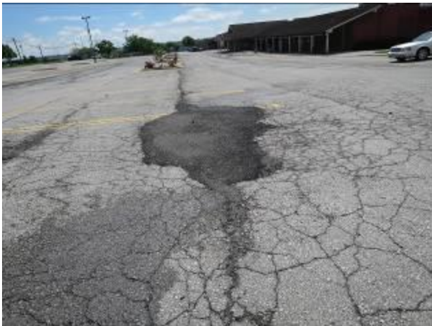
Deteriorated Parking Lot Fronting Vacant Building
