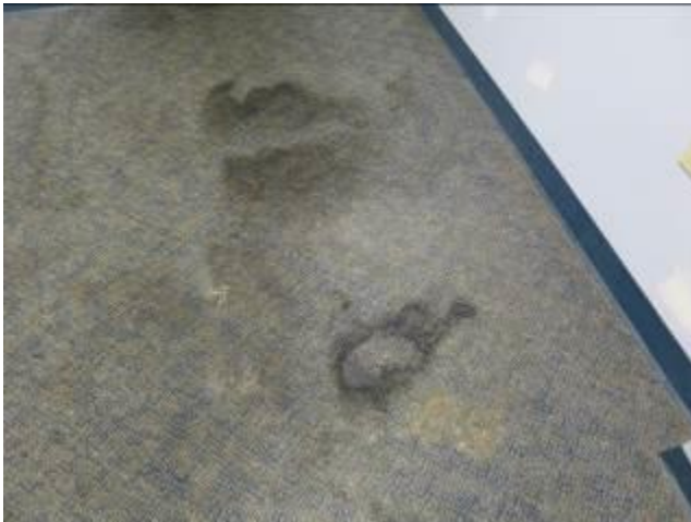
Damage & Mold In Carpets In Vacant Building
