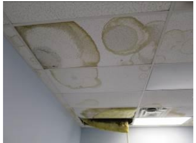
Ceiling Damage In Vacant Building
