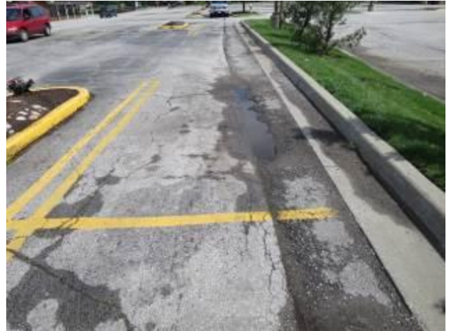
Deteriorated North-Central Parking Lot
