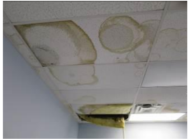
Mold In Water Damaged Ceiling Tile
