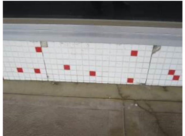
Wall Damage – Retail Strip Building
