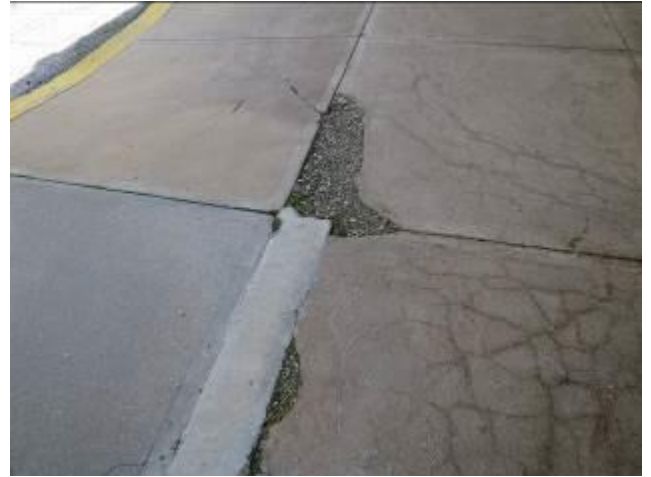
Deteriorated Sidewalk Retail Strip Building (N)
