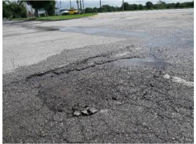
Parking Lot Damage
