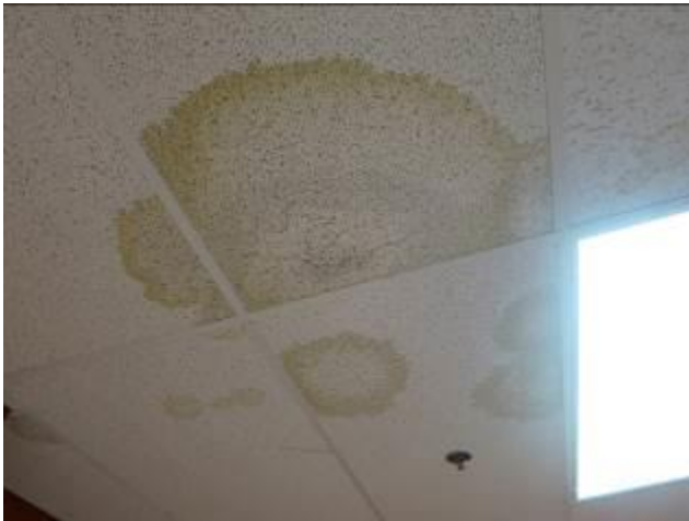
Ceiling Damage In Small Shops
