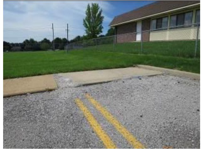
Deteriorated Sidewalk Daycare
