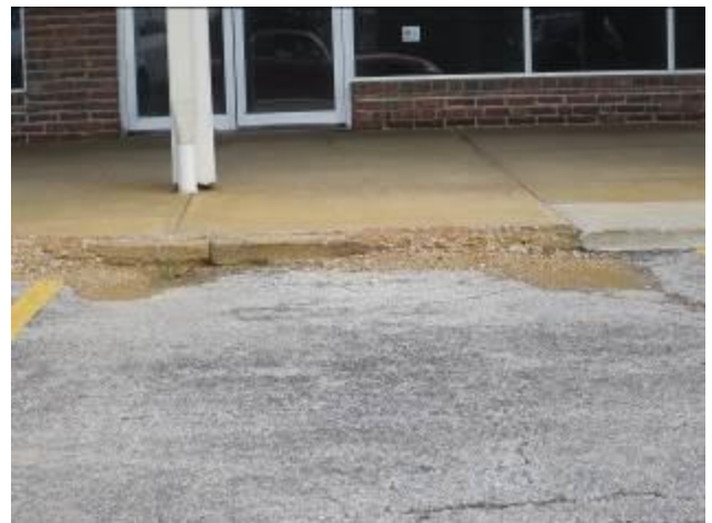
Deteriorated Curbing Retail Strip Building (E)
