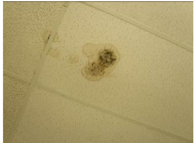
Ceiling Damage In Grocery
