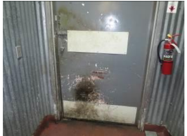
Rusting Interior Door – Retail Strip
