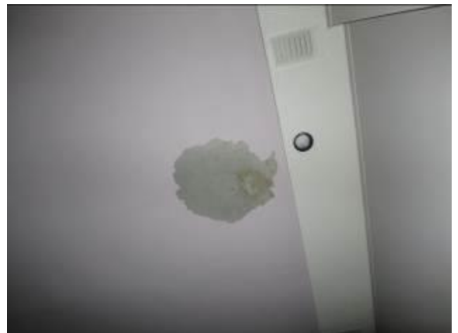
Ceiling Damage In Former Theater
