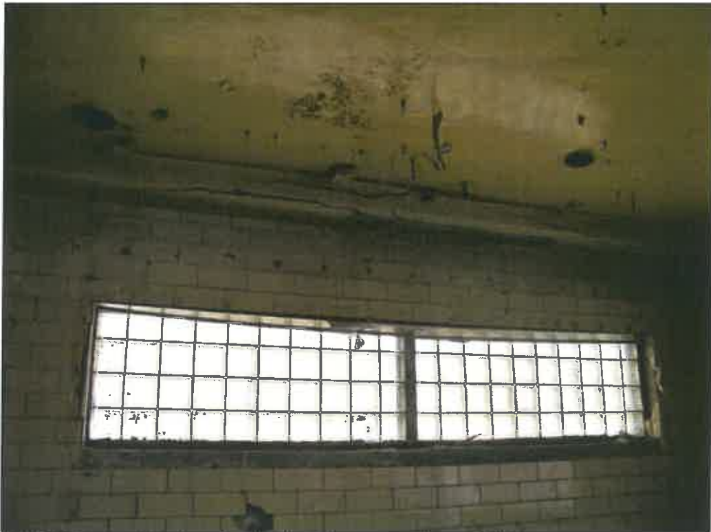
327 E. 31 st Street – interior – deterioration of structure, failure of finishes
