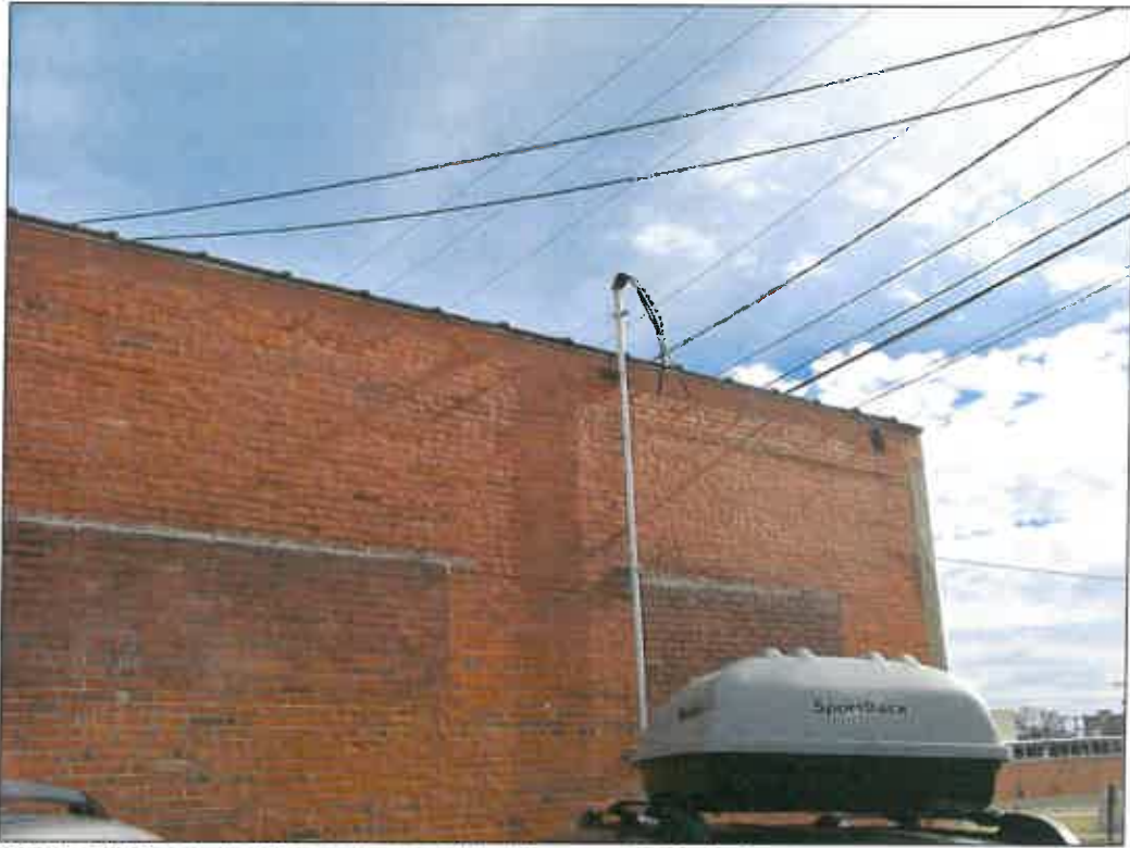
327 E. 31 st Street – looking east – electricity disconnected, lack of meter
