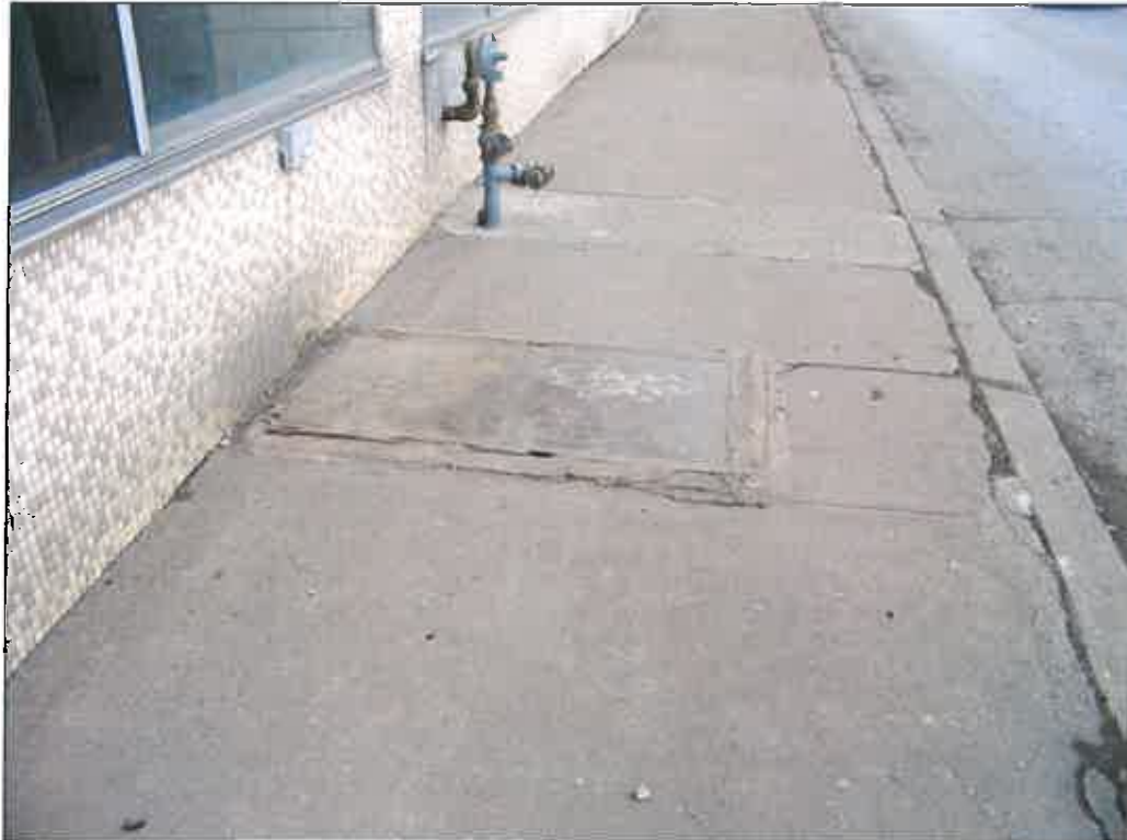
327 E. 31 st St – looking west – uneven/cracked sidewalk; deterioration of wall veneer
