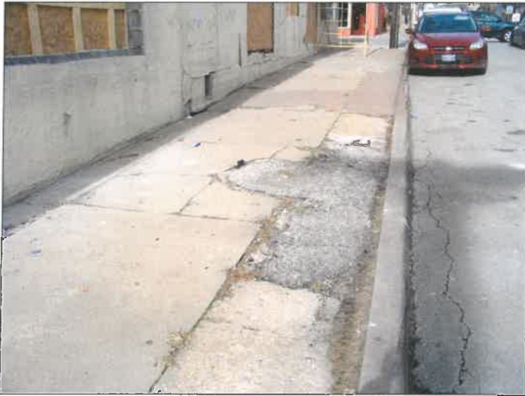
327 E. 31 st Street – looking north – uneven/cracked sidewalk; deterioration of walls, windows
