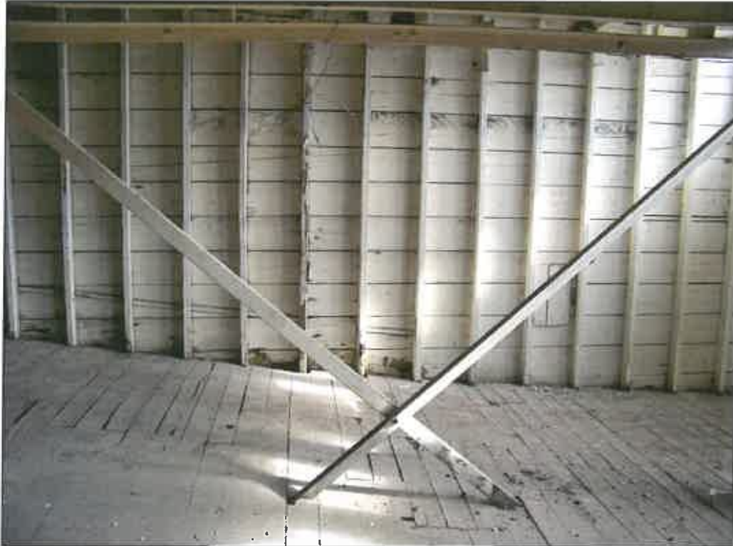
327 E. 31 st Street – interior – uneven floor
