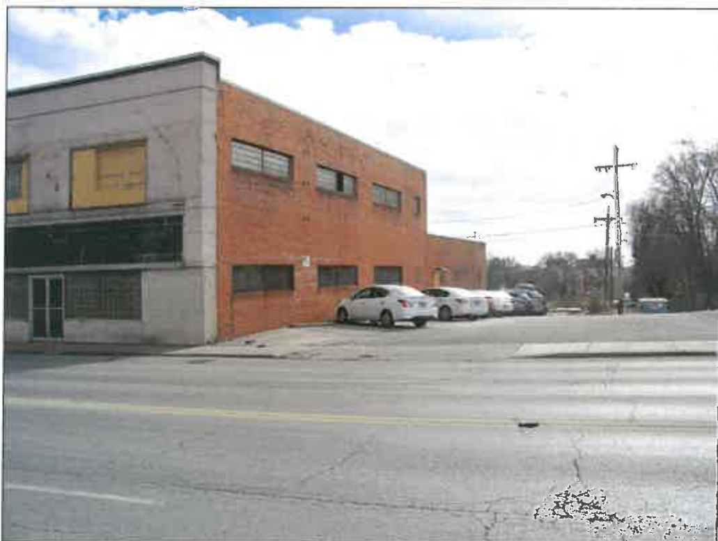
327 E. 31 st Street – looking southeast – deterioration of windows and wall veneer; failure of finishes
