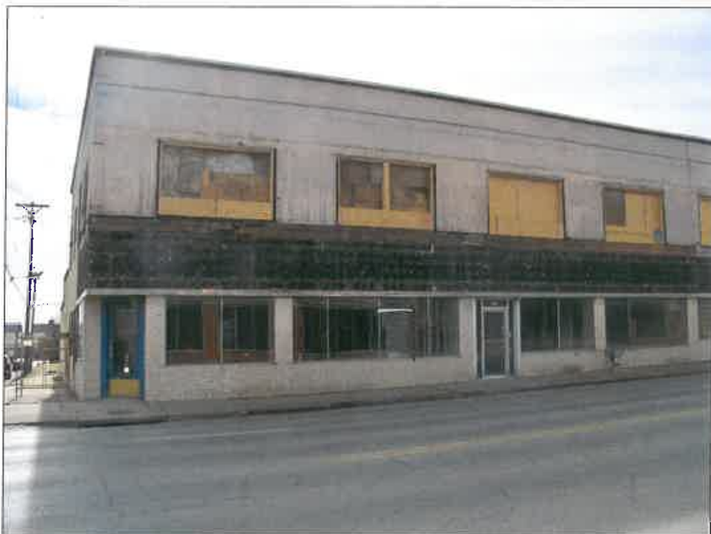
327 E 31 st Street – looking south – deterioration of windows, wall veneer, header joist, failure of finishes
