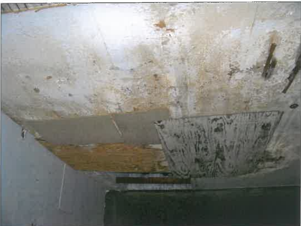
327 E. 31 st Street – interior – water damage due to leaking roof; failure of finishes
