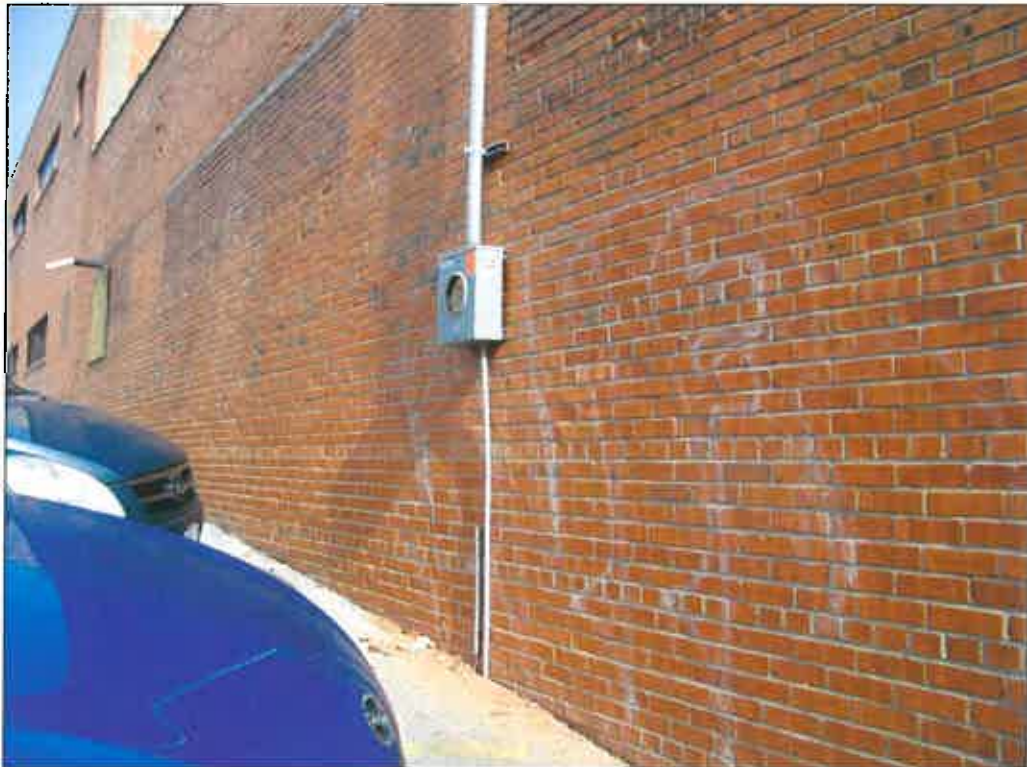
327 E. 31 st Street – looking east – graffiti; disconnected electricity (no meter)
