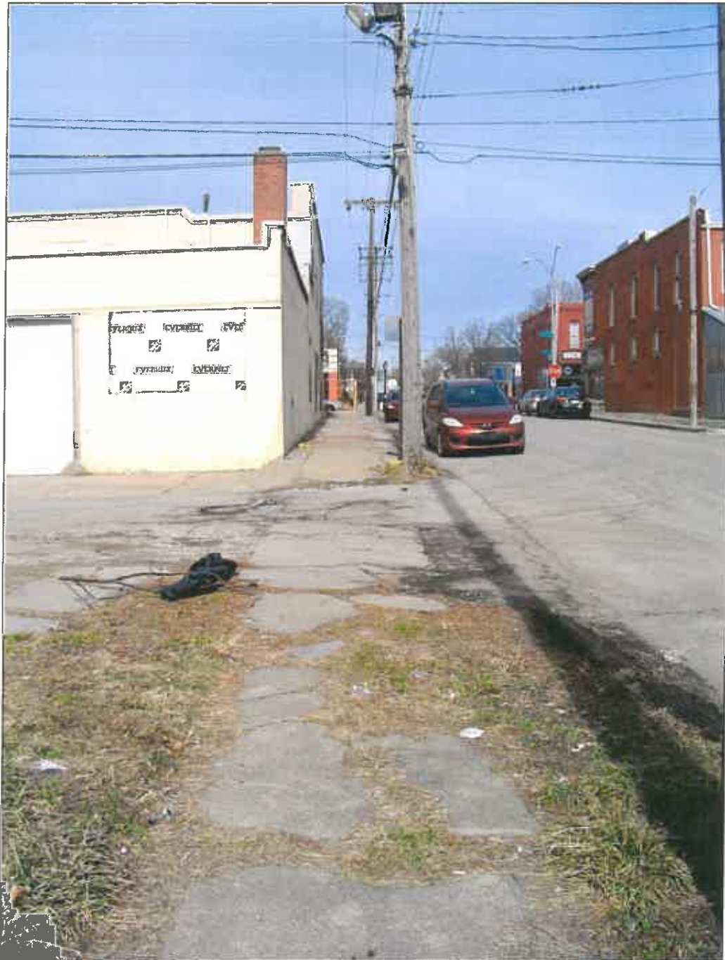
3108 Oak Street – looking north – cracked/uneven sidewalk; trash/debris; deterioration of wall veneer
