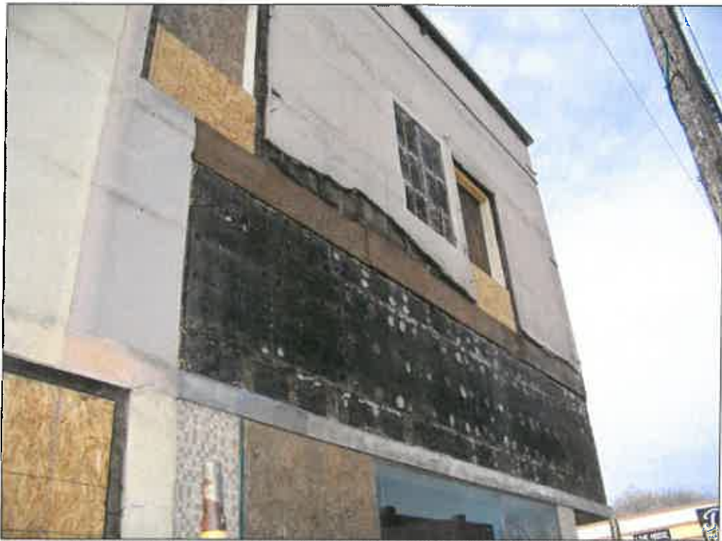
327 E. 31 st Street – looking northwest – deterioration of windows and wall veneer; failure of finishes
