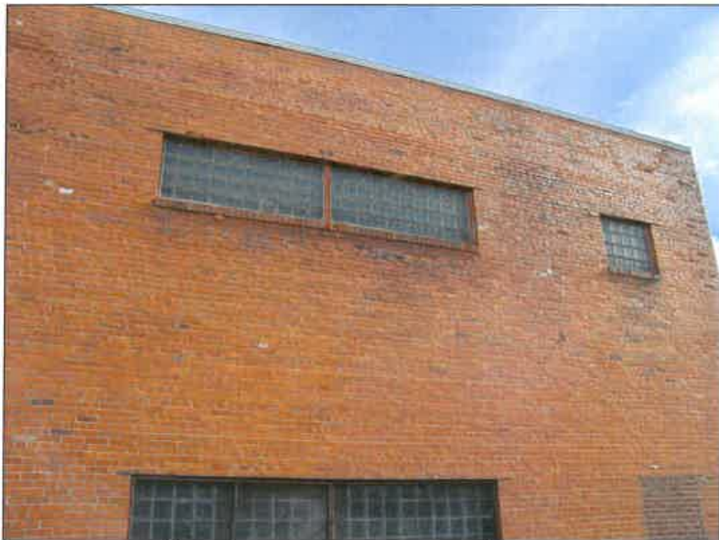
327 E. 31 st Street – looking east – deterioration of window lintels, brick masonry
