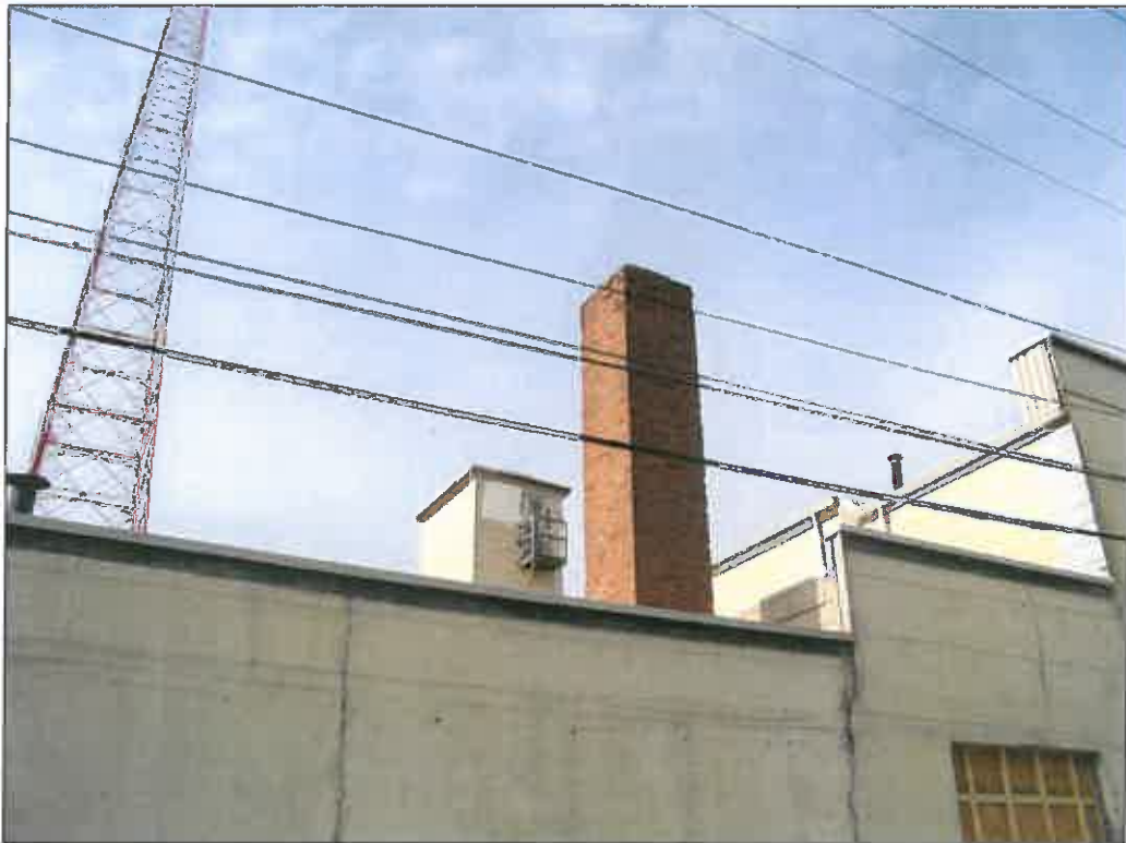
327 E. 31 st Street – looking west – masonry deterioration (chimney); deterioration of ladder, landing
