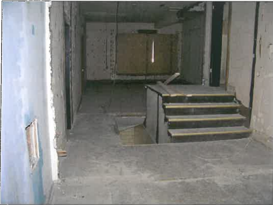
327 E. 31 st Street – interior – lack of railings; debris; lack of light
