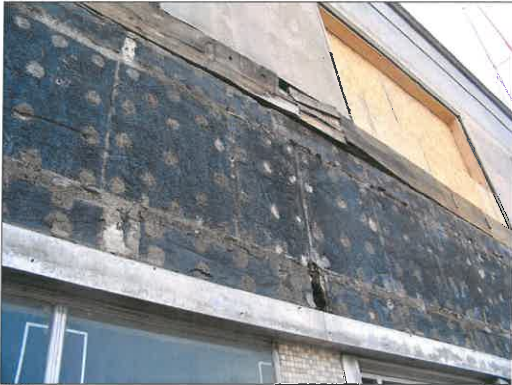
327 E. 31 st Street – looking southwest – deterioration of windows and wall veneer; failure of finishes
