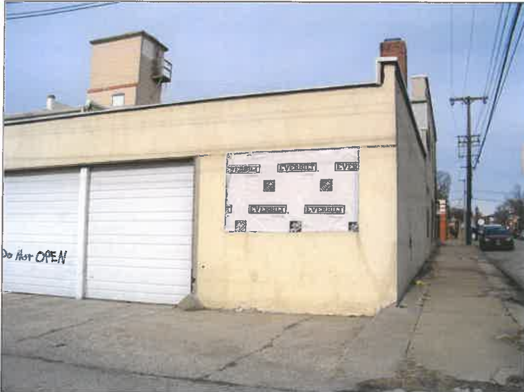
327 E 31 st Street – looking north – deterioration of wall veneer (stucco), windows, door assembly
