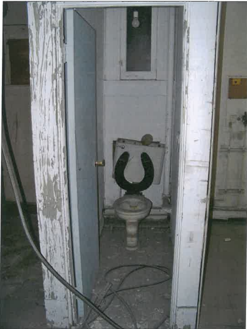
327 E. 31 st Street – interior – code noncompliance; loose electrical conduit; failure of finishes
