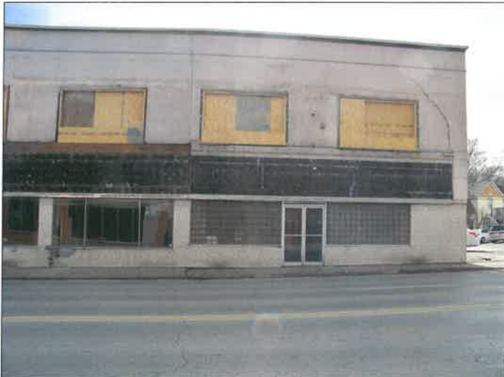
327 E 31 st Street – looking south – deterioration of wall veneer (stucco and tile), flashing, windows
