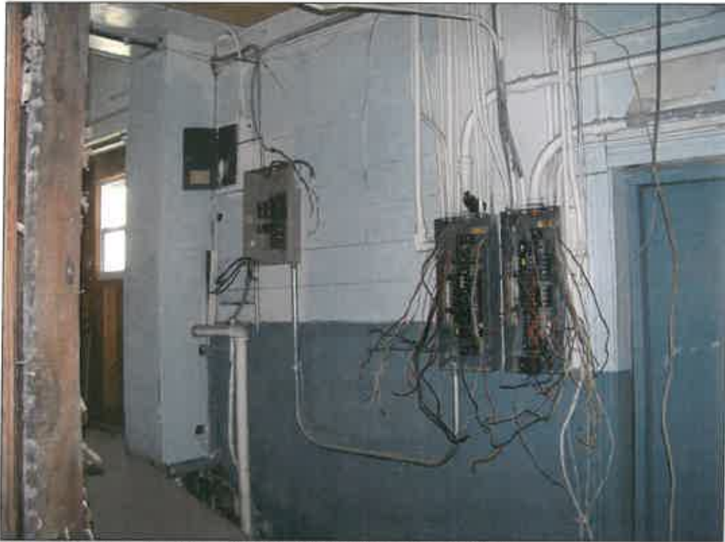
327 E. 31 st Street – interior – disconnected power; failure of finishes
