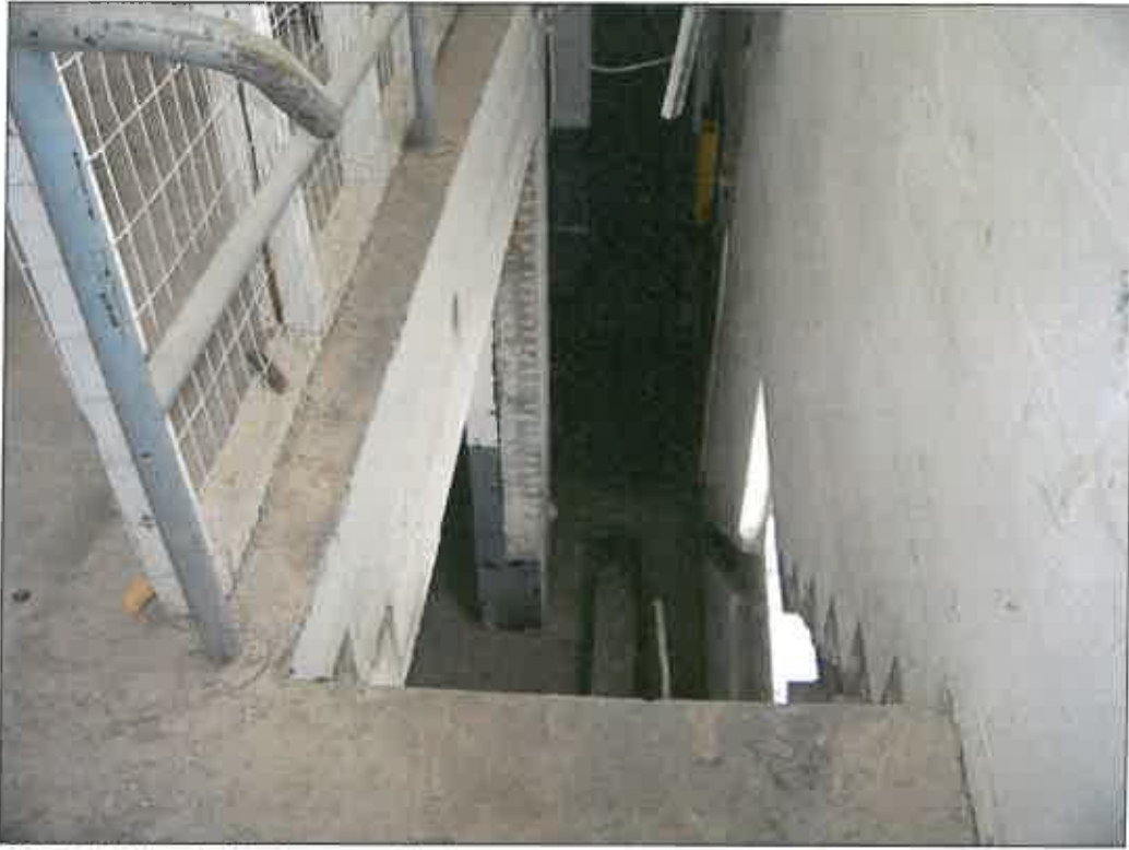
327 E. 31 st Street – interior – no stair; lack of railing
