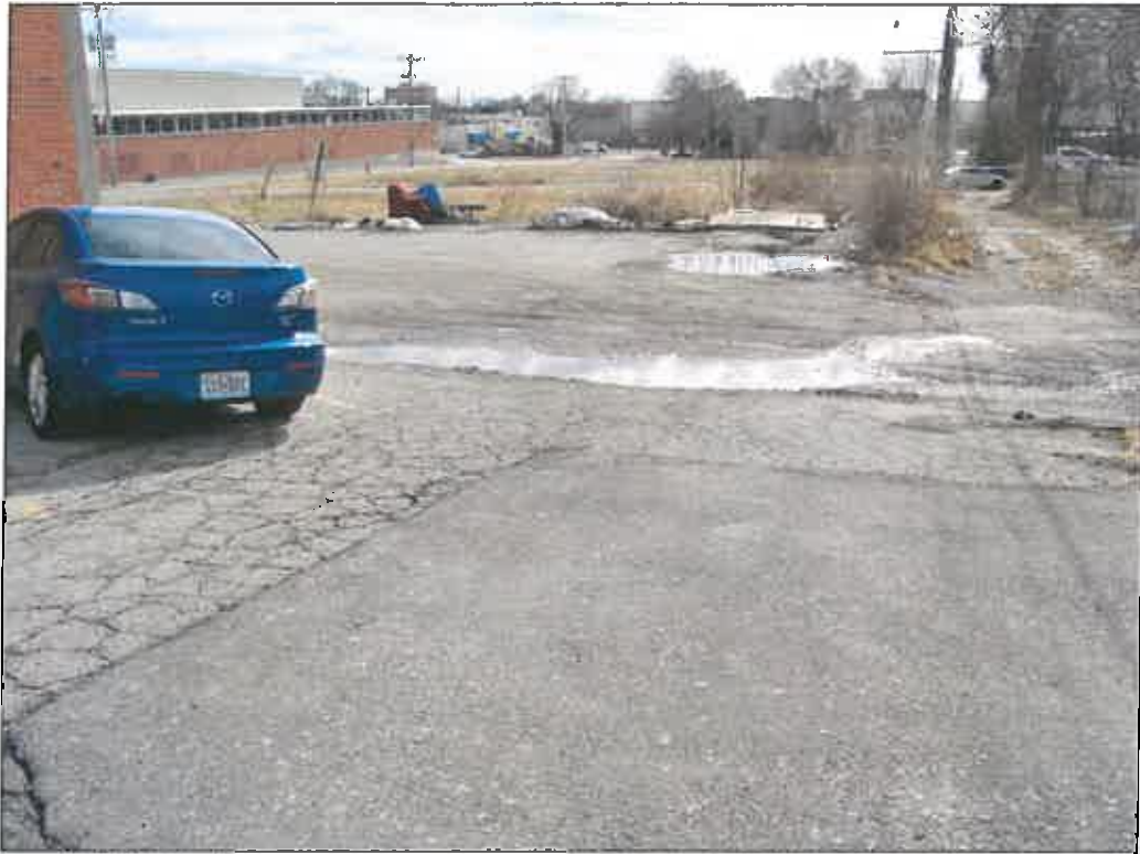
3108 Oak Street – looking south – trash/debris; overgrown vegetation; deterioration of pavement
