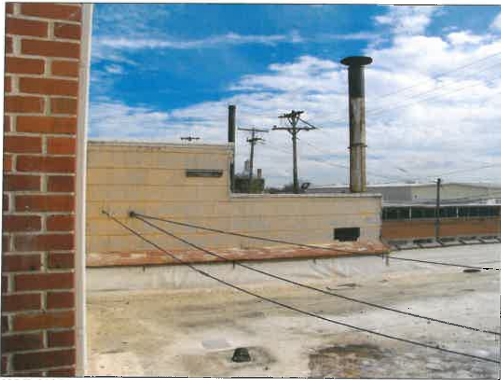
327 E. 31 st Street – looking southeast – deterioration of mechanical equipment
