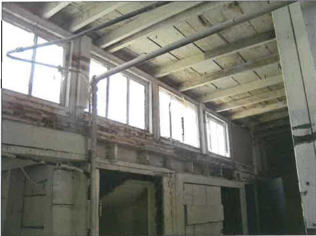
327 E. 31 st Street – interior – open, broken windows; failure of finishes
