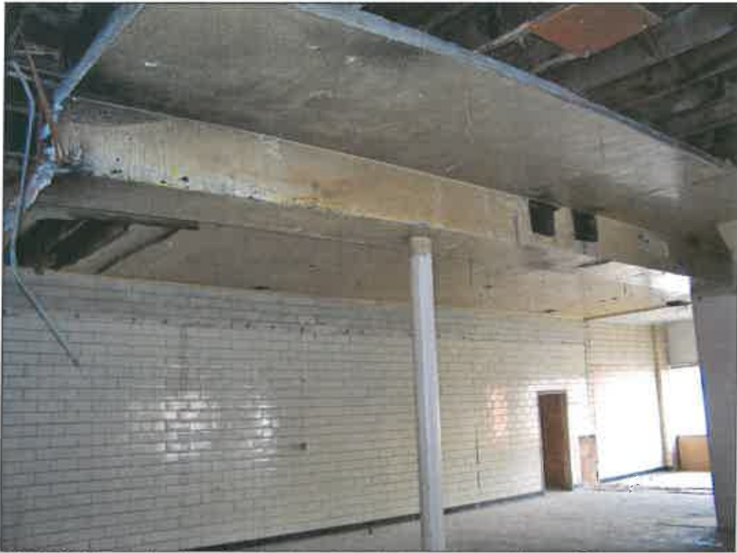
327 E. 31 st Street – interior – deterioration of mechanical system; evidence of fire
