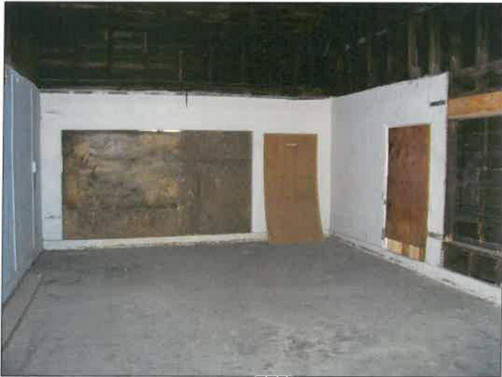
327 E. 31 st Street – interior – boarded windows; lack of power/light; water damage
