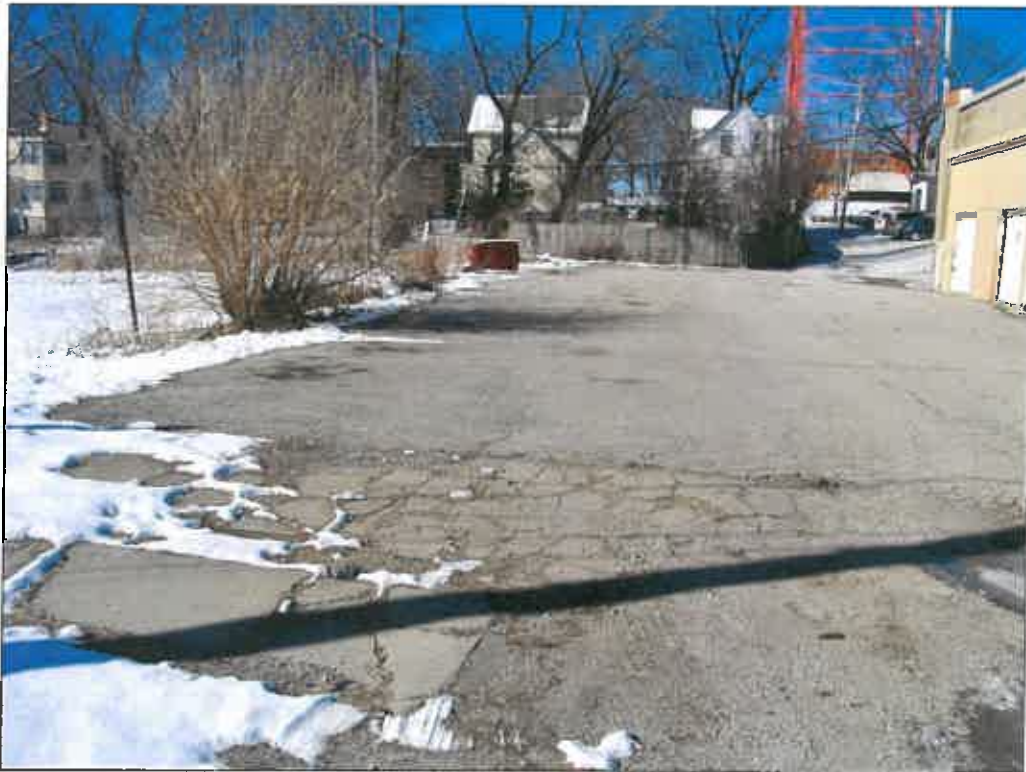
3108 Oak Street – looking west – lack of wheel stops, pavement markings, directional signage
