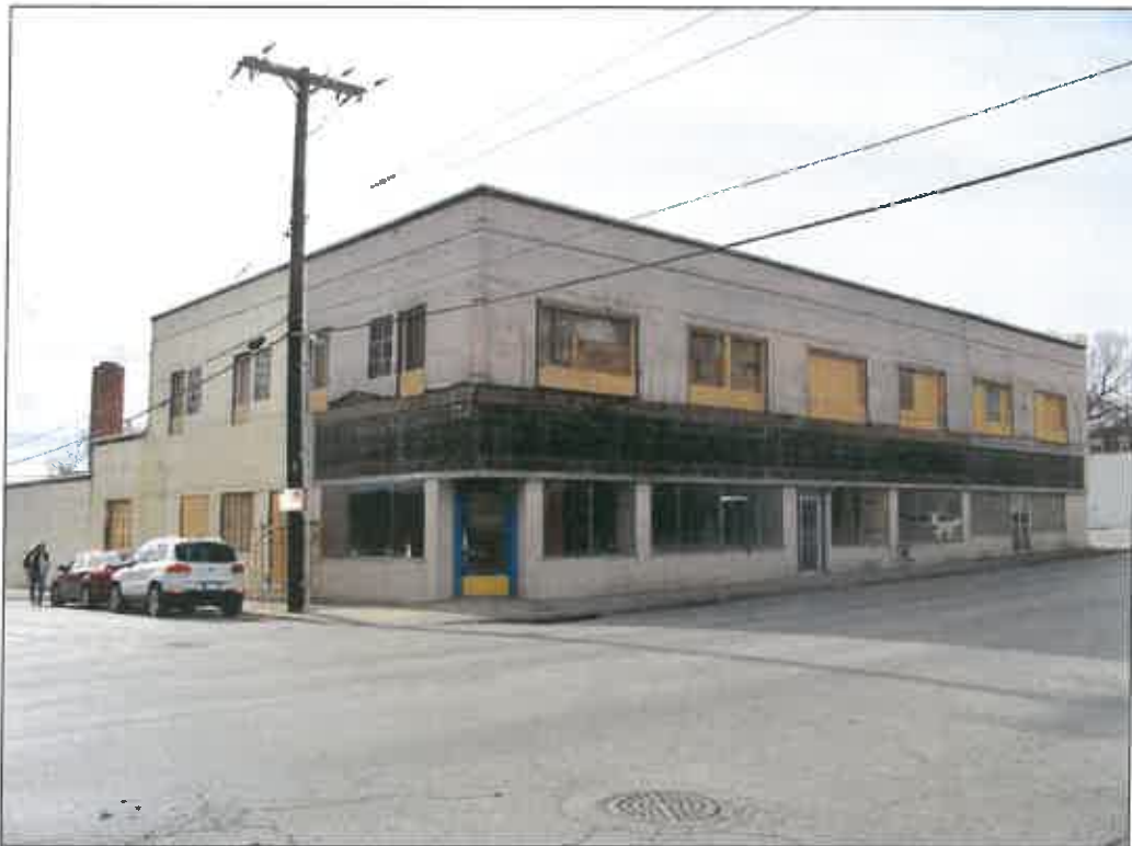
327 E. 31 st Street – looking southwest – deterioration of windows and wall veneer; failure of finishes.
