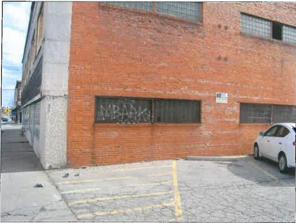
327 E. 31 st Street – looking east – graffiti; deterioration of pavement
