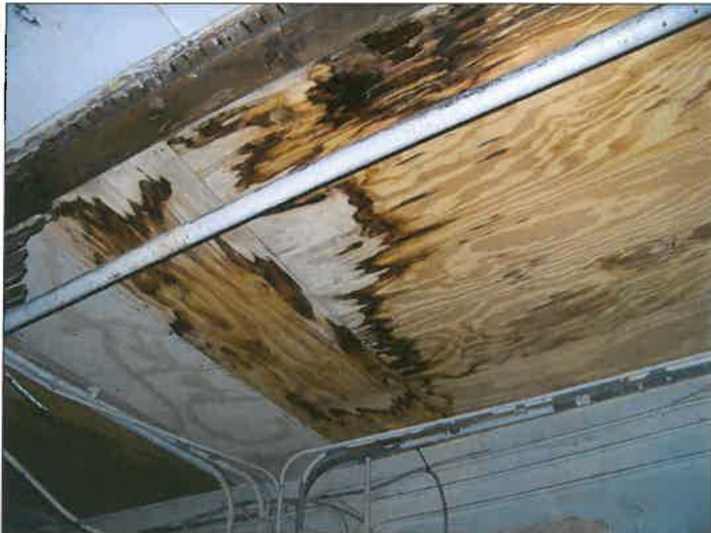
327 E. 31 st Street – interior – water damage due to leaking roof; failure of finishes
