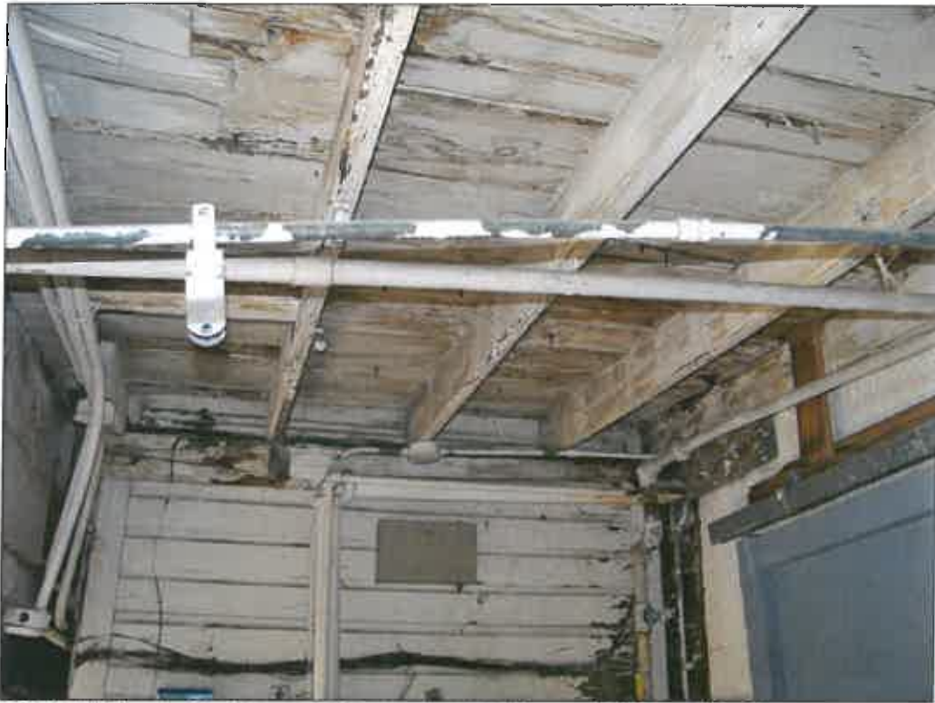
327 E. 31 st Street – interior – water damage due to leaking roof; failure of finishes
