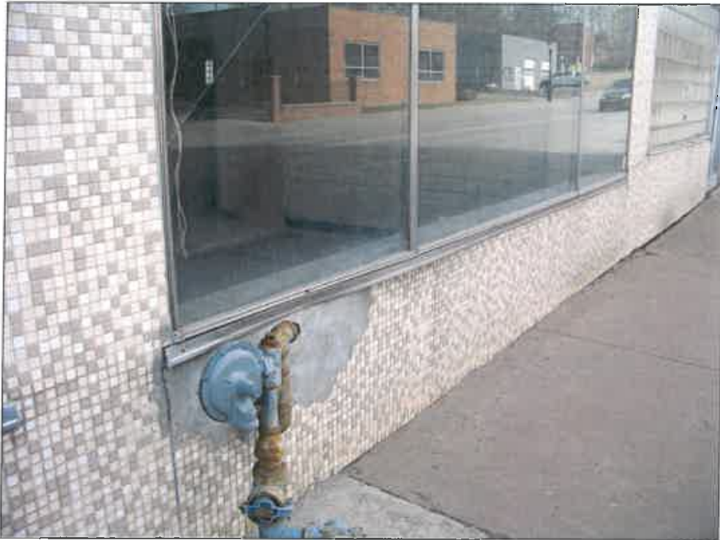
327 E. 31 st Street – looking south – deterioration of windows and wall veneer (tile); failure of finishes
