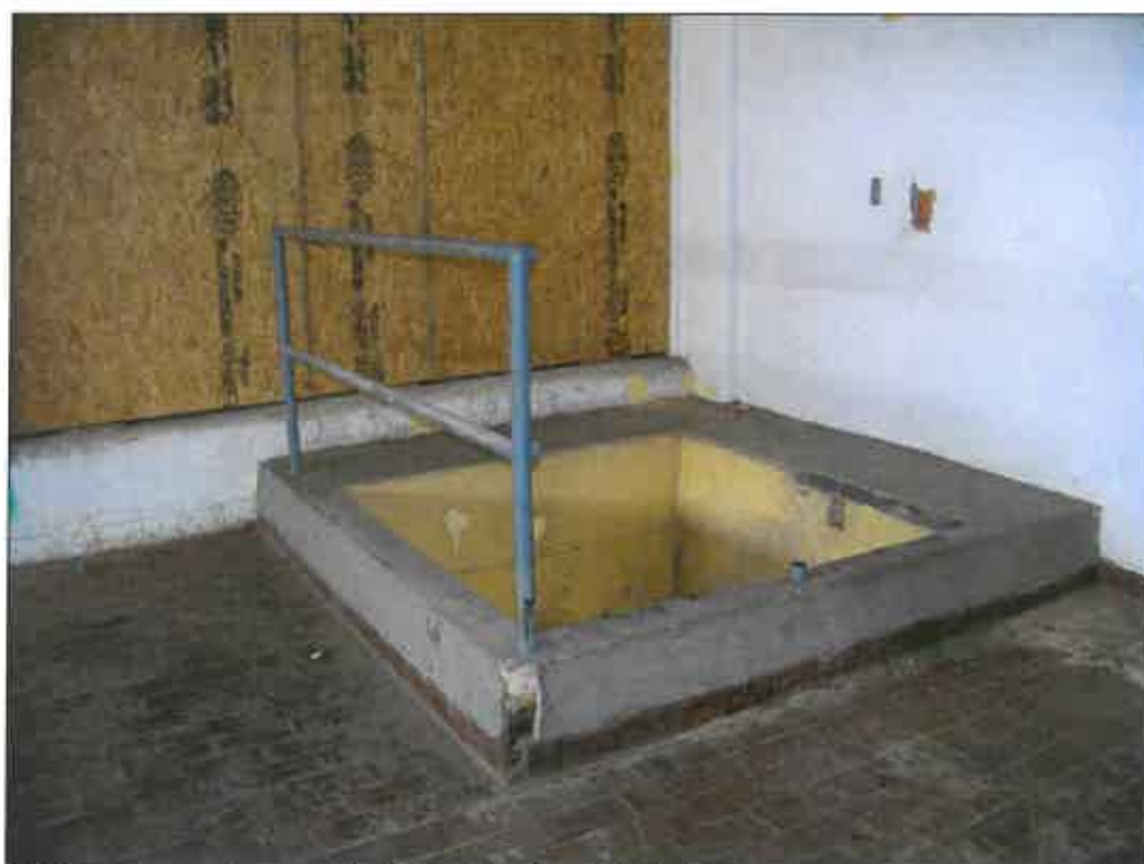
327 E. 31 st Street – interior – lack of railing; boarded window
