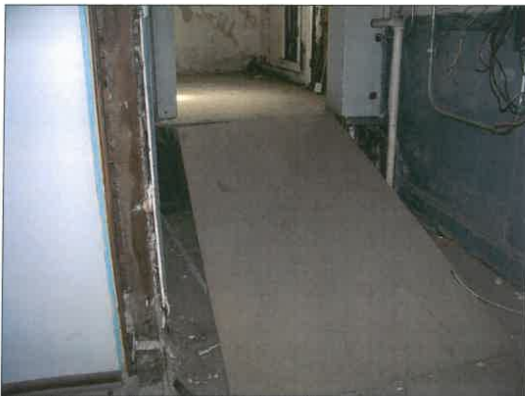
327 E. 31 st Street – interior – lack of code compliance; debris; general deterioration
