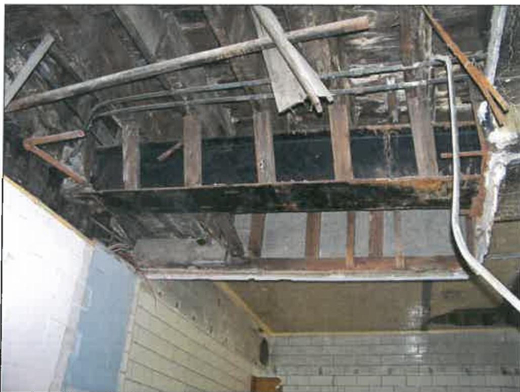
327 E. 31 st Street – interior – cracked structural beam
