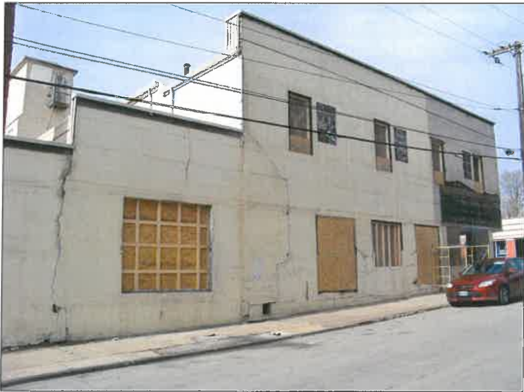
327 E. 31 st Street – looking west – deterioration of windows and wall veneer; failure of finishes
