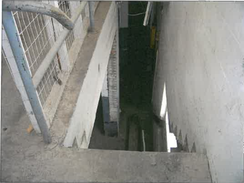
327 E. 31 st Street – interior – lack of railing, stairs
