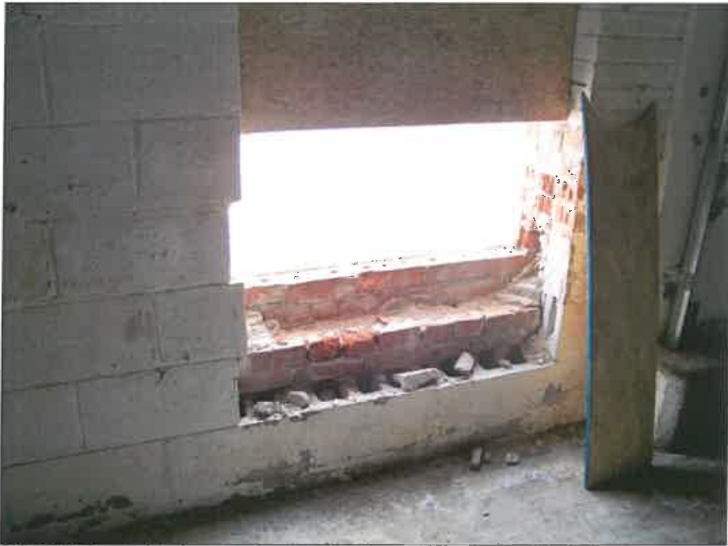
327 E. 31 st Street – interior – deterioration of wall
