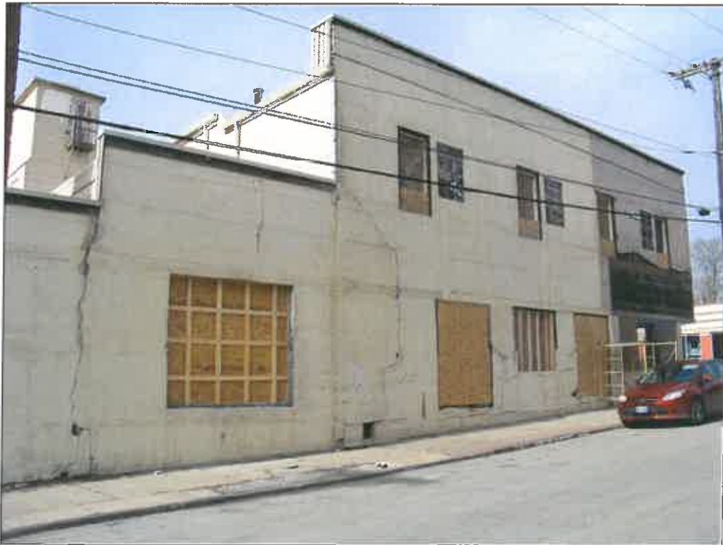
327 E. 31 st St – looking northwest – boarded windows
