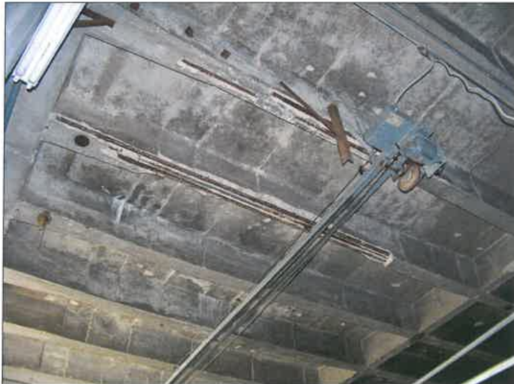
327 E. 31 st Street – interior – deterioration of structure
