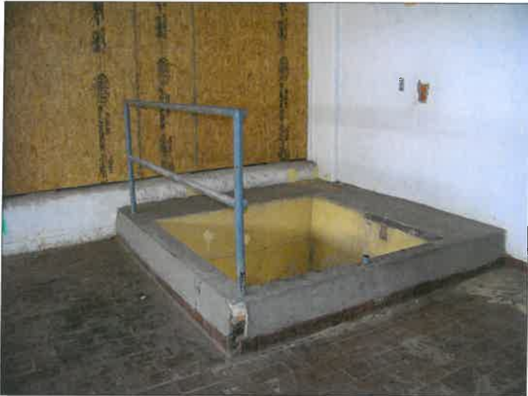
327 E. 31 st Street – lack of railing at floor opening
