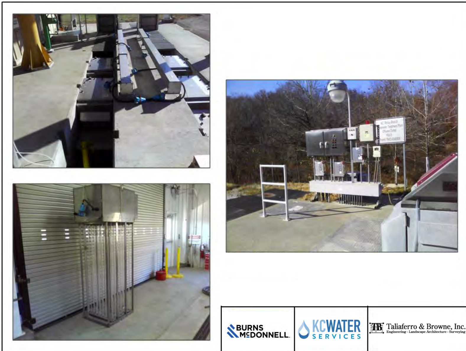
Figure 7-15: UV Disinfection System
