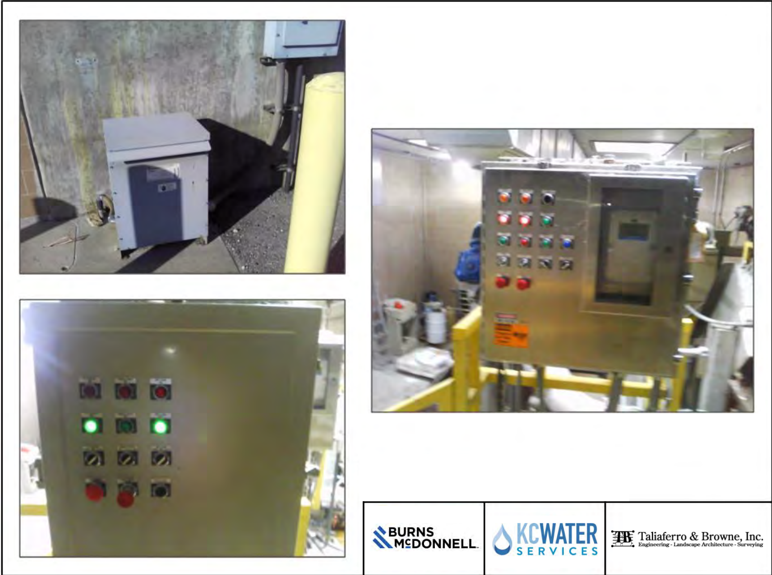
Figure 7-26: Headworks Building Electrical - Transformer T-1, Panels LCP-02-01-01 and LCP-02-01-02
