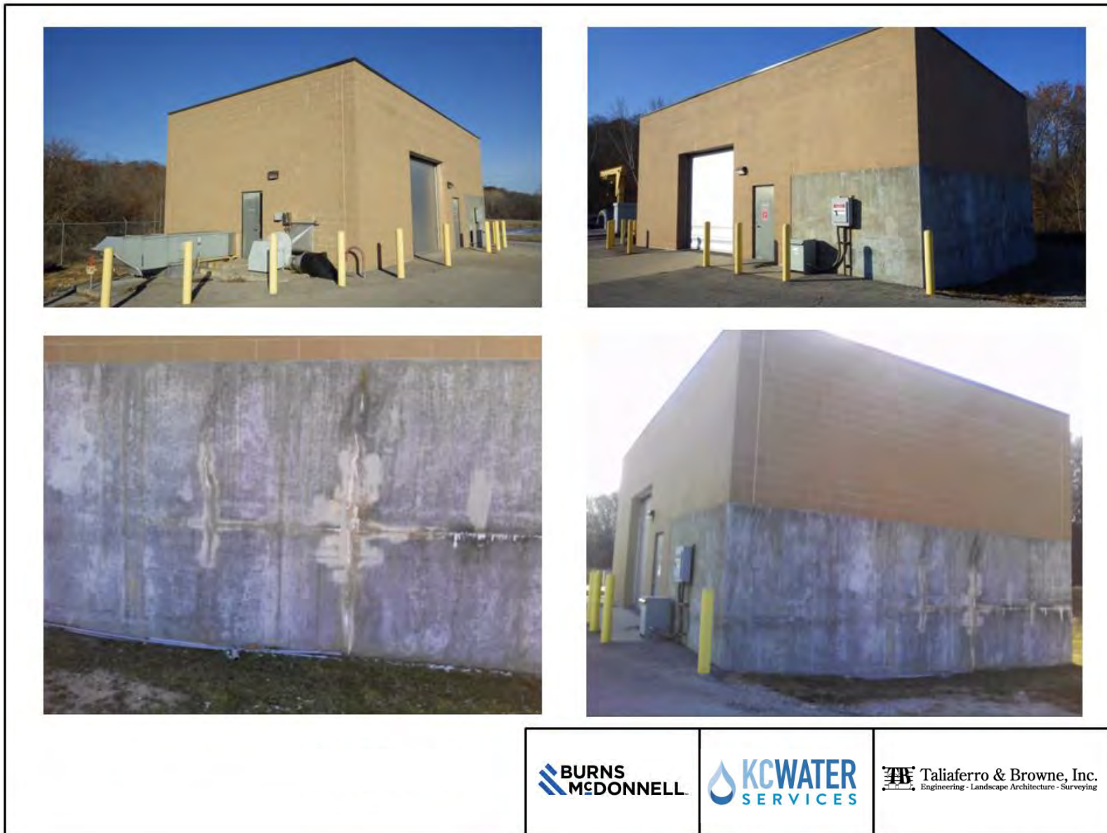
Figure 7-29: Headworks Building Structural - Chemical Degradation of the Concrete Wall -
