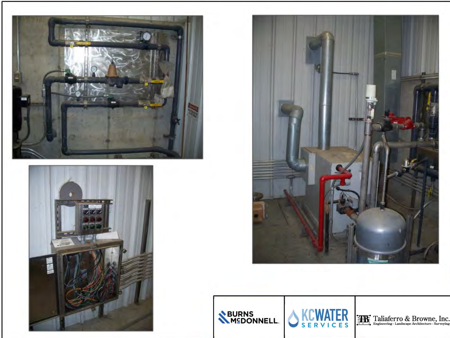
Figure 7-19: Biofilter Building HVAC Equipment
