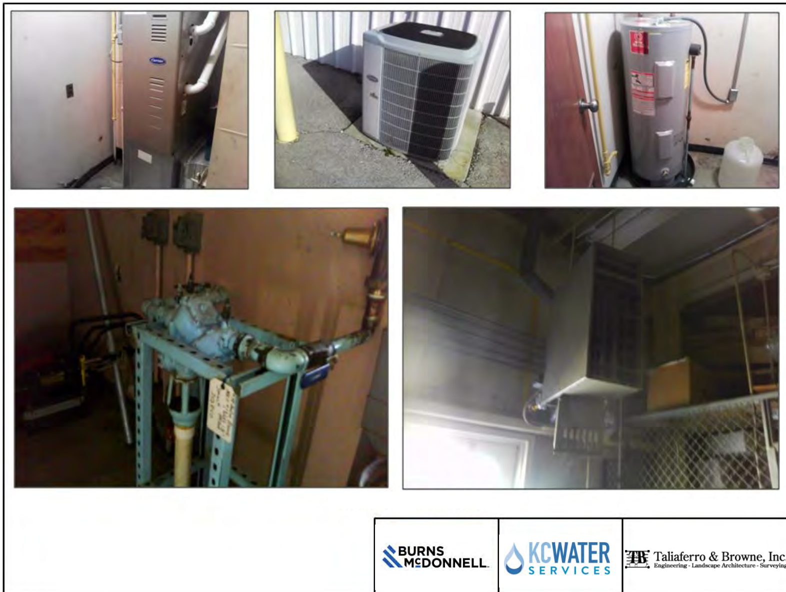
Figure 7-21: Control/Laboratory Building Mechanical Equipment
