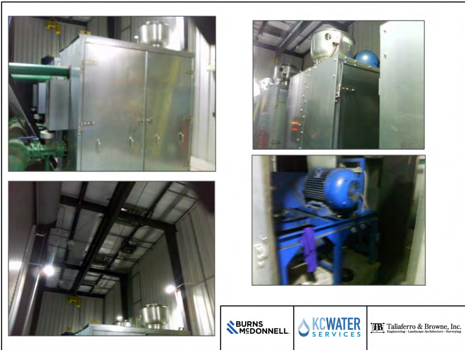
Figure 7-17: Blower Building Mechanical Equipment
