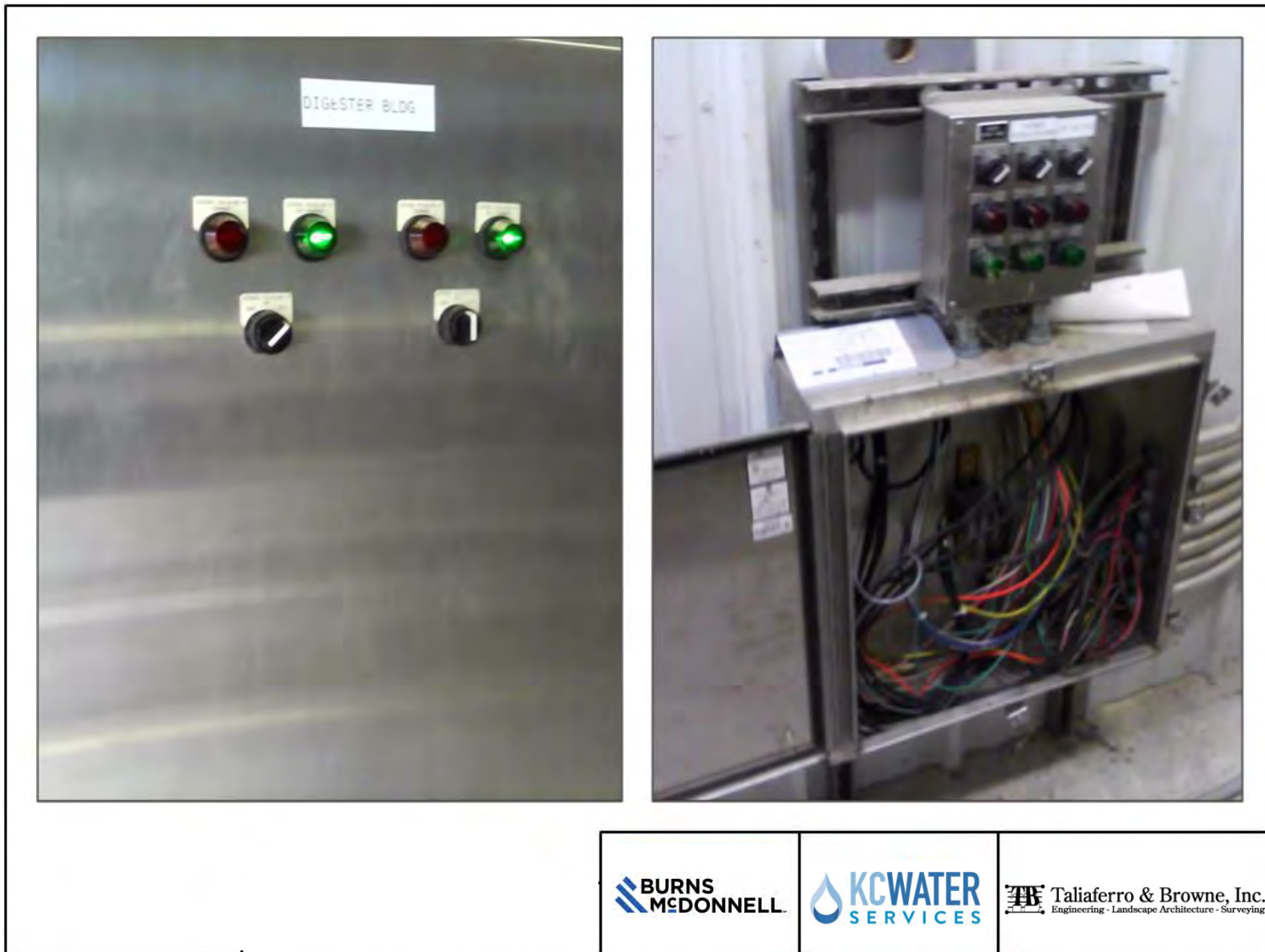
Figure 7-22: MCC-1 Building Electrical - Panels LCP-08-05-02, CP-09-01-02
