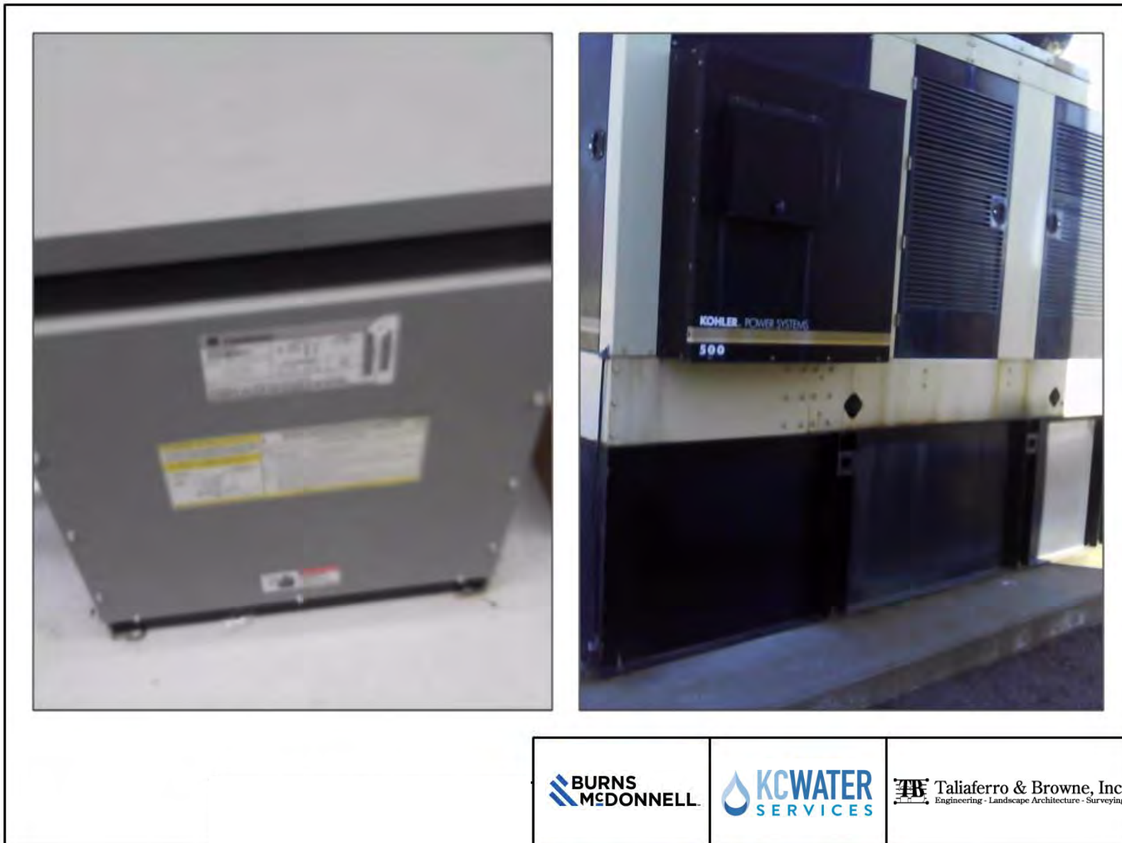
Figure 7-24: MCC-3 Building Electrical - Transformer T4, Emergency Generator
