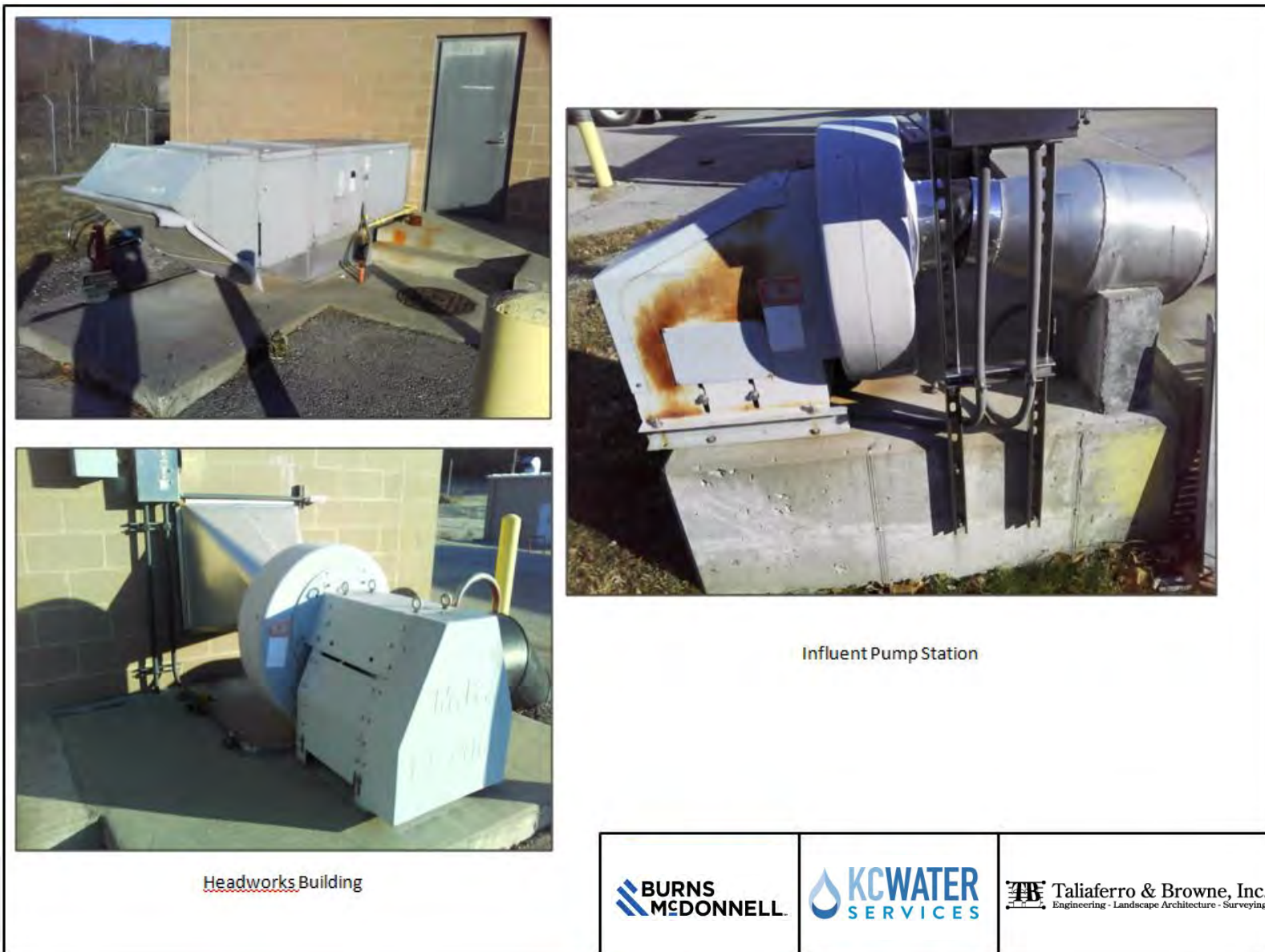
Figure 7-16: Influent Pump Station and Headworks Building HVAC Equipment
