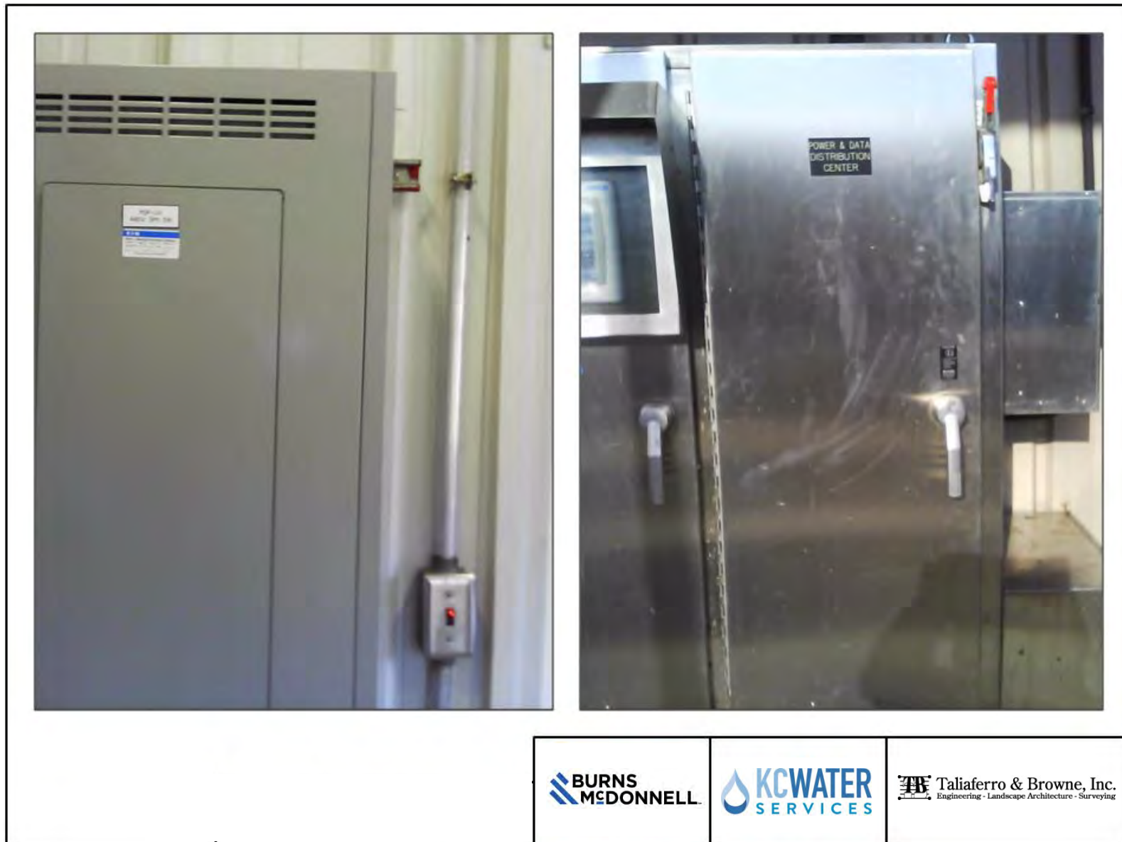
Figure 7-27: UV Disinfection Building Electrical - Panels PDP-UV and UV-PDDC
