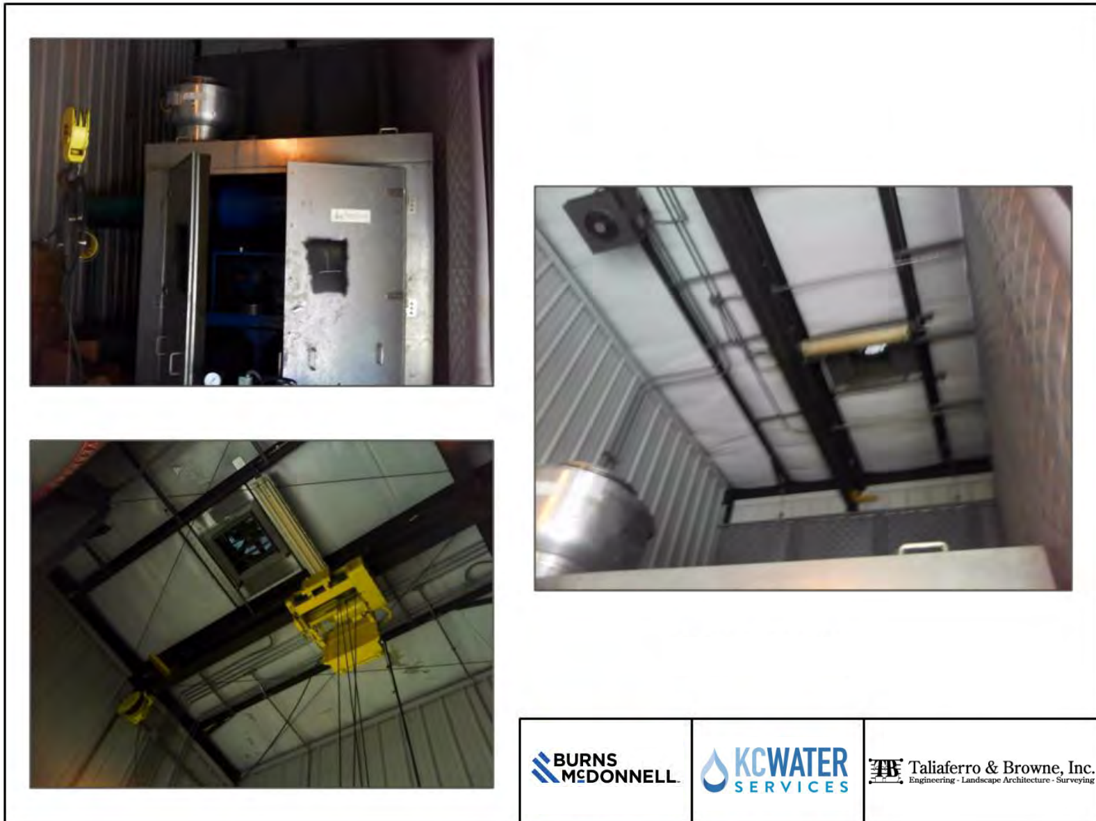
Figure 7-20: Sludge Process Building Mechanical Equipment
