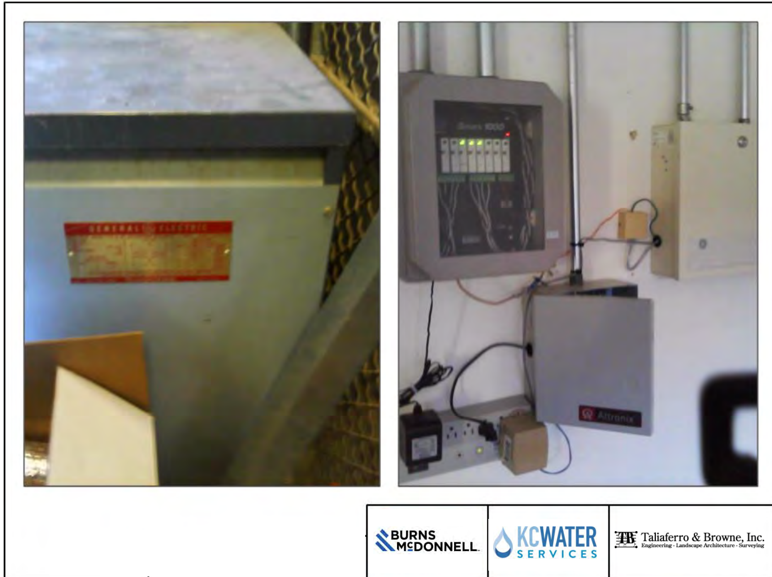
Figure 7-28: Control/Laboratory Building Electrical - Transformer T1, Security and Alarm Panel
