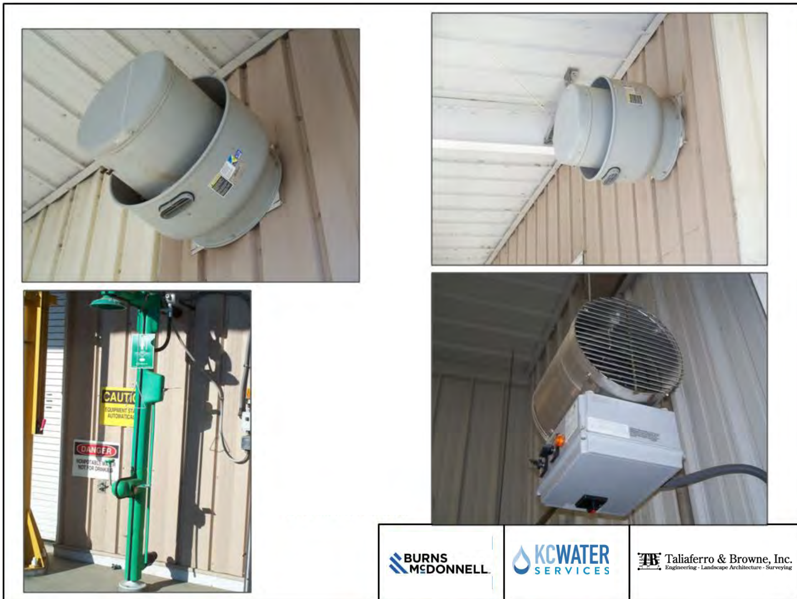
Figure 7-18: UV Disinfection Building Mechanical Equipment-
