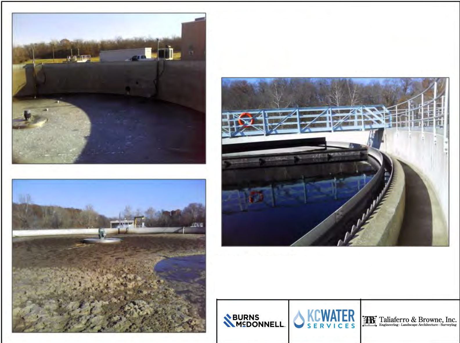
Figure 7-13: Aeration Basins and Secondary Clarifier 1
