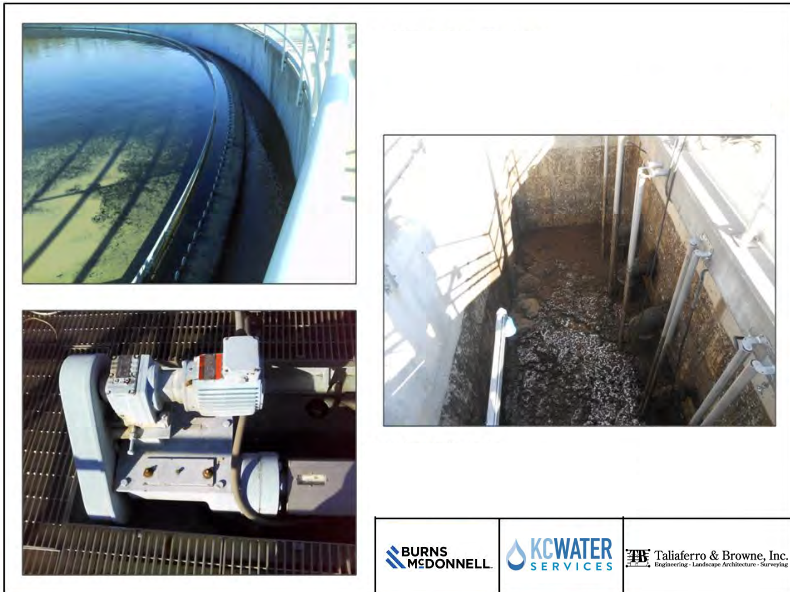
Figure 7-14: Secondary Clarifier 2 and RAS/WAS Pump Station
