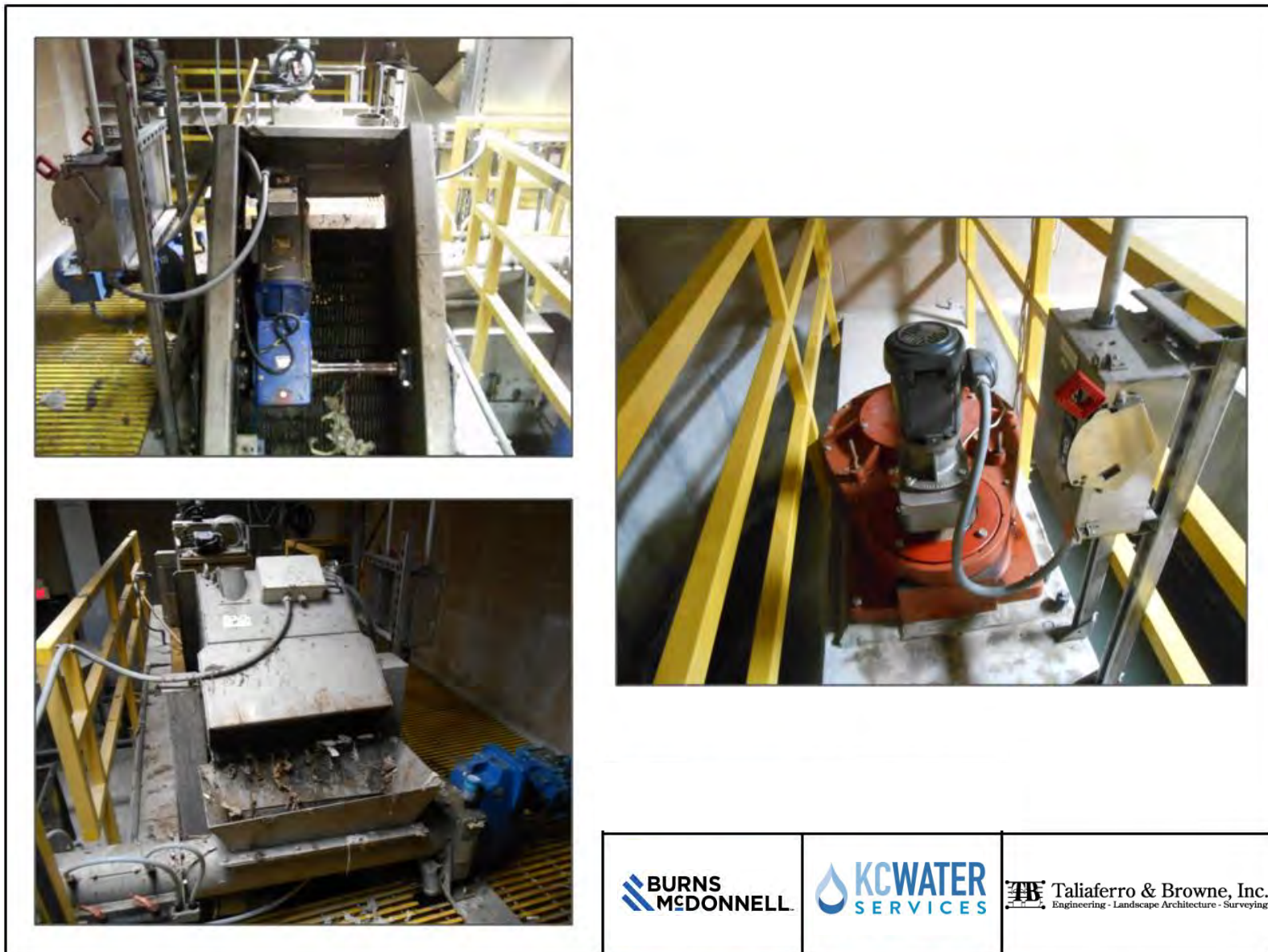
Figure 7-12: Screening and Grit Removal Process Equipment
