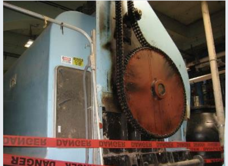
Housing for the River Intake Traveling Screens
