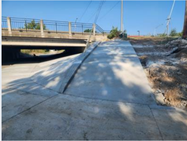
Concrete slope protection and trail replacement on the north end of the Wornall Bridge
