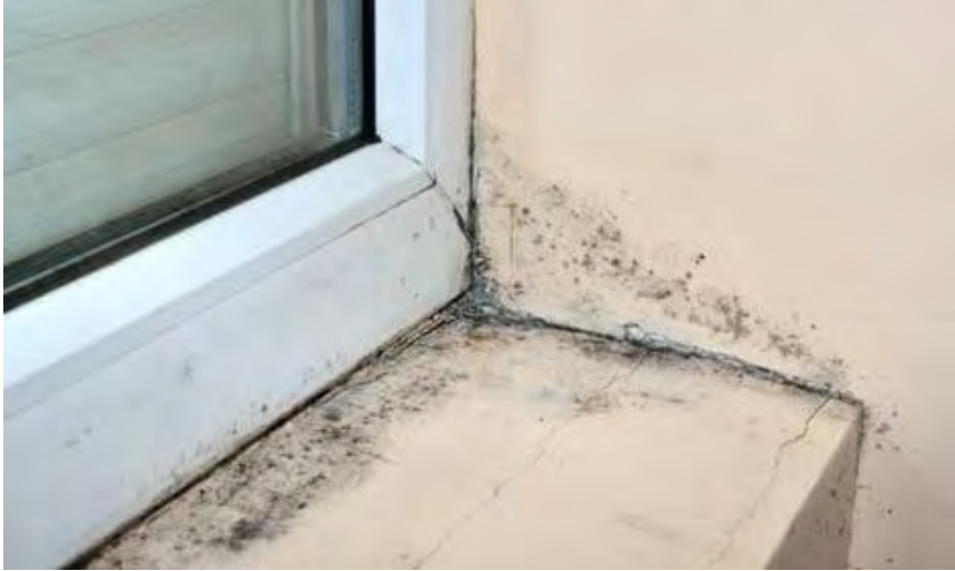
HOW WINDOW CONDENSATION CAUSES DAMAGE
