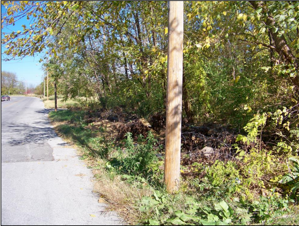
2941 – 3001 Woodland Avenue – Nonexistent pedestrian circulation, no curb and gutter; overgrown vegetation; trash/debris
