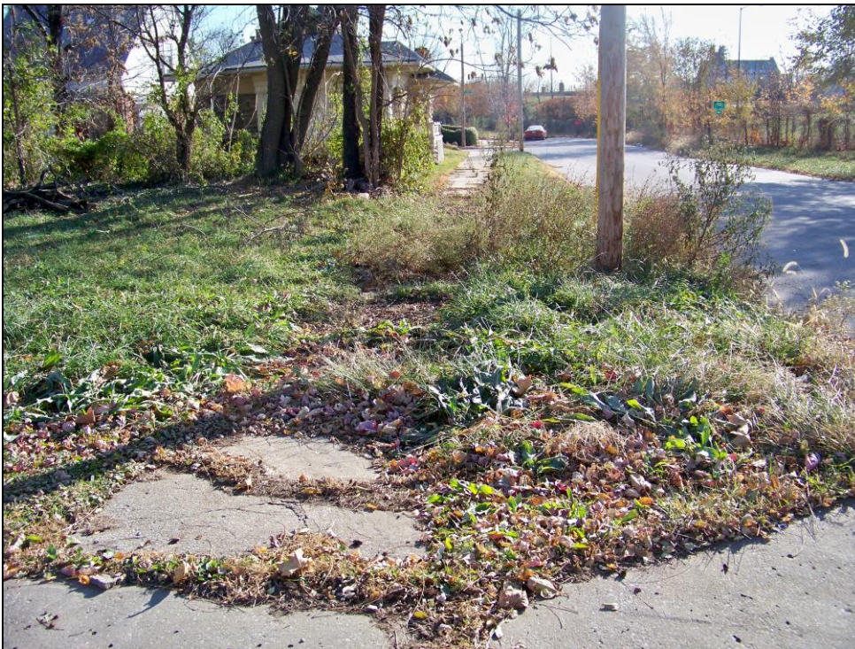
2937 Euclid Avenue – Broken/cracked sidewalk; overgrown vegetation
