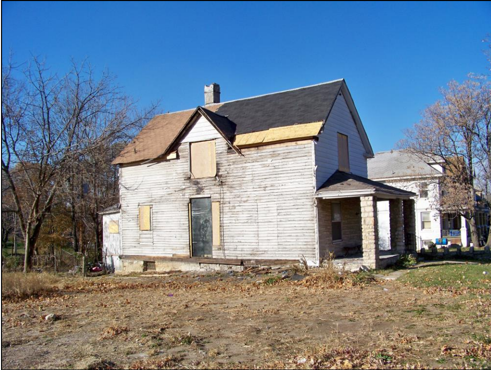
2938 Brooklyn Avenue – Deterioration of roof, walls, windows, doors, fascia/soffit, gutter/downspout; failure of exterior finishes
