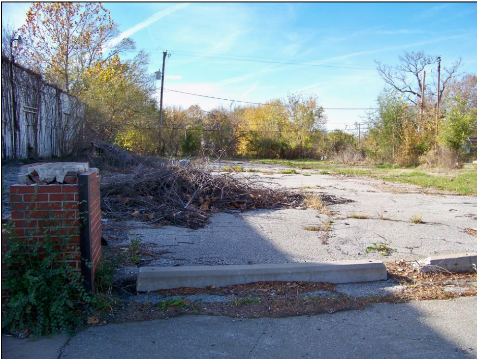
3012 Prospect Avenue – Deterioration of parking surface; trash/debris; overgrown vegetation
