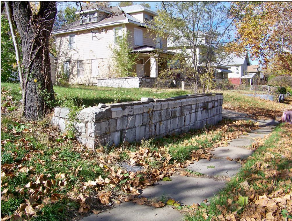
3028 Park Avenue – Deterioration of retaining wall; trash/debris; broken/cracked sidewalk
