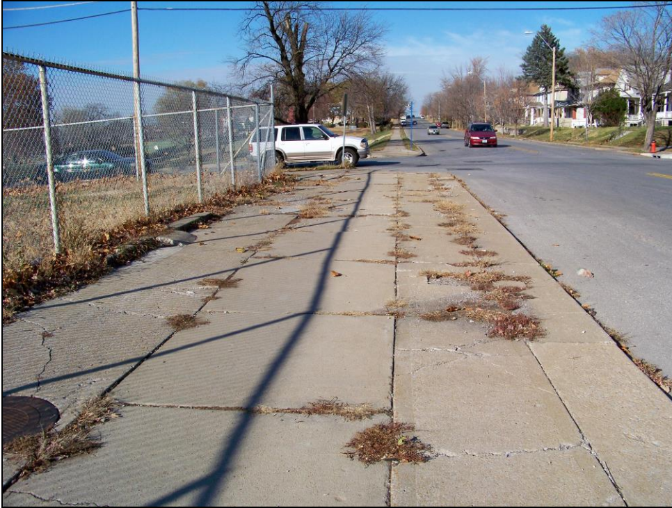
2902 Brooklyn Avenue – Broken/cracked sidewalk; overgrown vegetation
