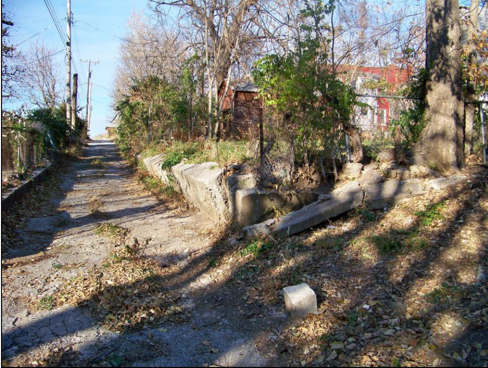
North-south Alley between 2700 block of Brooklyn Avenue and Park Avenue – Deterioration of alley, retaining wall, fence; overgrown vegetation
