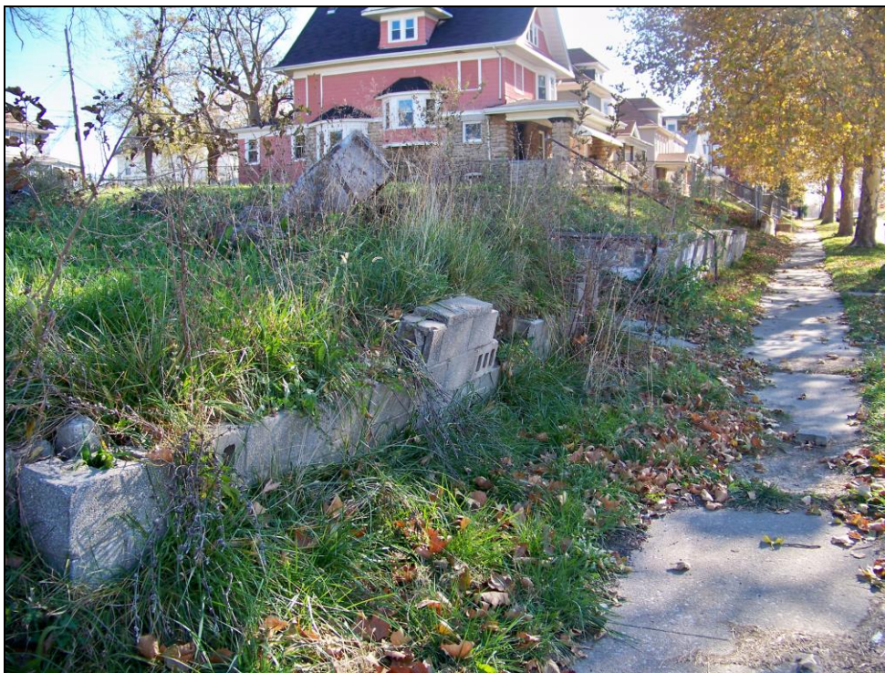
3105 Garfield Avenue – Overgrown vegetation; broken/cracked sidewalk; deterioration of retaining wall
