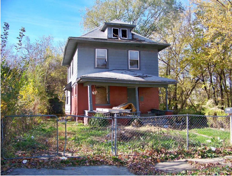
3028 Olive Street – Deterioration of roof, windows, doors; failure of finishes; trash/debris
