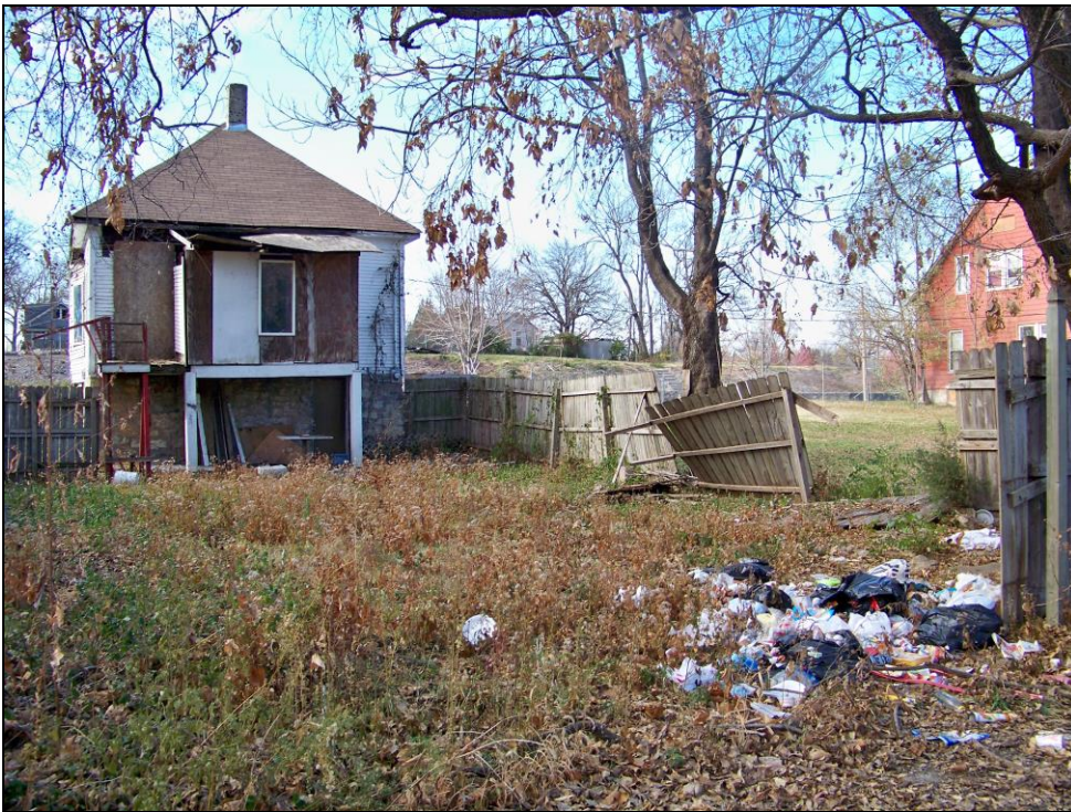
2913 Garfield Avenue –roof and wall deterioration; fascia deterioration; finishes failing; gutter and downspout deterioration; trash/debris; deterioration of fence
