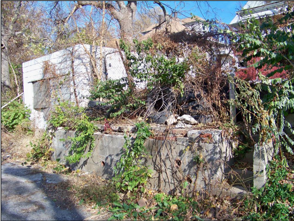
2838 Park Avenue – Trash/debris; overgrown vegetation; deterioration of retaining wall, garage
