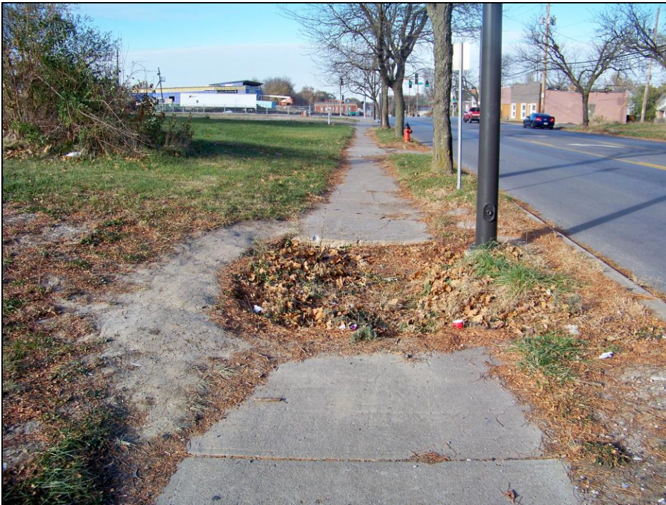
2700 block of Prospect Avenue – Deterioration of sidewalk; lack of landscaping
