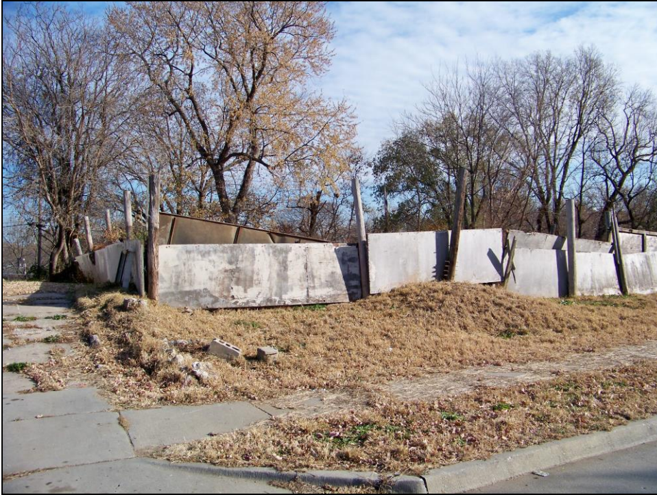
2927 Euclid Avenue – Deterioration of fence, driveway
