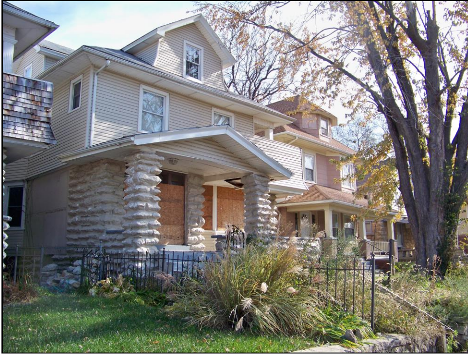
2805 Brooklyn Avenue – Inadequate lot size (narrow lot)
