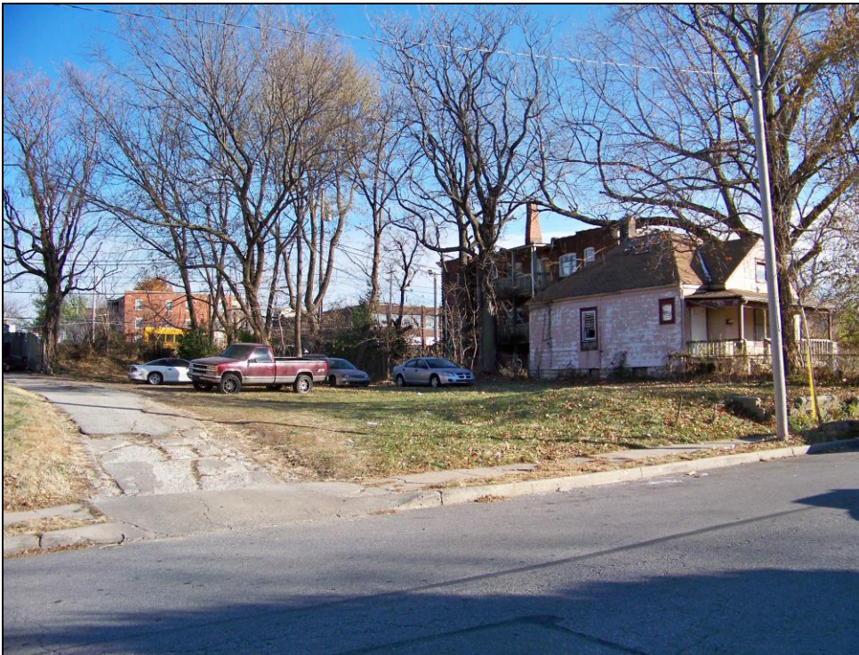
2935 Wabash Avenue – Improper parking surface; deterioration of driveway, parking surface
