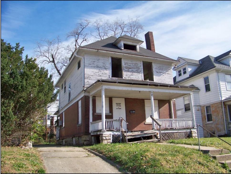
2841 Brooklyn Avenue – Deterioration of roof, steps, windows, doors: failure of finishes
