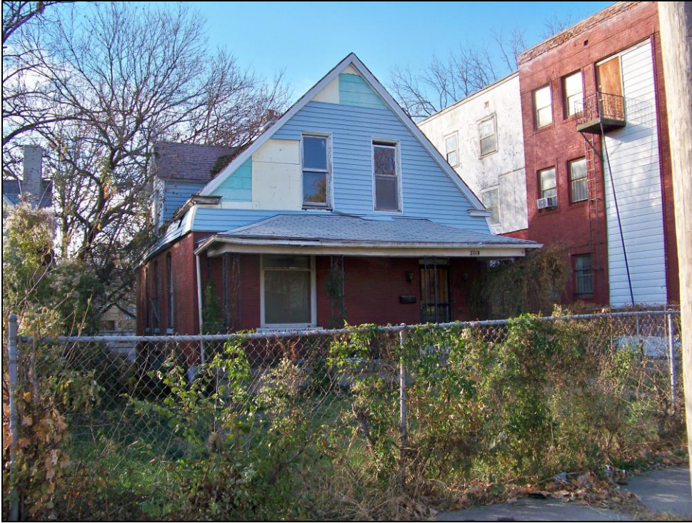
2718 Olive Street – Deterioration of roof, siding, windows, fence; overgrown vegetation
