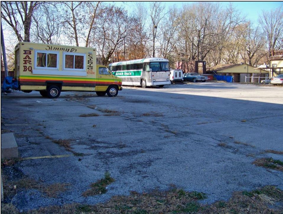
2920 Prospect Avenue – Deterioration of parking surface
