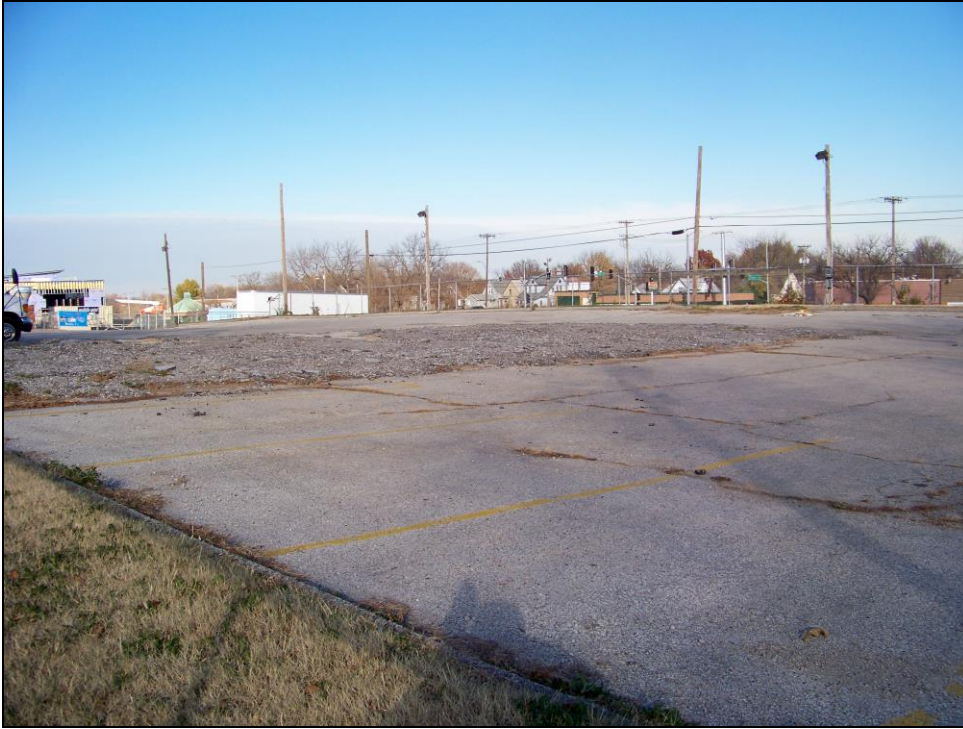
2725 Wabash Avenue – Deterioration of parking surface
