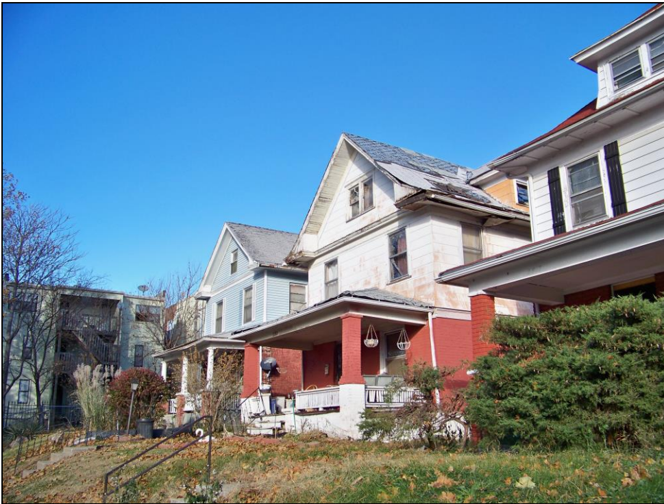
2815 Wabash Avenue – Deterioration of roof, soffit; failure of finishes
