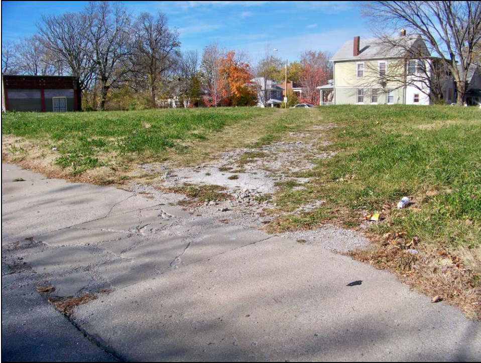
2202 E. 31 st Street – Poor vehicular access; deterioration of drive
