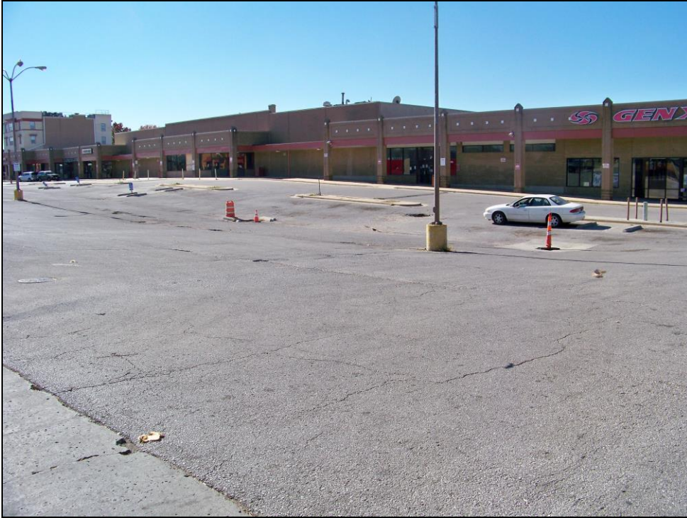
3110 Prospect Avenue – Deterioration of parking surface
