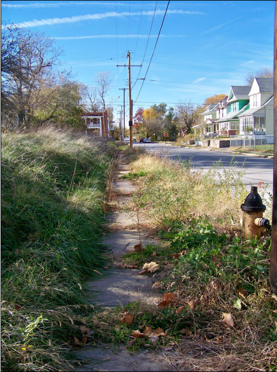
3000 Park Avenue – Cracked or uneven sidewalk; overgrown vegetation
