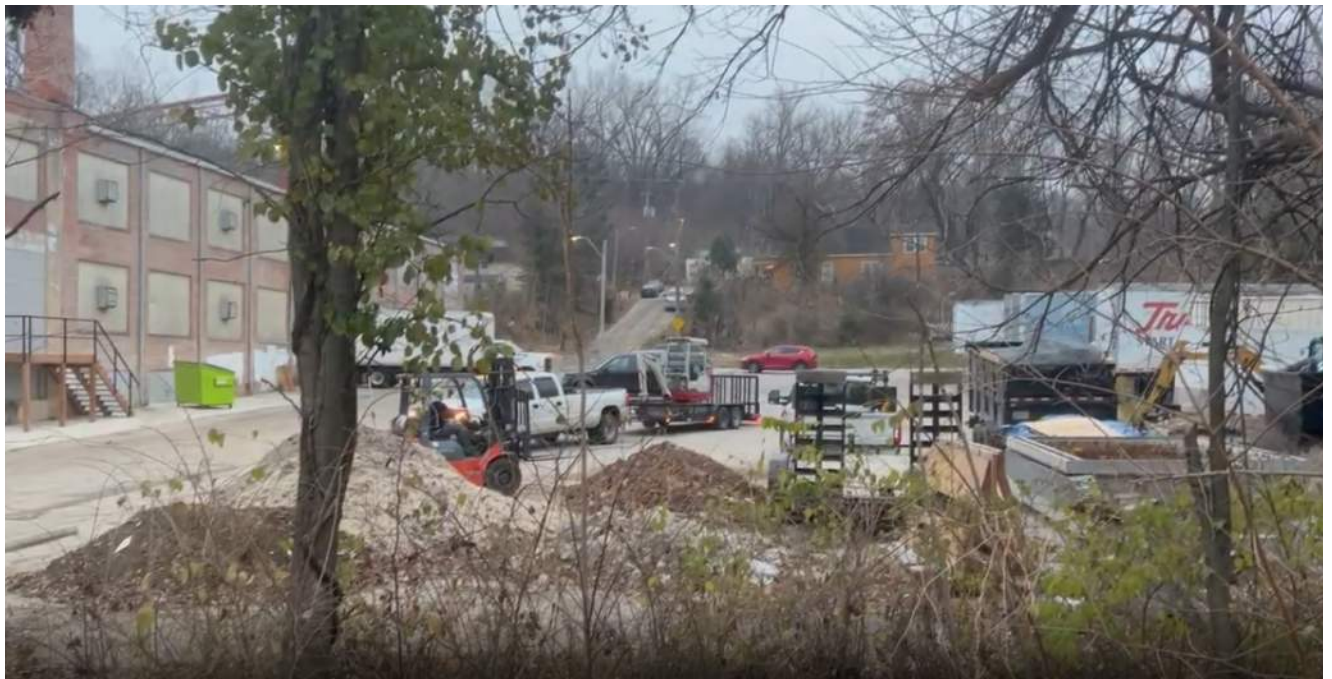
2/20/26 1:00PM; 12/12/25 7:32AM: Select examples of dumping construction debris on site.
