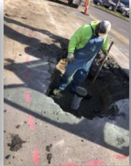
Adjusting a Valve Standpipe
