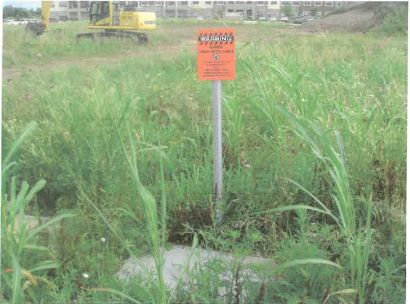
Photo 14 - Fiber optic cable located along southern utility easement.
