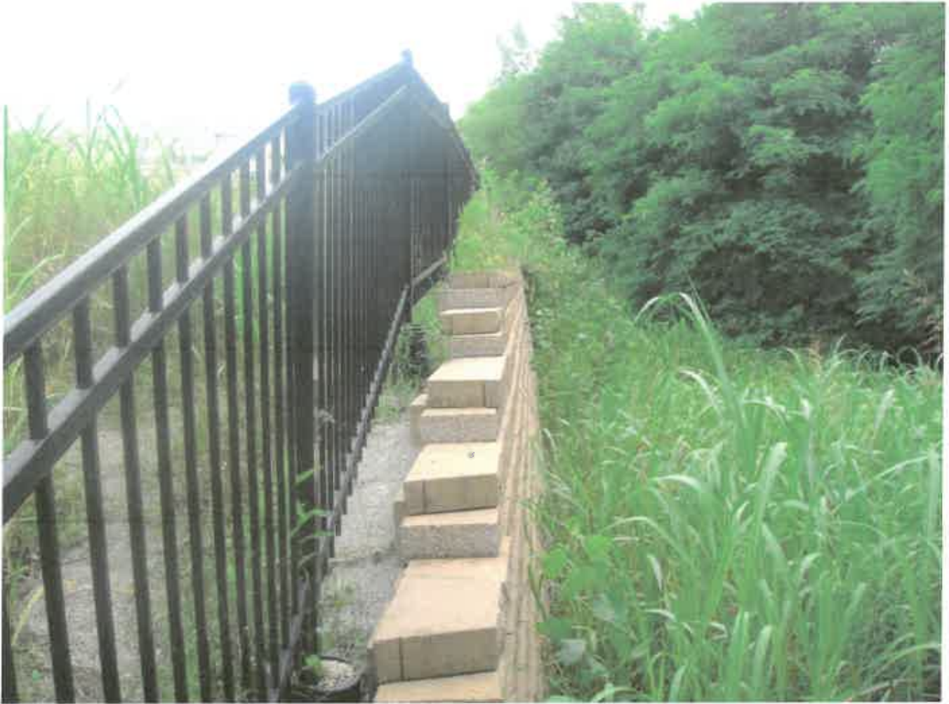
Photo 7 - Retaining wall along eastern property boundary. Wall is approximately 20' in height at this location.
