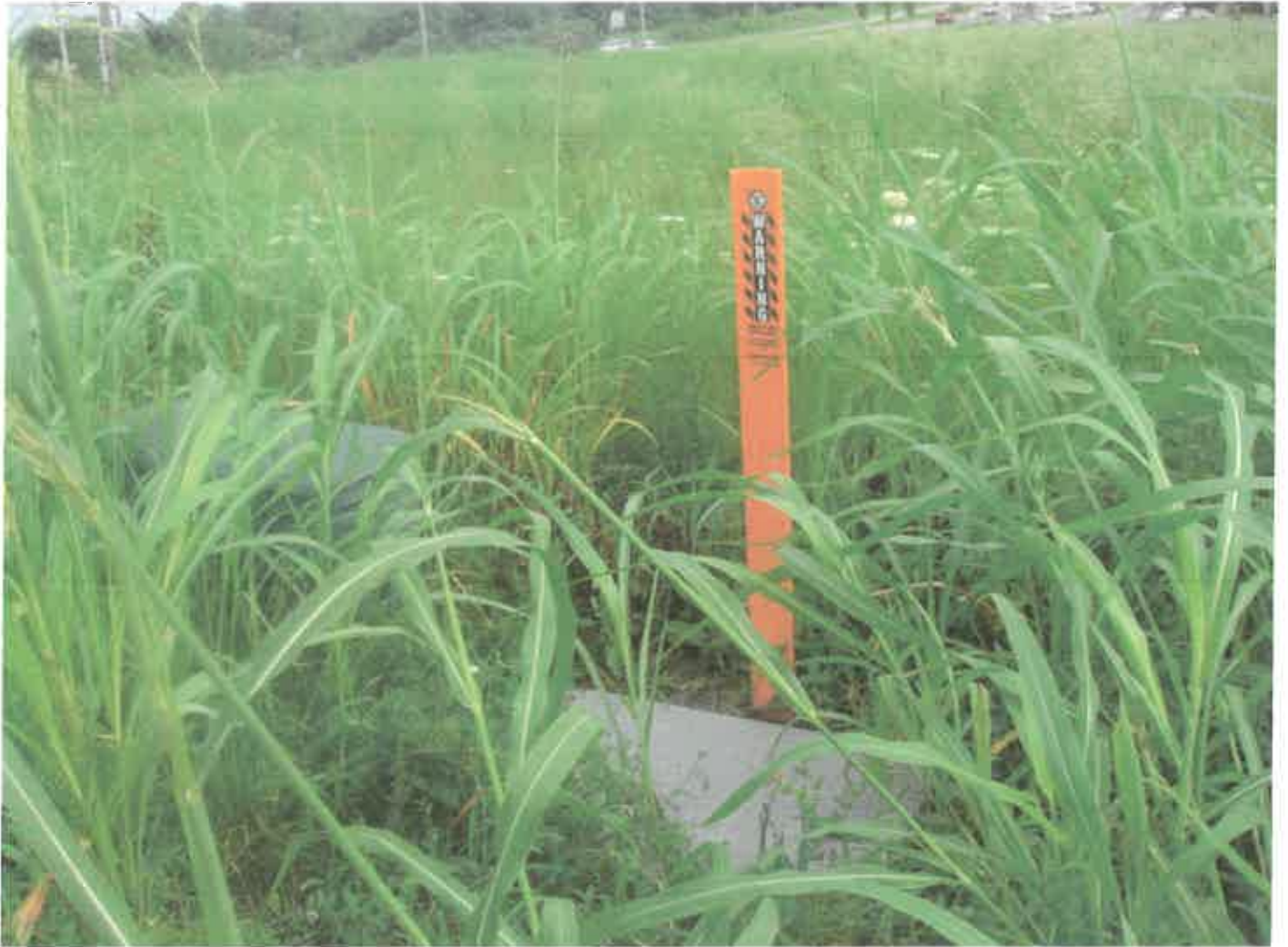
Photo 15 - Utility infrastructure located along southern utility easement.
