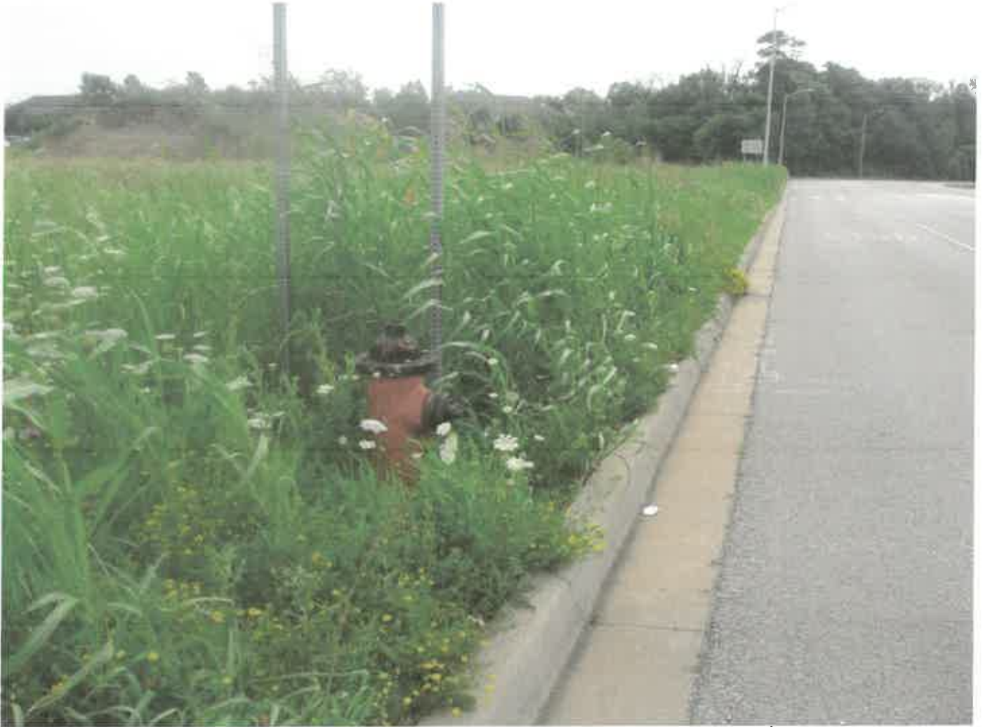
Photo 16 - Fire hydrant located along southern utility easement. NW 88 th Street to right.
