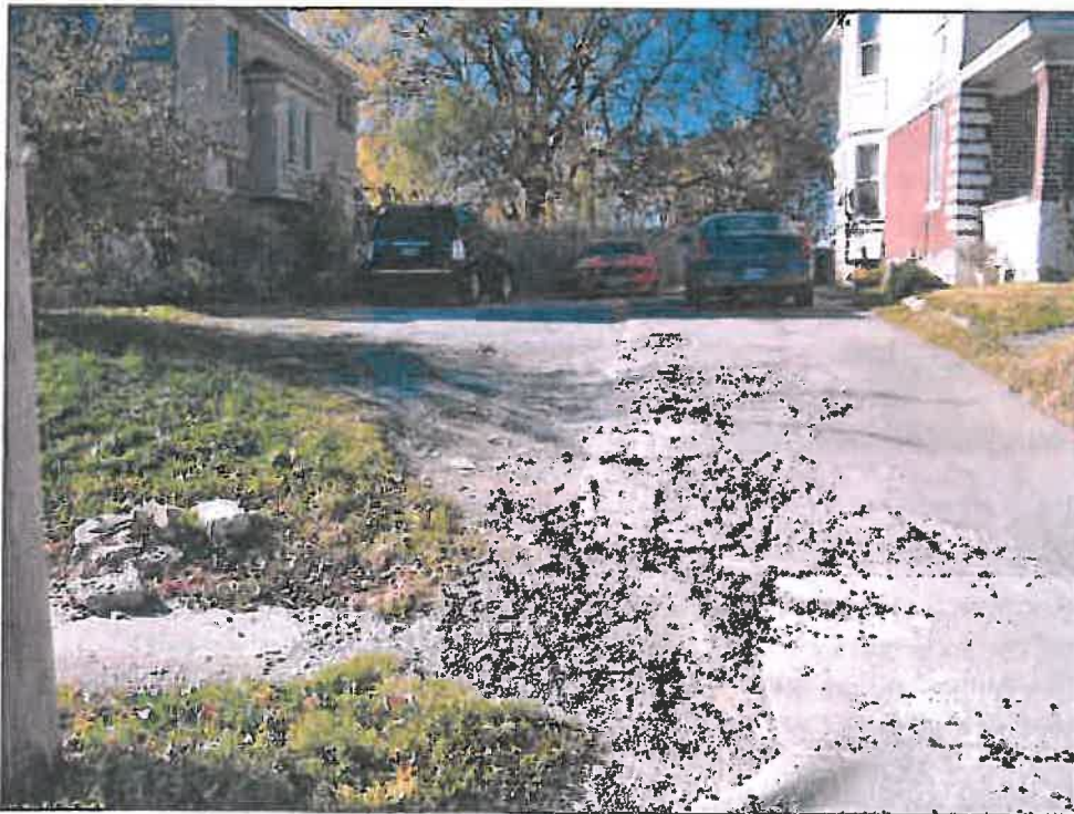
3116 Brooklyn Avenue – Deterioration of parking surface and driveway, sidewalk
