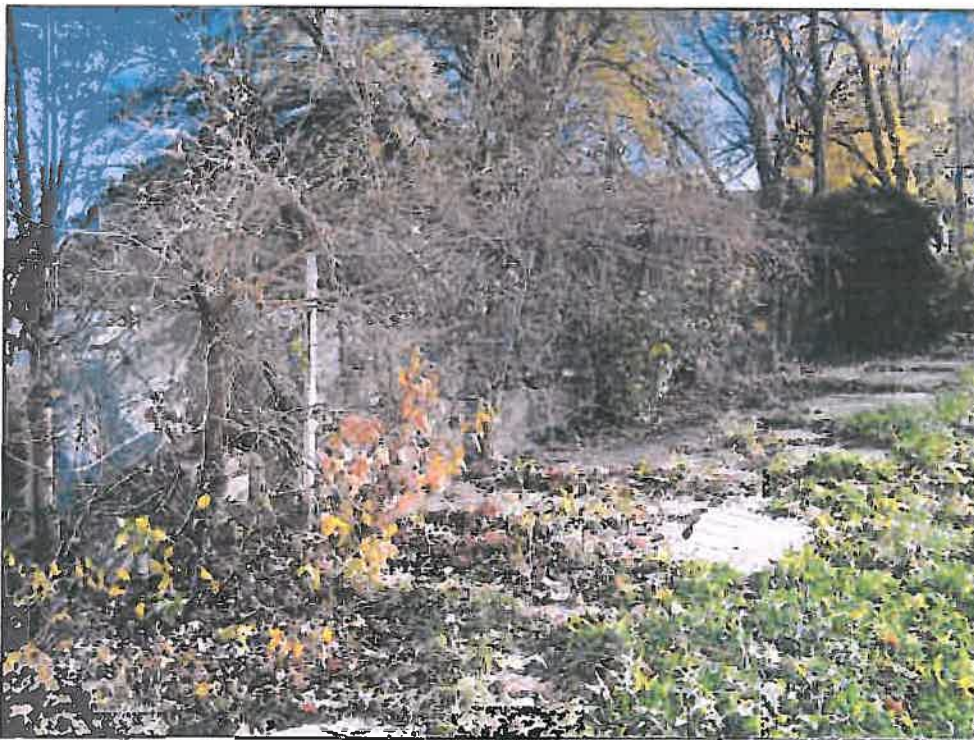
2209 E. 30 th Street – Overgrown vegetation; deteriorated driveway and fence
