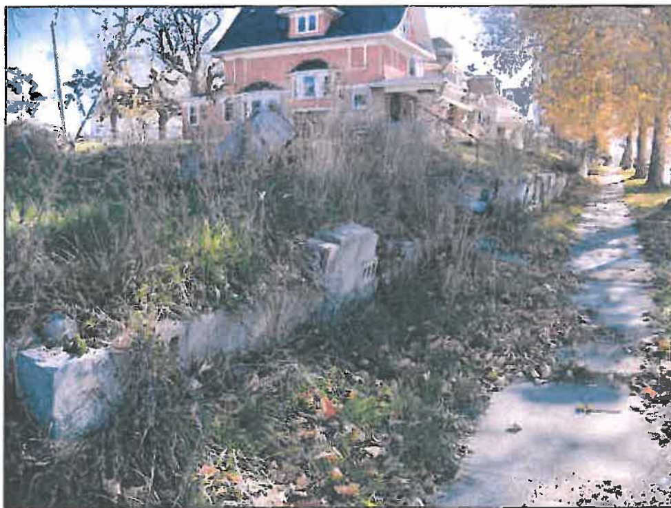
3105 Garfield Avenue – Overgrown vegetation; broken/cracked sidewalk; deterioration of retaining wall
