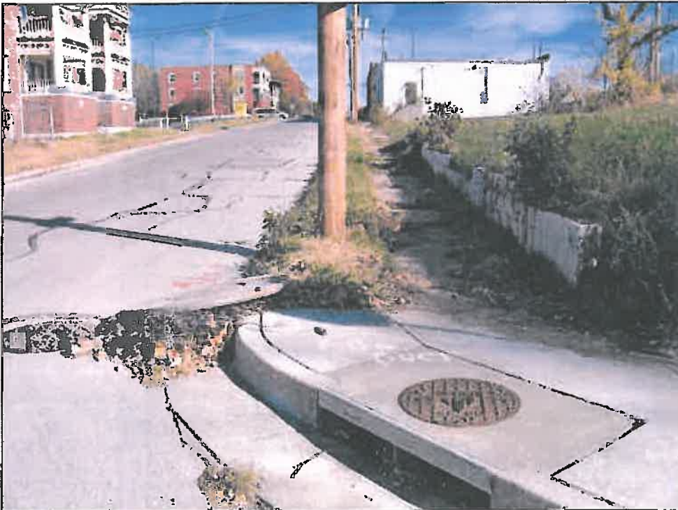
2501 E. 30 th Street – Broken/cracked sidewalk; overgrown vegetation; deterioration of retaining wall
