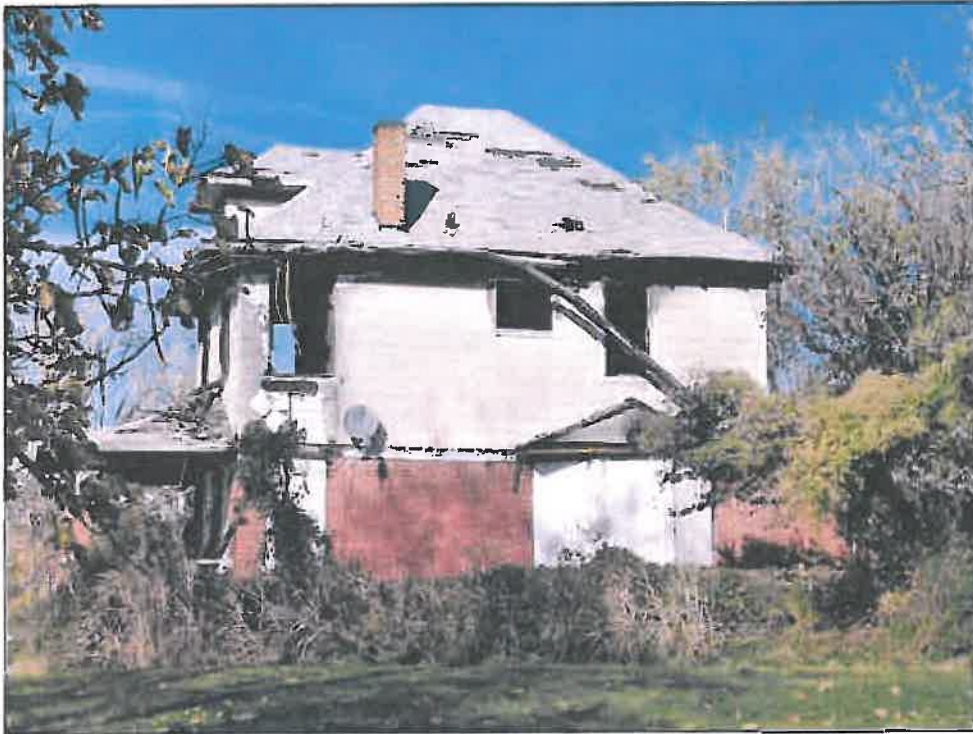
3015 Wabash Avenue – wall/siding and roof deterioration; window deterioration; fascia deterioration; finishes failing; debris
