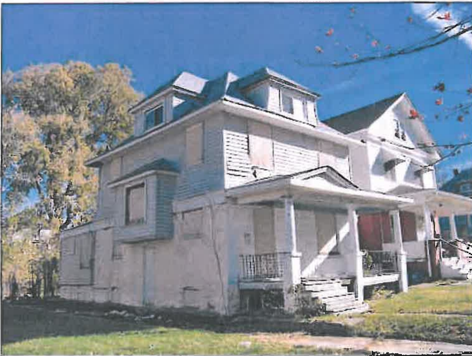
3021 Olive Street – Deterioration of windows, doors, siding; overgrown vegetation
