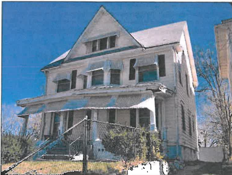
3121 Woodland Avenue – Deterioration of roof, fascia/soffit, awnings, retaining wall, driveway
