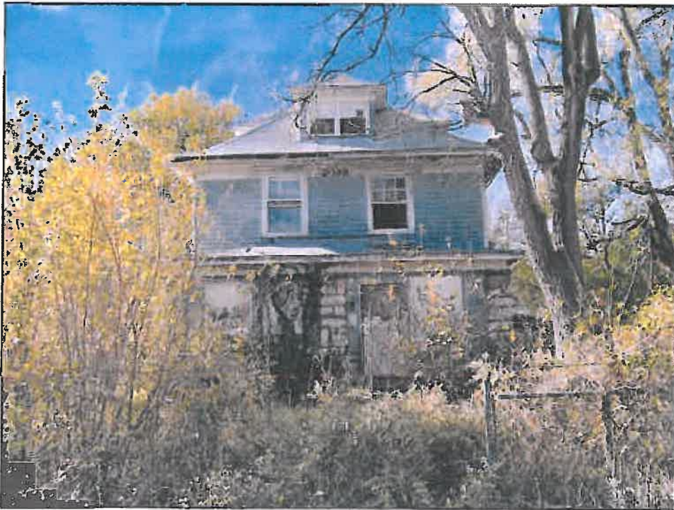
3036 Olive Street – Deterioration of roof, windows, walls/siding; doors; finishes failing; weeds
