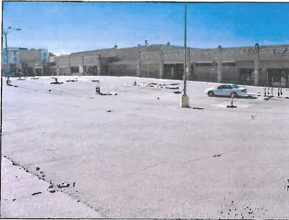
3110 Prospect Avenue – Deterioration of parking surface
