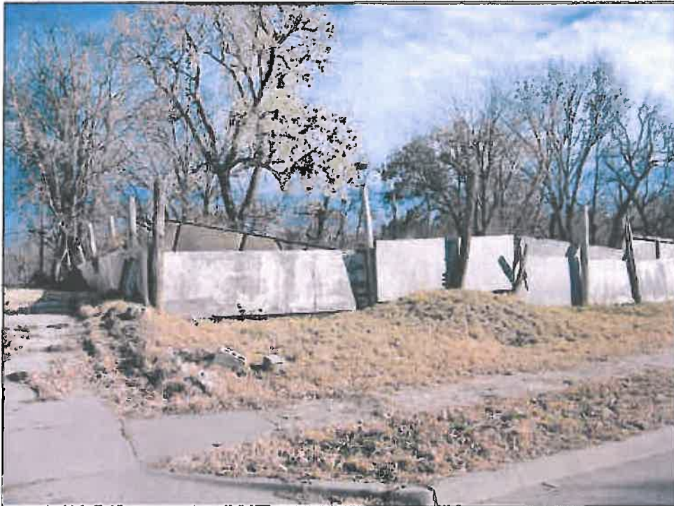
2927 Euclid Avenue – Deterioration of fence, driveway
