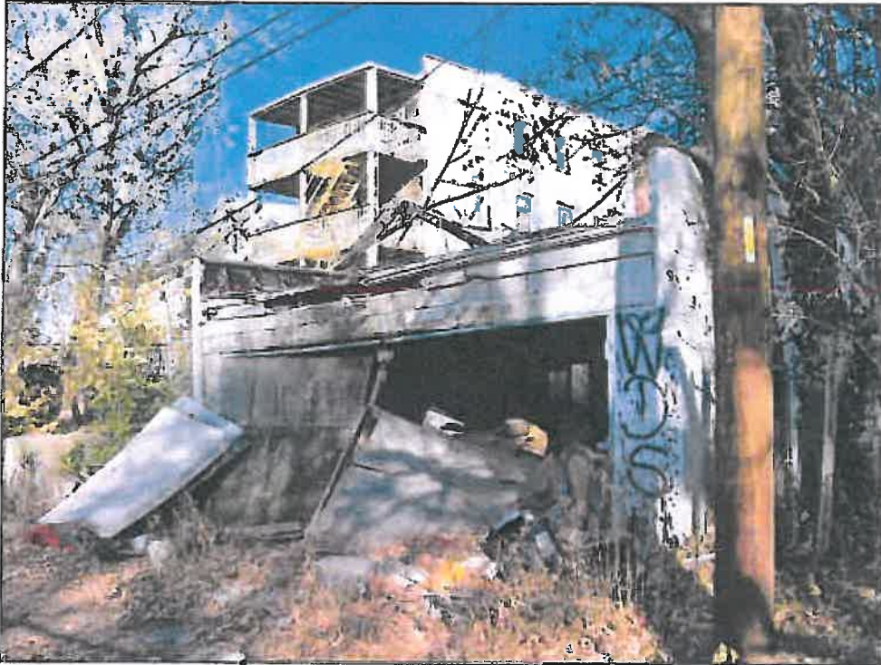
2718 Olive Street – Trash/debris; overgrown vegetation; graffiti; deterioration of garage
