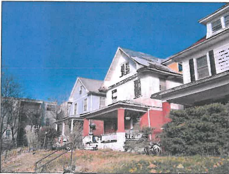
2815 Wabash Avenue – Deterioration of roof, soffit; failure of finishes
