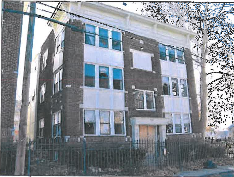
2503 E. 28 th Street – Deterioration of windows, doors; failure of finishes
