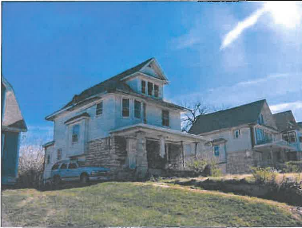
3021 Woodland Avenue – Deterioration of roof, doors, windows fascia/soffit; overgrown vegetation
