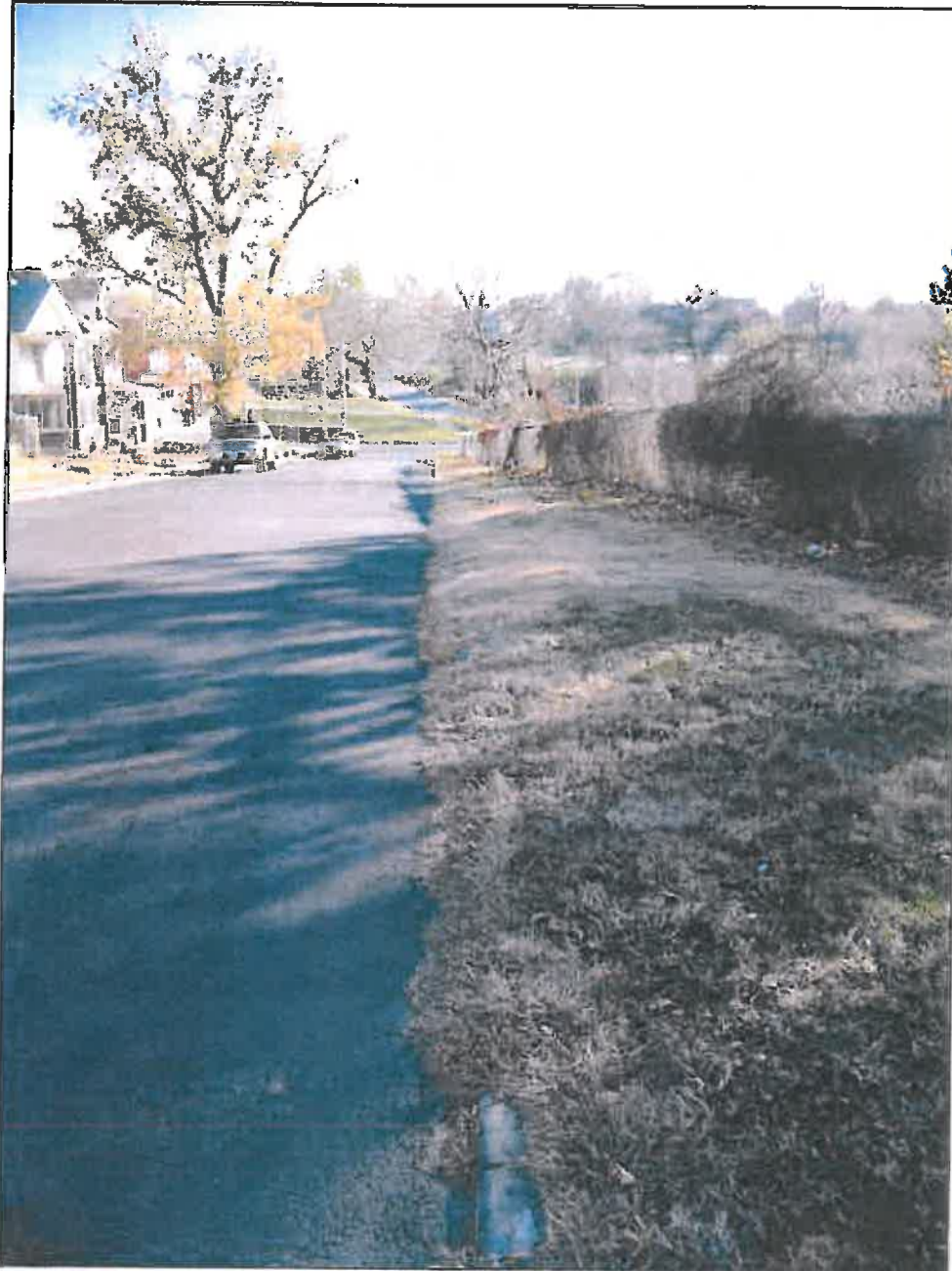
2700 block of Garfield Avenue – non-existent pedestrian circulation, curb and gutter
