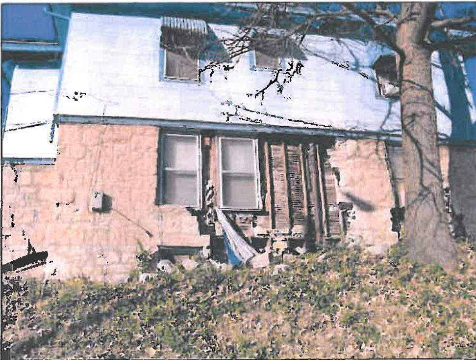
2746 Brooklyn Avenue – Deterioration of wall
