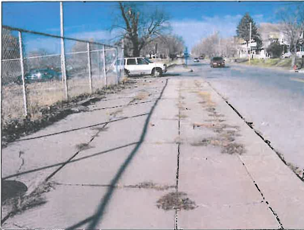
2902 Brooklyn Avenue – Broken/cracked sidewalk; overgrown vegetation
