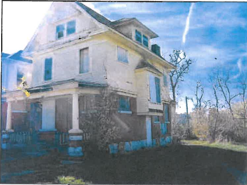
3040 Wabash Avenue – Walls deteriorating; windows and doors deteriorating; fascia deteriorating; finishes failing; trash/debris; weeds
