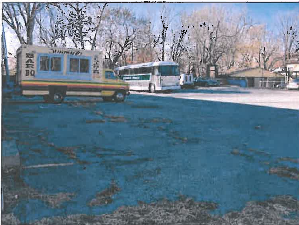
2920 Prospect Avenue – Deterioration of parking surface
