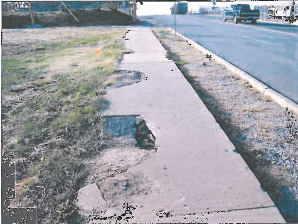
2500 block of E. 27 th Street – Deterioration of sidewalk; lack of landscaping
