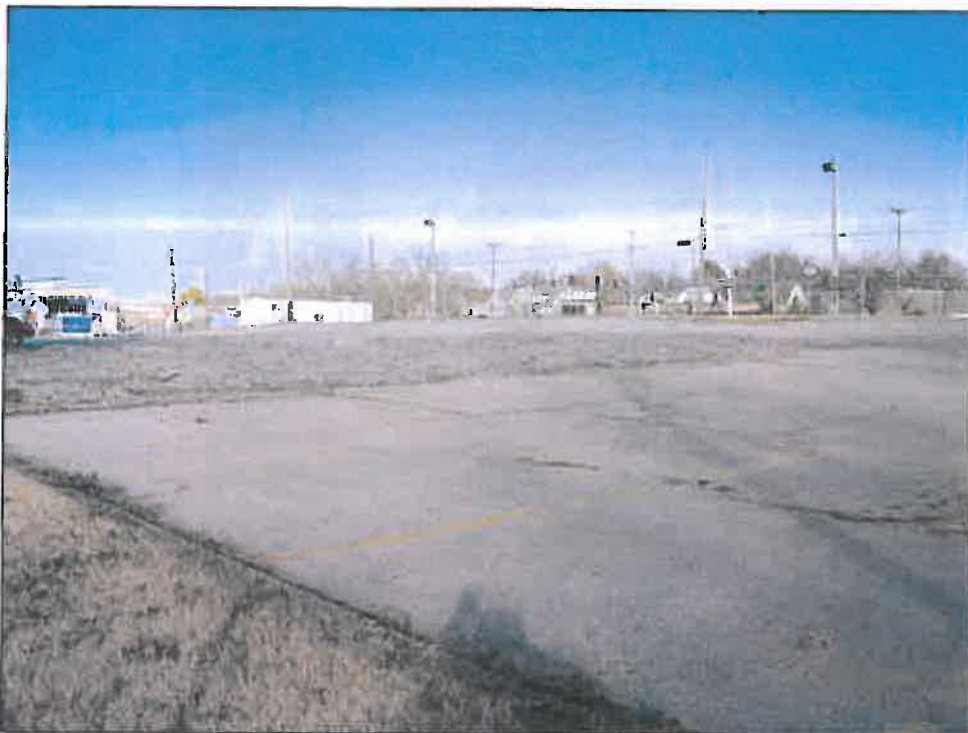
2725 Wabash Avenue – Deterioration of parking surface
