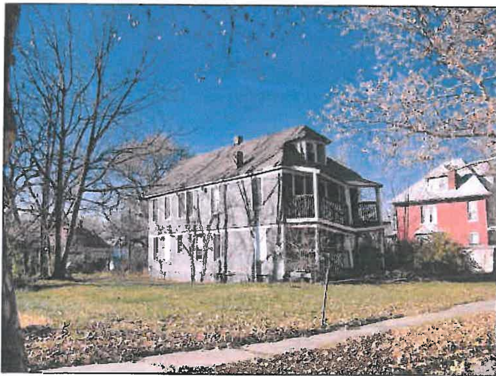
2932 Park Avenue – Deterioration of roof, windows, doors, porch
