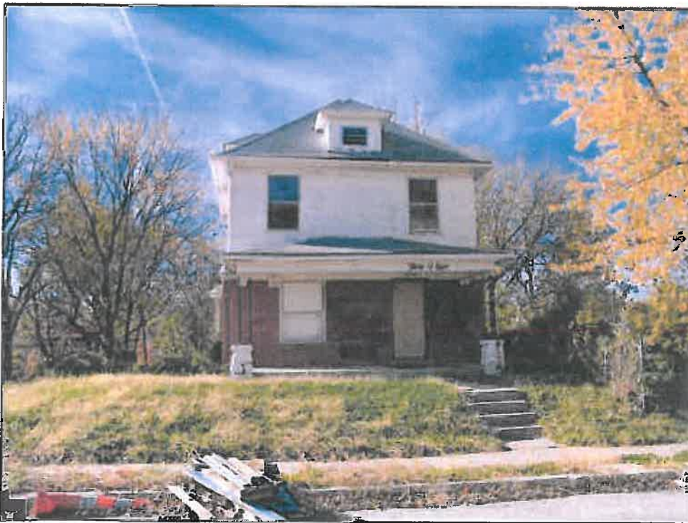
3008 Wabash Avenue – Window and door deterioration; vacant building, trash/debris; deterioration of roof and walls; weeds
