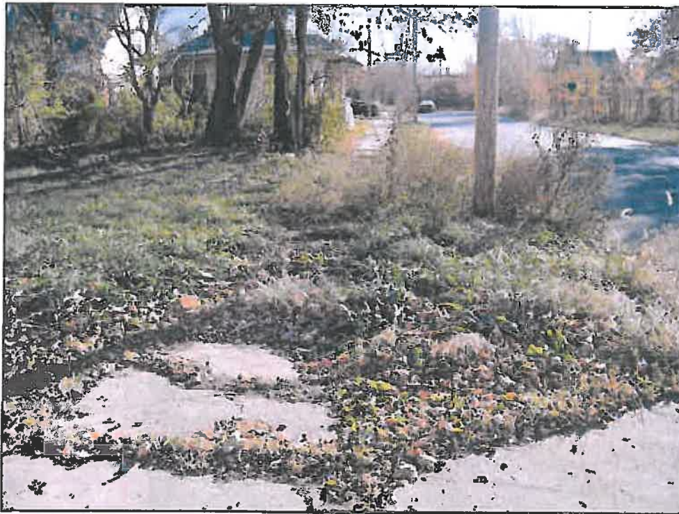
2937 Euclid Avenue – Broken/cracked sidewalk; overgrown vegetation
