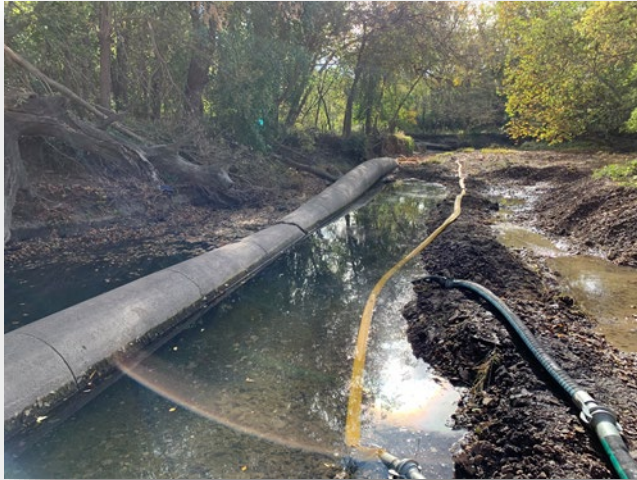
Site 42- Dyke Branch at Holmes Road / $1,500,000 estimated cost / temporary emergency repair already completed
