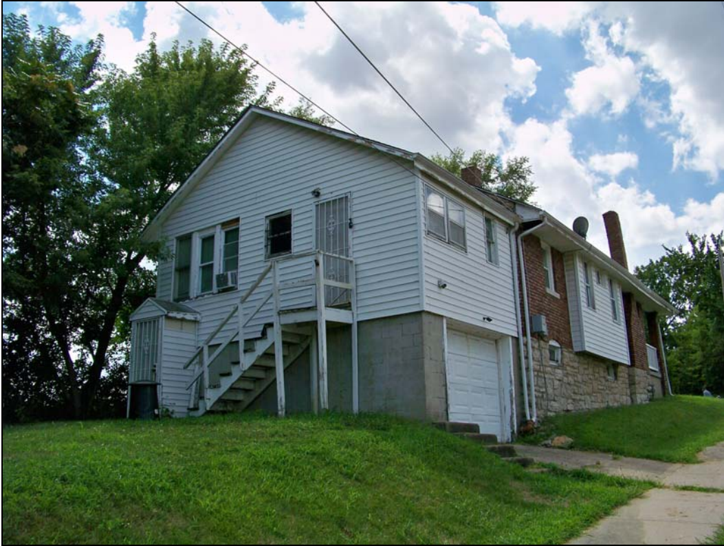
4900 block of Montgall Avenue – failure of finishes; deterioration of wall, windows
