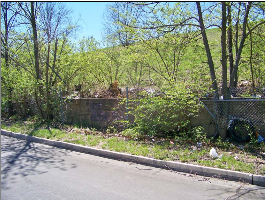
4900 block of Montgall Avenue – deterioration of fence, retaining wall
