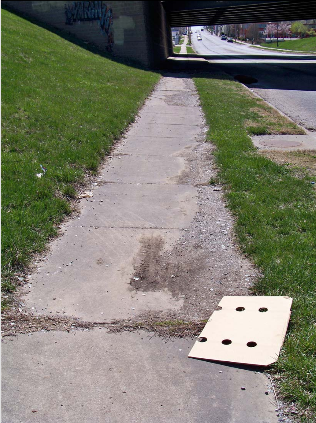
4900 block of Prospect Avenue – deterioration of sidewalk; trash/debris
