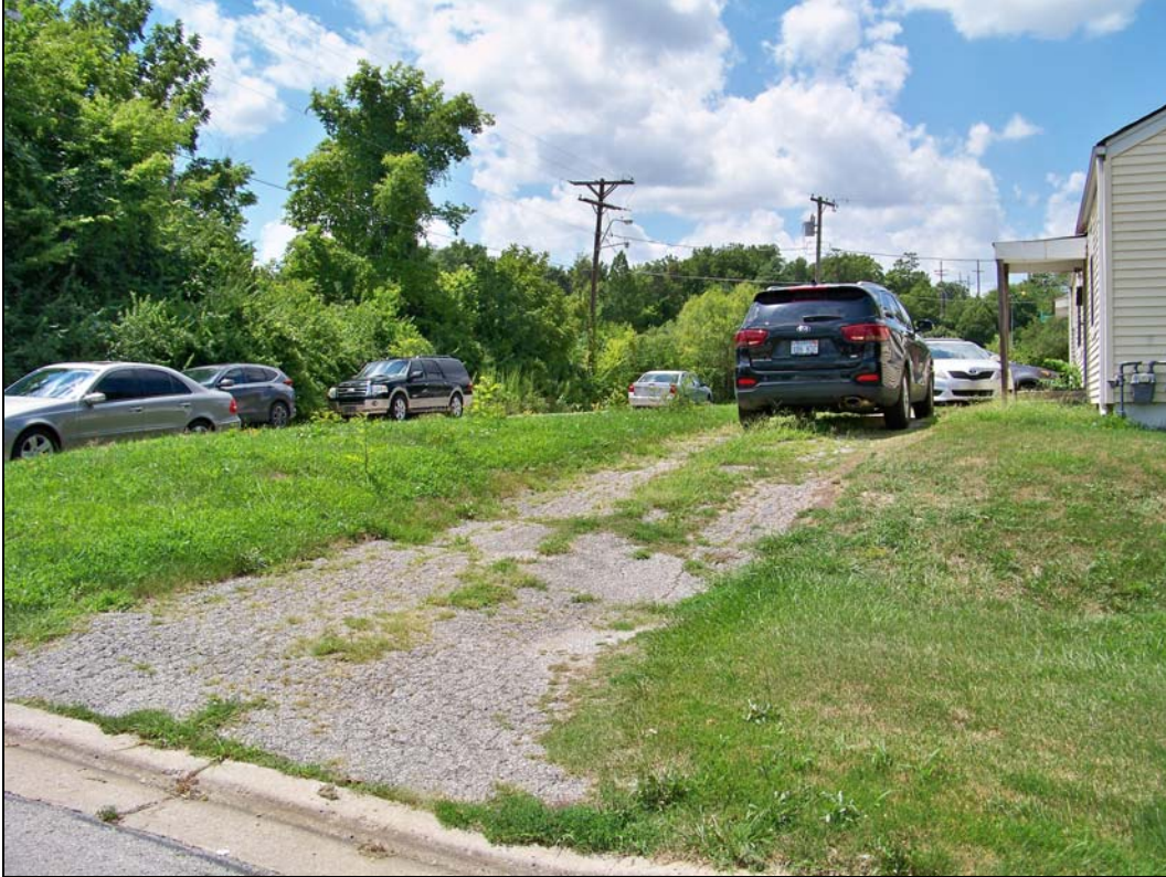
4800 block of Montgall Avenue – deterioration of driveway
