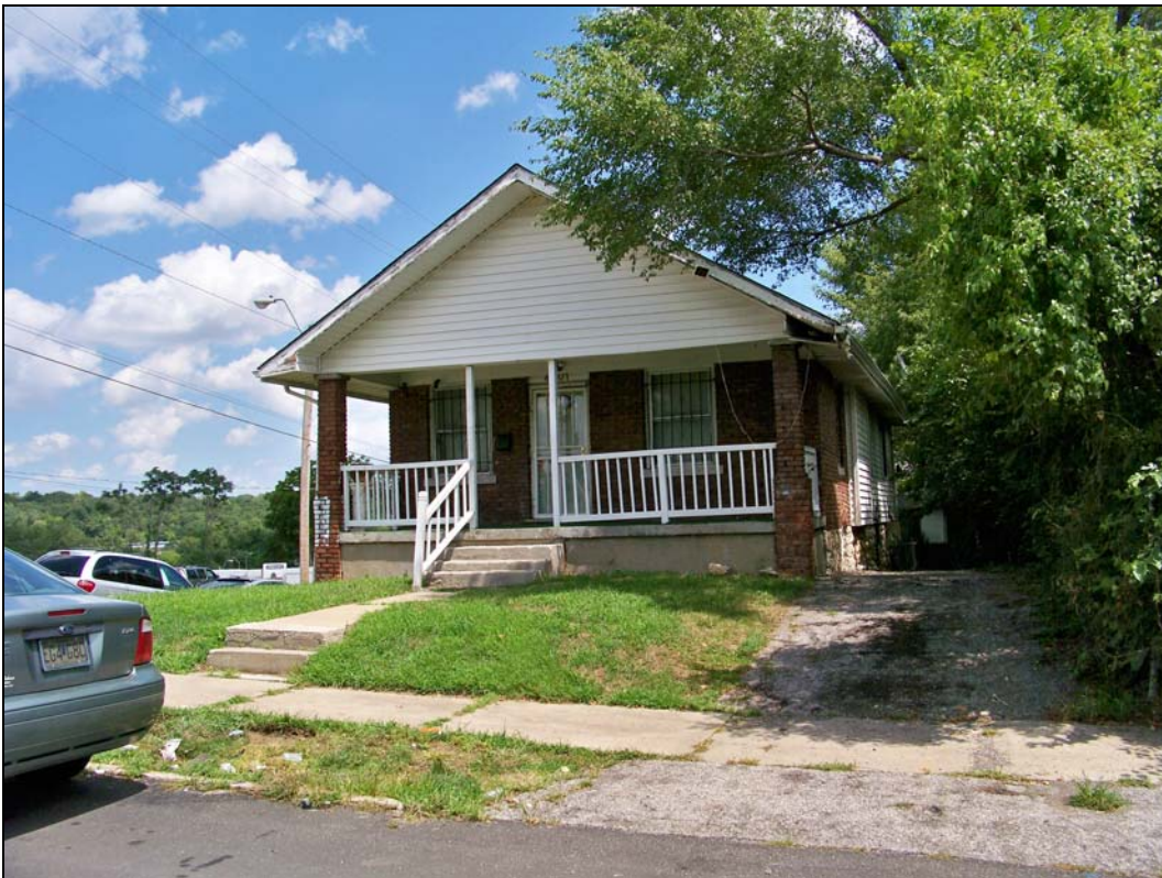
4900 block of Montgall Avenue – failure of finishes; deterioration of fascia, gutter/downspouts, driveway
