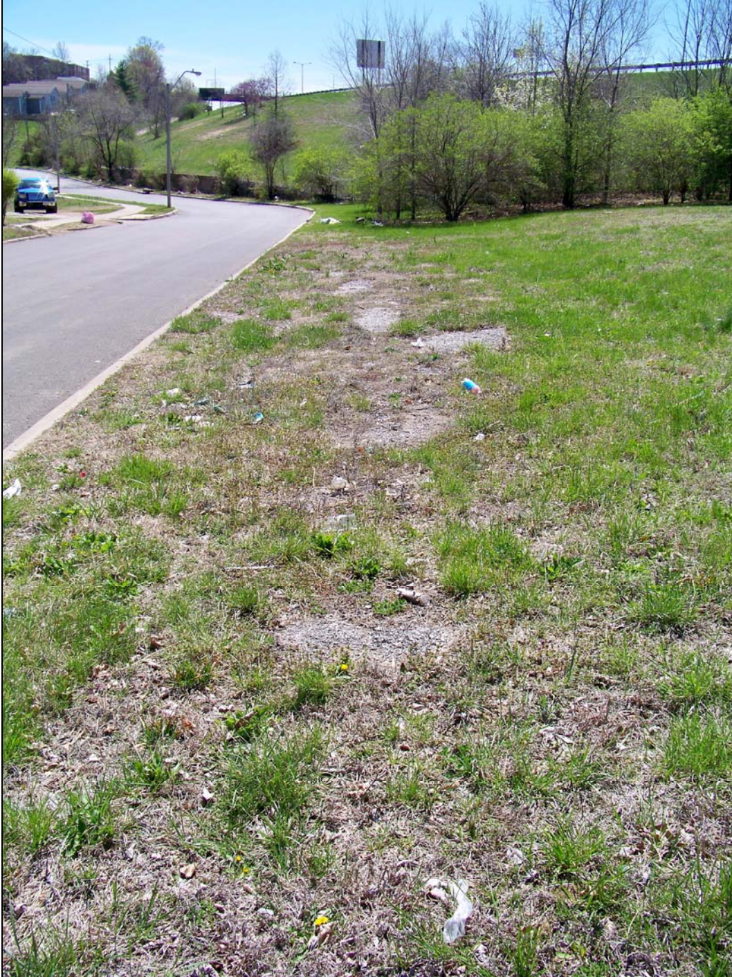
4900 block of Montgall Avenue – deterioration of sidewalk
