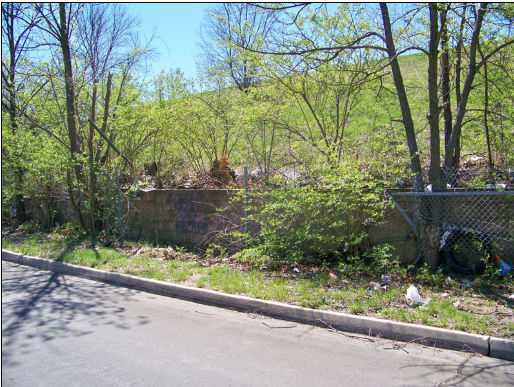
4900 block of Montgall Avenue –trash/debris; overgrown vegetation; graffiti; deterioration of fence, wall
