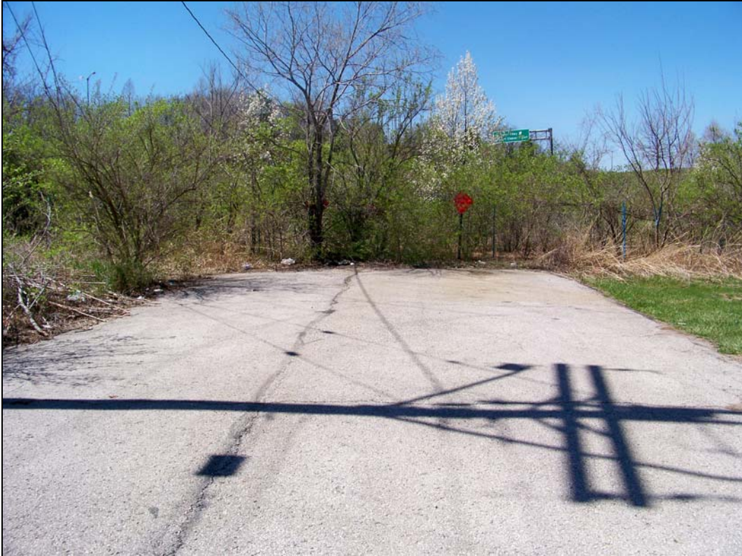
2600 block of E. 49 th Street – dead end street not code compliant; overgrown vegetation; trash/debris
