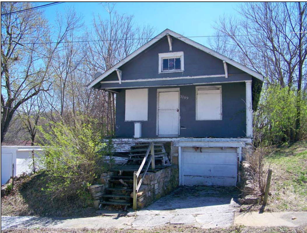
2700 block of E. 49 th Street – dangerous building; deterioration of doors, windows, structure
