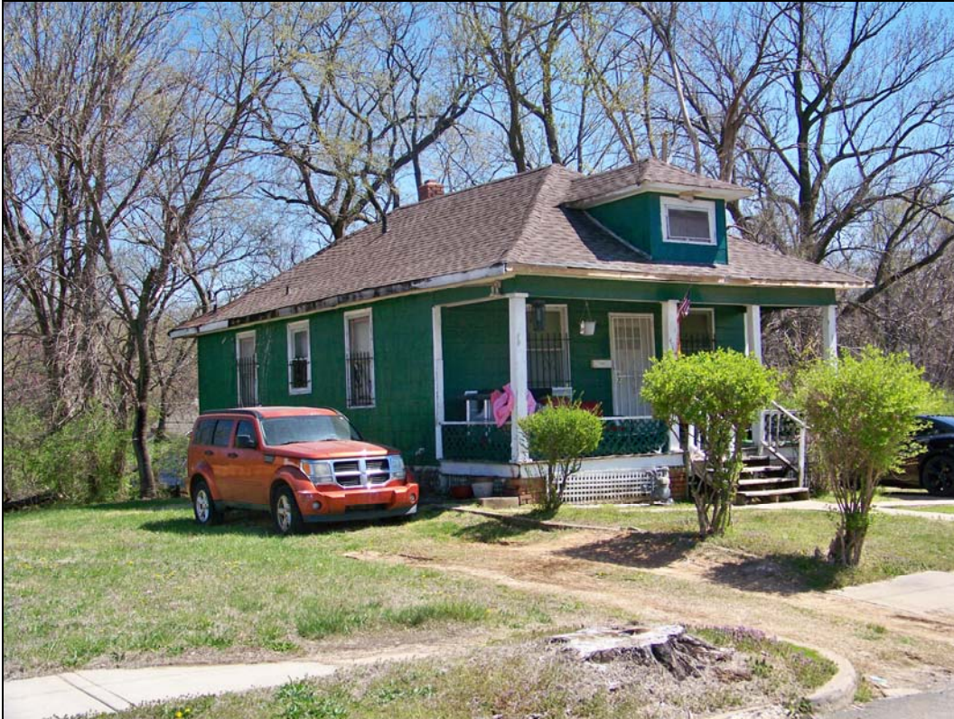
4900 block of Montgall Avenue – deterioration of roof, fascia, soffit, siding; failure of finishes
