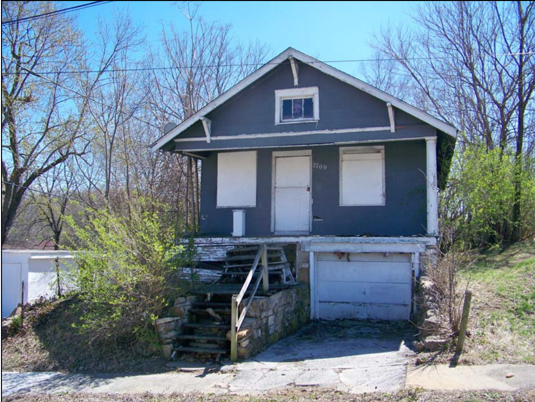
2700 block of E. 49 th Street – deterioration of stairs, driveway; porch column missing
