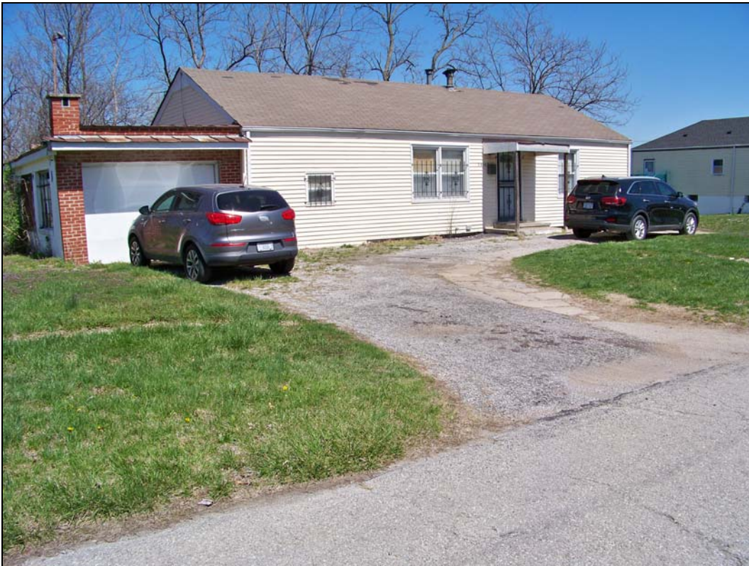
4800 block of Montgall Avenue – deterioration of driveway
