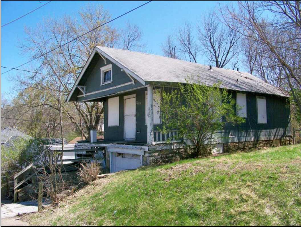
2700 block of E. 49 th Street – dangerous building; deterioration of roof; failure of finishes
