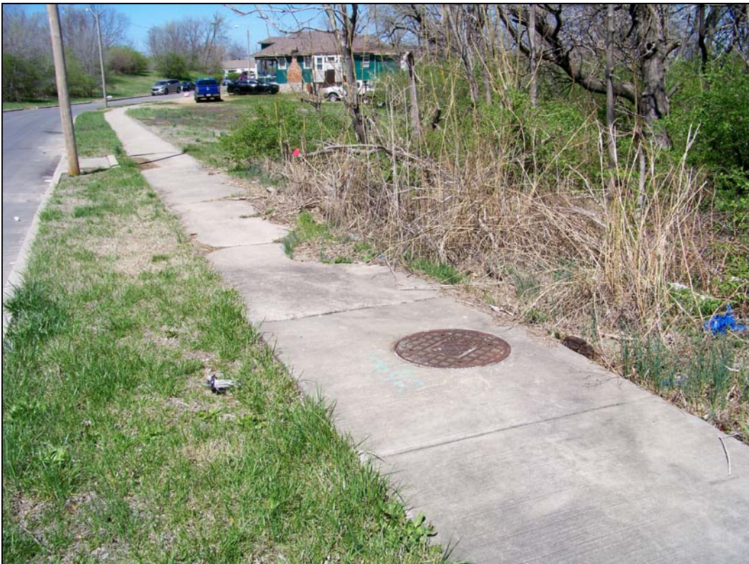
4900 block of Montgall Avenue – deterioration of sidewalk
