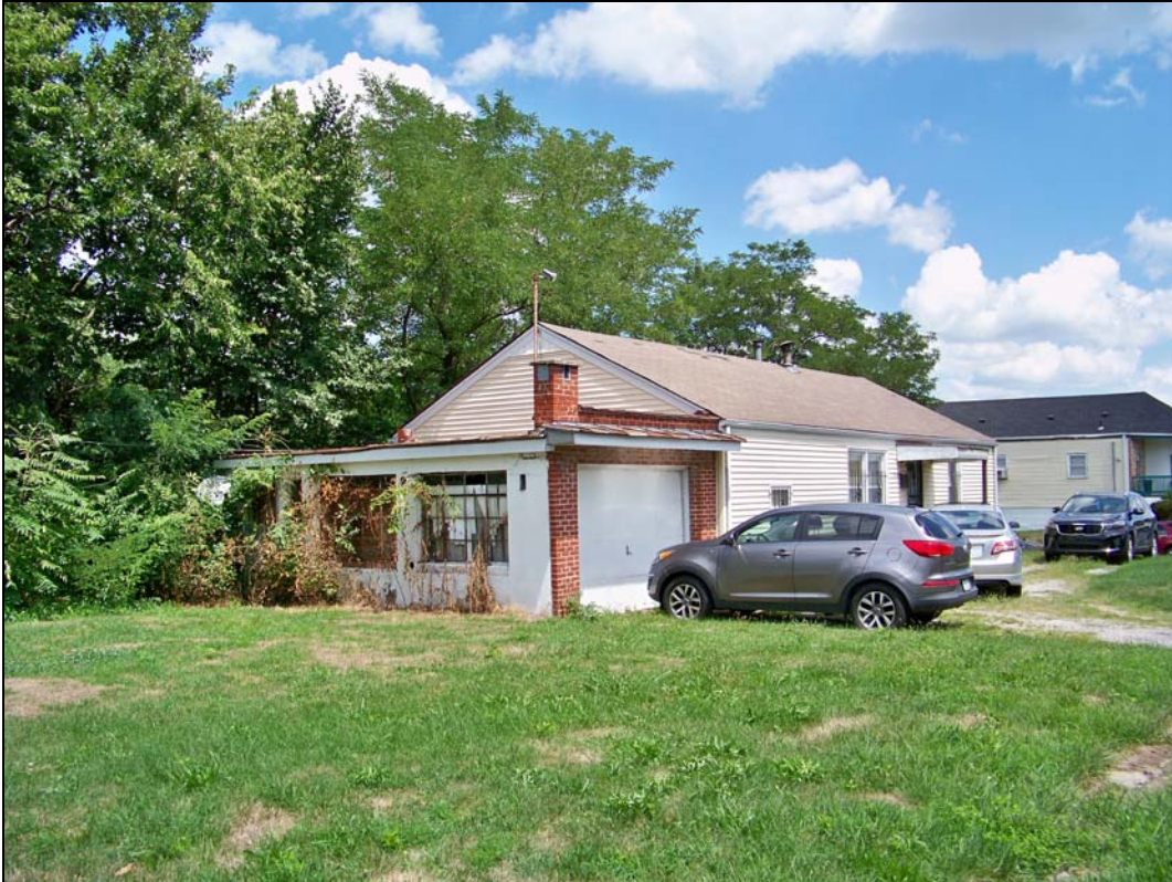
4800 block of Montgall Avenue – deterioration of roof, windows, walls, overhang
