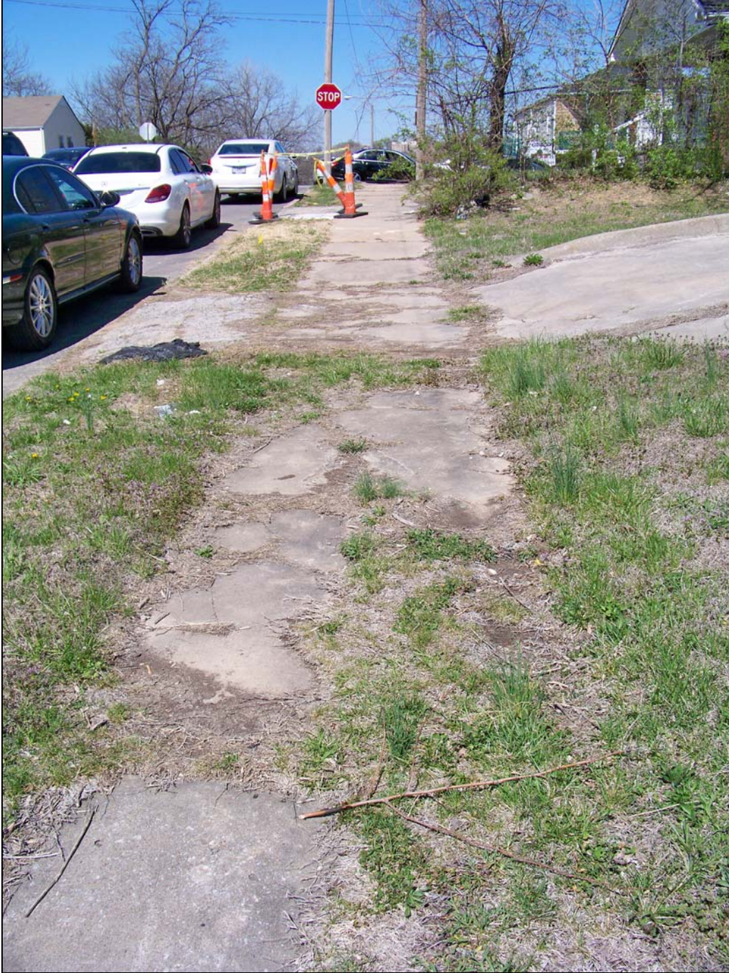
4900 block of Montgall Avenue – deterioration of sidewalk
