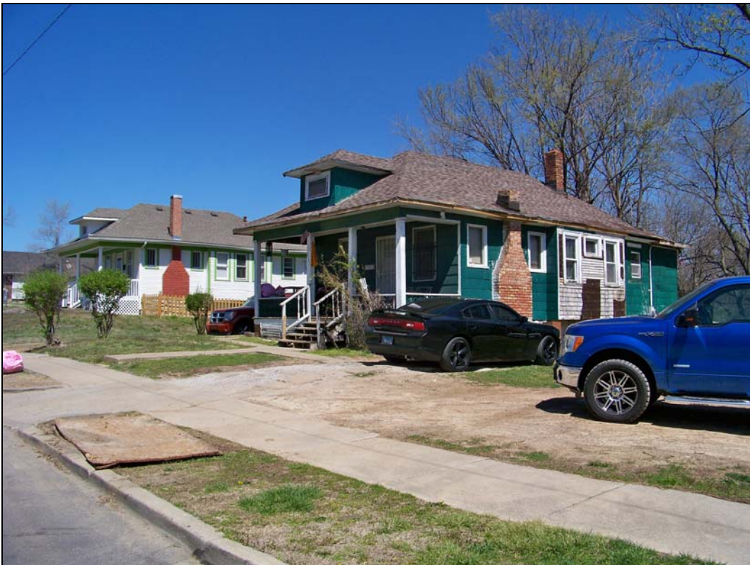
4900 block of Montgall Avenue – deterioration of roof, fascia, soffit, siding; failure of finishes
