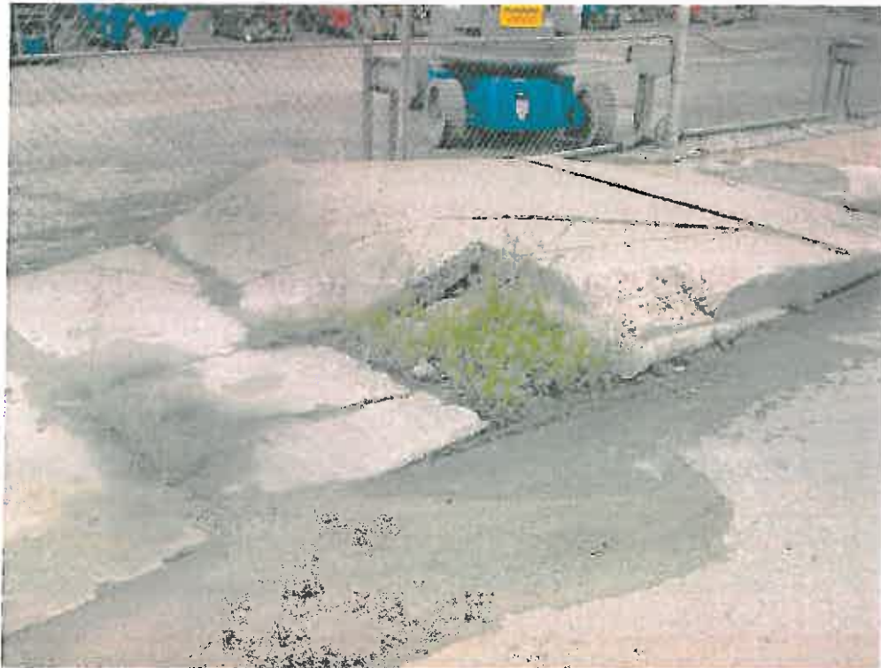
Severely damaged sidewalk (1600 block Cherry St.)
