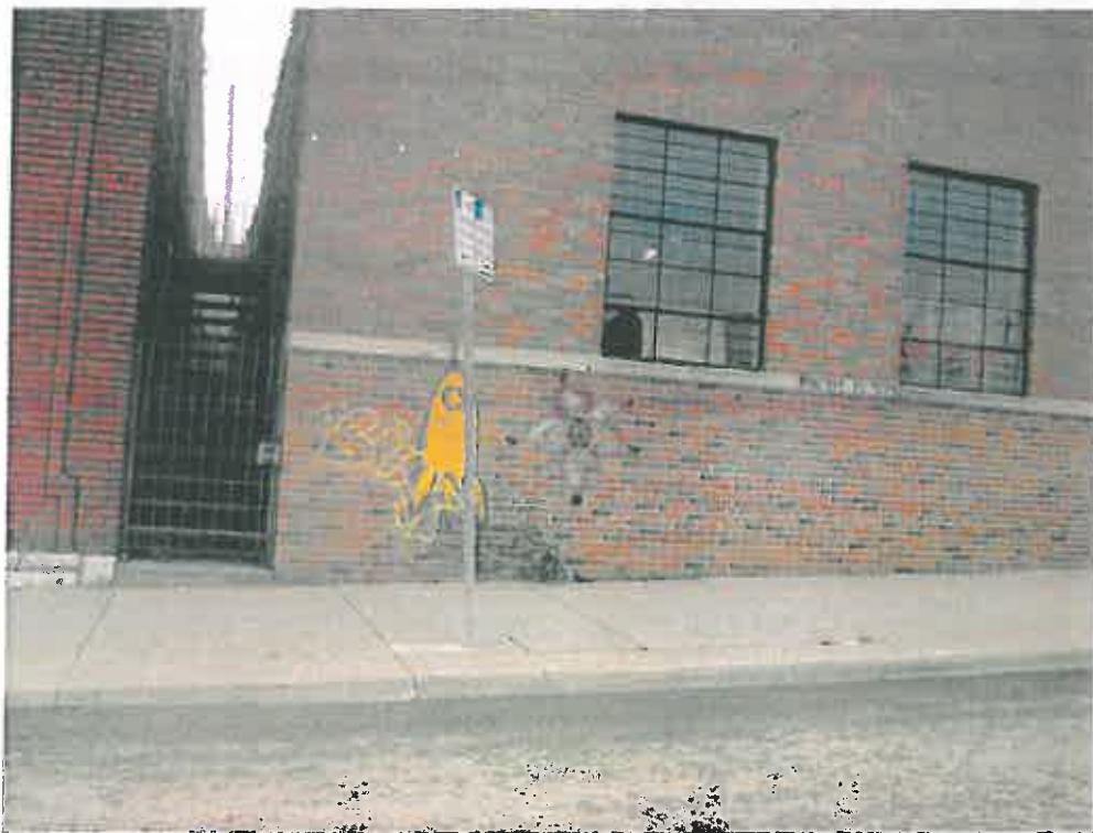
Broken windows and excessive graffiti (1700 block Holmes St.)
