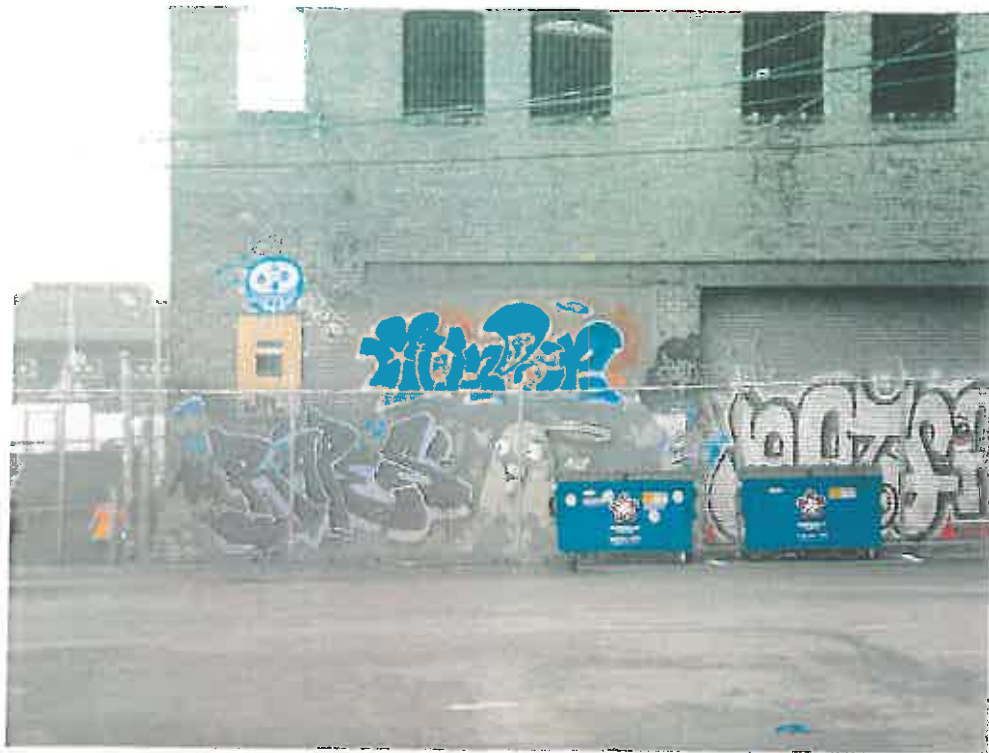
Significant graffiti (alleyway, 1700 block Locust to Cherry Streets)
