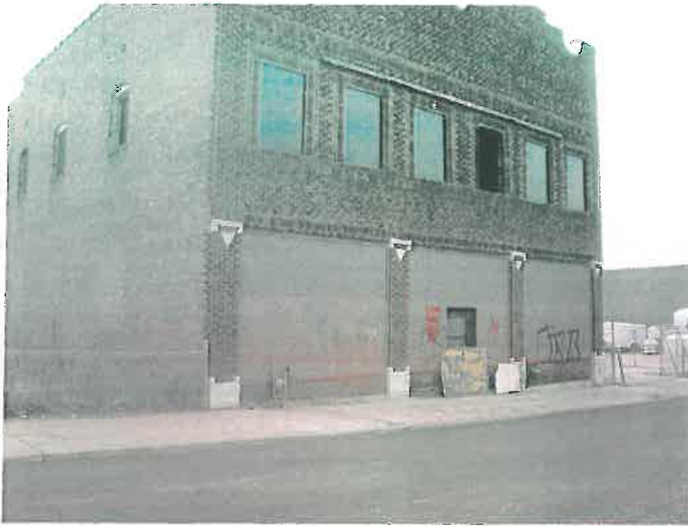
Boarded building (1707 Locust St.)
