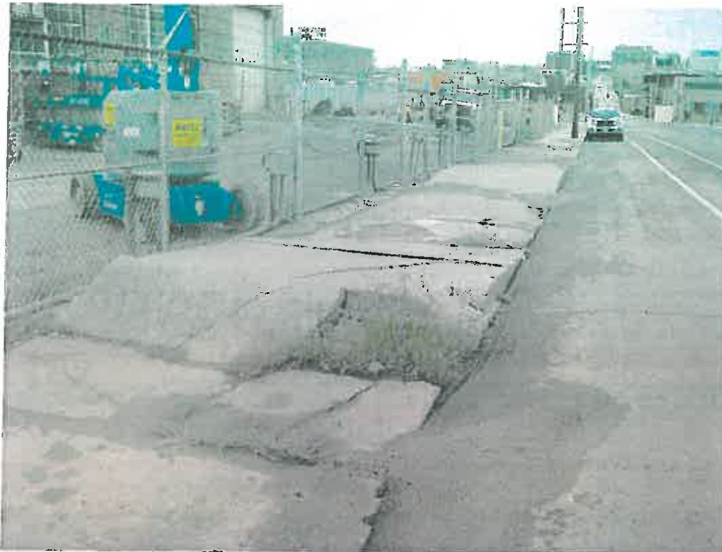
Damaged, deteriorated sidewalk – (1600 block Holmes St.)
