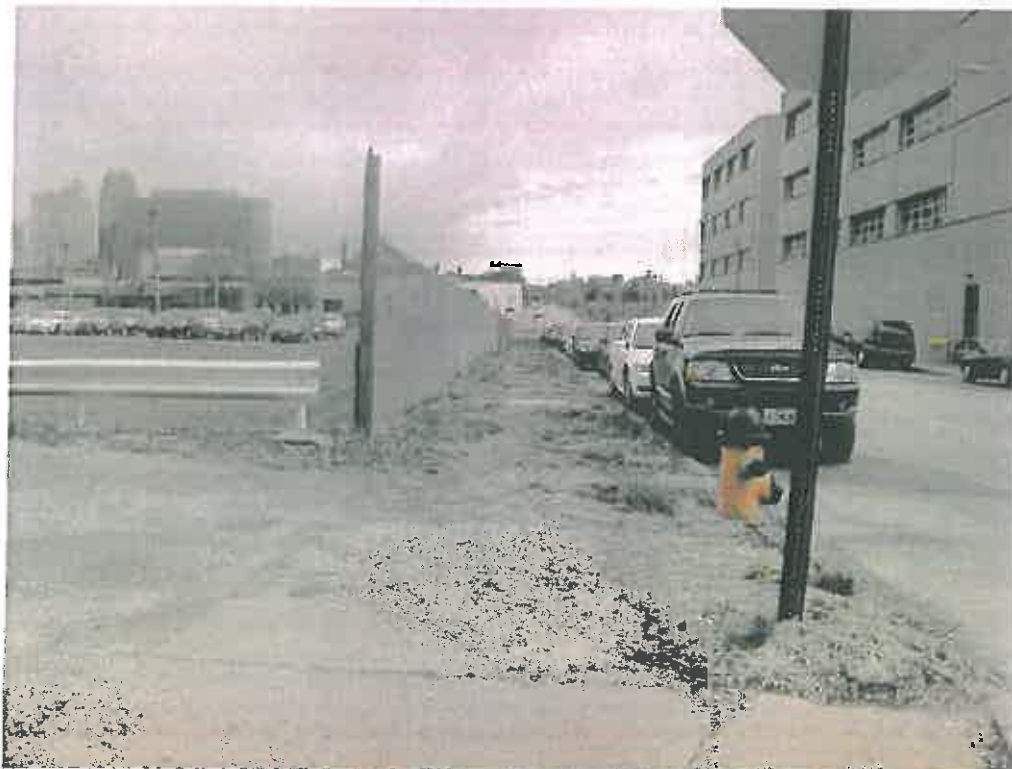
Significantly deteriorated, missing sidewalk – (1800 block Campbell St.)
