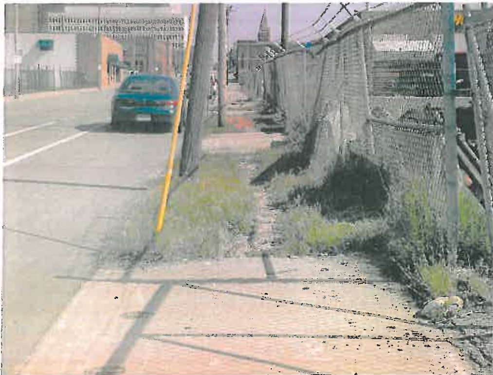
Substandard sidewalk (1700 Block Holmes St.)
