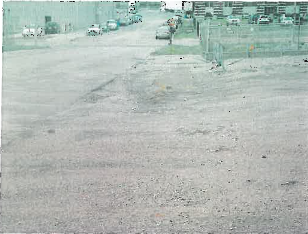
Missing or significantly deteriorated sidewalk - (1700 block Campbell St.)
