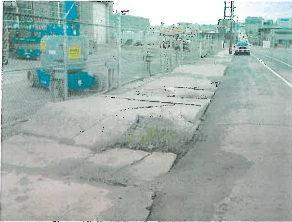
Deteriorated Sidewalk (1600 block Holmes St.)
