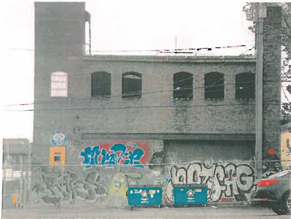
Rear 1707 Locust (Excessive graffiti, lack of window systems-open to the elements.)
