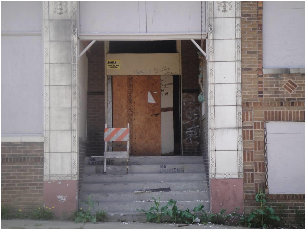
Photo 3 – View of the northern entrance to the subject building. Note the general lack of maintenance, as well as the lack of adequate ADA access. Lack of ADA access is a contributing factor to the overall inadequacy and outmoded design of the facility.
