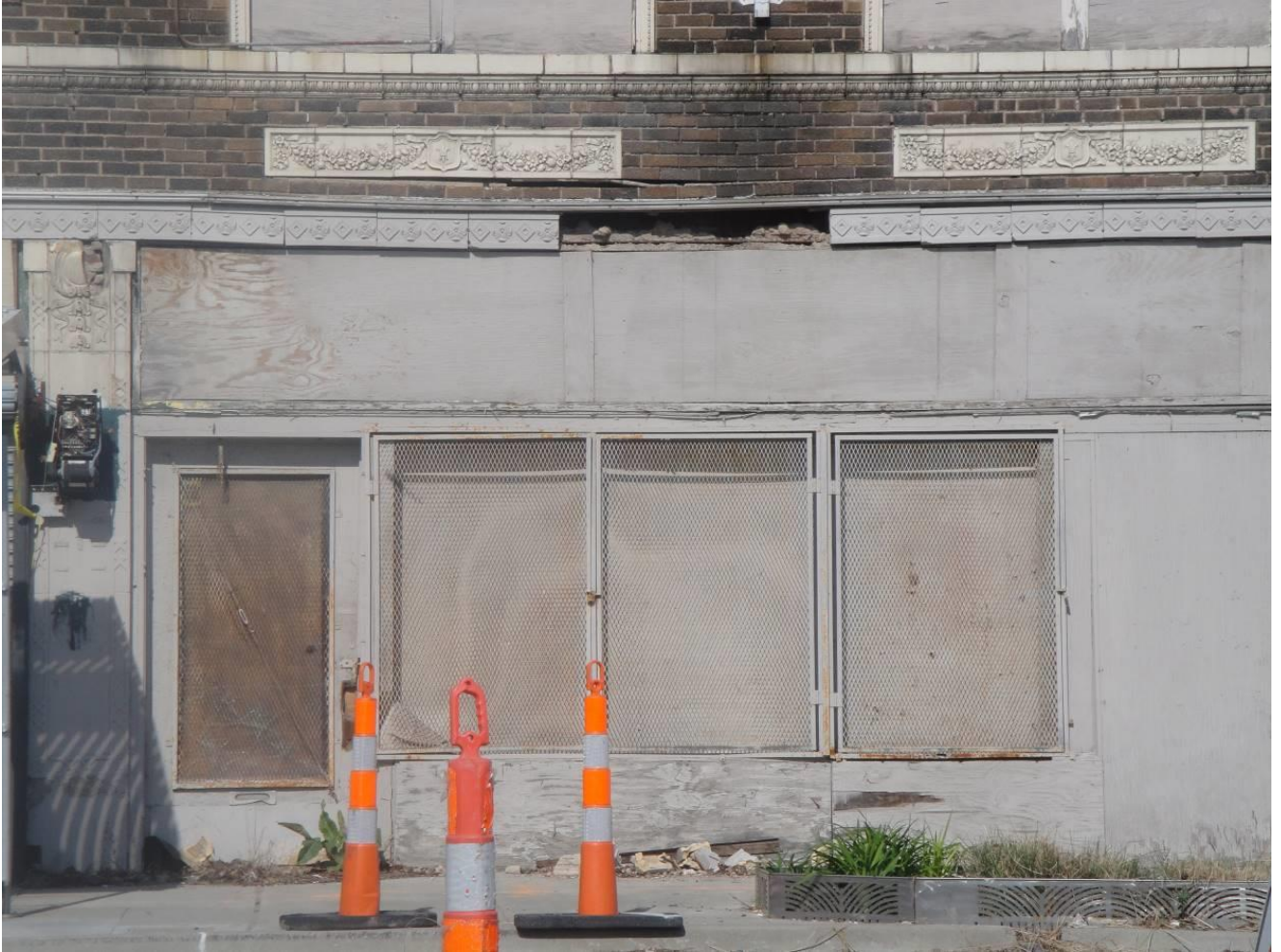
Photo 9 – Detail of the eastern façade of 2700 Troost. Note façade deterioration due to the lack of downspout.
