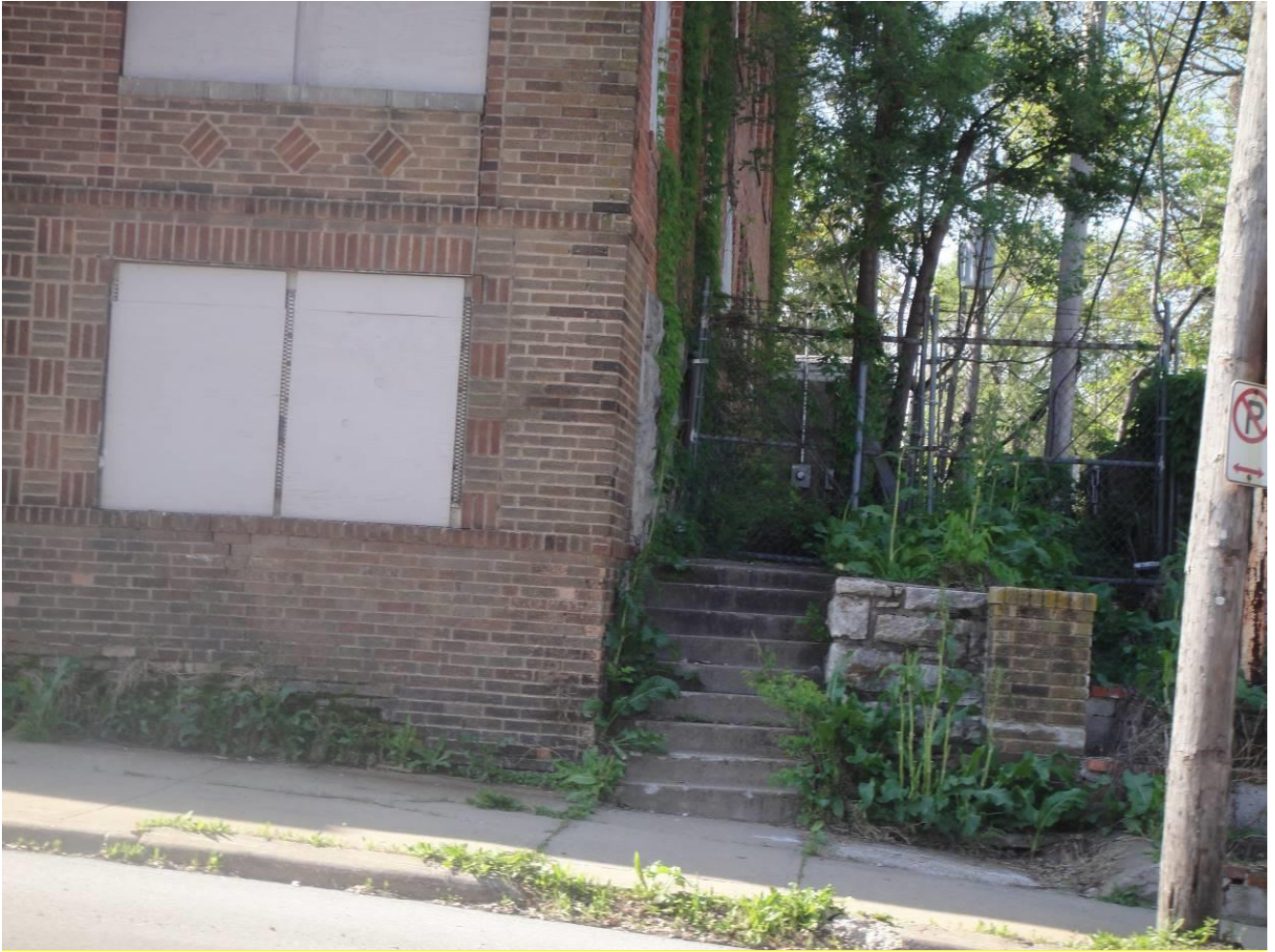
Photo 5 – Western access to the subject property and facility. This area is poorly lit and conducive to illegal dumping and vagrancy.
