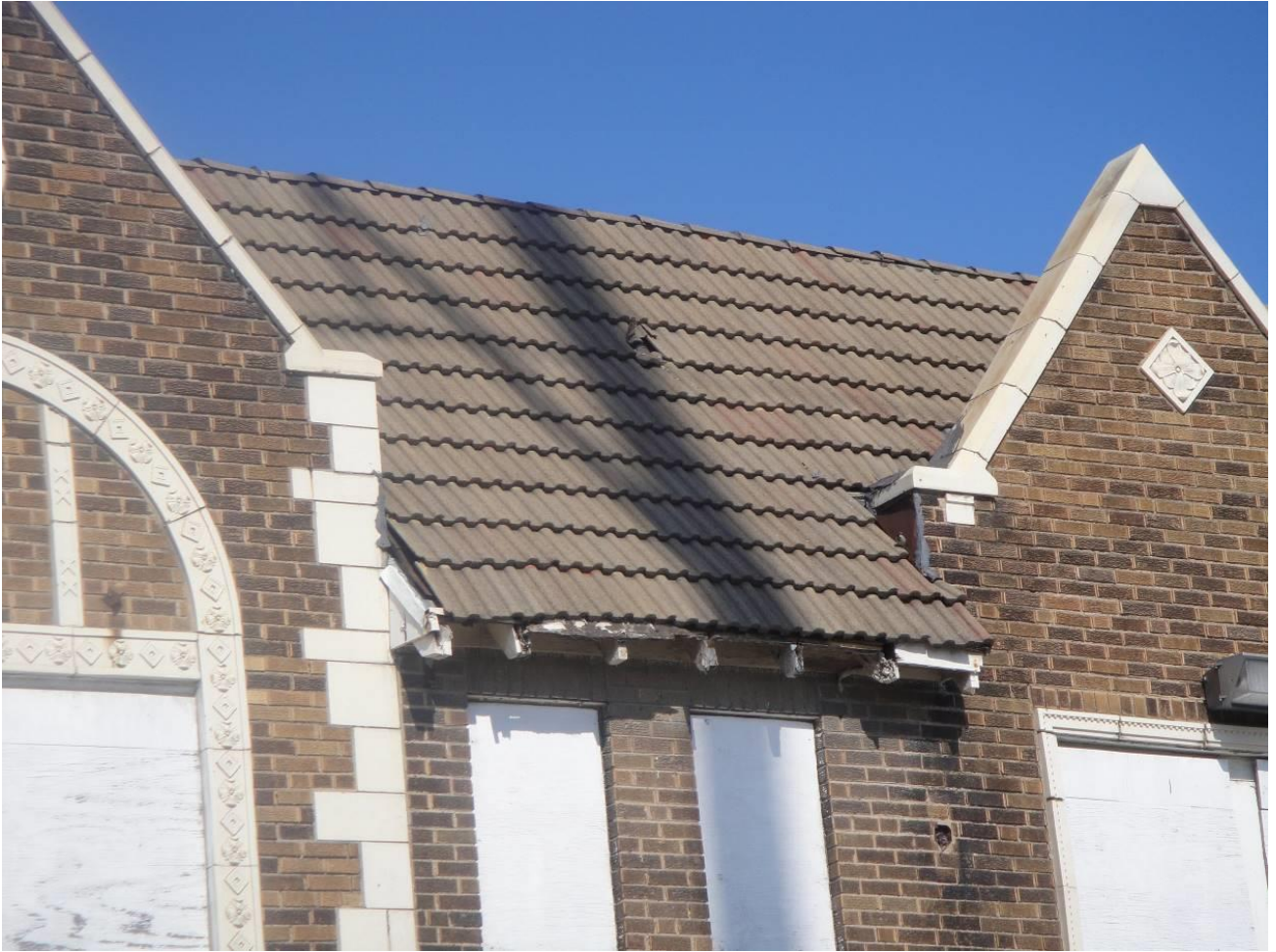
Photo 10 – View of the parapet detail along the eastern façade of the subject building. Note scattered, damaged roof materials. Roofing material appears to be original to facility. Also note lack of gutter and downspout systems to facilitate the discharge of excess rain-water away from the building structure. If deteriorated conditions persist, they could lead to water infiltration which would decrease value of property and deter potential tenants and shoppers, constituting an economic liability and contributing in the inability to pay reasonable taxes.
