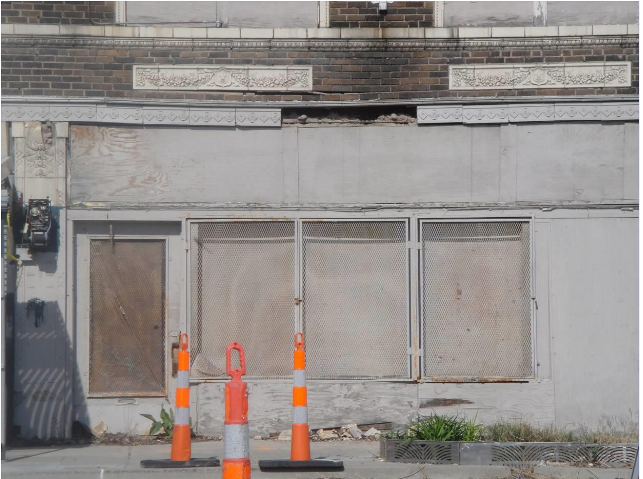
Photo 4 – Detail of the eastern façade of 2700 Troost. Note façade deterioration due to the lack of downspout.
