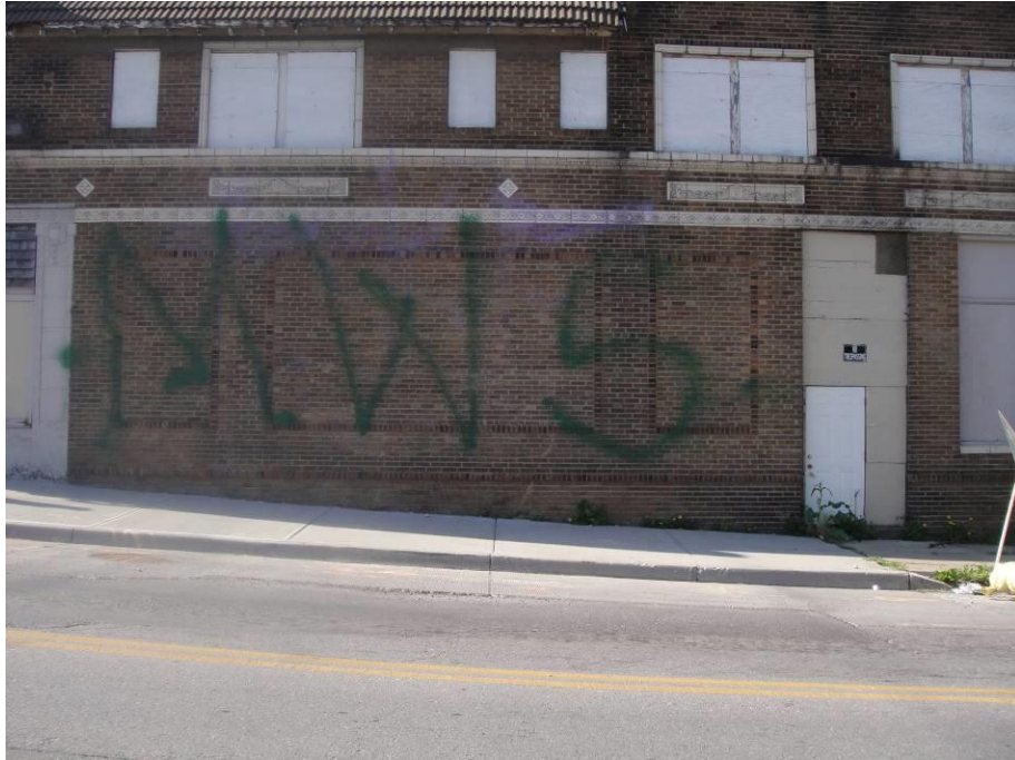
Photo 6 – Graffiti along the northern façade of the subject building. The presence of graffiti continues the perception of a underutilized and vacant facility and can cause a economic and social liability to the surrounding neighborhood.
