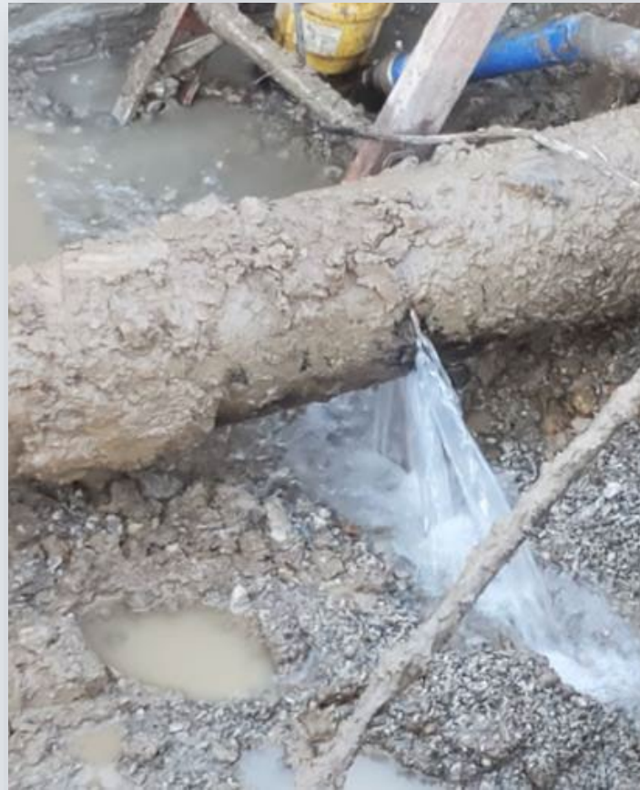
Broken water main leaking
