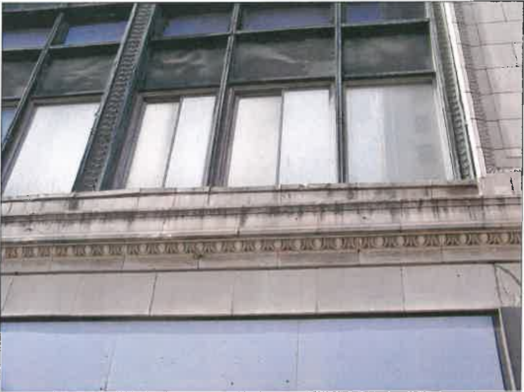
Front façade – deterioration of mortar resulting in loose terra cotta; copper curtain wall requires restoration
