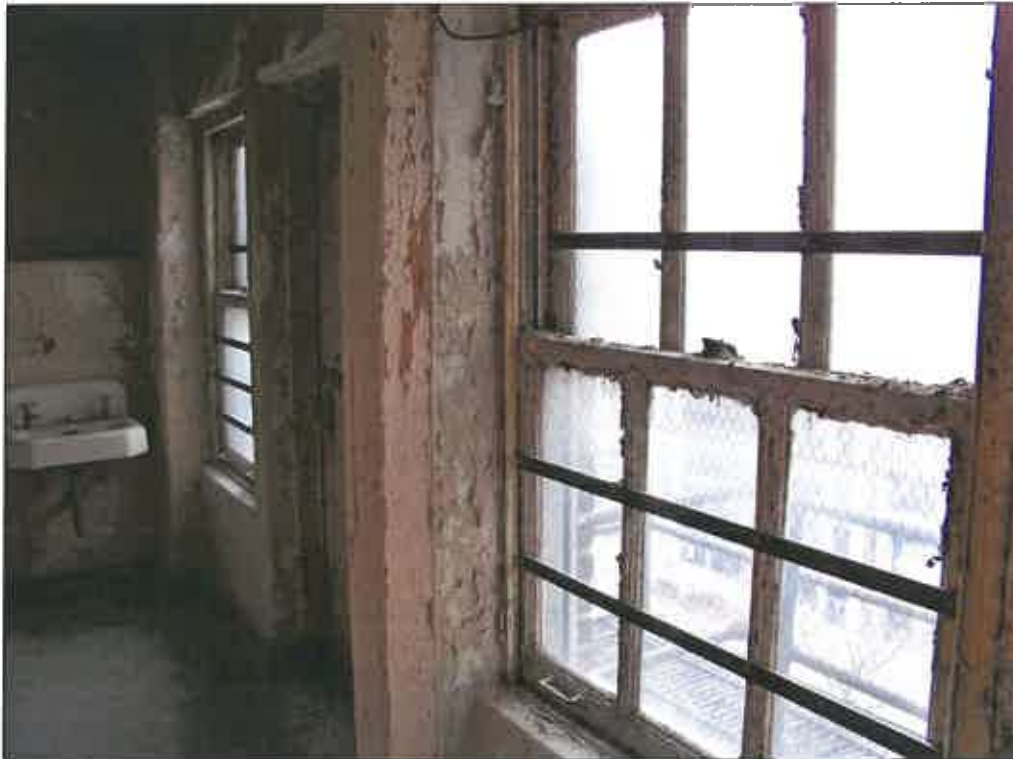
Interior – failure of finishes
