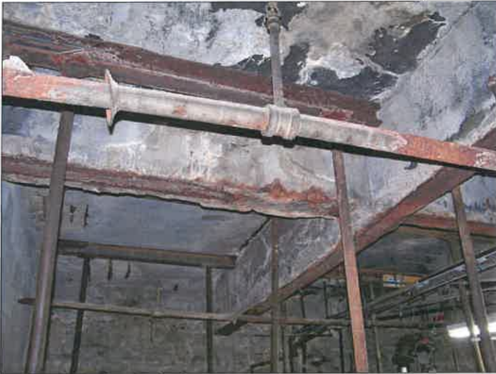
Interior – deterioration of steel and concrete structural components, supports
