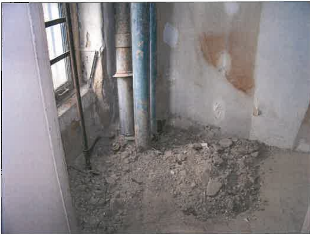
Interior – failure of finishes; debris
