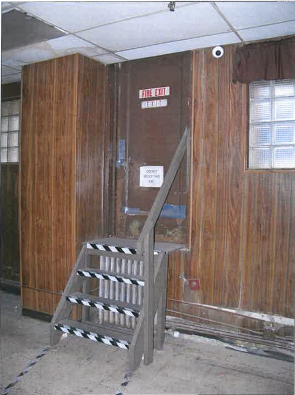
Interior – improper access to fire exit, lack of emergency lighting
