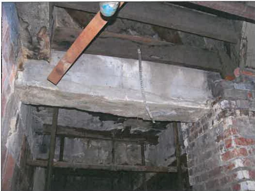
Interior – deterioration of heavy mill lumber beams, brick piers
