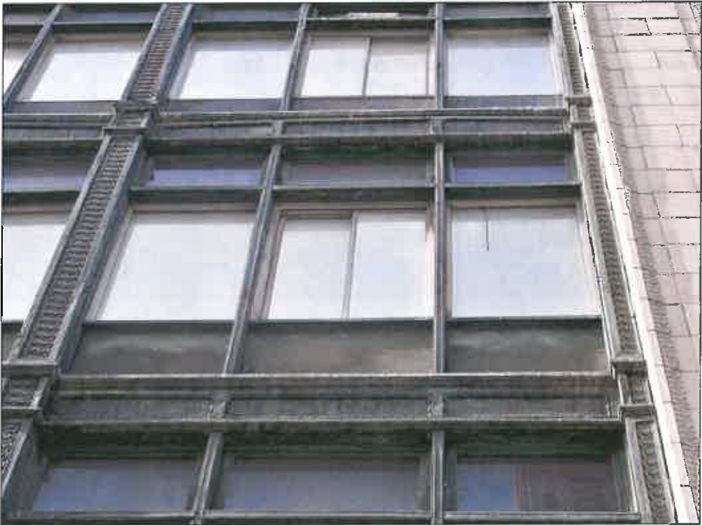
Front façade – deterioration of windows; copper curtain wall requires restoration
