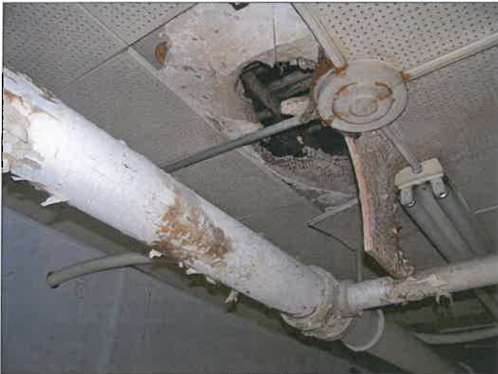
Interior – evidence of water intrusion, deterioration of ceiling
