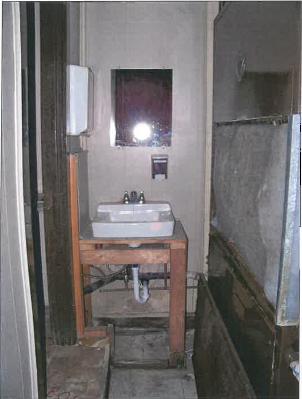
Interior – restroom with poor accessibility, improper clearances
