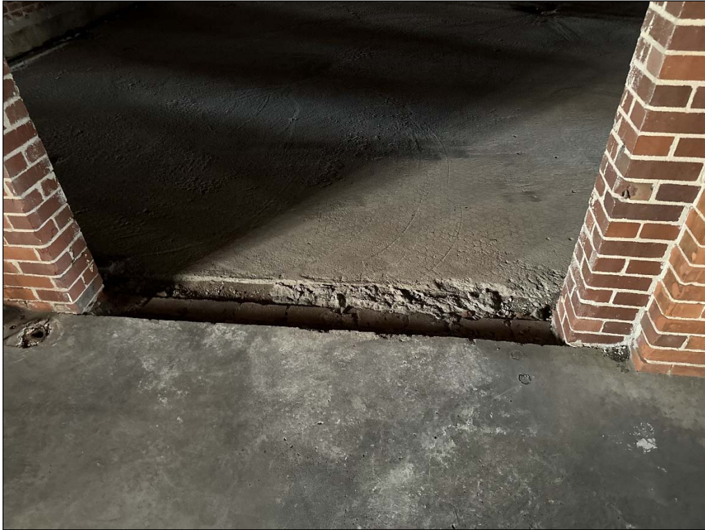
1905 Walnut Street – interior – uneven floor
