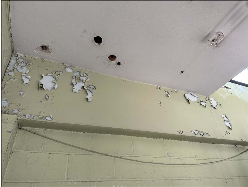
100 E. 20 th Street – interior – failure of finishes
