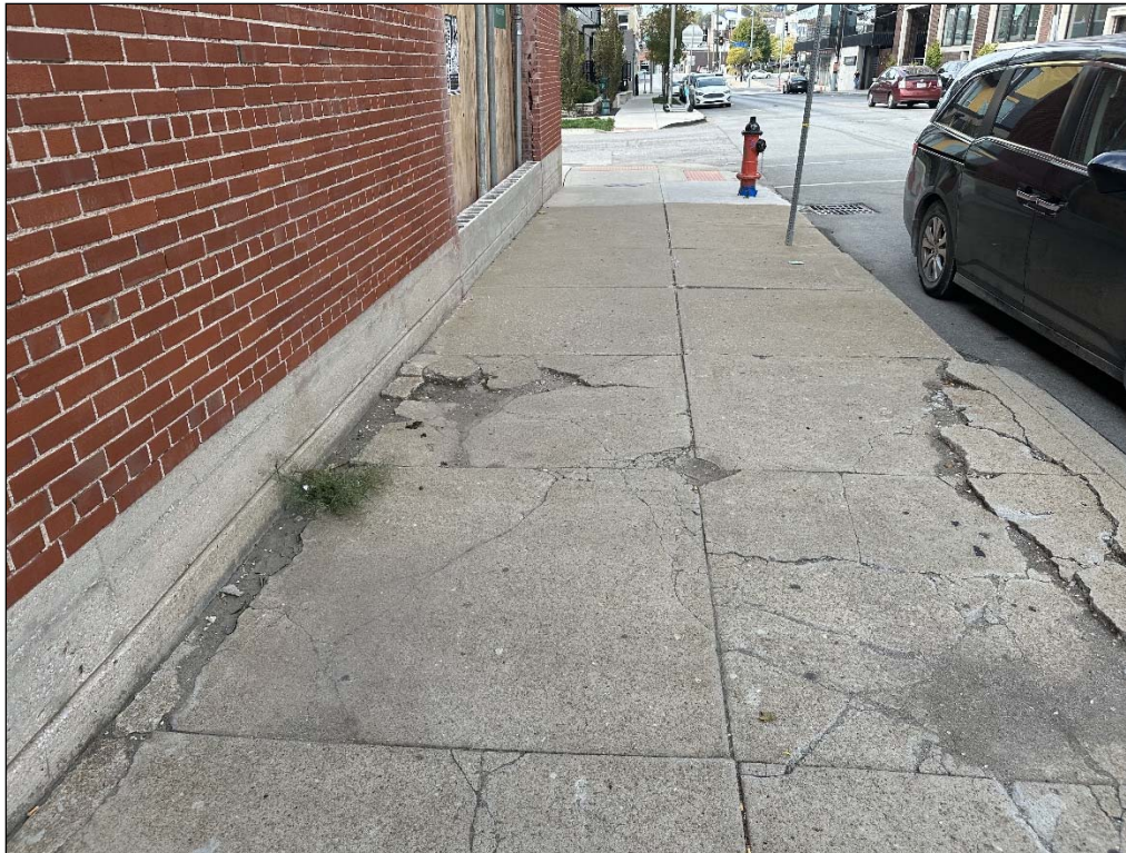
1905 Walnut Street – looking west – deteriorated sidewalk
