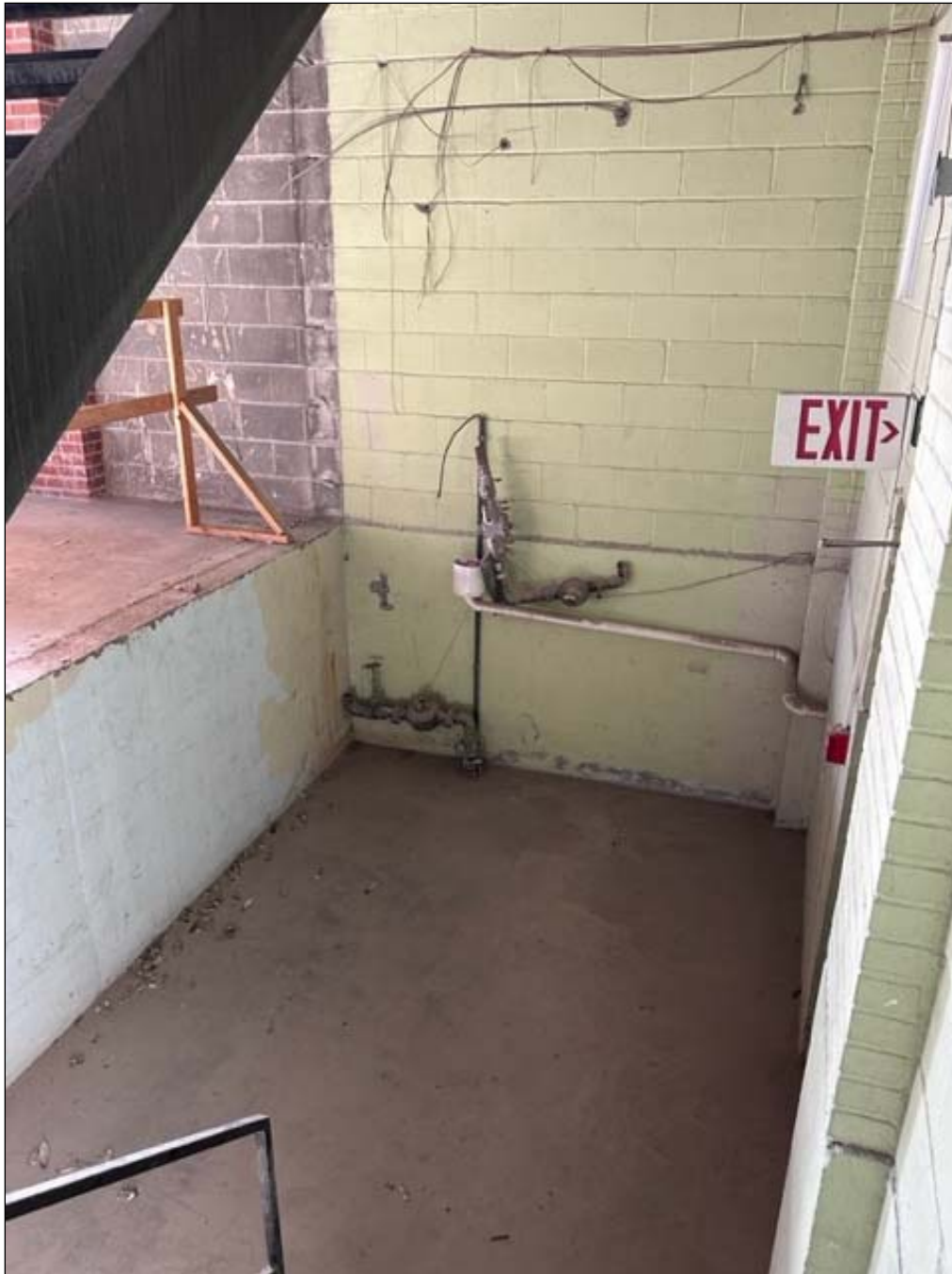
100 E. 20 th Street – interior – disconnected building systems
