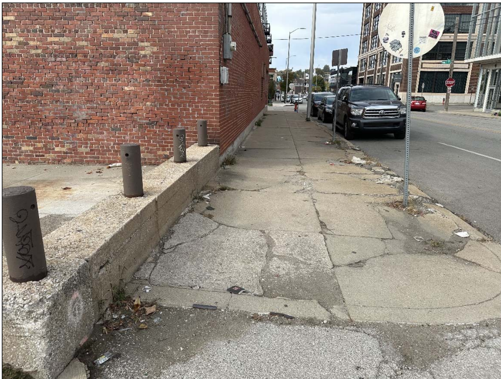
1905 Walnut Street – looking west – deteriorated sidewalk
