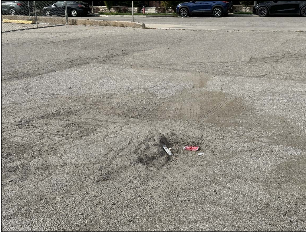
1905 Walnut Street – looking southwest – uneven pavement
