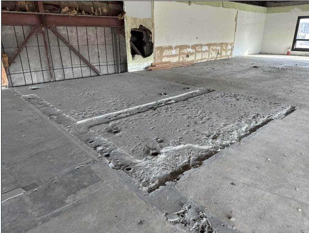
100 E. 20 th Street – interior – uneven floor
