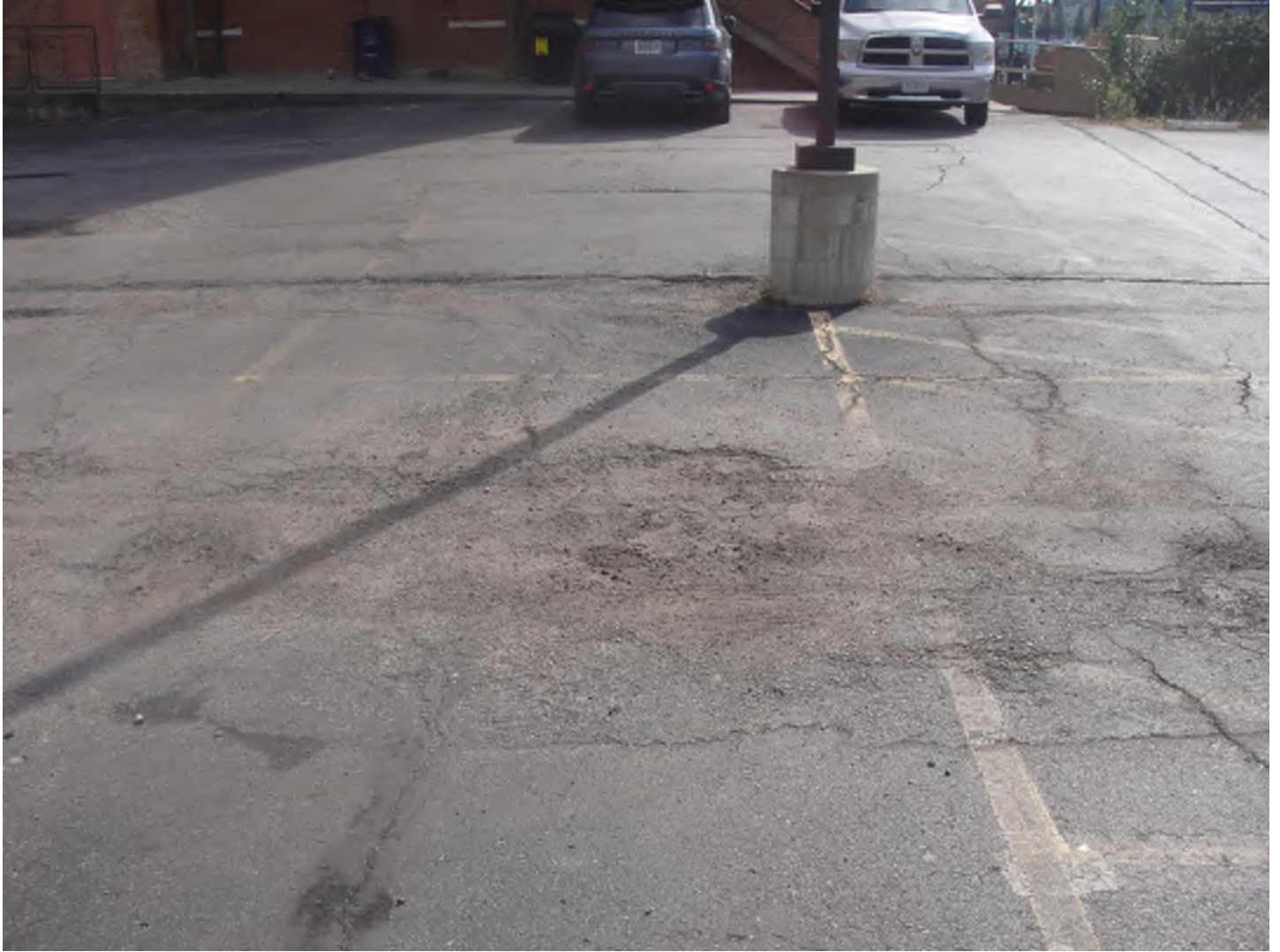
Photo 6 – Block 138. Deteriorated surface paving scattered across the site.
