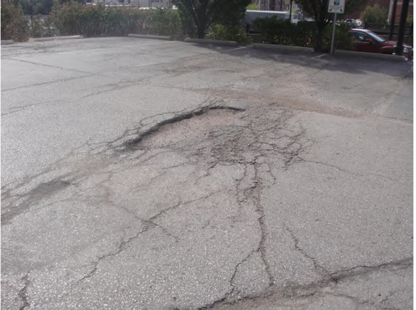
Photo 5 – Block 138. Deteriorated surface paving scattered across the site.
