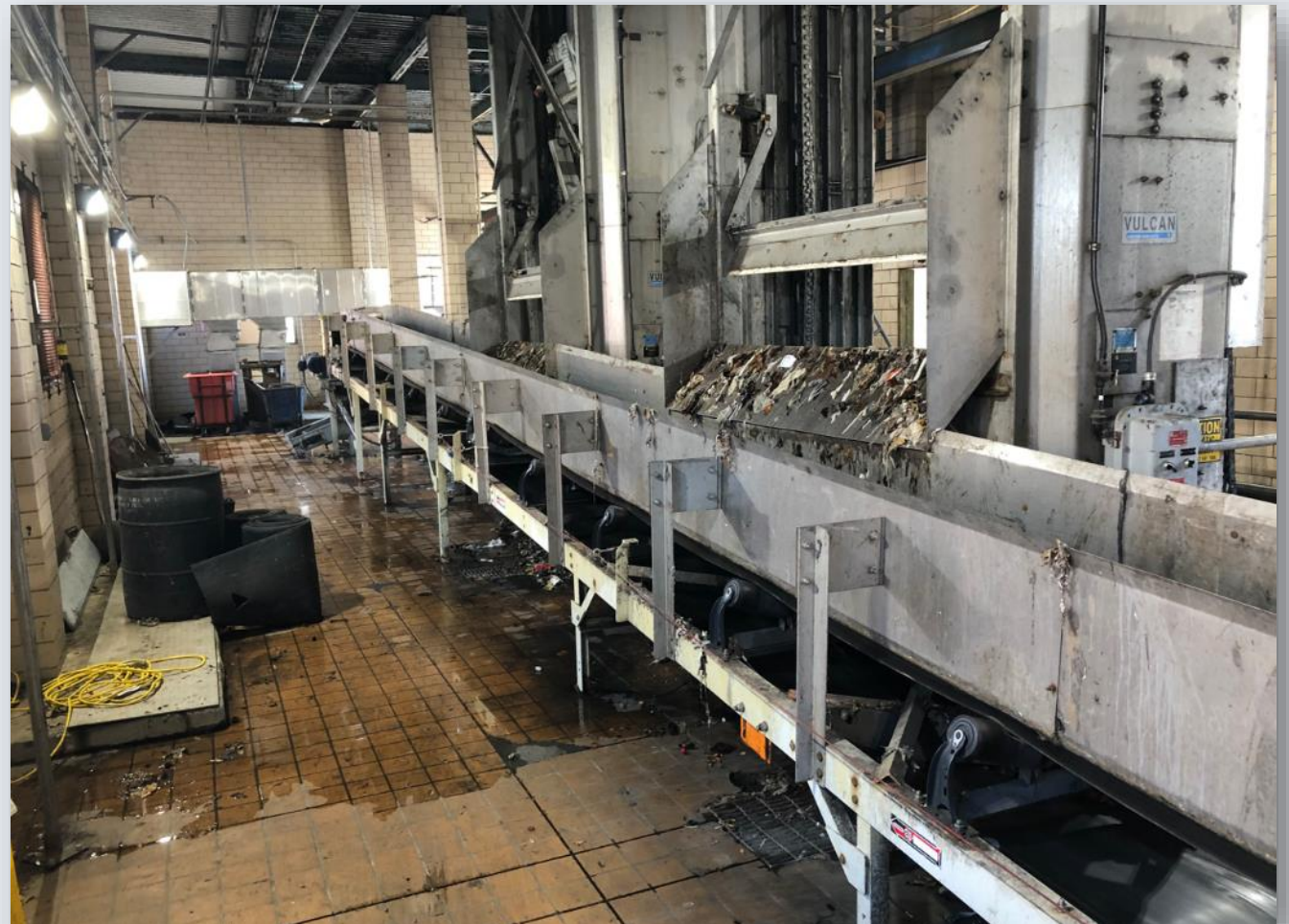
Existing Screenings Conveyor
