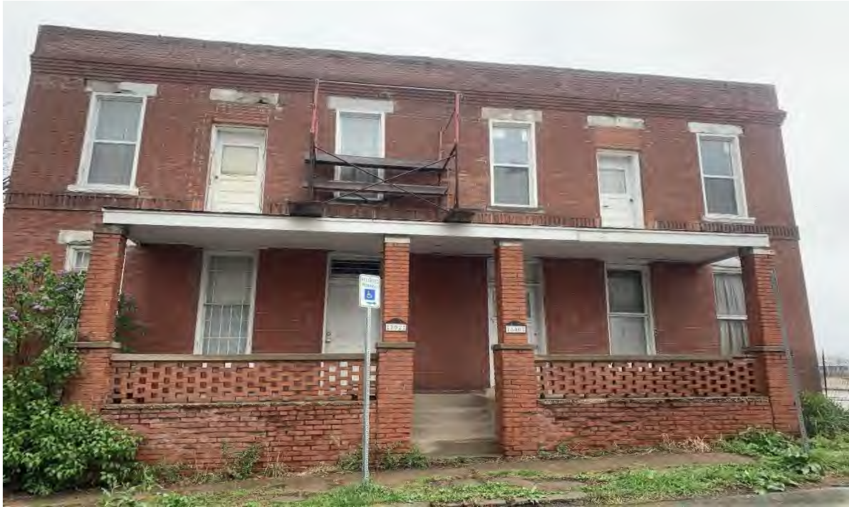
Figure 5. 802 W. 16th St. House in disrepair.
