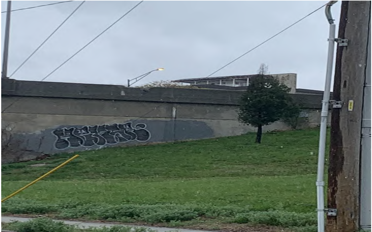
Figure 13. 20th and Washington. Graffiti on freeway wall
