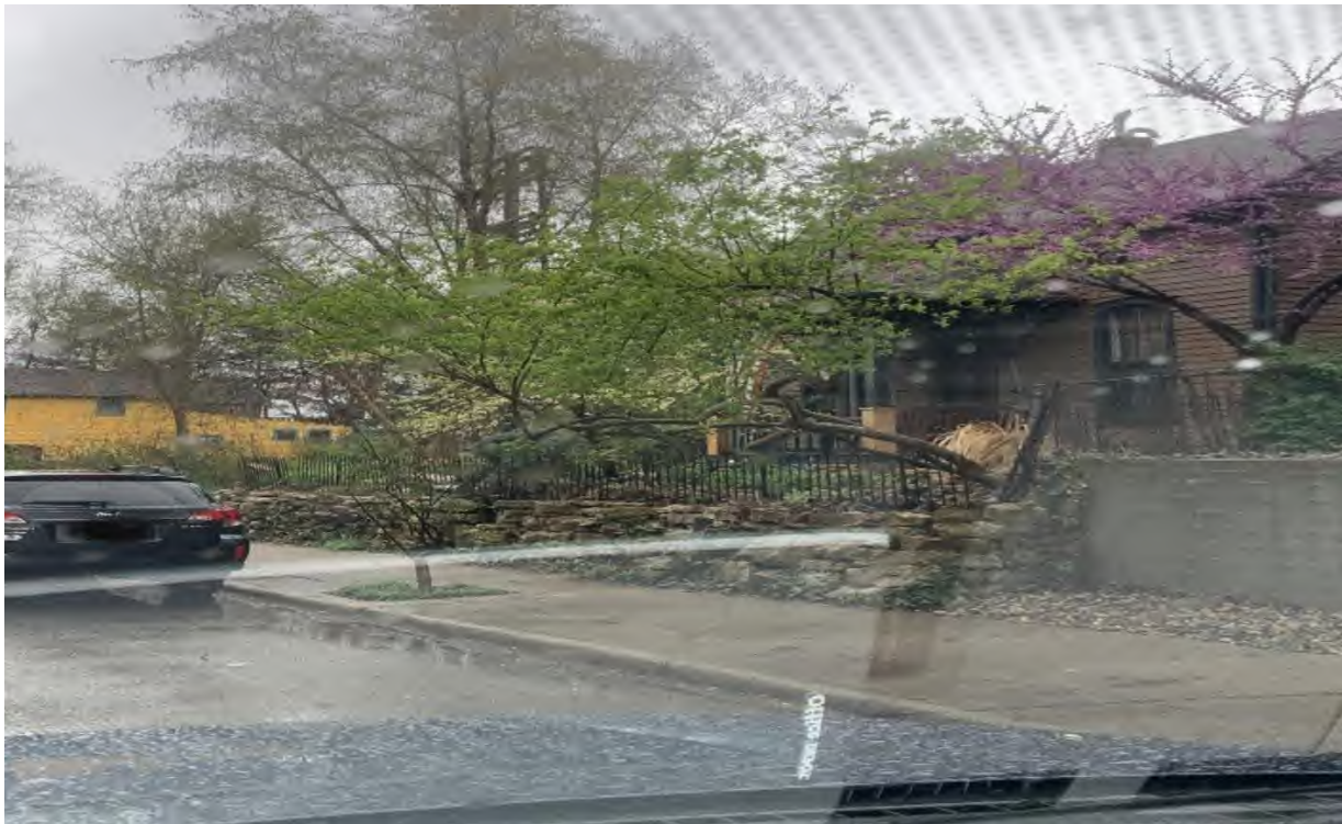
Figure 8. 1601 Madison Ave. Tree growing over into sidewalk.
