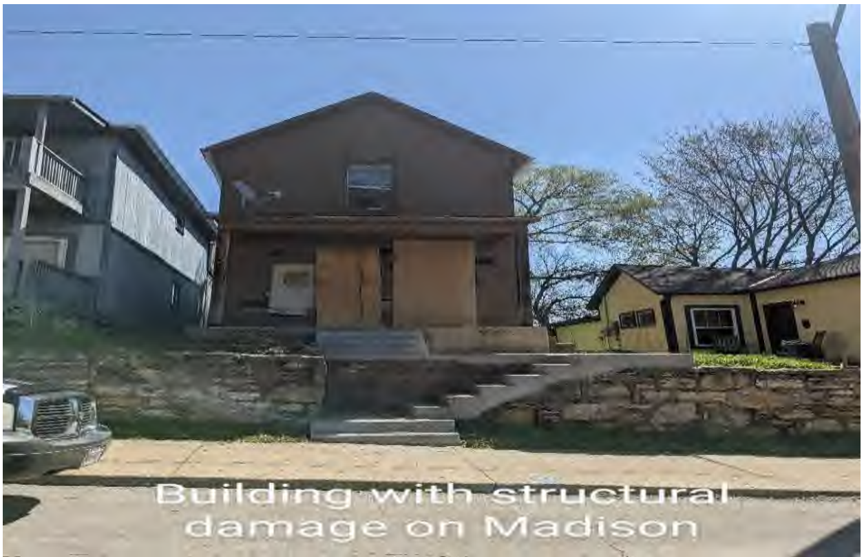
Figure 12. 2141 Madison Ave. Disrepair.
