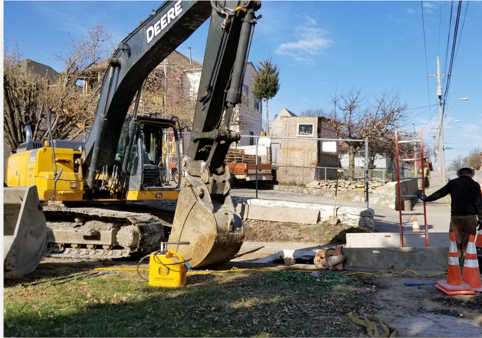
Contractor performing an open cut point repair of a sanitary sewer main.
