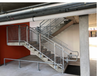
GALVANIZED STEEL GUARDRAIL WITH MESH INFILL
