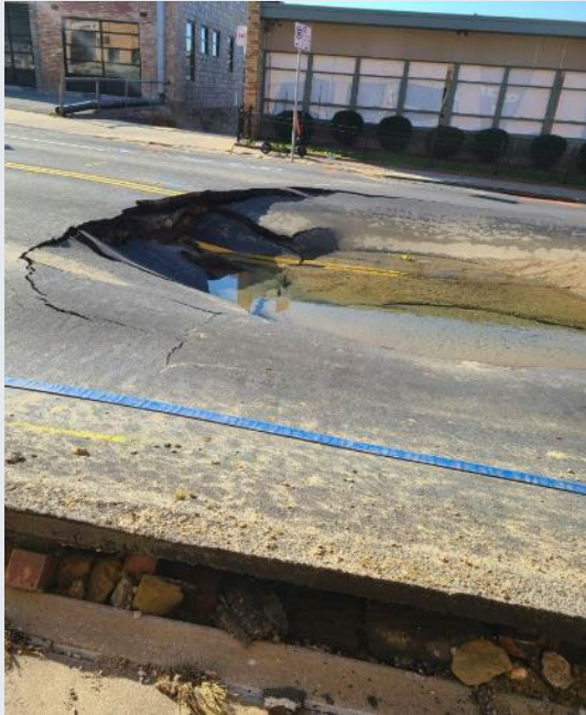
Street collapse due to a water main break
