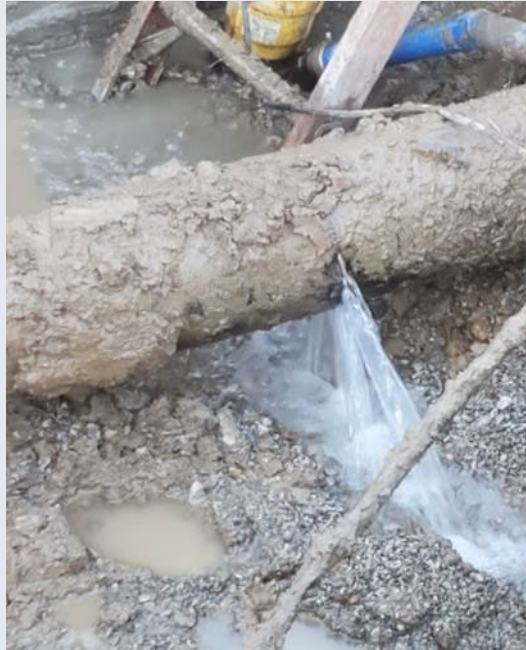
Broken water main leaking
