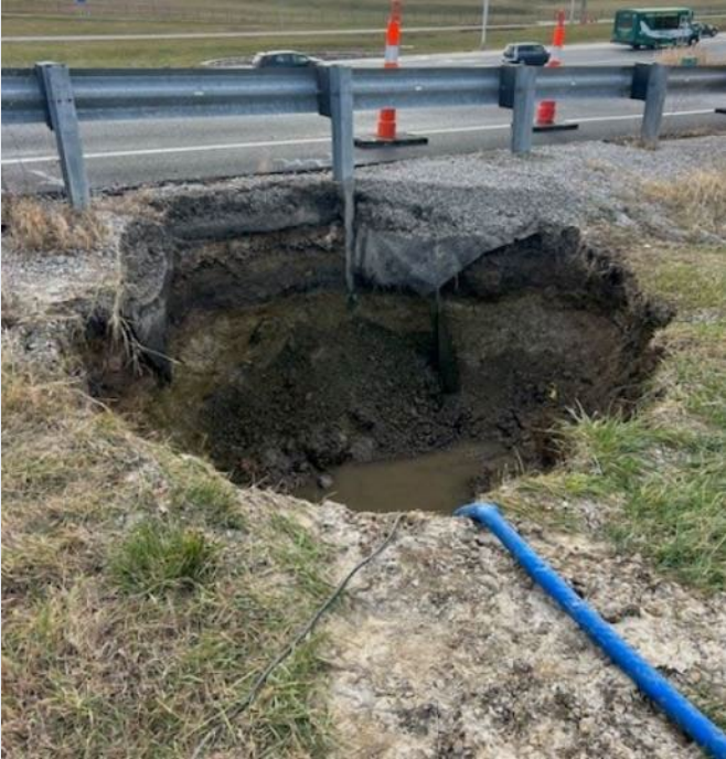
Water Main Break Aftermath
