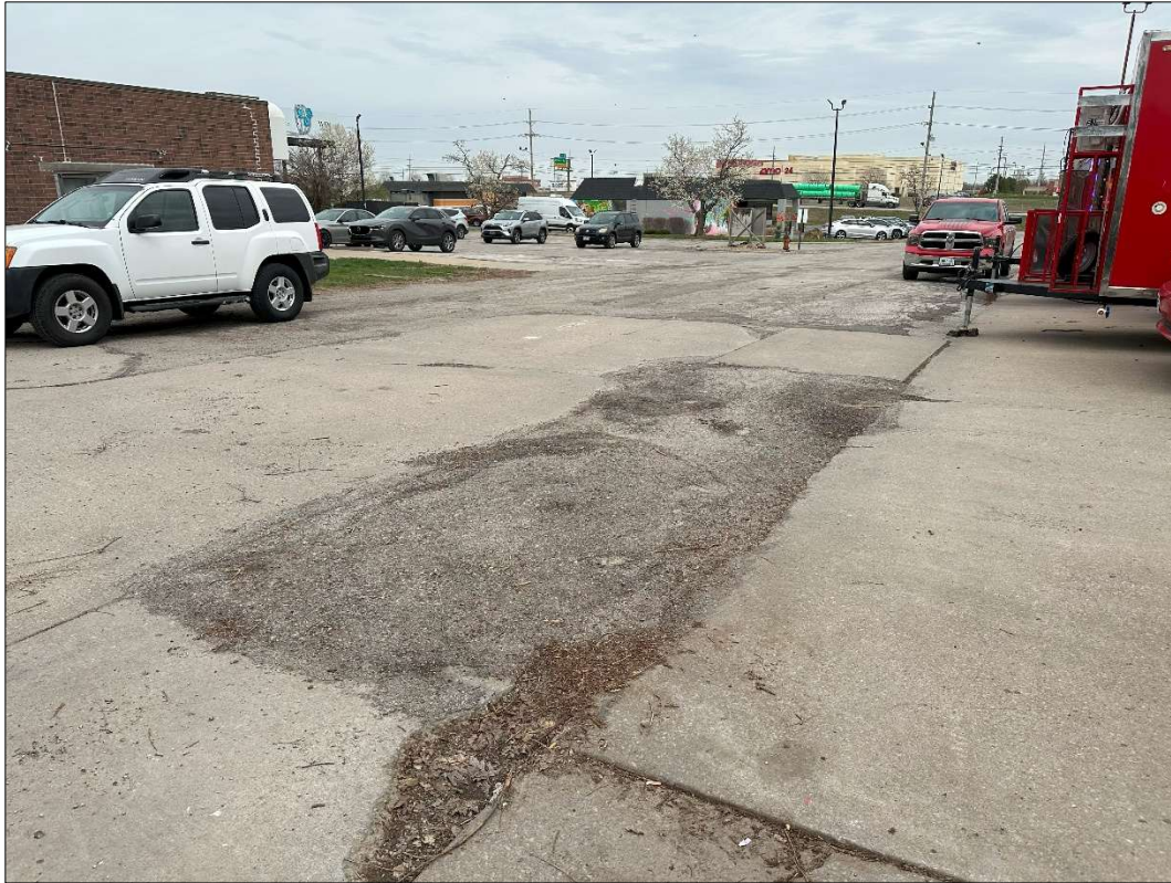
Tiffany Plaza – looking northeast – deterioration of pavement
