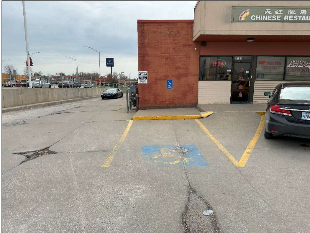
Frolics Plaza – looking southwest – Substandard ADA curb ramp; damaged sidewalk; deterioration of drive
