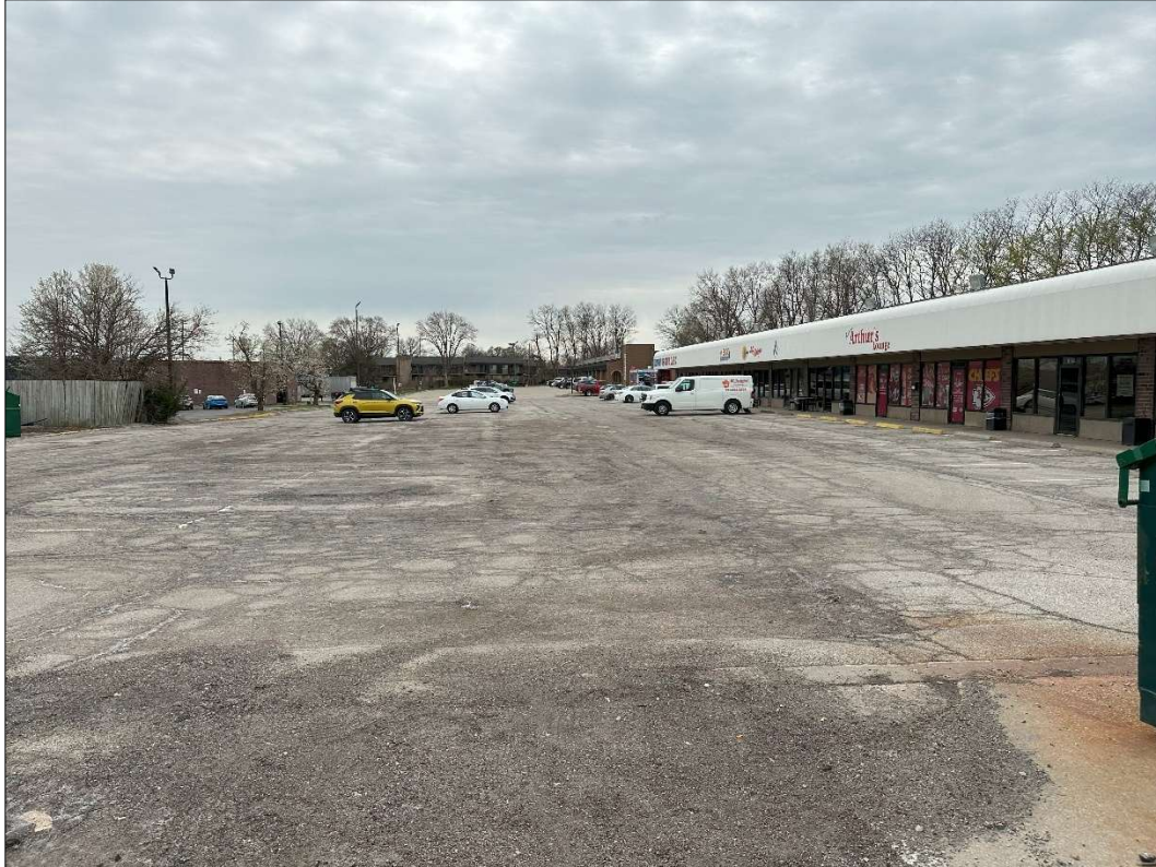
Tiffany Plaza – looking south – deterioration of parking lot, uneven pavement
