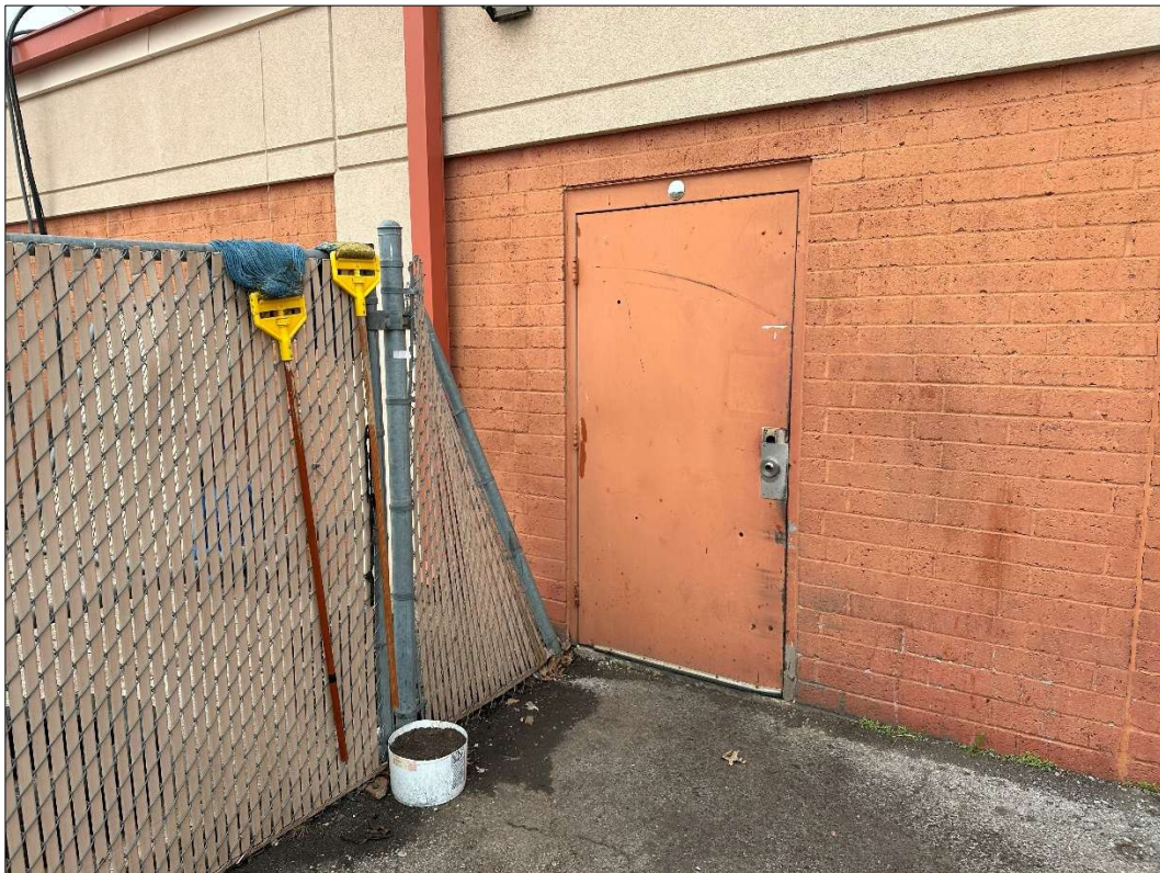
Frolics Plaza – looking north – deterioration of door; failure of finishes
