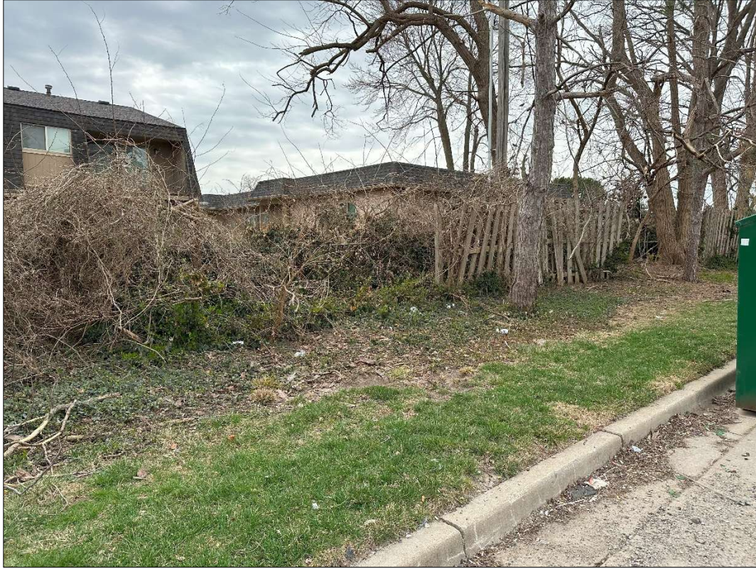
Tiffany Plaza – looking southwest – deterioration of fence; overgrown vegetation
