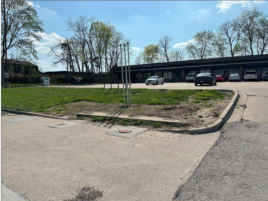
Tiffany Plaza – looking west – deterioration of pavement; lack of landscaping
