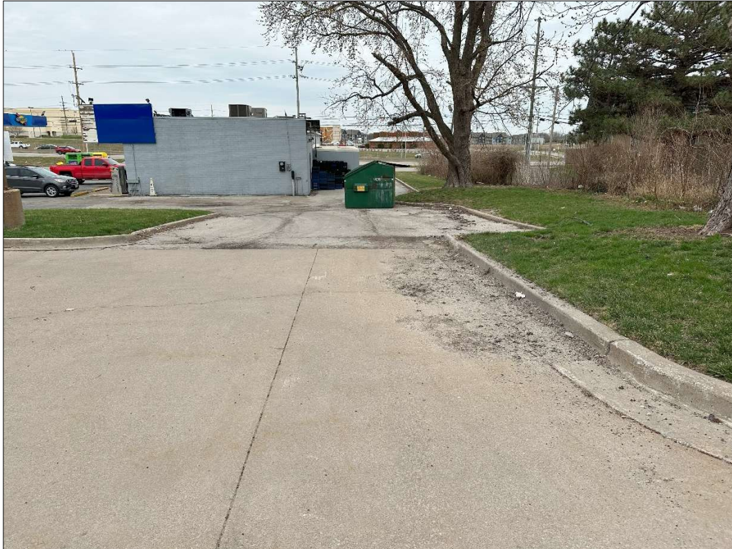
Tiffany Plaza – looking east – deterioration of pavement; unenclosed dumpsters
