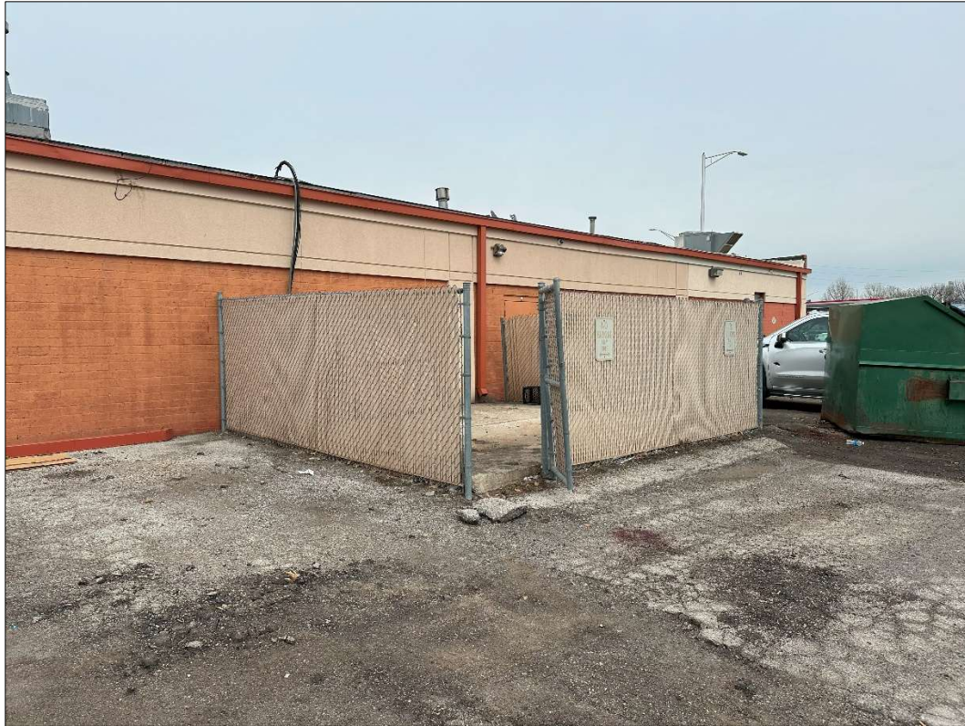
Frolics Plaza – looking northeast – deterioration of trash enclosure, pavement
