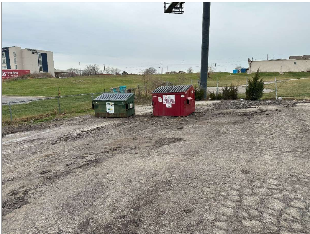
Frolics Plaza – looking west – deterioration of pavement
