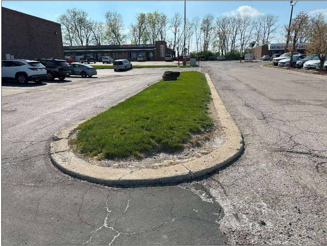
Tiffany Plaza – looking west – lack of landscaping; deterioration of pavement
