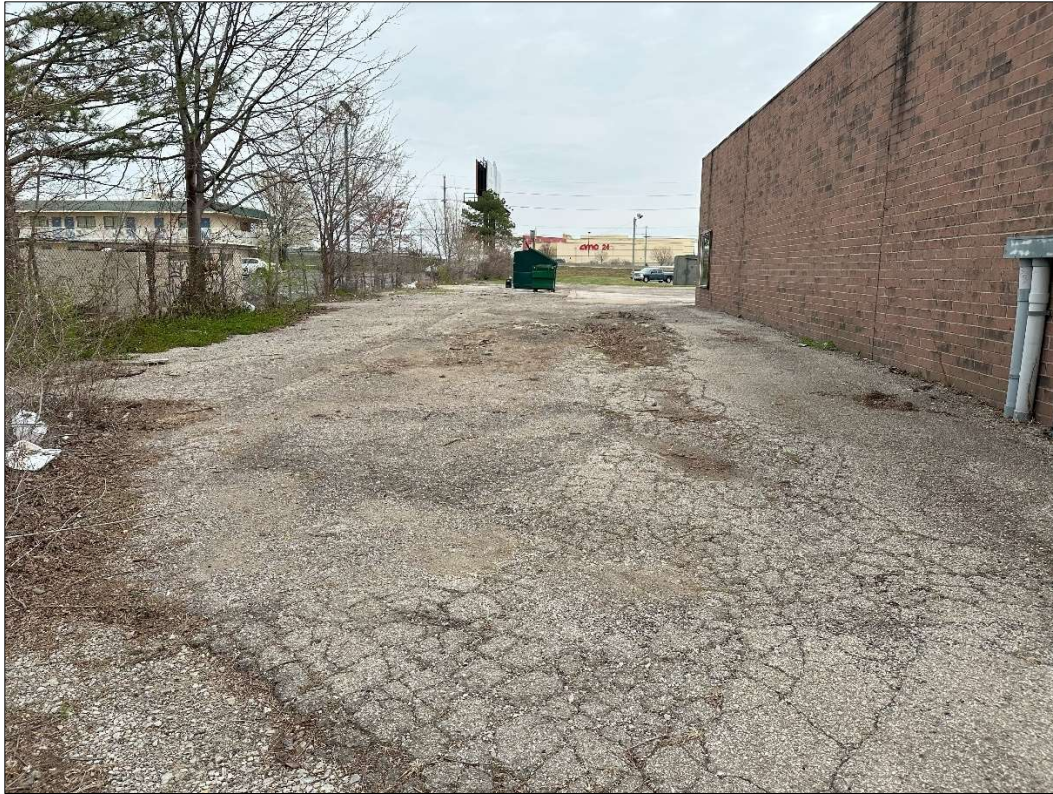
Tiffany Plaza – looking east – uneven pavement; overgrown vegetation
