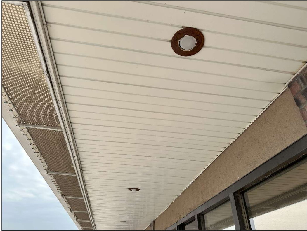
Tiffany Plaza – looking south – lighting needs upgrade to LEDs
