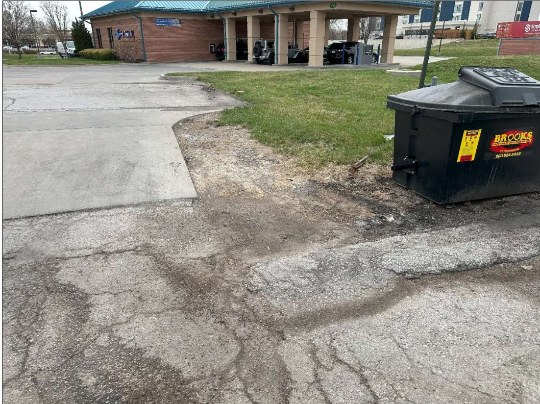
Frolics Plaza – looking south – deterioration of pavement; lack of landscaping, curb
