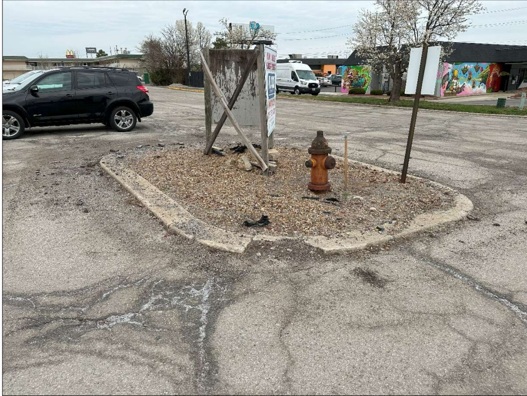
Tiffany Plaza – looking northeast – deterioration of pavement, curb; lack of landscaping
