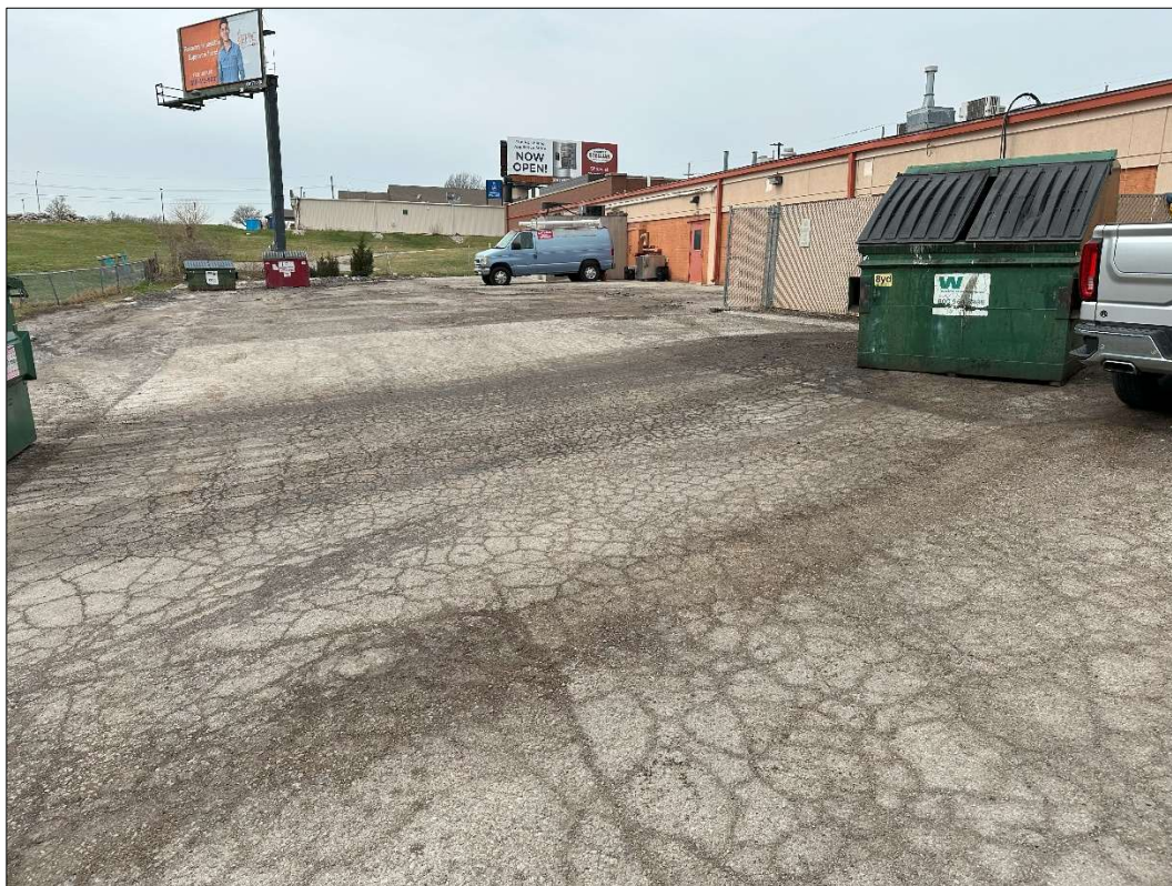
Frolics Plaza – looking west – deterioration of pavement
