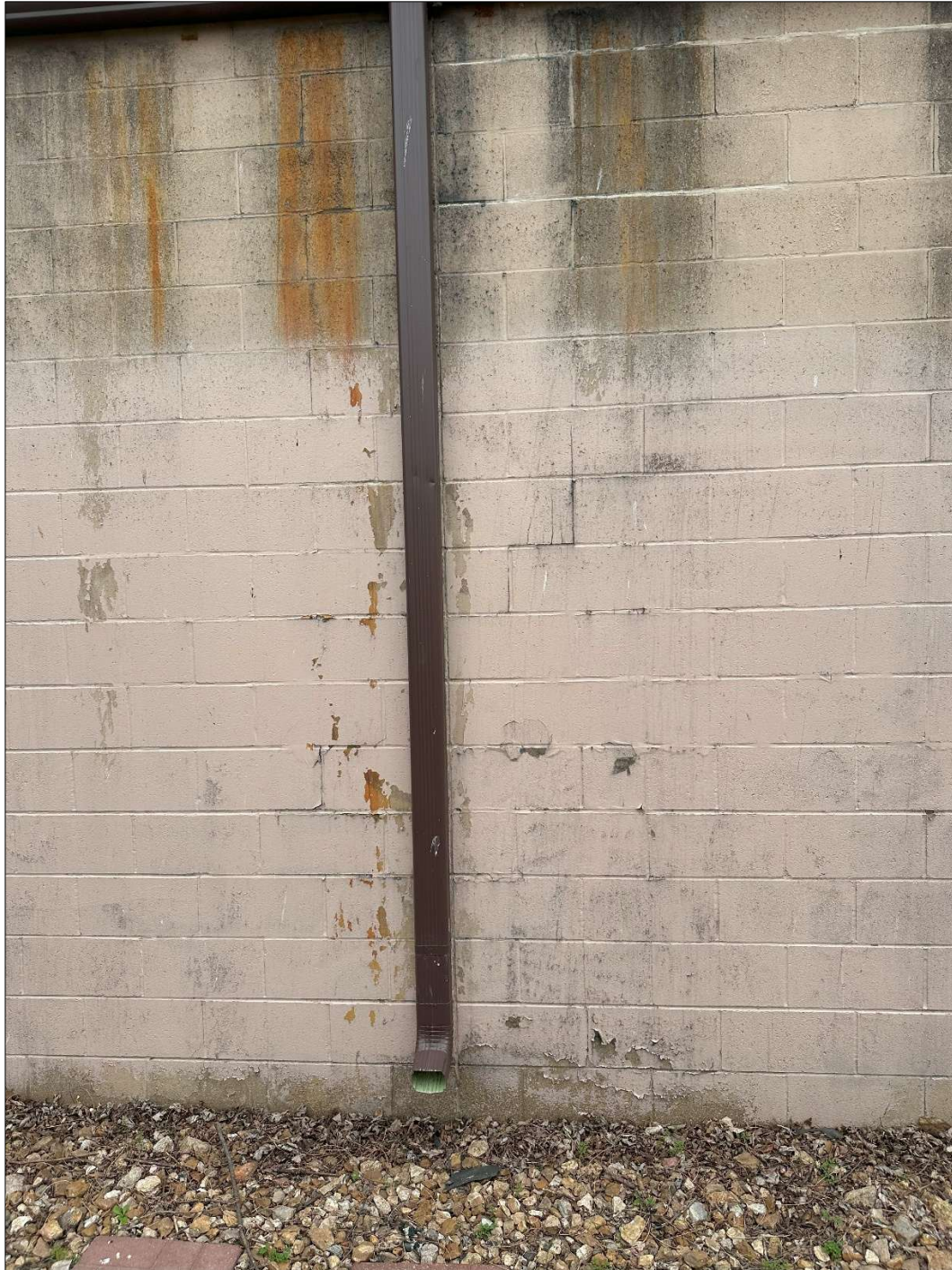
Tiffany Plaza – looking east – failure of finishes
