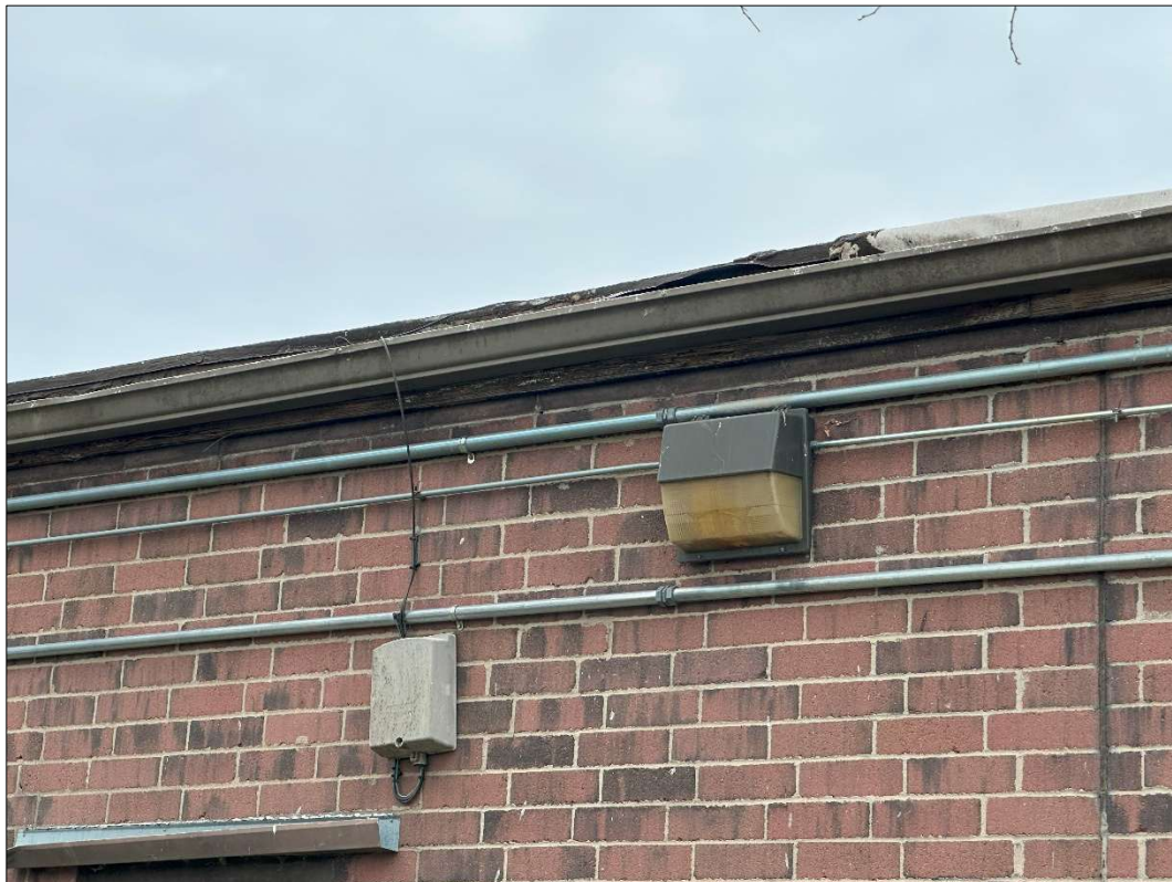
Tiffany Plaza – looking northeast – deterioration of light fixtures on west side of building
