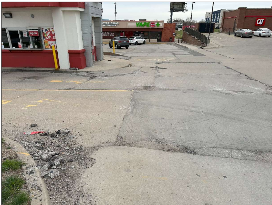
Frolics Plaza – looking south – deterioration of pavement
