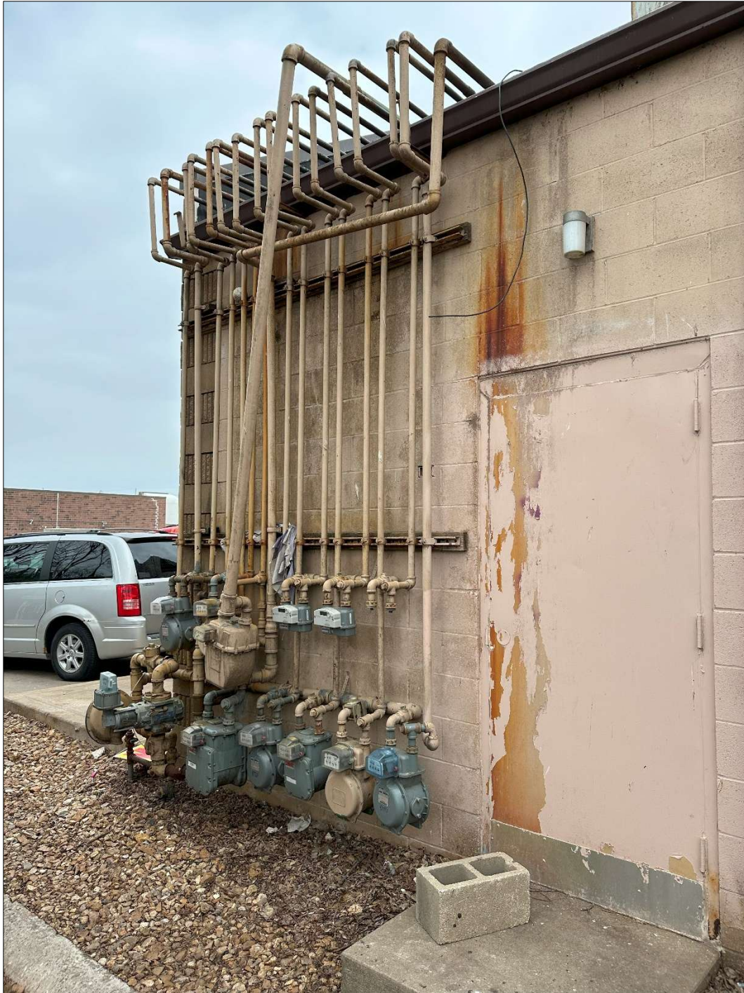
Tiffany Plaza – looking northeast – failure of finishes; deterioration of door
