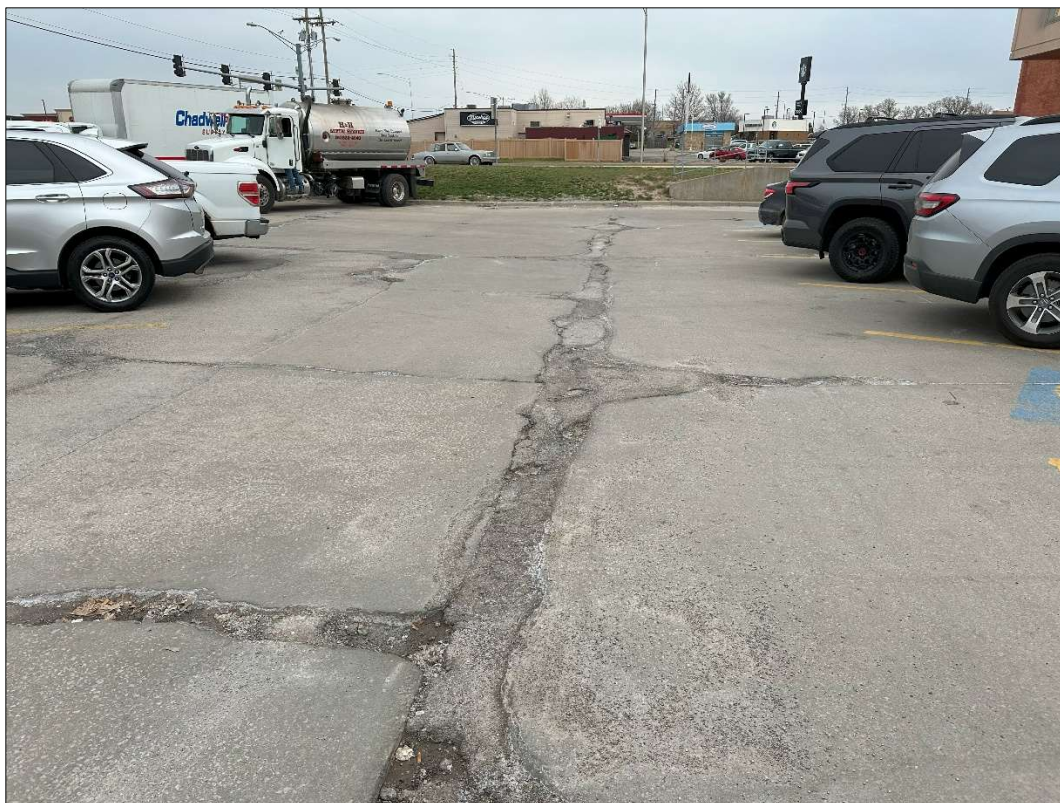
Frolics Plaza – looking east – deterioration of pavement
