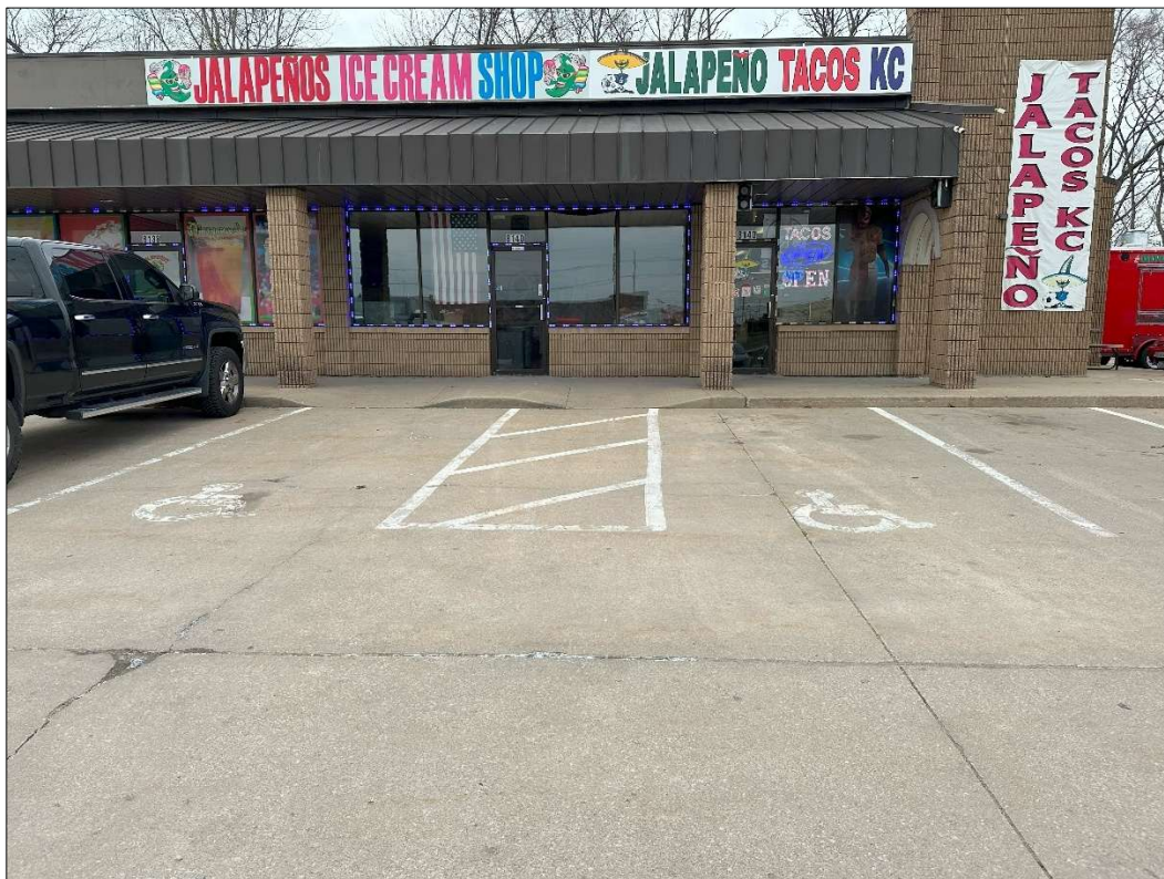
Tiffany Plaza – looking west – lack of ADA compliant signage, access to sidewalk
