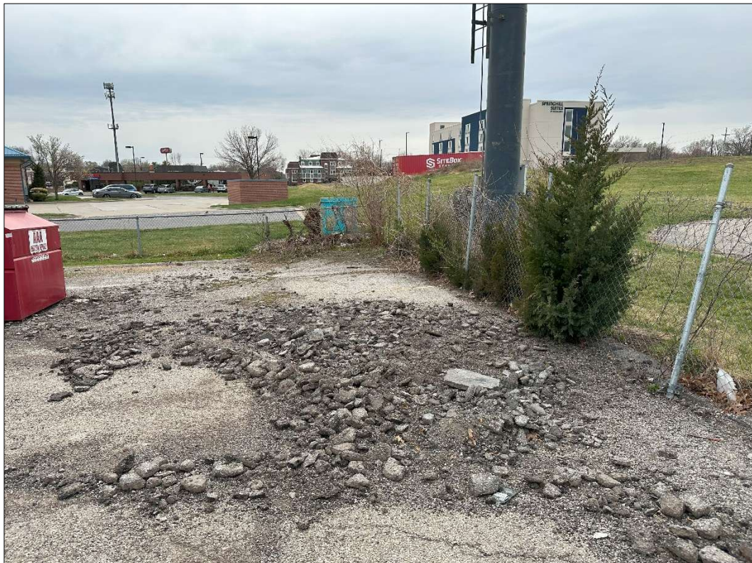
Frolics Plaza – looking south – deterioration of pavement, fence; neglected vegetation
