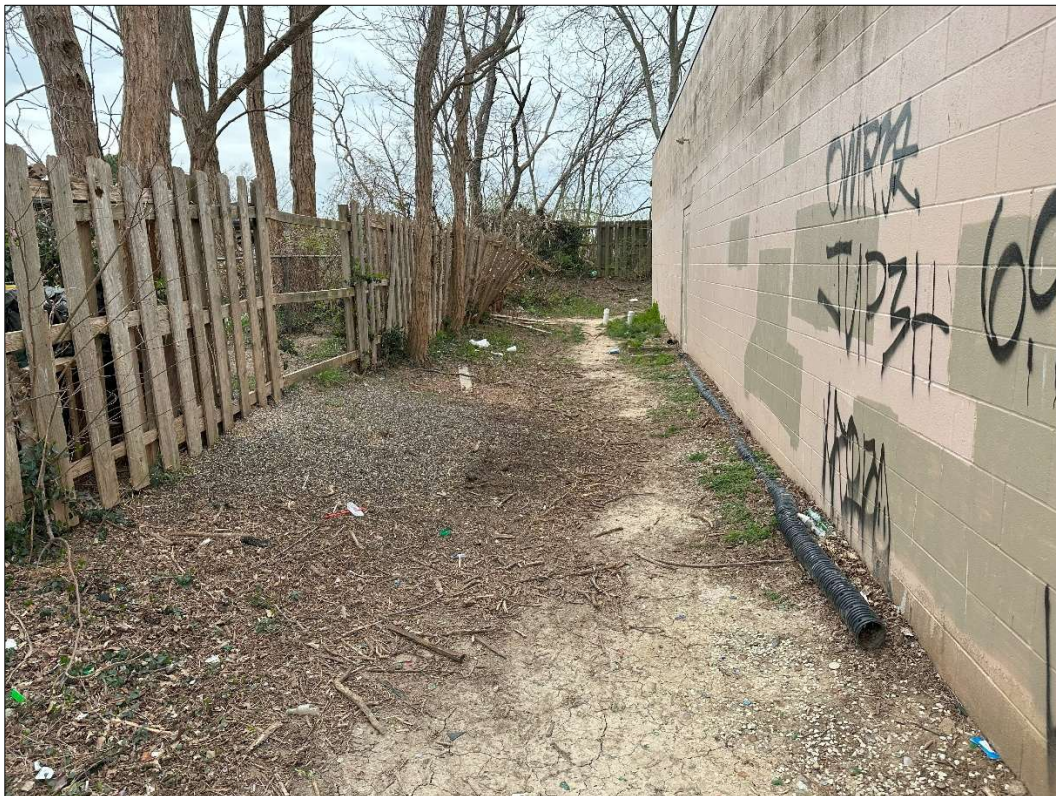
Tiffany Plaza – looking west – deterioration of fence; lack of landscaping
