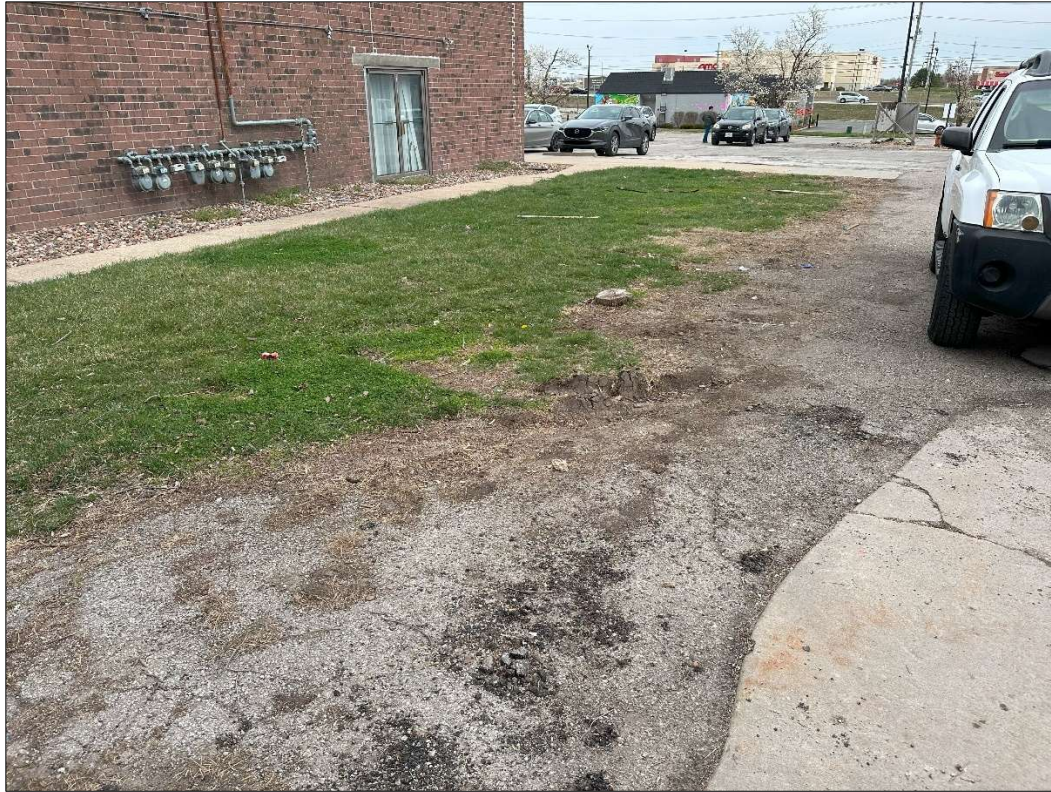
Tiffany Plaza – looking east – uneven pavement
