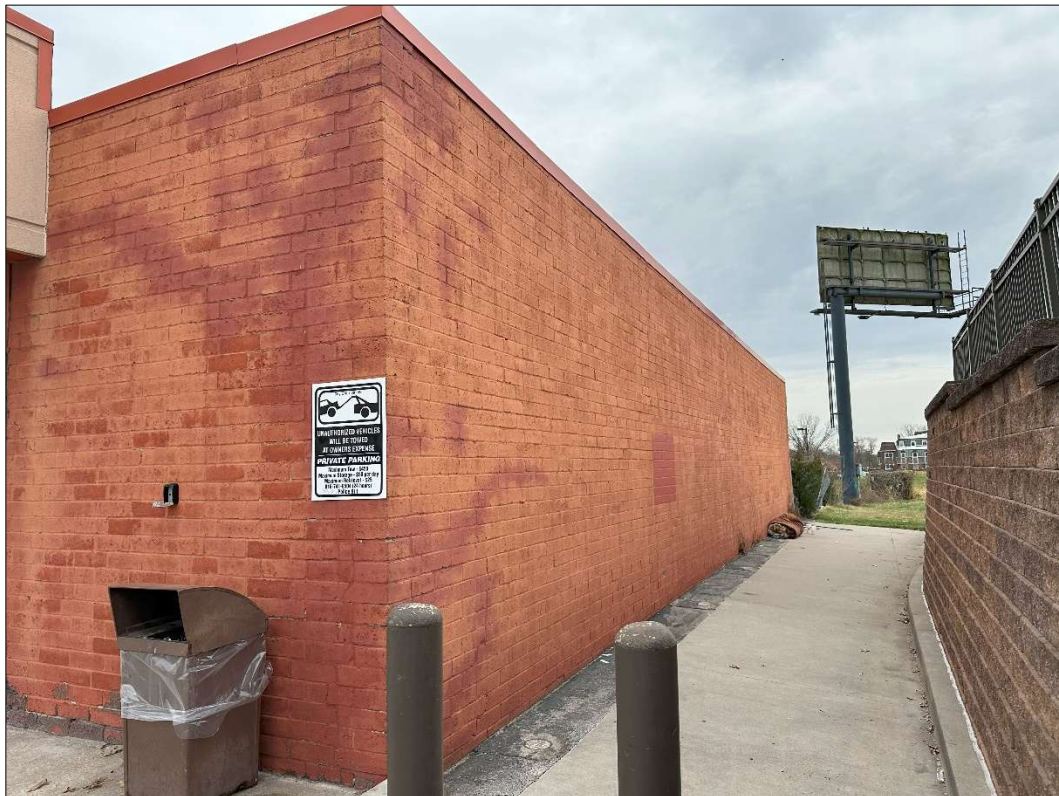
Frolics Plaza – looking south – failure of finishes; masonry tuckpointing required
