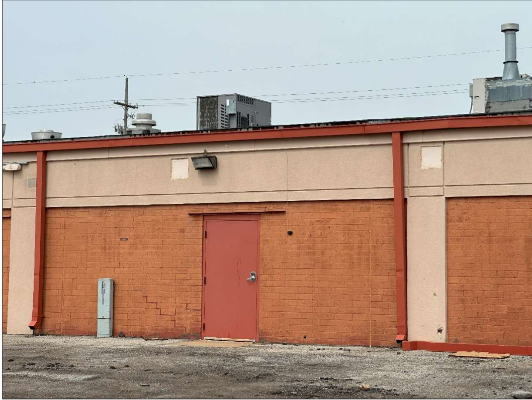
Frolics Plaza – looking north – failure of finishes; masonry tuckpointing required
