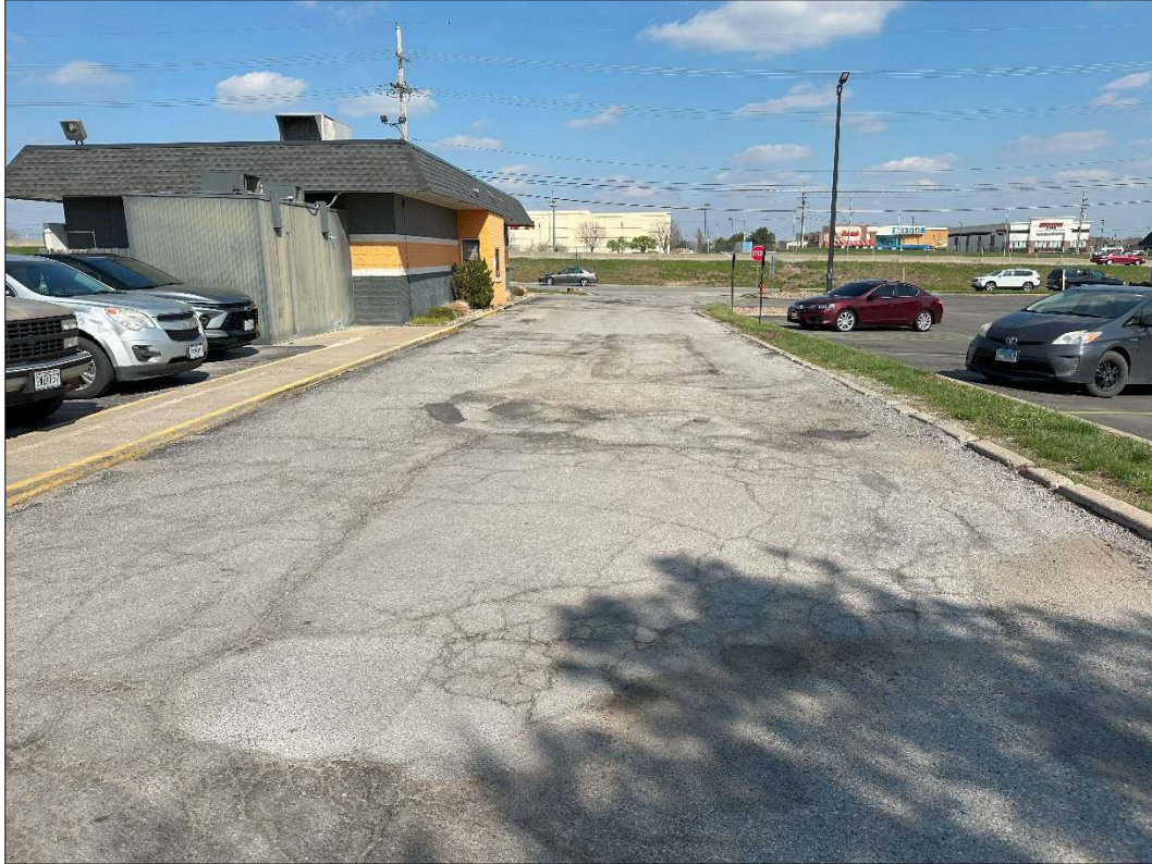
Tiffany Plaza – looking east – deterioration of pavement at In-A-Tub
