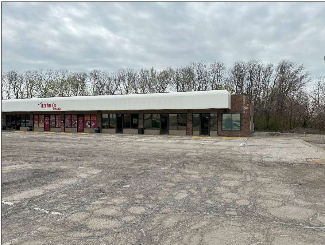
Tiffany Plaza – looking west – deterioration of pavement
