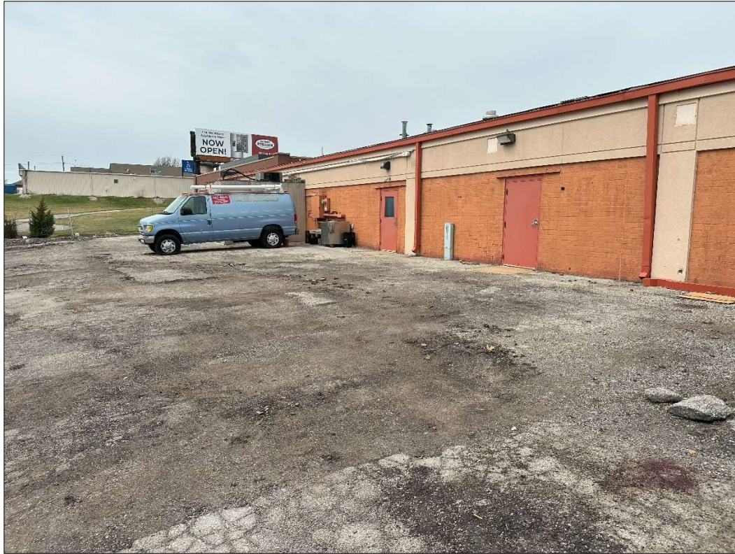
Frolics Plaza – looking northwest – deterioration of pavement, trash/debris
