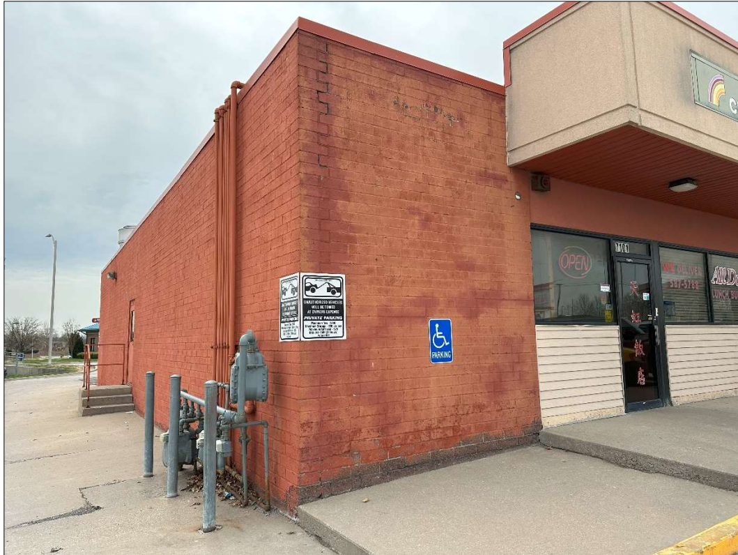
Frolics Plaza – looking southwest – failure of finishes (masonry, EIFS); tuckpointing necessary
