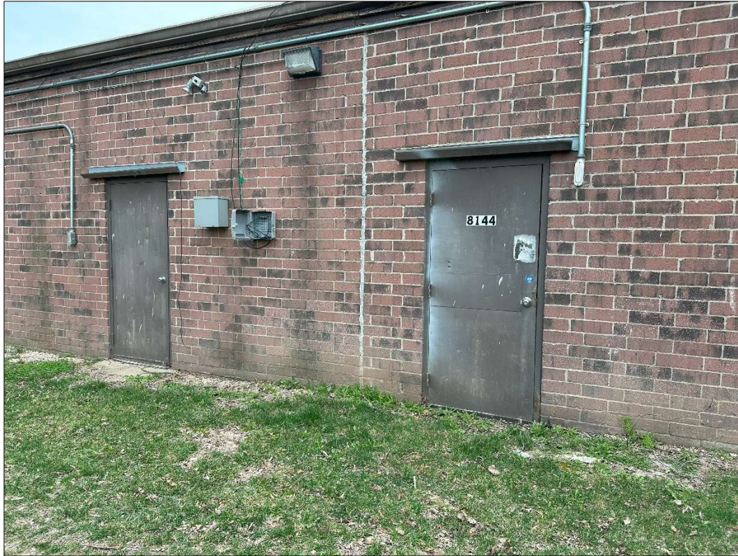
Tiffany Plaza – looking northeast – deterioration of rear entry doors, awnings; failure of finishes
