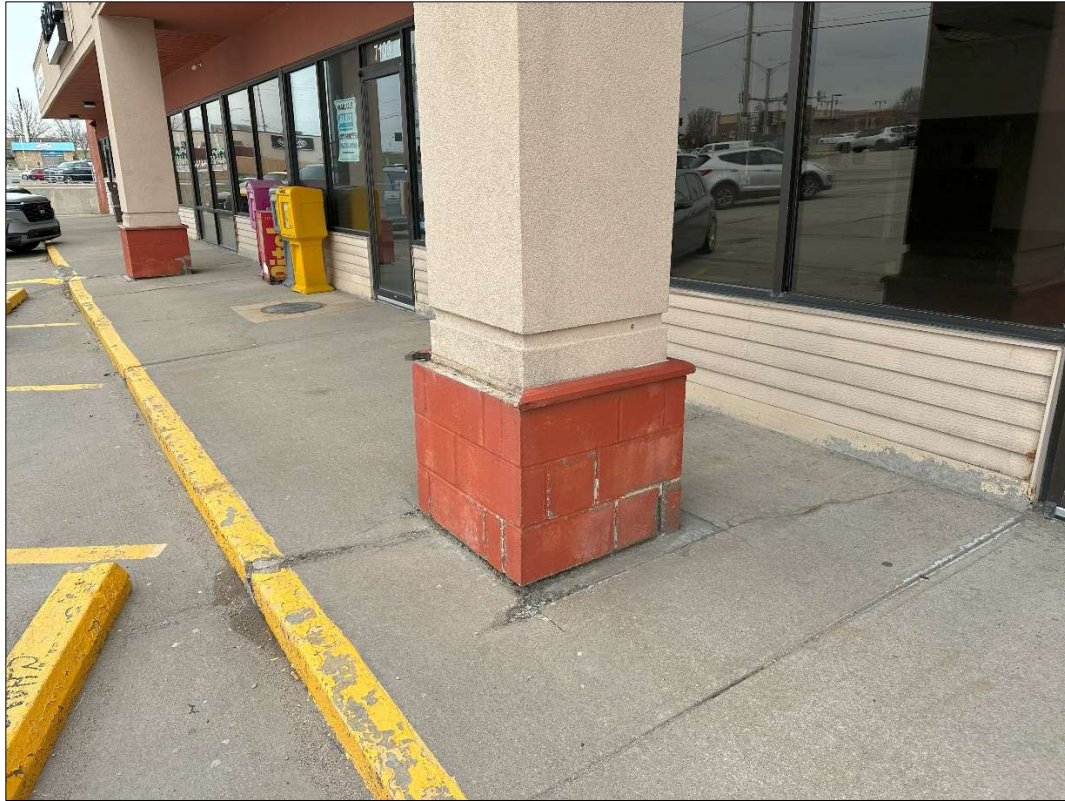
Frolics Plaza – looking southeast – failure of finishes; deterioration of masonry
