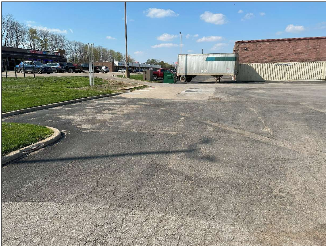
Tiffany Plaza – looking north – deterioration of pavement; lack of landscaping at Sunoco/World Liquors
