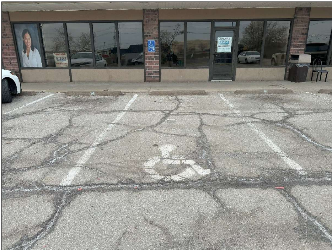
Tiffany Plaza – looking west – lack of ADA compliant access to sidewalk
