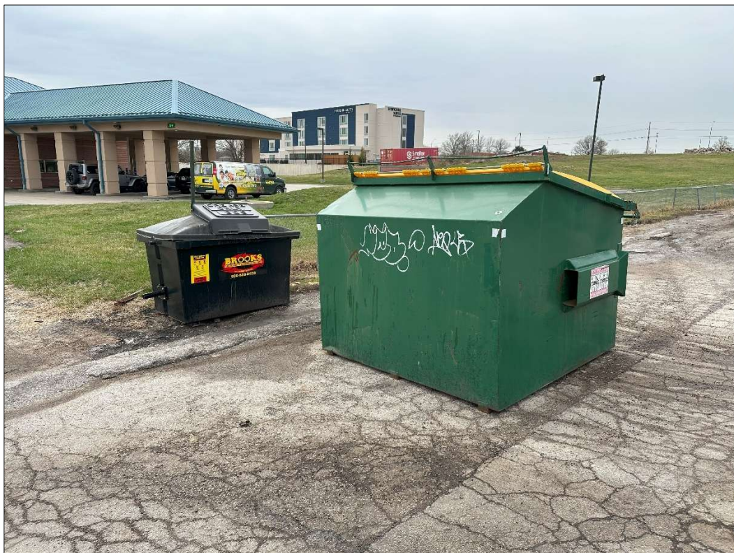
Frolics Plaza – looking southwest – graffiti; deterioration of pavement
