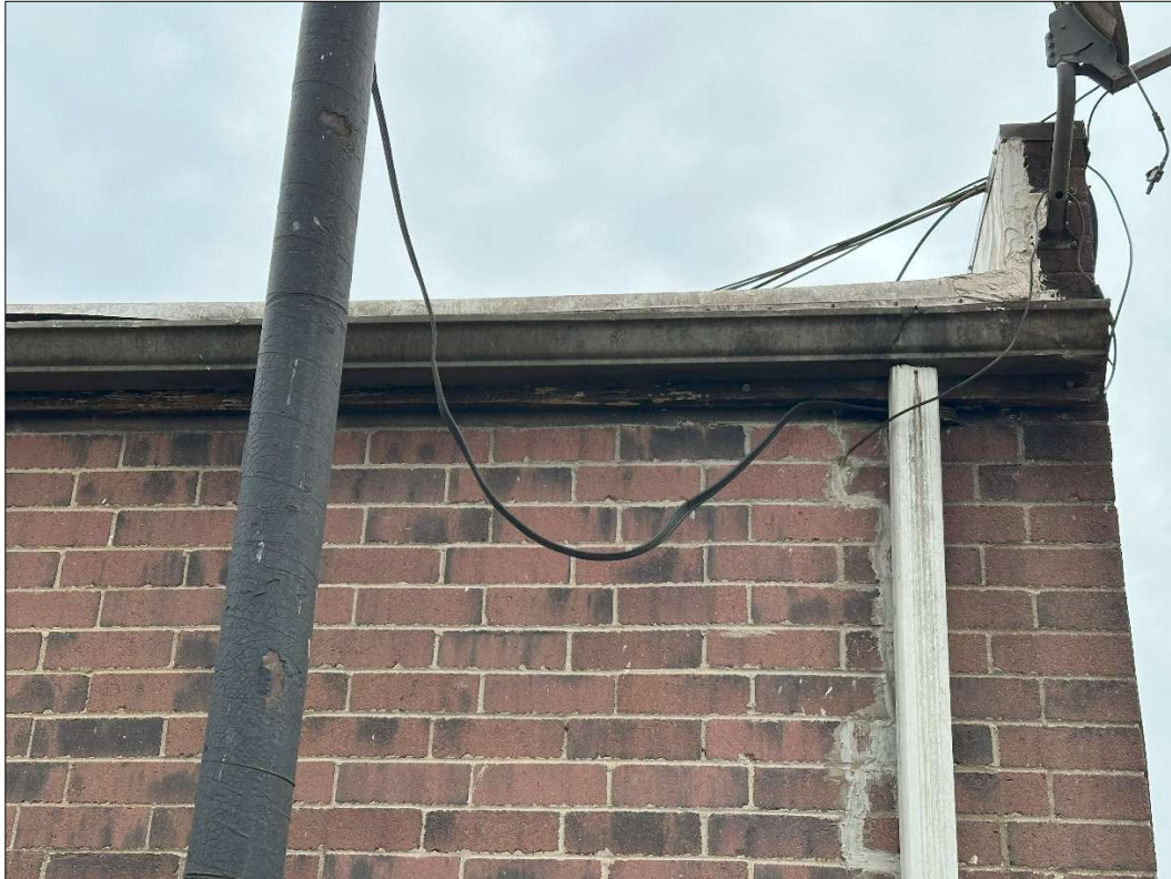
Tiffany Plaza – looking east – deterioration of gutters, downspouts
