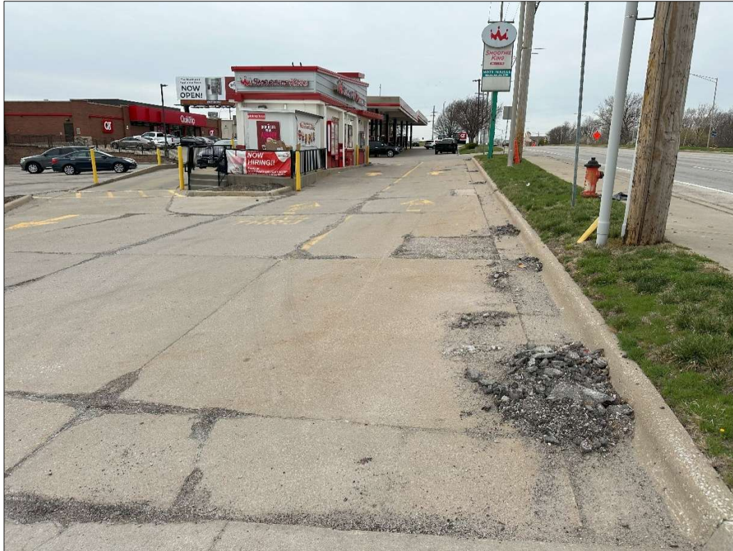
Frolics Plaza – looking west – deterioration of pavement
