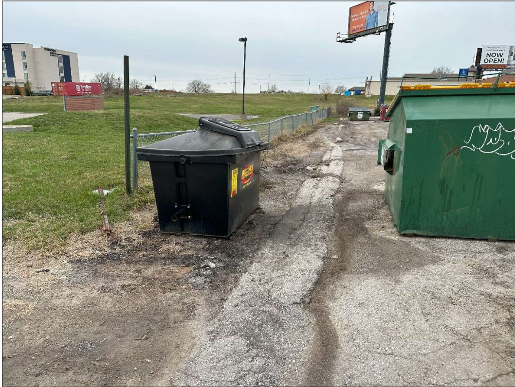
Frolics Plaza – looking southwest – deterioration of pavement, fence; unenclosed dumpsters; lack of landscaping
