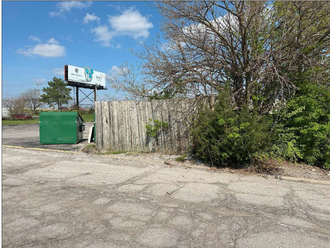
Tiffany Plaza – looking east – deterioration of trash enclosure at In-A-Tub, pavement; lack of landscaping
