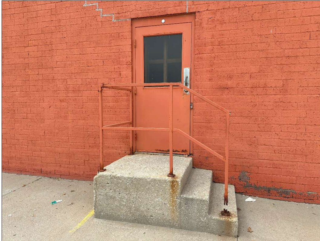
Frolics Plaza – looking west – deterioration of railing, steps
