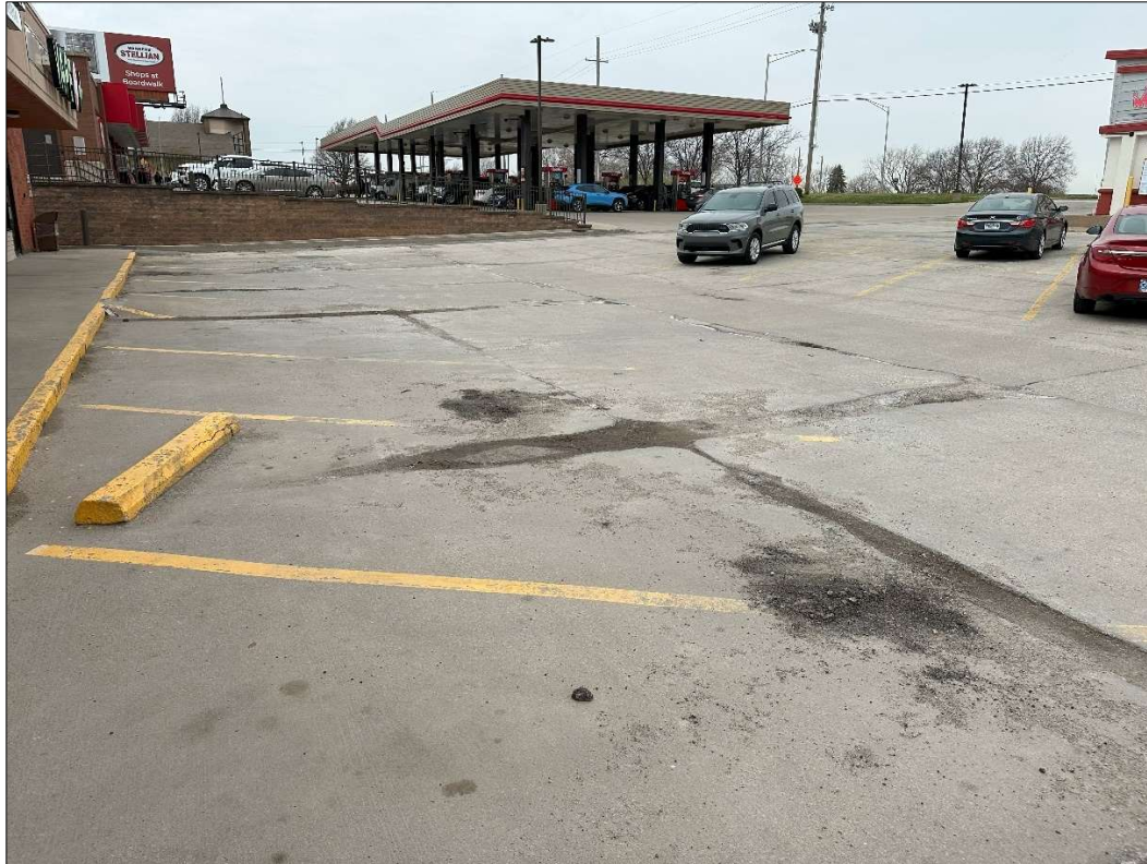
Frolics Plaza – looking west – tripping hazards due to deterioration of pavement
