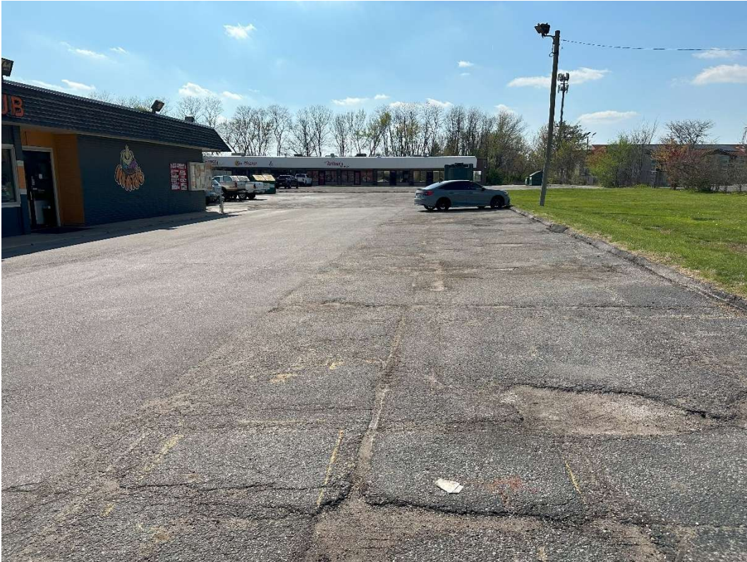
Tiffany Plaza – looking west – deteriorated surface parking lot – uneven pavement
