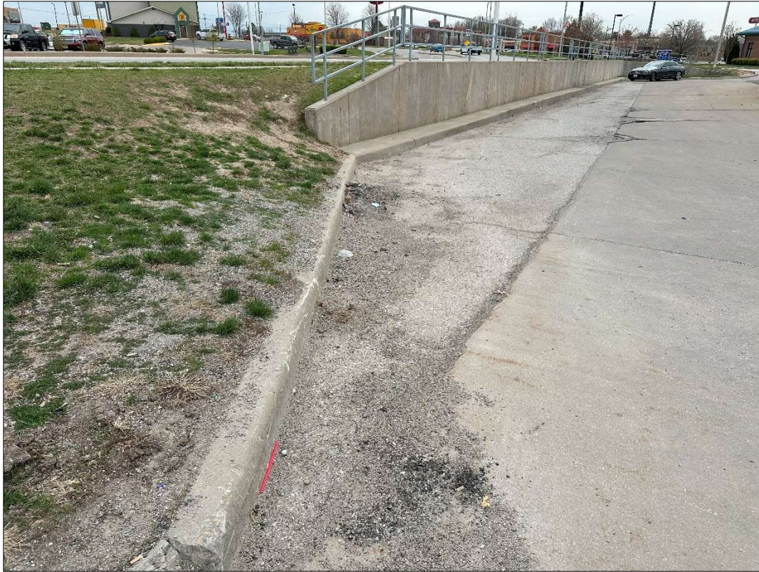
Frolics Plaza – looking southeast – deterioration of pavement
