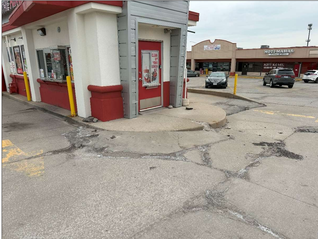
Frolics Plaza – looking southeast – deterioration of pavement; trash/debris
