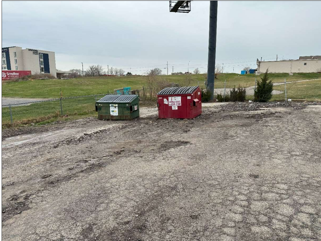
Frolics Plaza – looking west – deterioration of pavement; unenclosed dumpsters
