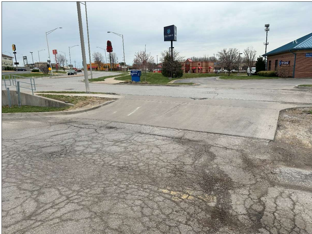
Frolics Plaza – looking southeast – deterioration of pavement; lack of curb, landscaping
