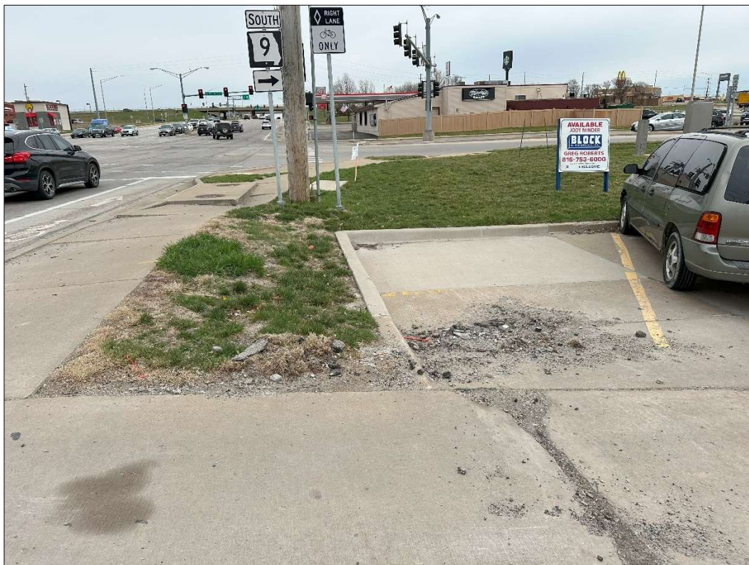
Frolics Plaza – looking east – uneven pavement; trash/debris
