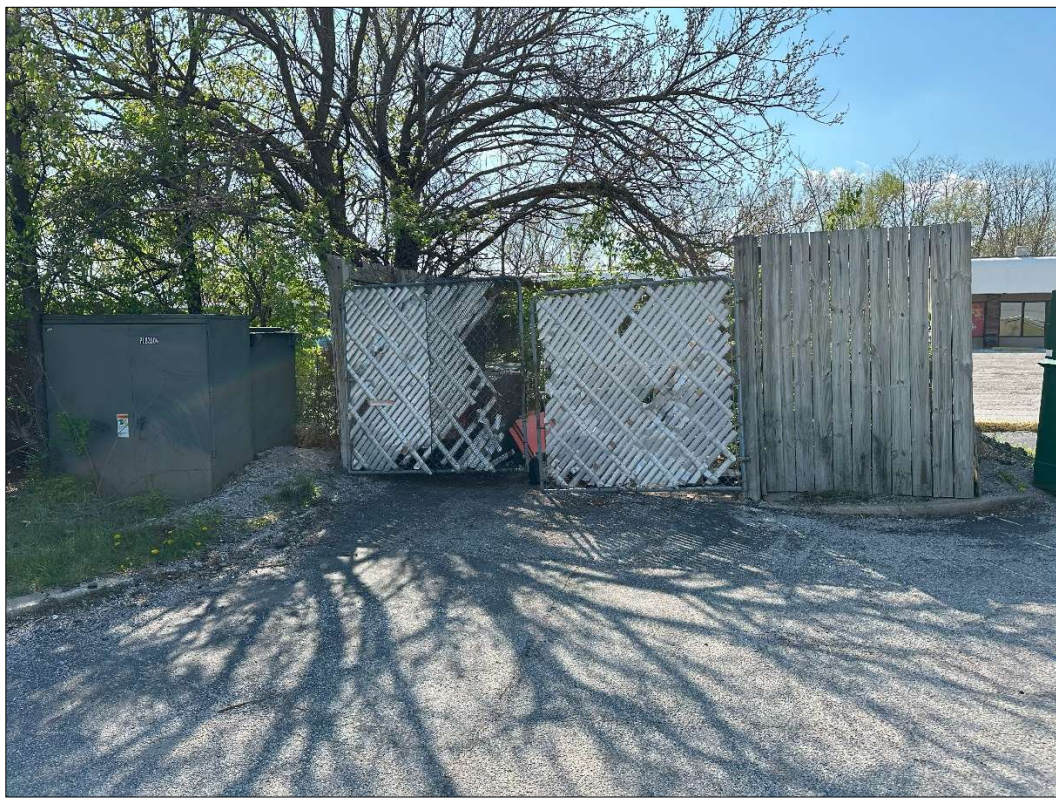
Tiffany Plaza – looking west – deterioration of trash enclosure at In-A-Tub
