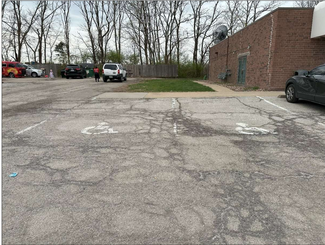
Tiffany Plaza – looking west – uneven pavement; lack of ADA signage
