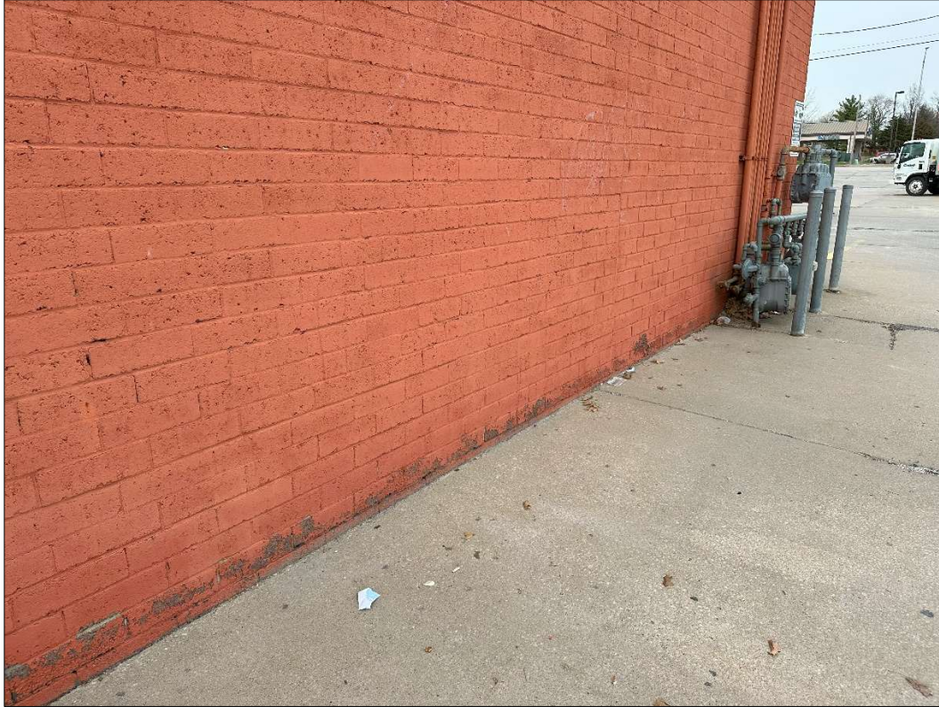
Frolics Plaza – looking northwest – failure of finishes
