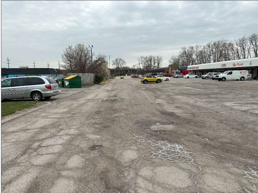
Tiffany Plaza – looking south – deterioration of pavement; unenclosed dumpsters
