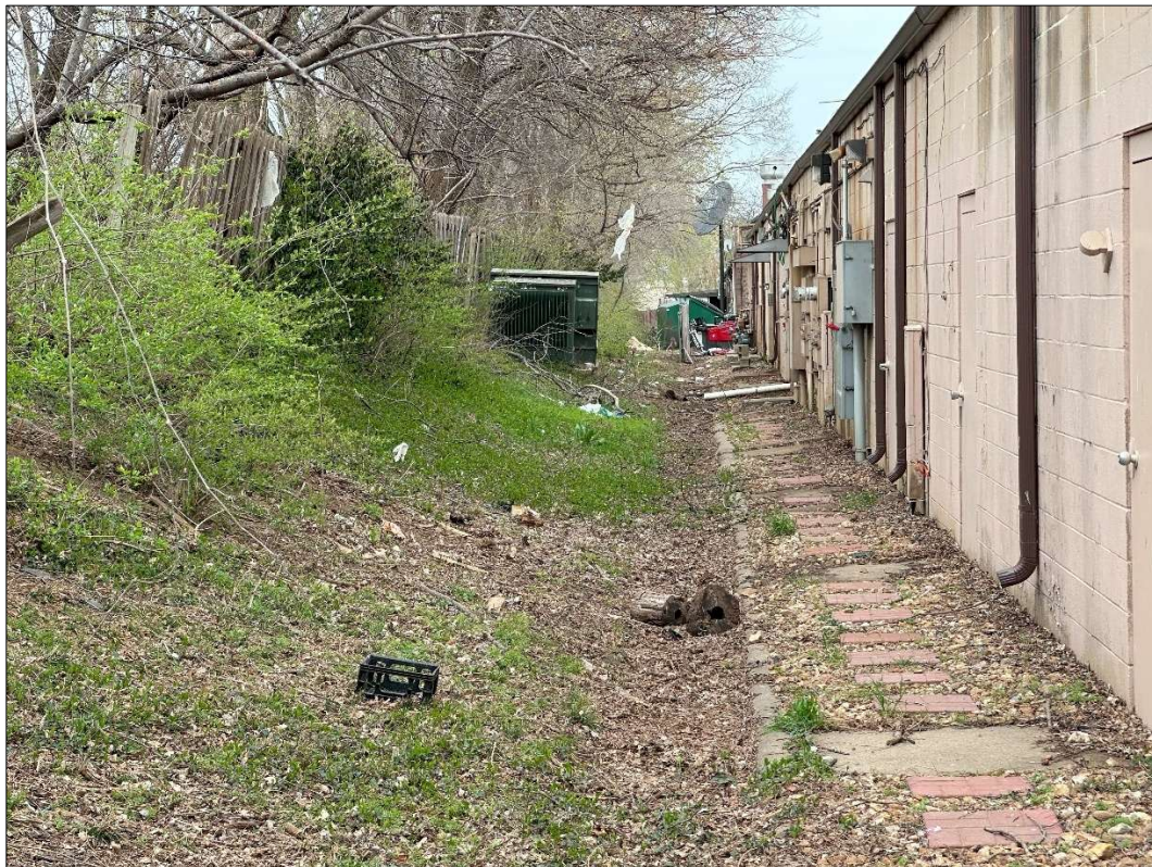
Tiffany Plaza – looking north – trash/debris; overgrown vegetation; deterioration of sidewalk
