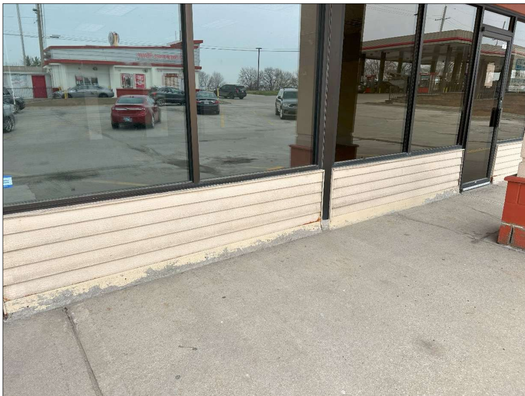
Frolics Plaza – looking south – failure of finishes; damaged door
