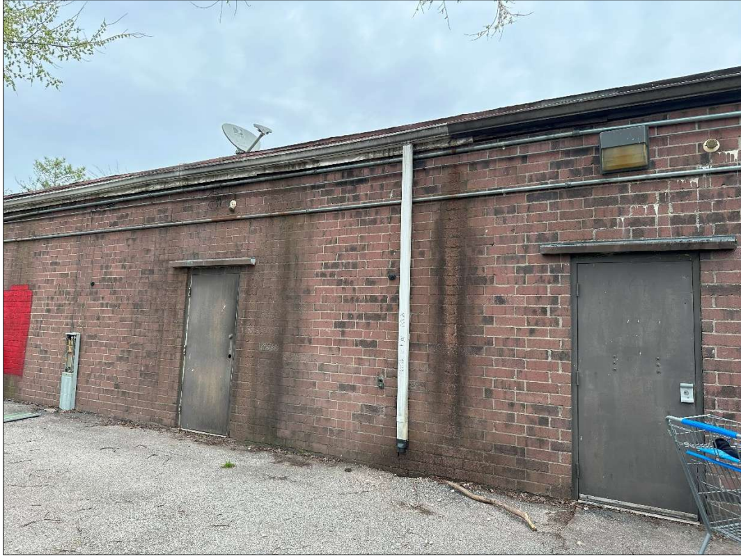
Tiffany Plaza – looking northeast – deterioration of rear entry doors, awnings, gutters, downspouts
