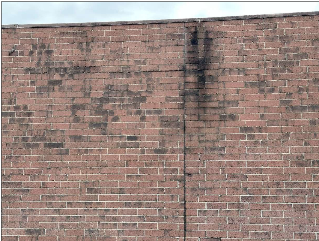
Tiffany Plaza – looking south – tuckpointing of masonry required
