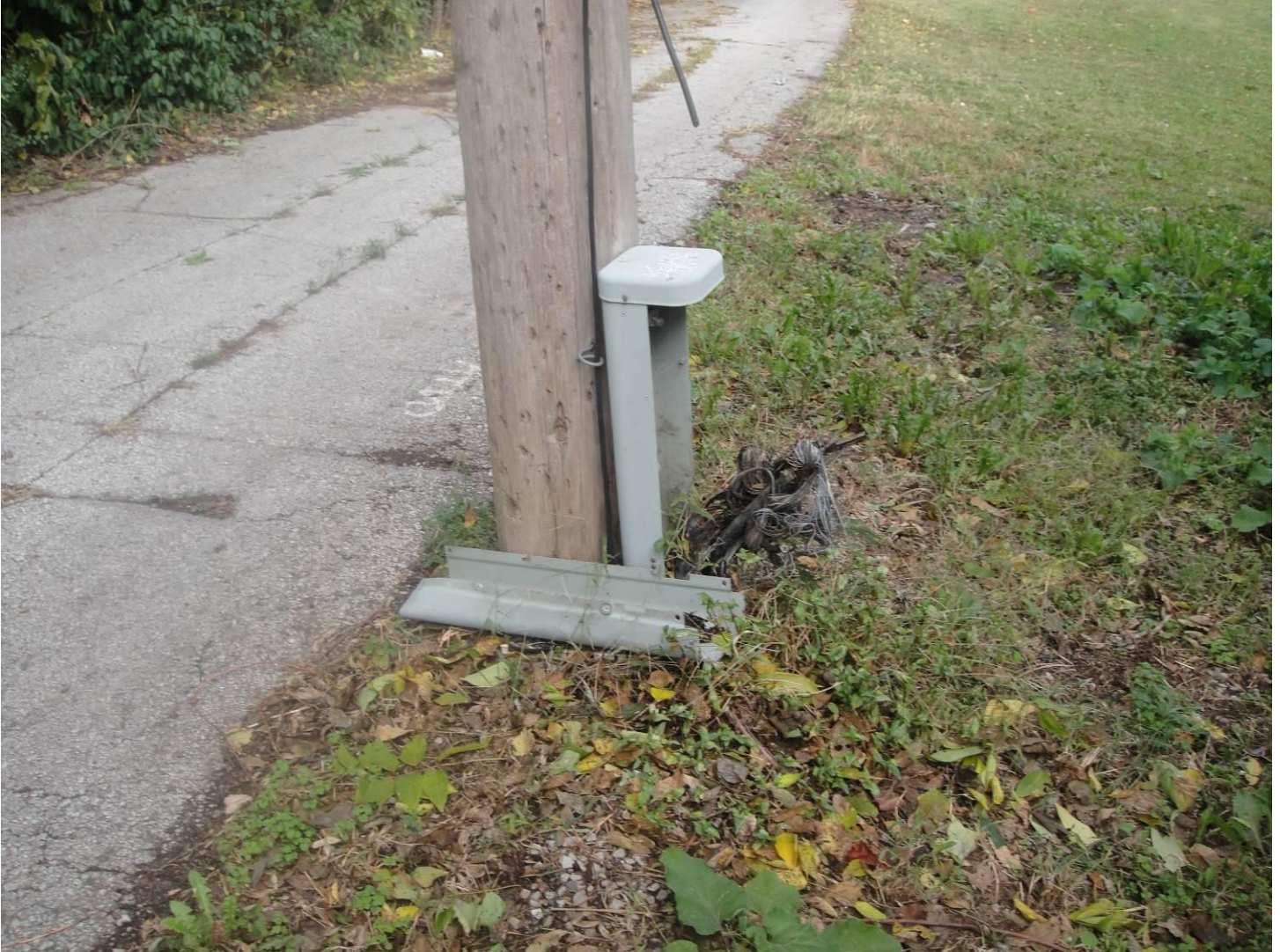
Photo 23 – Damaged utility along alleyway.
