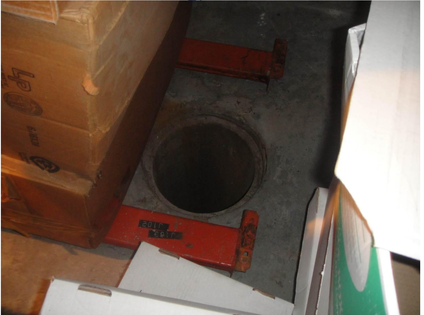
Photo 7 – 2534 Campbell, basement monitoring well location. Monitoring well is currently out of service.
