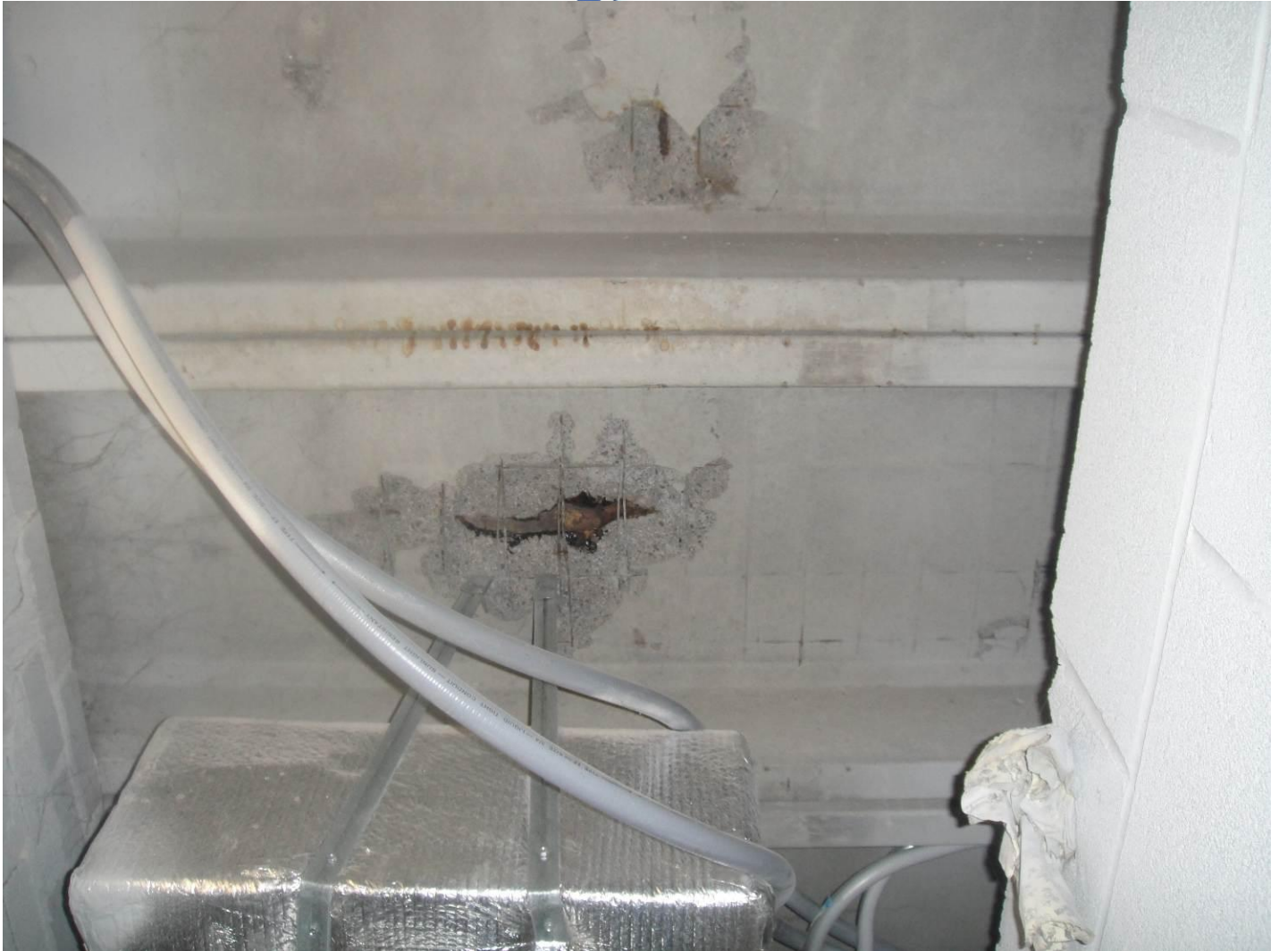
Photo 8 – 2534 Campbell, ceiling deterioration.
