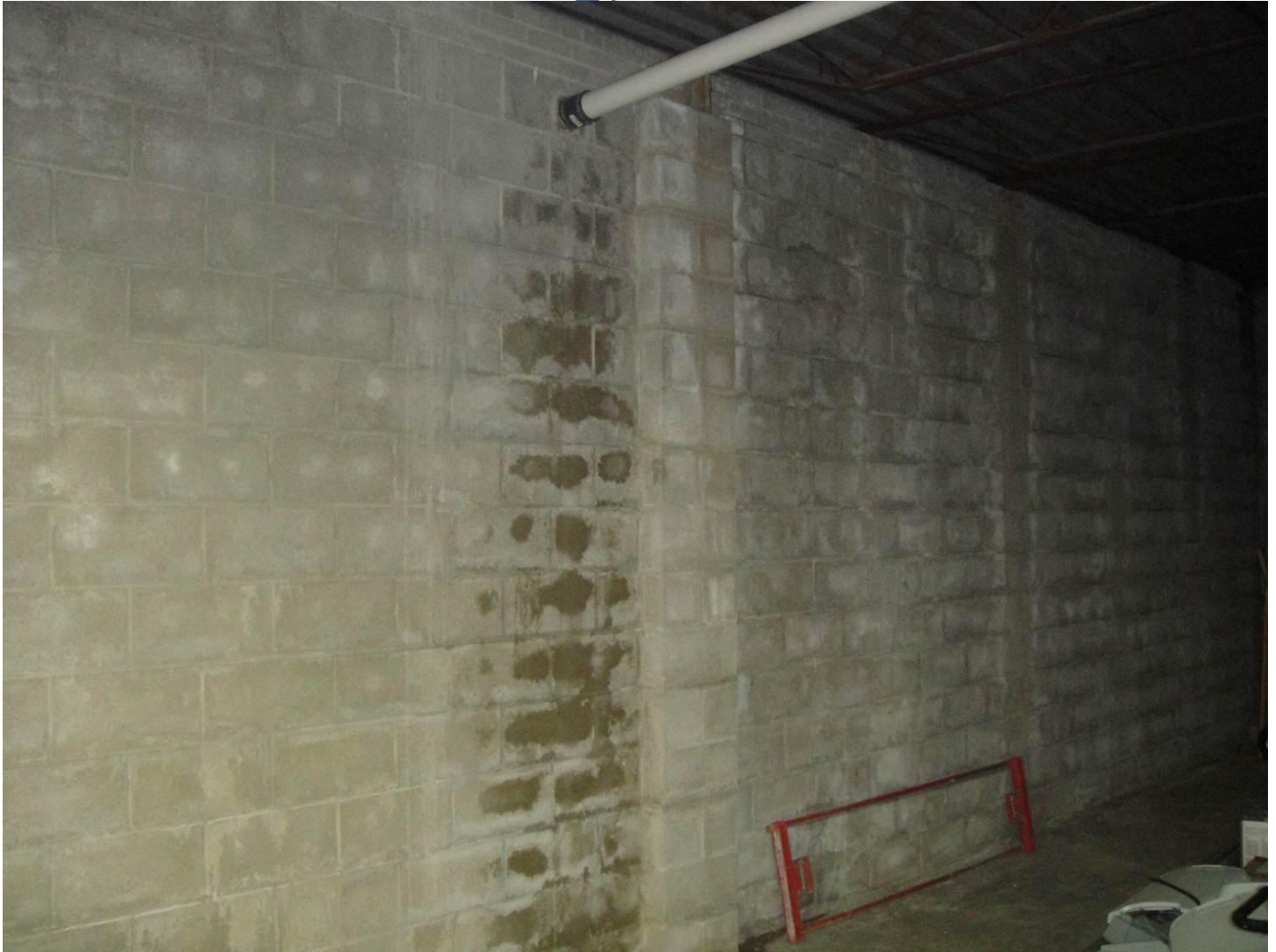
Photo 9 – 2534 Campbell, water damage.
