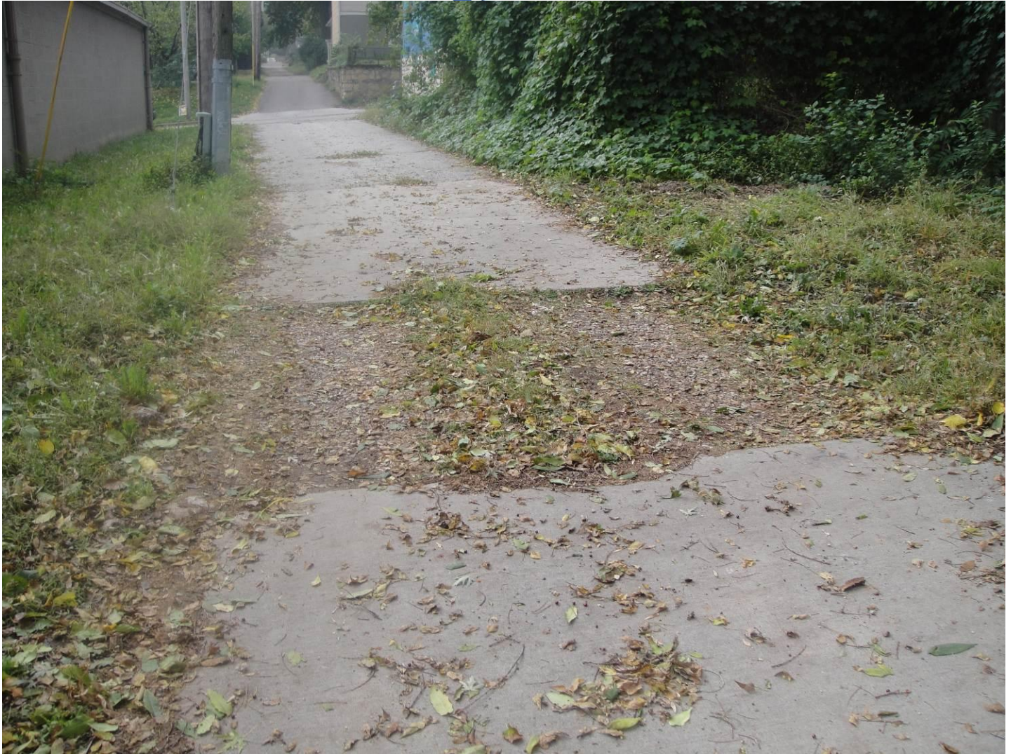
Photo 24 – Deteriorated alleyway. Photo looking south.
