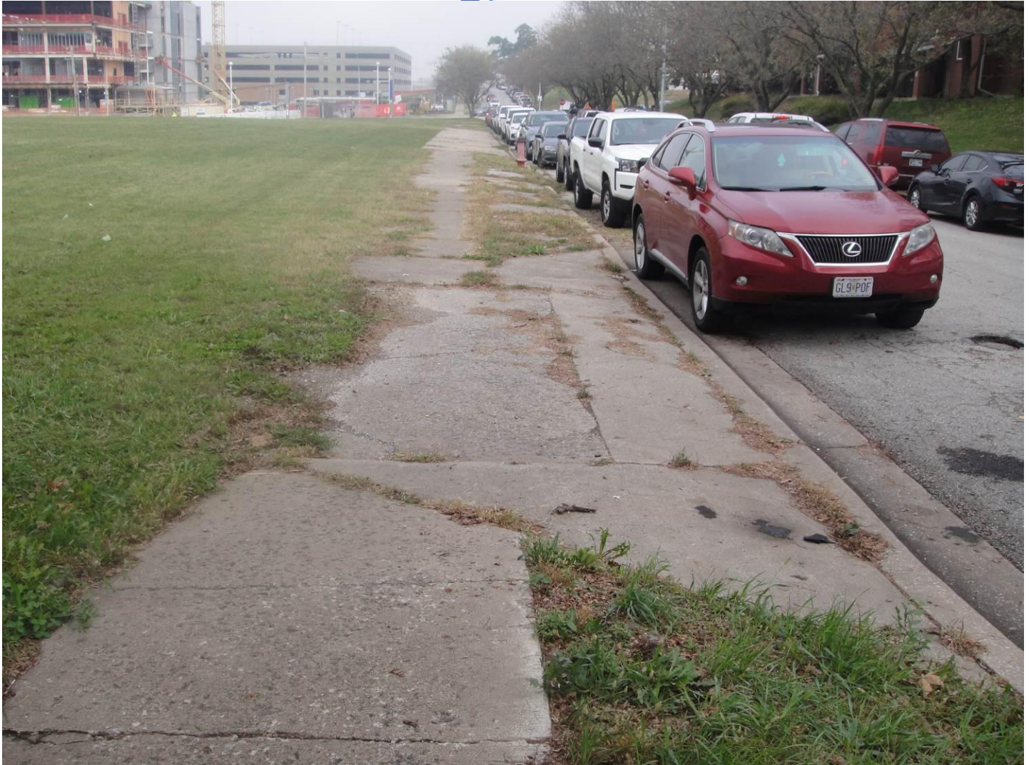
Photo 11 – Severely deteriorated sidewalk and curb-cut. Photo looking north along Campbell Street.
