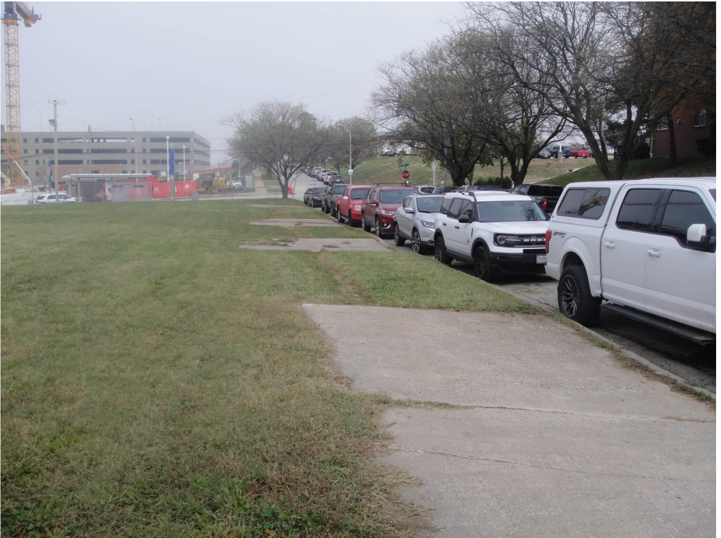
Photo 13 – Photo looking north along Campbell Street. Note deteriorated state of sidewalk.
