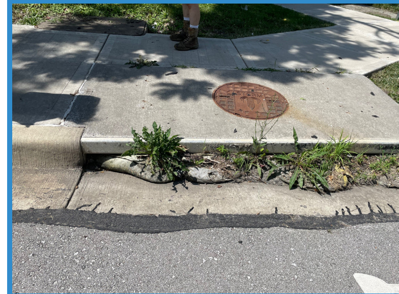
Figure 30. Blocked stormwater inlet - impacting drainage in the area
