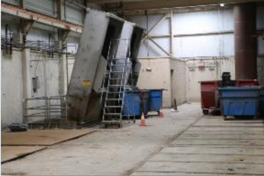
Trash Removal System at the Birmingham Pump Station
