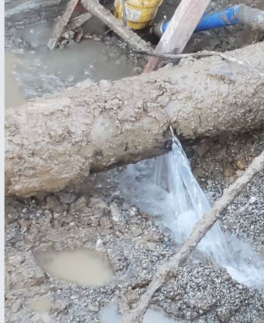
Broken water main leaking
